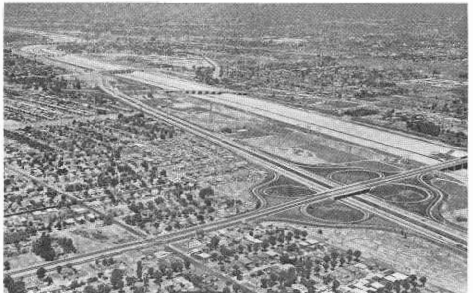
The completed cloverleaf interchange with Artesia Avenue is shown center right in this view looking northeasterly, while in the left background may be seen construction in progress north of Atlantic Avenue.
