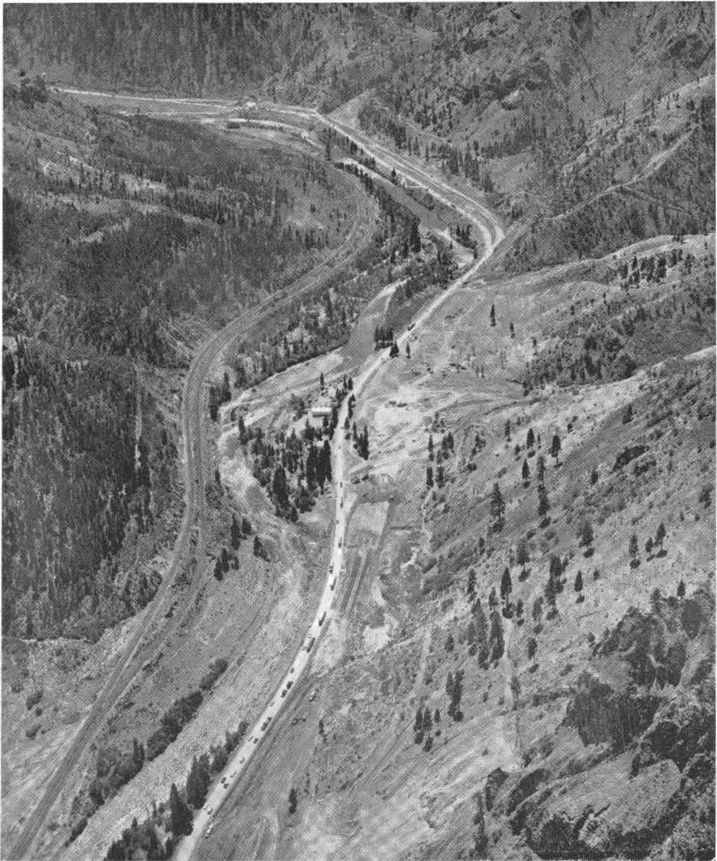
Traffic is shown passing through the construction area in this photograph of US Highway 40 work between Truckee and the Nevada state line
