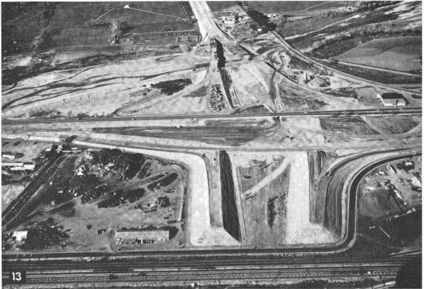
PHOTO No. 13—Construction now underway by Charles McCloskey and Crowell and Larson includes the junction of the Riverside Freeway and the San Bernardino Freeway. Embankments being built in the foreground of the photo will be the northerly terminus of the Riverside Freeway. The San Bernardino Freeway enters the interchange area on the left side of the photo, and turns northward to enter the City of San Bernardino in the background. Bridge construction in the center of the photo spans the Santa Ana River. This $3,300,000 contract is expected to be completed in February, 1958. The present US 99 crosses from west to east in the middle of the photo.
