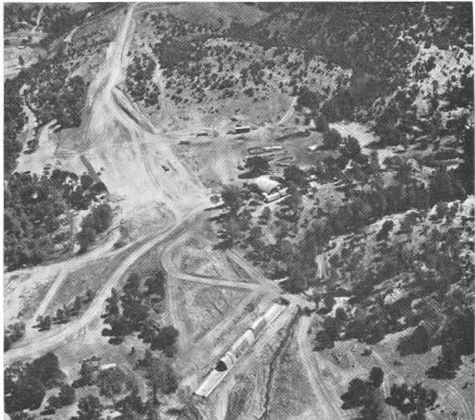
Near future intersection of the new highway and the Pentz-Cherokee Road. Contractor's main camp is shown in center of the photo and a 15-foot concrete arch culvert in the foreground.
