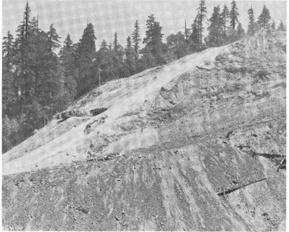
An earthmover being towed up the face of the cut. Lower earthmover is a loaded machine on the "down road."
