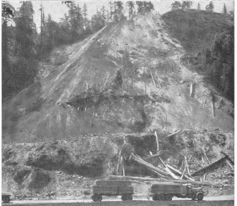
UPPER—One of four 400-horsepower "donkey" engines used to hoist the earthmovers up the steep up-ramp. LOWER—The earthmovers were automatically engaged to the heavy towing cable by the ingenious hook mounted on a metal sled which engaged a cable loop affixed to the tractor frame.
