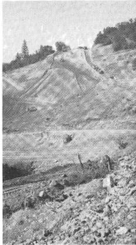
Cut and fill operation in the vicinity of Yankee Hill Road. The top of the fill will be near the roadway just above the earth-moving equipment to the right of the scene.
