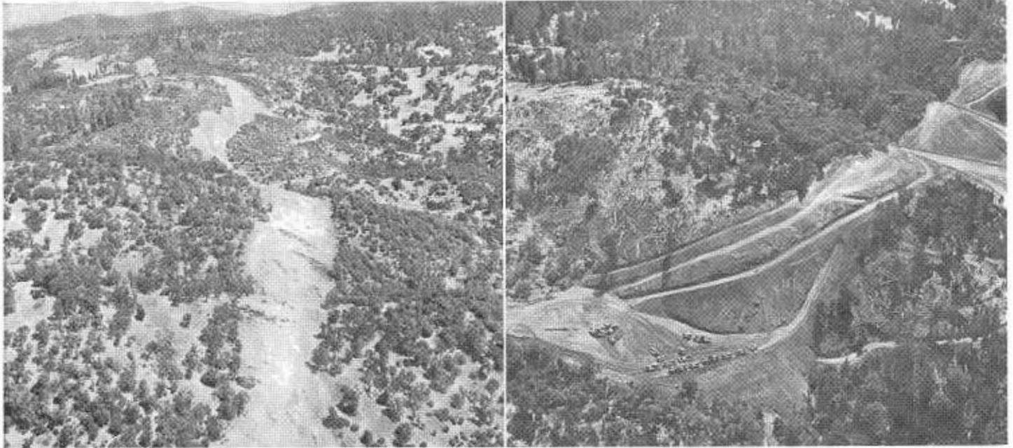
LEFT—Looking east along cleared area east of the West Branch of the Feather River showing the type of terrain through which the new roadway will pass in this area. RIGHT—Cut and fill operation in the vicinity of the Yankee Hill Road showing the rough terrain in this sector.
