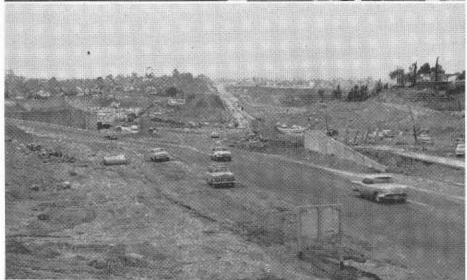
UPPER—View looking east on US 80 with Baltimore Driving Overcrossing in foreground and City of La Mesa beyond. CENTER—Looking east on US 80 showing Lake Murray Boulevard Overcrossing during construction.—LOWER—Looking west on US 80 showing construction of US 80—State Sign Route 67 interchange in the foreground.
