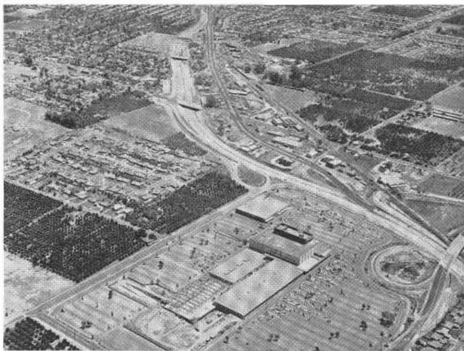
Looking southeast along construction of Santa Ana Freeway through City of Anaheim. In foreground, Broadway-Anaheim shopping center.
