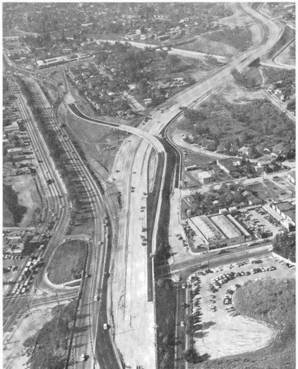
Looking northwest along Hollywood Freeway Extension. Lankershim Boulevard is in foreground. During construction traffic uses inbound lanes of Hollywood Freeway and Ventura Boulevard to left.
