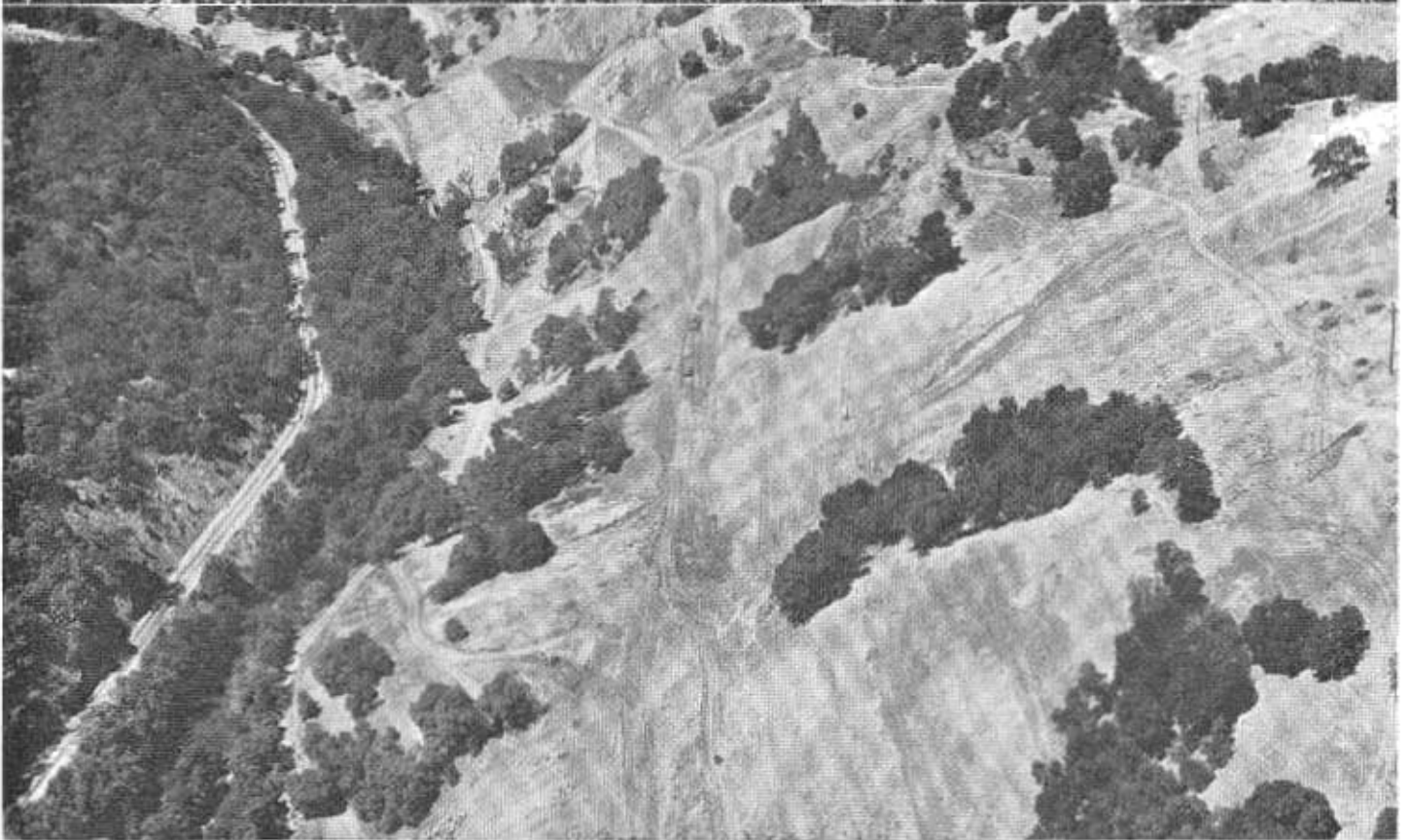
UPPER—In Lake County, Sign Route 53 is being constructed as a modern two-lane freeway. This aerial is looking southward toward Clearlake Highlands and Clear Lake (right background). LOWER—Heavy sidehill construction in the canyon of the East Branch of the Russian River in Mendocino County featured the relocation of Sign Route 20 between Calpella and Potter Valley Road.
