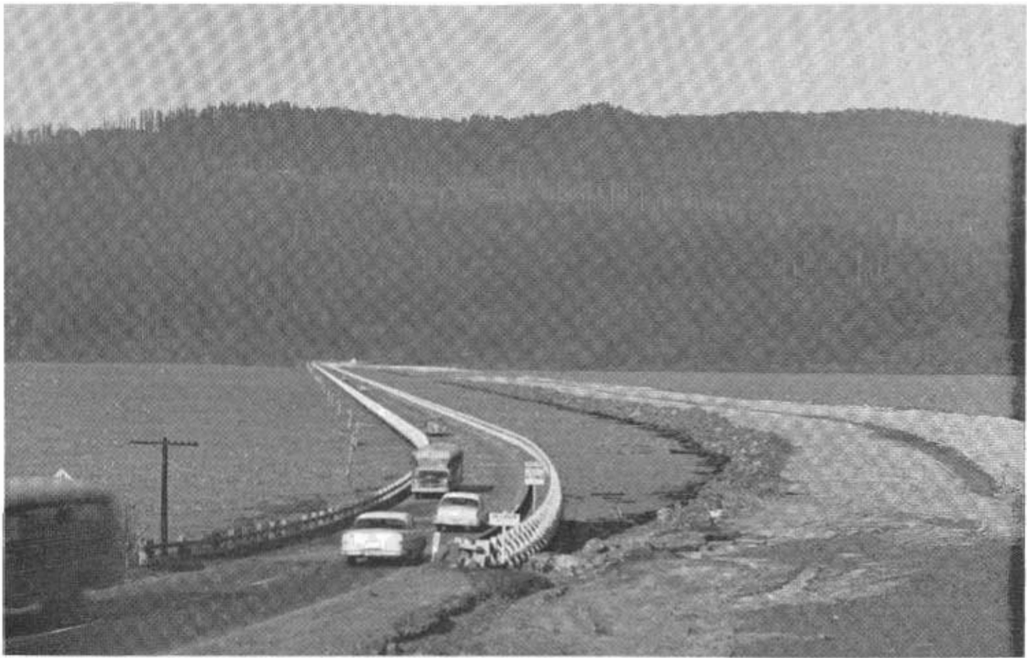
A four-lane fill between Patricks Point Park and the north shore of Big Lagoon will replace the 4,000-foot timber trestle (left)
