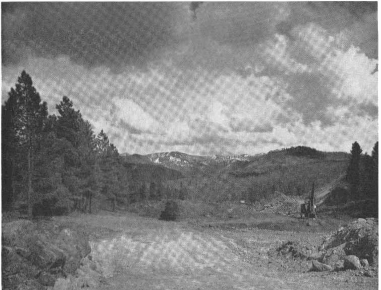
Freeway construction on US 40 near Floriston in Sierra County. The section from Floriston to the Nevada state line will be completed this summer.
