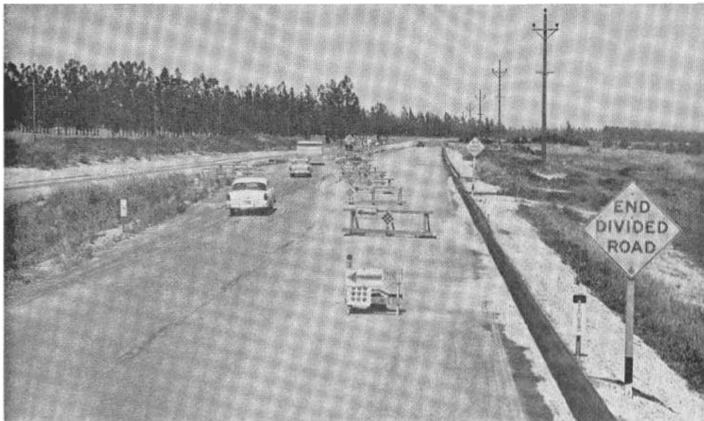
The detour at the beginning of the freeway project between King City and Greenfield during construction. Effective barricades such as this get traffic moving over the detour without delays. Some 9,000 vehicles a day use this section of US 101.
