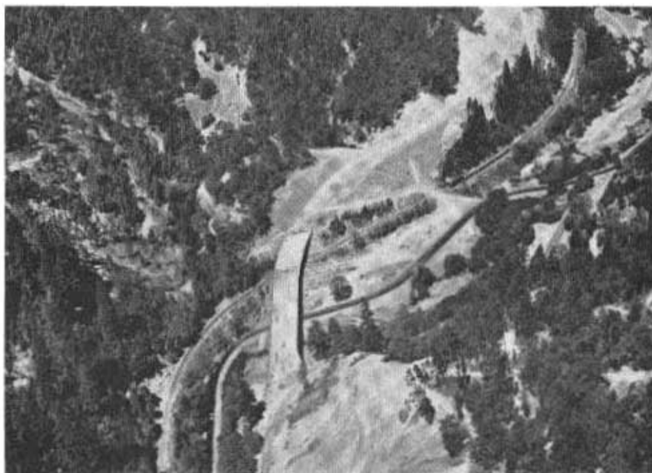
This four-lane structure over Outlet Creek and the Northwestern Pacific Railroad is part of the US 101 freeway construction north of Willits.
