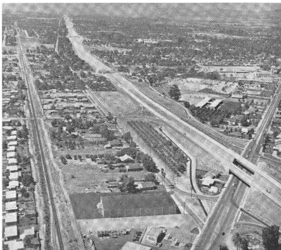
Looking northward toward Cajon Pass from the Highland Avenue (Sign Route 30) separation showing construction of the new US 66-91-395 freeway. LOWER—At present, the southern terminus of the Riverside Freeway is at Arlington Avenue in Riverside; however, construction is under way for another five and one-half miles south.
