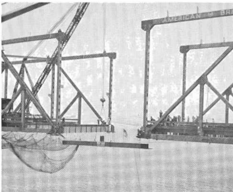
Starting the final closure between the two cantilever arms with the American Flag flying in the traditional custom of bridge builders throughout the Country. To make the final closure at this point six 500-ton jacks were used to jockey the suspended span into position so that bolting the final joints would be possible.
