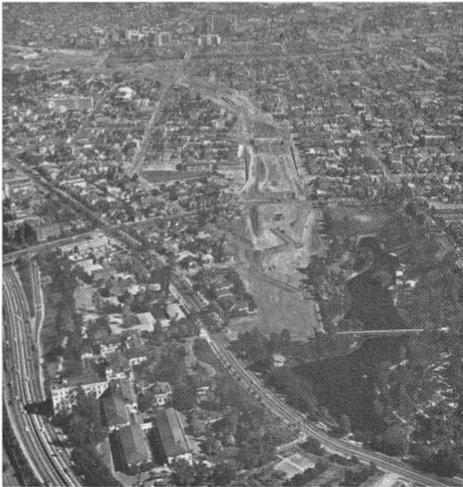
Construction on the Golden State Freeway is under way in the Boyle Heights area of East Los Angeles. Mollenbeck Park is in the right foreground; Los Angeles County General Hospital in the background.
