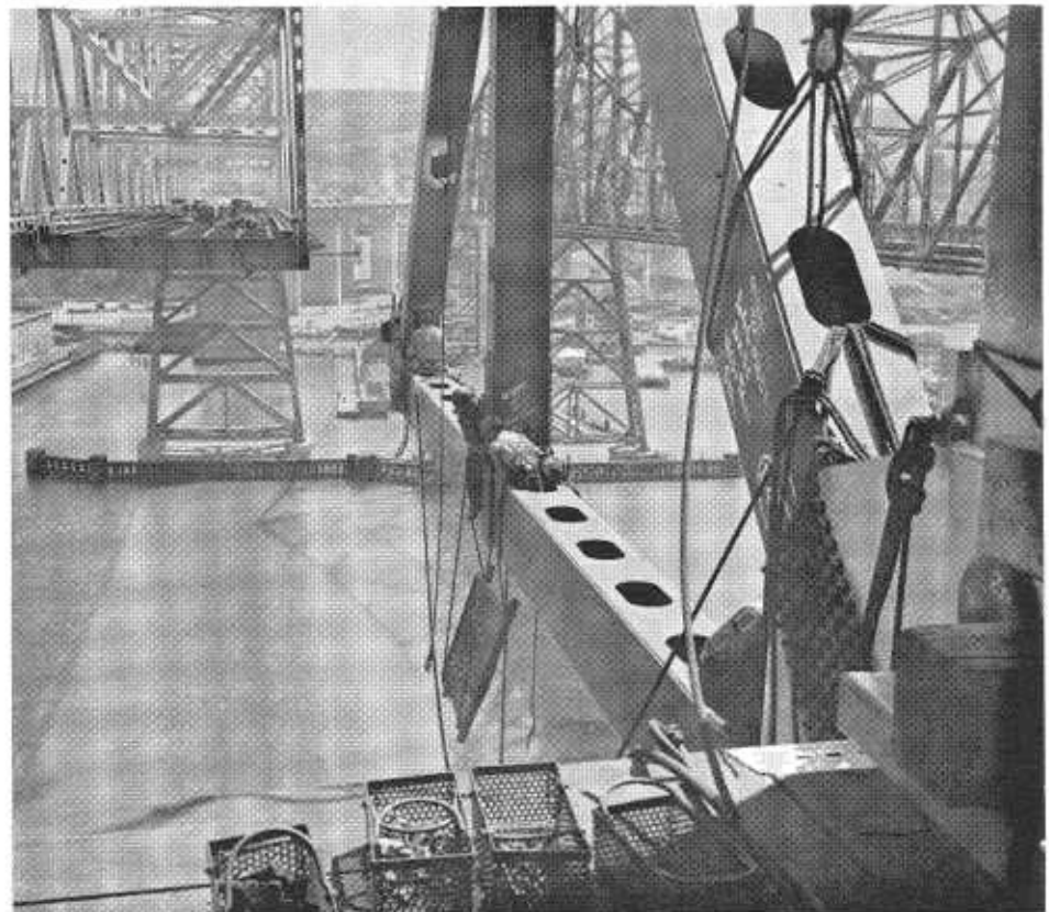
UPPER—For erection of the south anchor arm, steel was brought to the site by water from the Richmond assembly yard on barges. It was lifted into place by a 146-ton tower derrick mounted on two barges and assisted by stiff leg skid travelers. Most of the steel members were erected by cantilevering out; however, near each of the end towers eight panels of the suspended span were temporarily used as falsework, a portion of which can be seen in the lower left hand corner of the picture. LOWER—The bridge grows piece by piece to join with the other half of the cantilever span 145 feet above the waters below.
