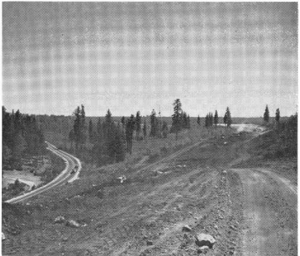
UPPER—Work progresses on the new Yuba River Bridge at the south city limits of Marysville on U. S. Highway 99E. LOWER—A view of freeway construction looking eastward from near the foot of Airport Hill in Placer County. Present US 40 (left) will serve as the westbound lane of the new freeway. The eastbound lane is under construction (right).
