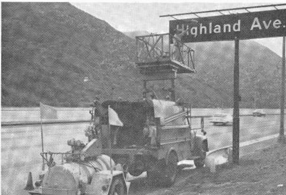
UPPER—On sections where an inside lane must be closed to wash signs, the work is done during a time when traffic is light, usually from daylight to 9 a.m. on Sunday. A flagman is always used to afford further protection to the men and equipment. LOWER—Signs such as this one on the Cahuenga Pass section of the Hollywood Freeway are cleaned from a tower lift on a truck parked on a paved shoulder.
