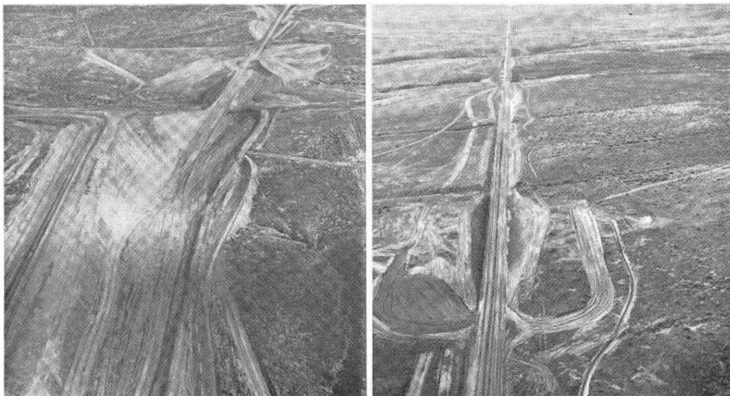
LEFT—The deepest cut (65 feet) and the highest fill (70 feet) are shown in the aerial with the detour on the left. RIGHT—This view southward from the middle of the job shows the relocated private road connections taking shape.
