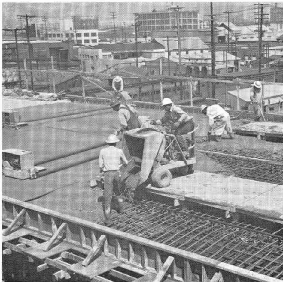
This crew is pouring concrete for the deck of the westbound distributor roadway over the Santa Fe Railway yard.
