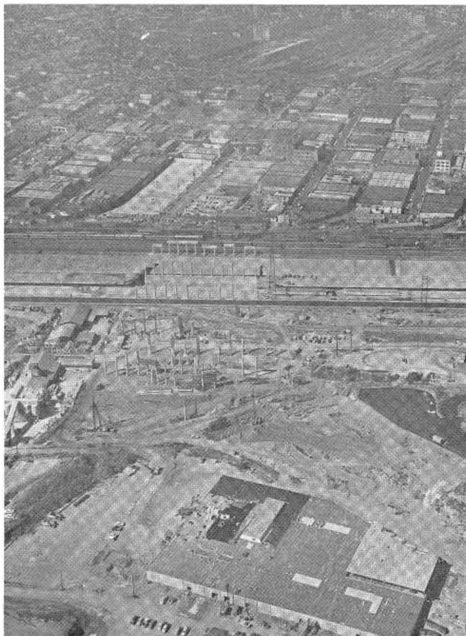
This view of the construction area was taken just after the erection of the reinforced concrete columns which will support the six parallel bridges over the river.
