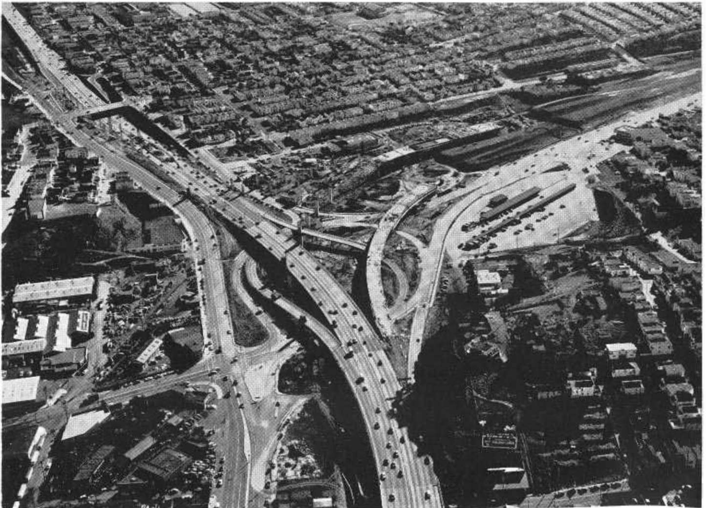
When completed this interchange on the James Lick Memorial Freeway (Bayshore) in San Francisco will connect with the first unit of the Southern Freeway under construction in the right middleground.
