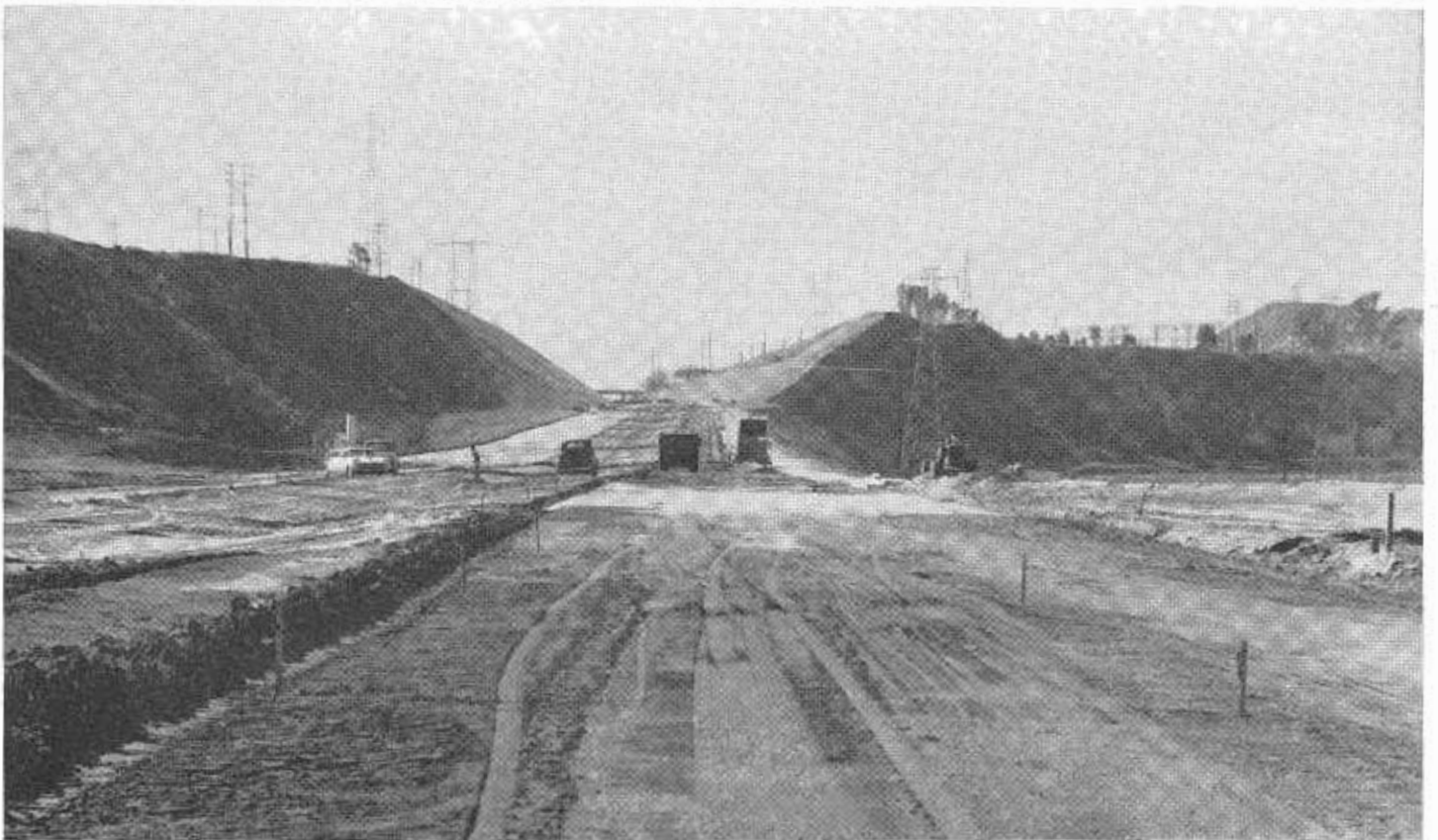
UPPER—Work is progressing on the south end of the "Missing Link" section of the Riverside Freeway near the City of Riverside. The interchange in the distance will connect US 91 and 395. LOWER—The Grand Terrace Cut on the "Missing Link" section of the Riverside Freeway.
