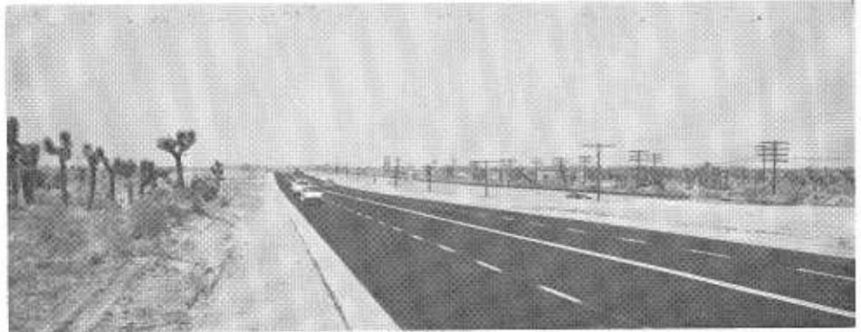
An eight-mile section of the US 6 in Los Angeles County was opened to traffic on April 15th. Reconstruction of this section of US 6, which is also known as the Sierra Highway, extends from Avenue R in Palmdale to Avenue I in Lancaster and involved four-laning the highway at a cost of $600,000. Work on the project was started last September.
