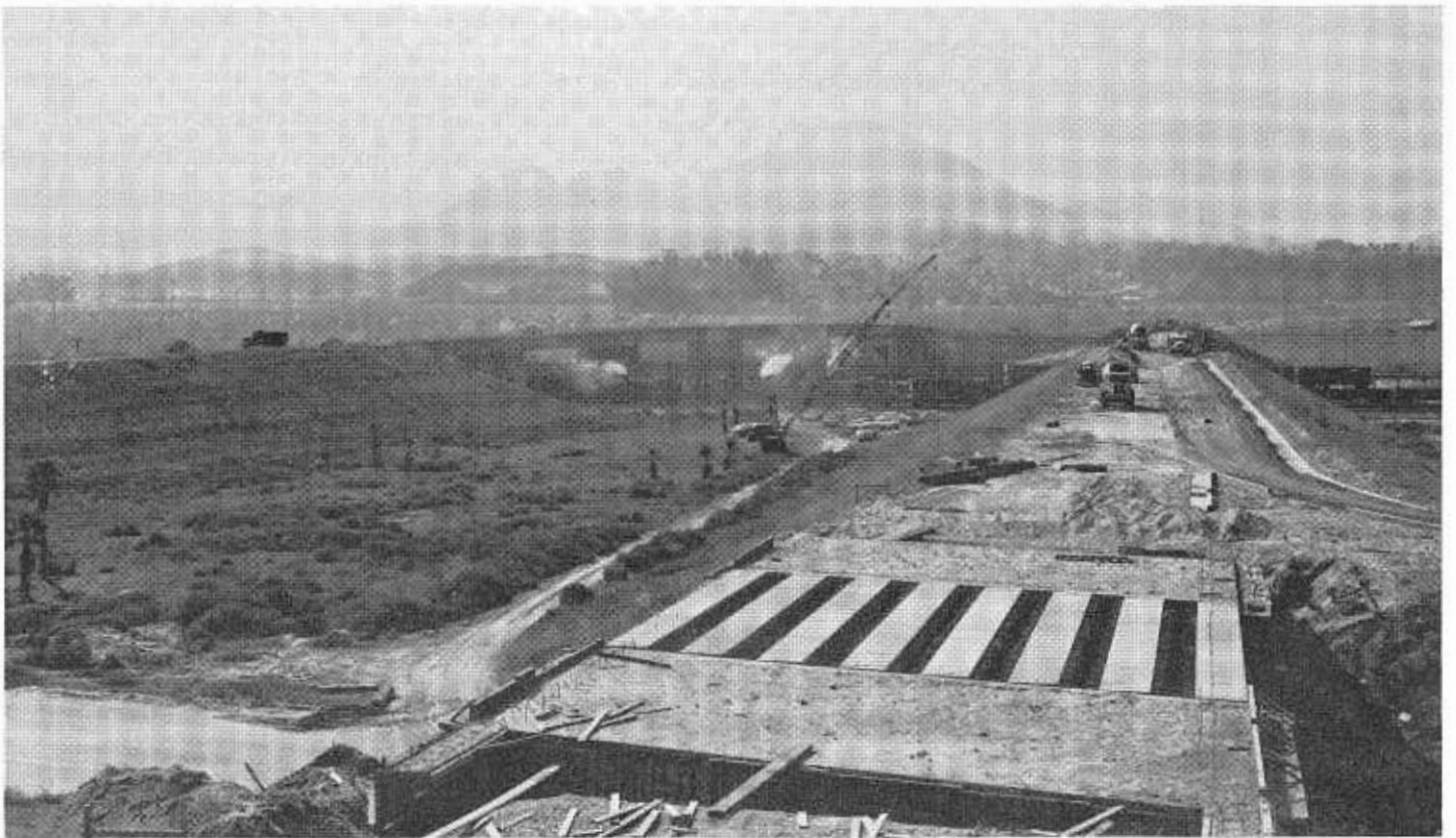
UPPER—This construction scene is on the Corona Freeway near Pine Avenue south of Chino. LOWER—A view of construction near the north end of the "Missing Link" section of the Riverside Freeway showing the Colton-Loma Linda Yard Overhead structures just south of the interchange with the San Bernardino Freeway.
