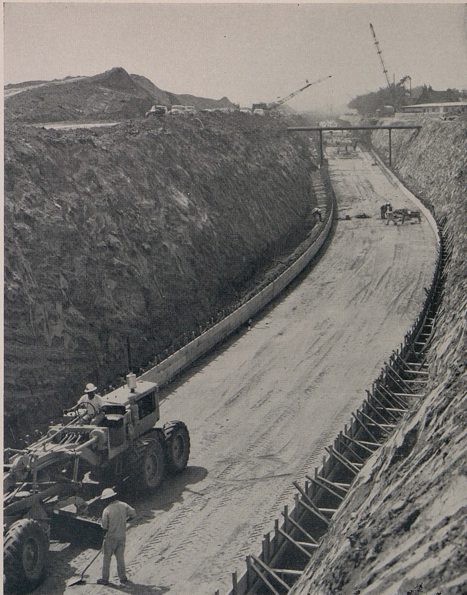
This photo shows the form work in place for the bottom slab of the Burbank-Western Storm Drain Channel.
