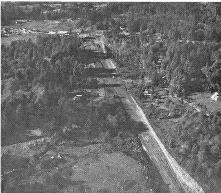
A northward view of the project with the Trinidad Interchange under construction in the background.
