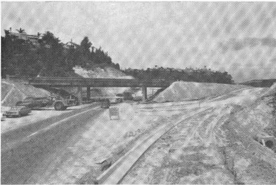
A view of the Aldine Drive Undercrossing now under construction on Fairmount Boulevard in San Diego.
