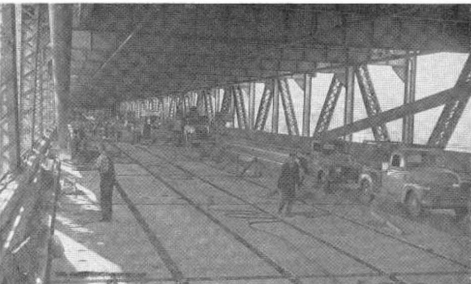
Deck slabs in place ready for pouring of concrete into the joints.
