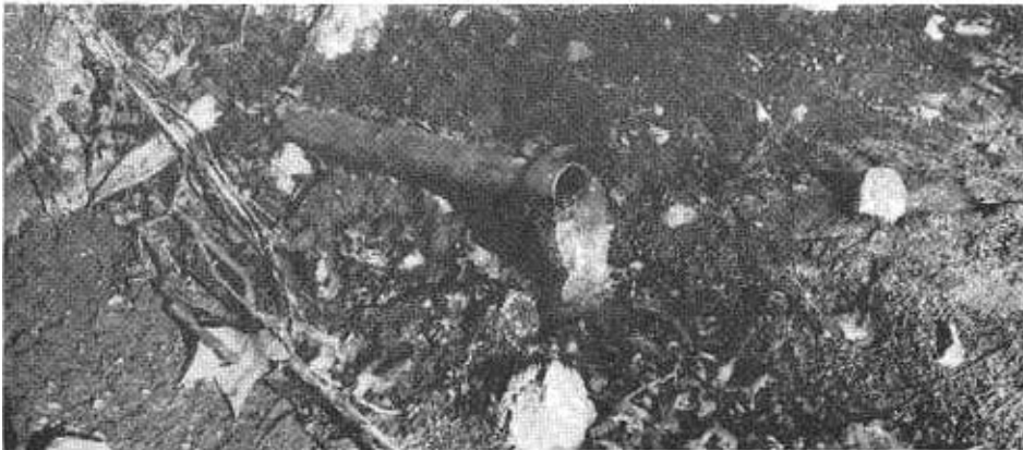
A typical horizontal drain installation. Notice the ice at the outlet. The photo was taken in January.
