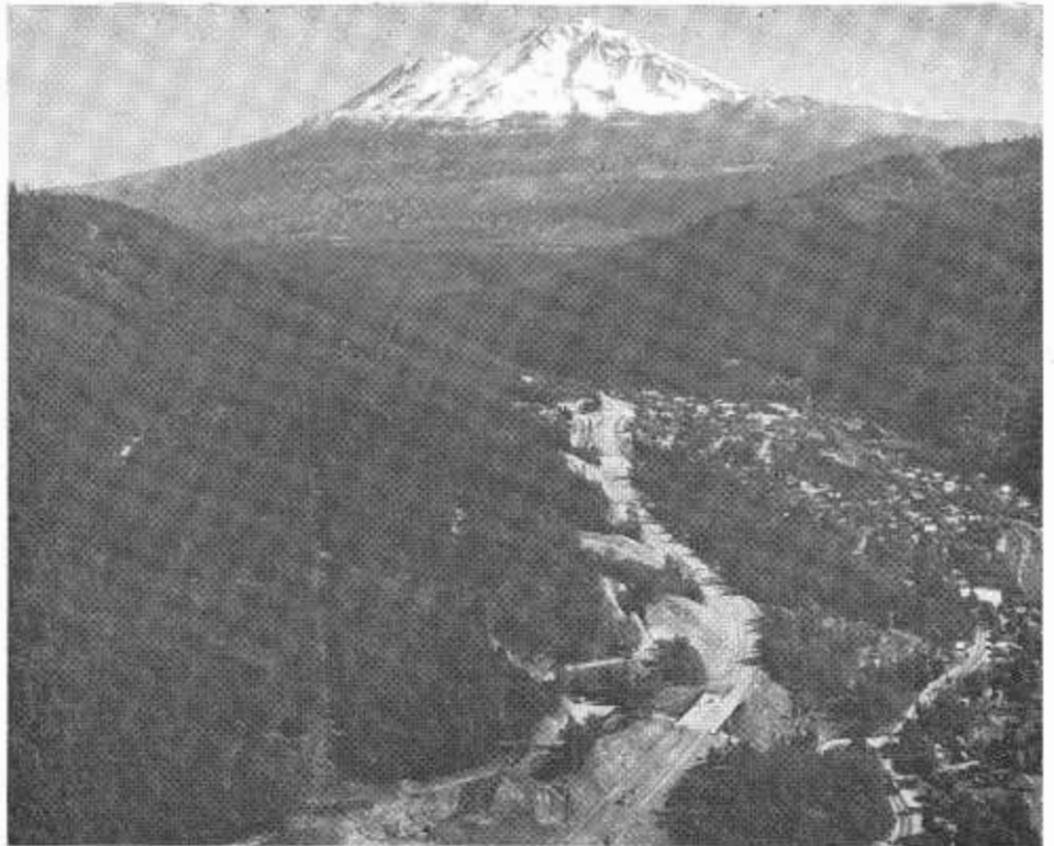
Slide removal operations on the Dunsmuir Freeway section of US 99. The Panorama Undercrossing is in the foreground. Mount Shasta in background.
