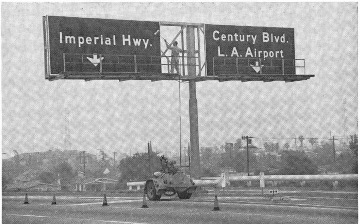
Cleaning a sign on the Harbor Freeway in Los Angeles. This late model sign has a catwalk for the use of maintenance personnel.
