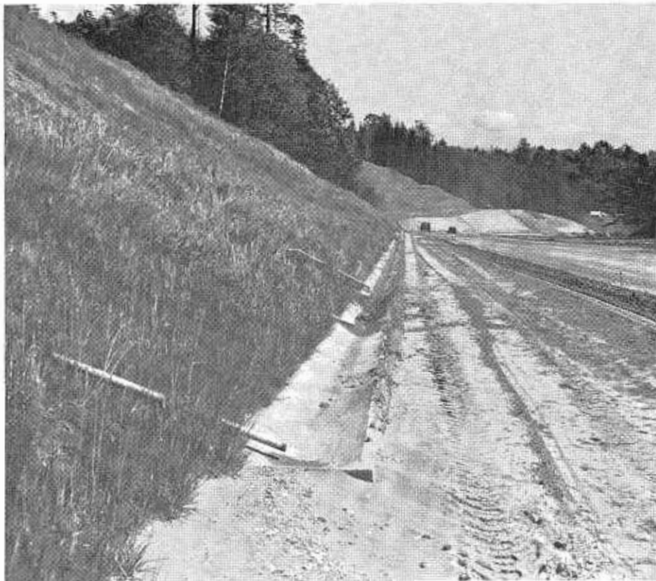
The big slide mentioned in the accompanying article was drained with horizontal drains, two outlets of which are shown in the above photo. The paved gutter prevents erosion of the cut slopes by water from the drains. The slopes were seeded and the heavy growth of grass protects the cut slopes from erosion.
