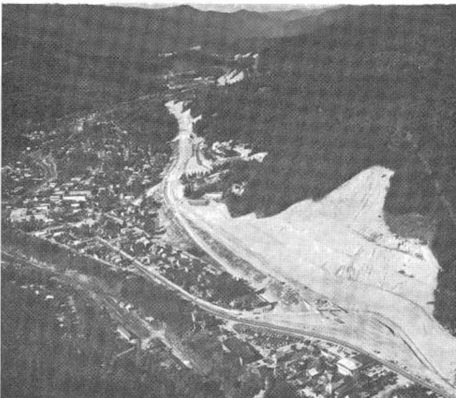
An aerial of the "Big Cut" at the north end of Dunsmuir. The slide area still to be removed can be seen in the right foreground.
