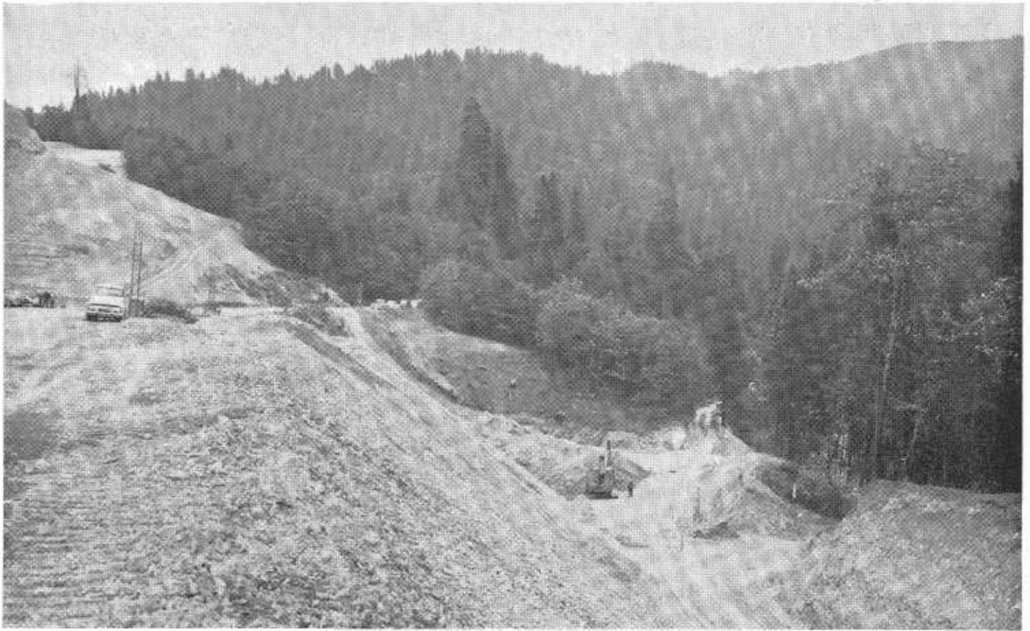
A typical stabilization trench used in construction of the freeway. The outlet trench is in the center foreground.
