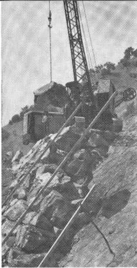
Construction in the early 1940's on the access road to General Grant National Park.
