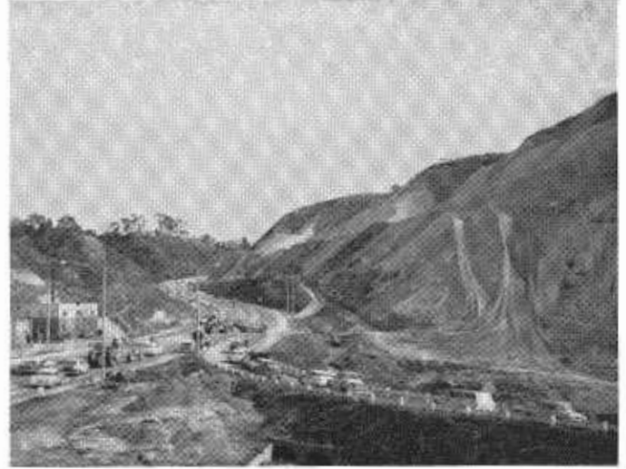
A view of the construction area looking south along US 395 showing more equipment being taken across the roadway under traffic control.
