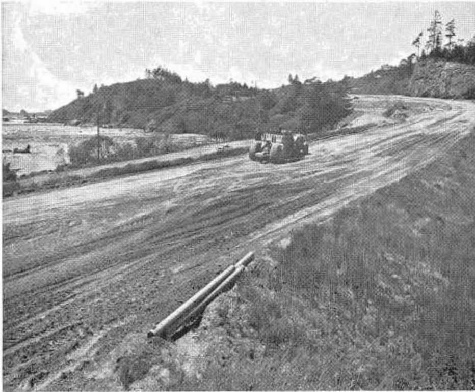
A photo of the freeway under construction with Little River Beach to the left. Note the heavy growth of grass on the planted slopes resulting from winter rains in Humboldt County.
