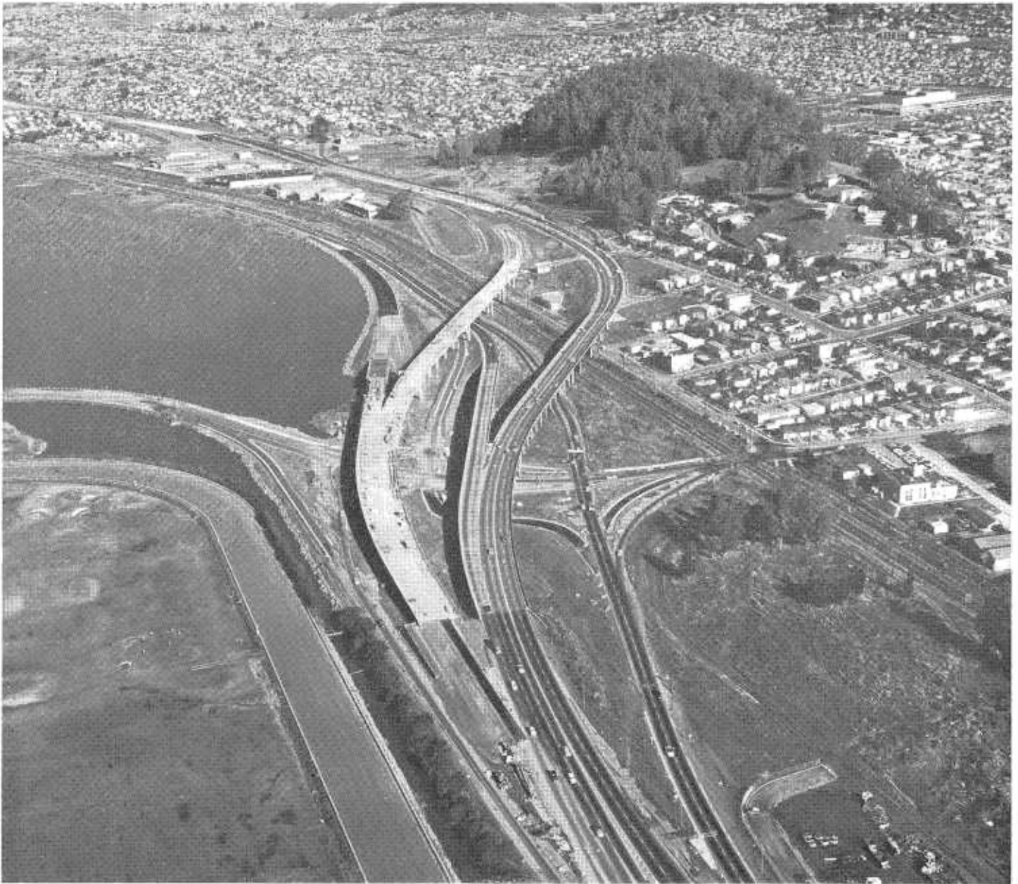
Looking northward at construction of the El Cerrito overhead showing tree-covered Albany Hill and (lower left) a portion of the racetrack at Golden Gate Fields.
