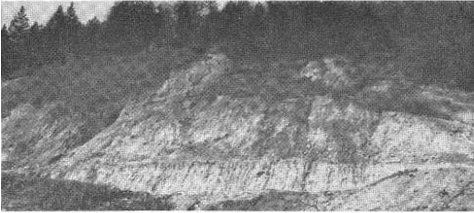
This is a photo of typical slide conditions encountered in the Sacramento River Canyon.
