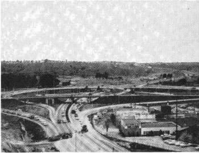
This photo taken during the reconstruction of the US 80-395 Interchange shows equipment crossing US 80 under traffic control.
