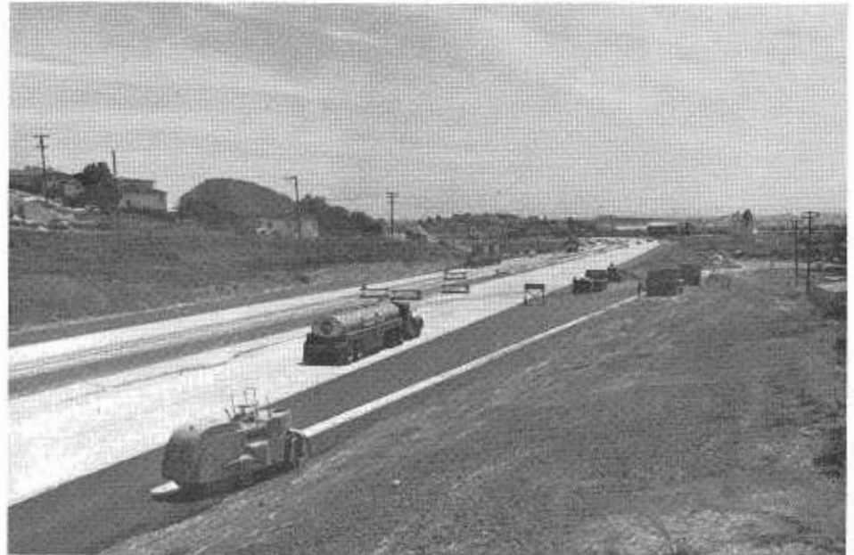
This photo taken during the final phases of construction shows the offramp at Carlson Boulevard for southbound traffic.
