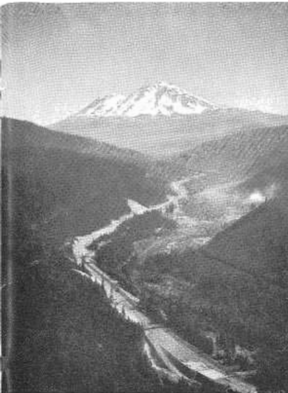
FRONT COVER—Freeway construction on US 99 in the rugged Sacramento River Canyon looking north from Castle Crags State Park to towering Mt. Shasta in the background. The deep cut in the foreground is on Kettlebelly Ridge. The freeway passes to the left of the City of Dunsmuir which can be seen in the upper portion of the canyon. (See the article "Dunsmuir Freeway" in this issue.) Photo by M. R. Nickerson
