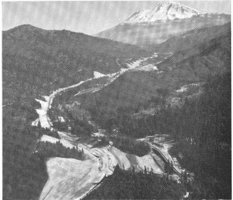
Slide removal operations on the Castilla section of the freeway, adjacent to the "Big Fill" area. View is northward.
