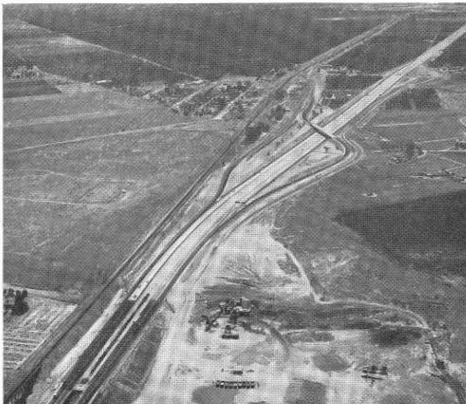
This view southward shows the Herndon Avenue Overcrossing, at the north end of the project. Old highway at left.
