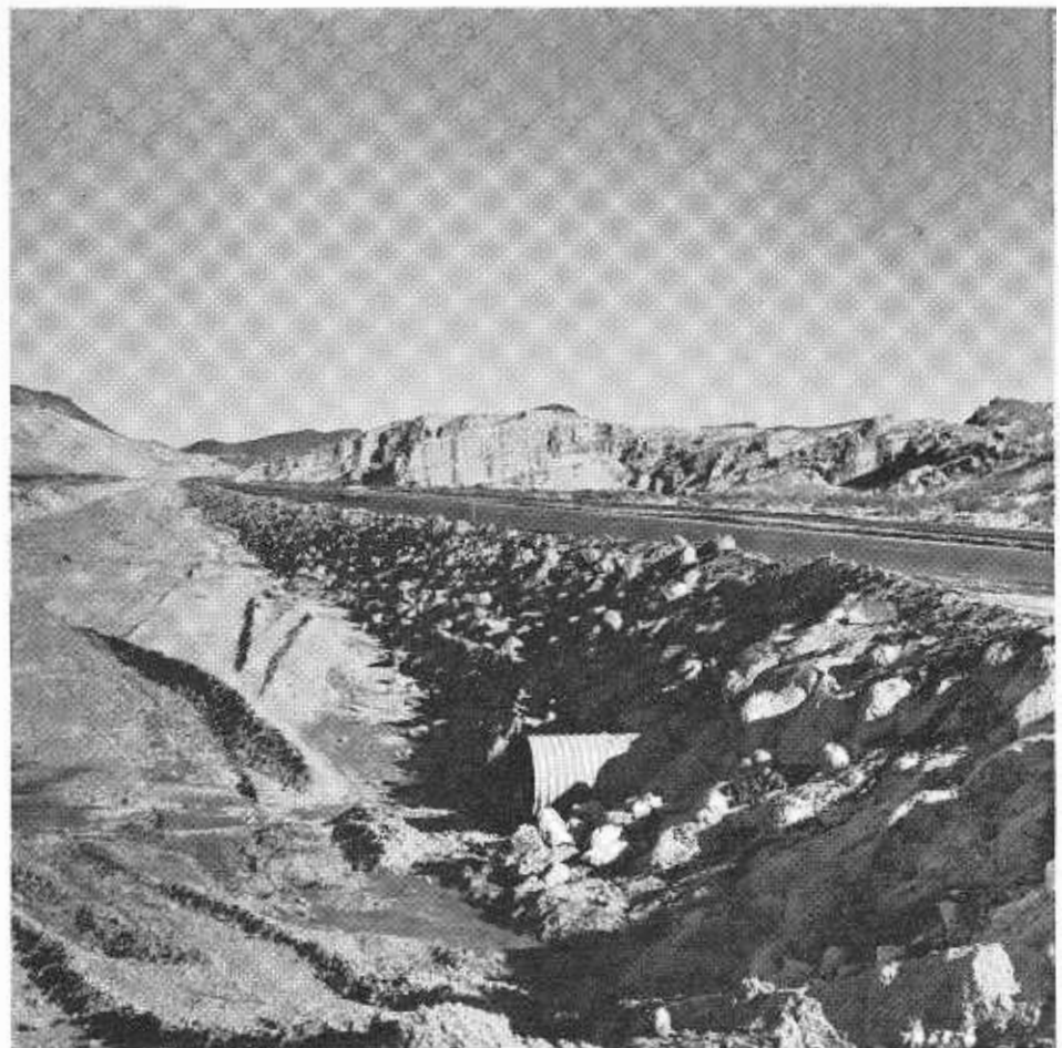
New realigned four-lane section climbing out of main wash of Red Rock Canyon. The grouted rock slope protection extends 12 feet below the interception channel.
