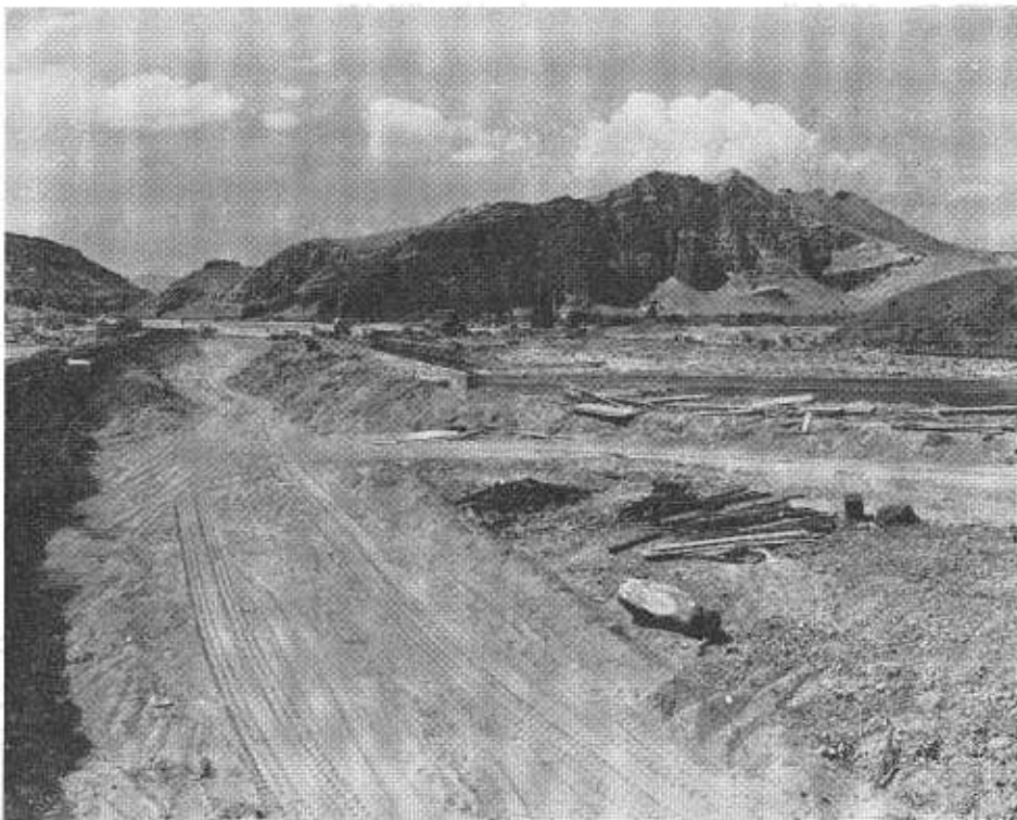
New bridge across main wash of Red Rock Canyon during construction. Note sand fill used instead of conventional falsework for deck slab.
