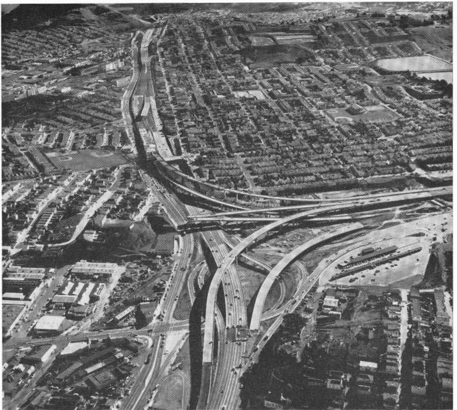
James Lick Memorial (Bayshore) Freeway in San Francisco at the site of construction for the Southern Freeway Interchange. Aleman Interchange in foreground, looking south.
