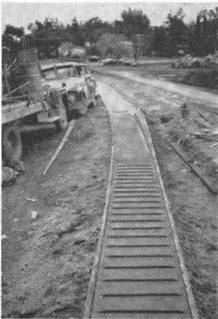
This photo shows a portion of the scored concrete shoulder strip which is described in more detail in the accompanying article.
