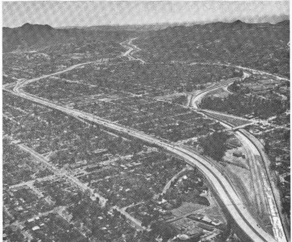
Construction on the Ventura Freeway near Laurel Canyon Boulevard. The Los Angeles River is to the right and Cahuenga Pass in the background. The view is southeast.
