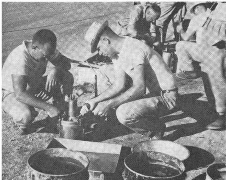
A crew carries on tests to determine the percentage of air in mixtures of concrete. Note the series of wash buckets in the foreground.
