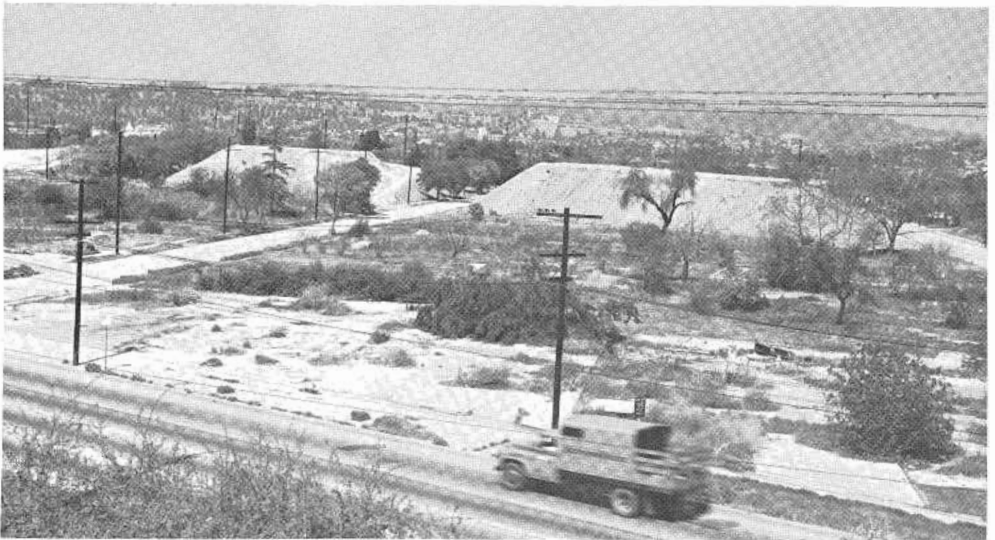
Disposal sites on the Golden State Freeway in the vicinity of Riverside Drive and Alessandro Street, viewing northerly across Riverside Drive, with City of Glendale in the background.
