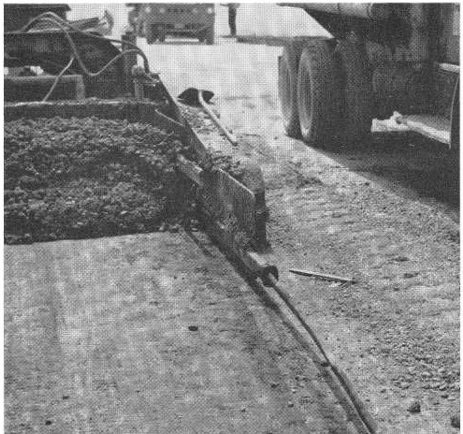
Closeup showing method used to insert keyway section in front of slip form paver. This is done only on initial lanes.
