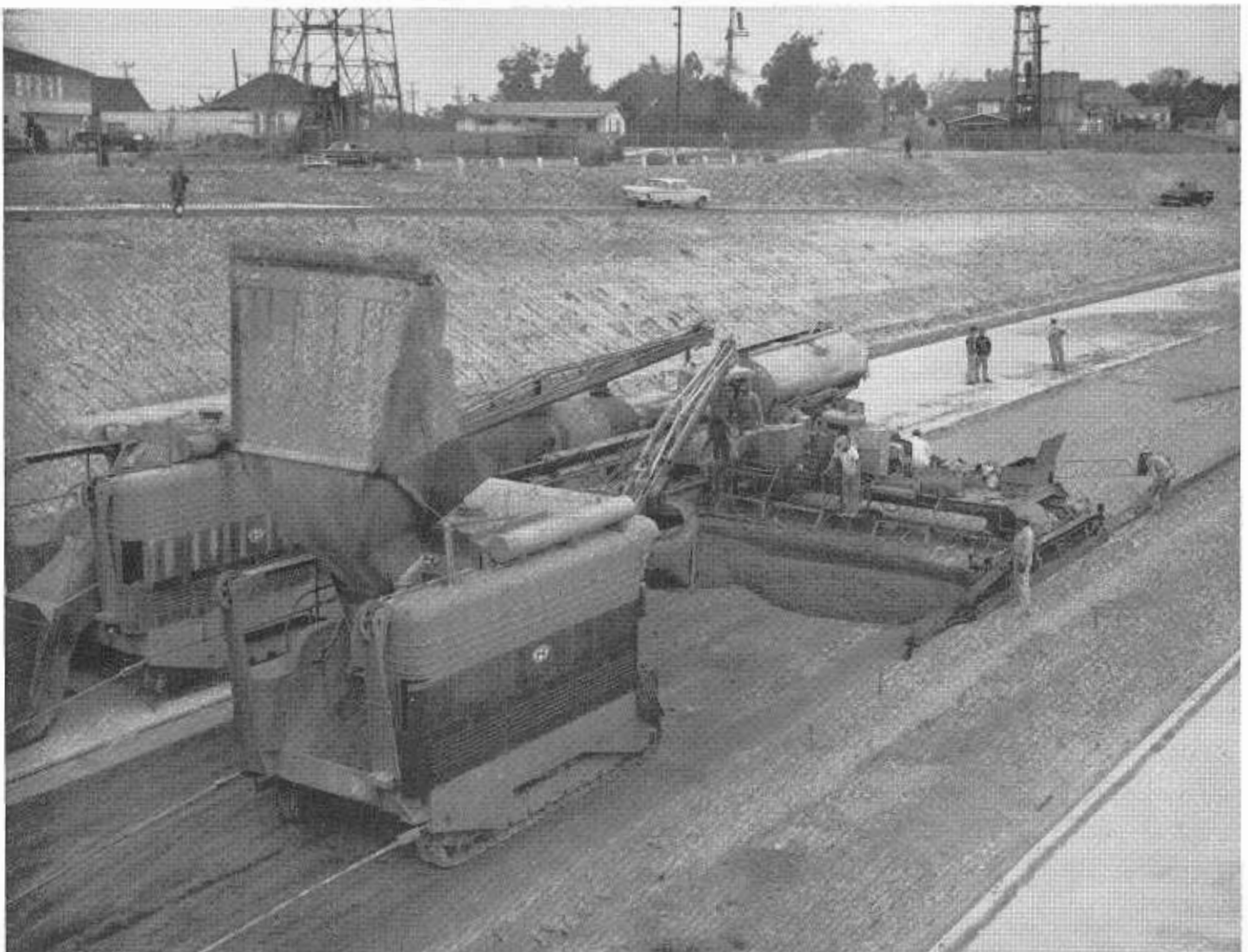
Slip form paver being fed by two dual-drum concrete paving mixers. Man standing on platform in front of machine is placing center tiebars.
