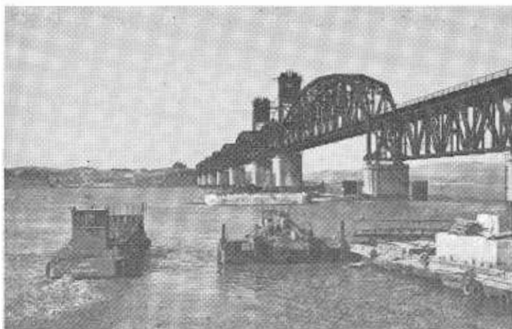
The box footing for Pier 12 has been floated into place and anchored in position. The next operation will be to rig up for drilling the 78-inch holes for the steel caissons.
