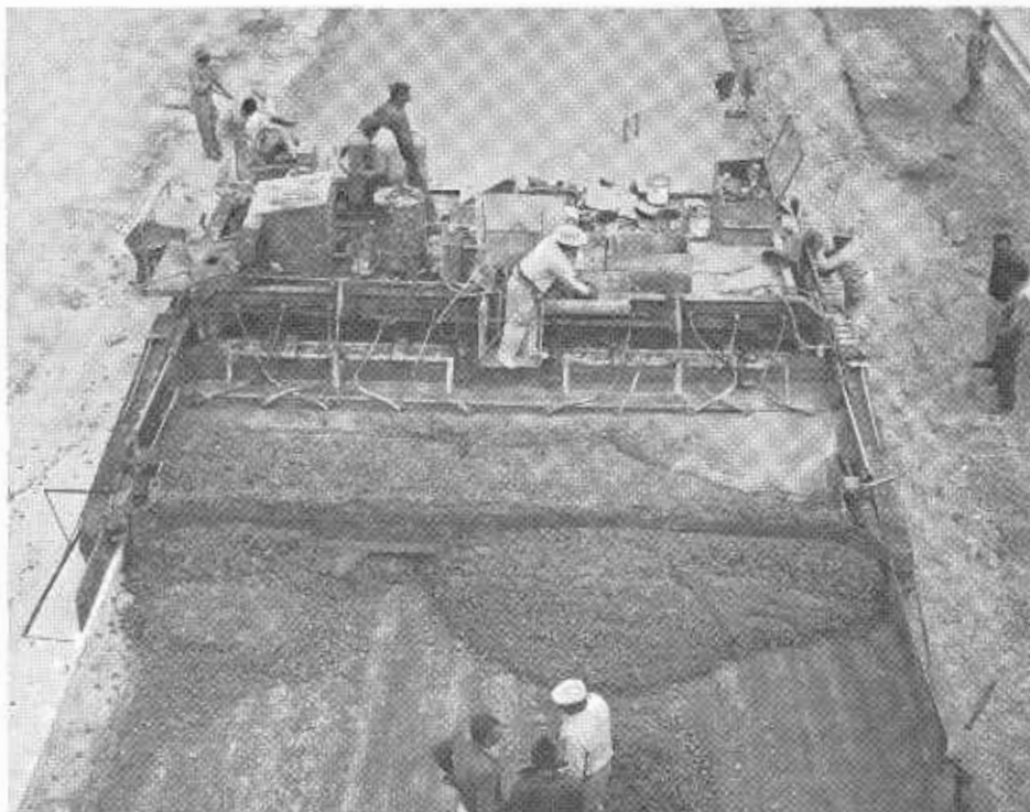
The screed is now at its forward limit of travel. The position of the 10 internal vibrators will be noted behind the screed.
