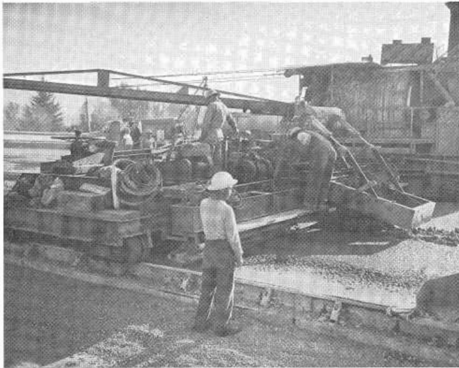
A crew spreads concrete and places center dowels on the East Contract.
