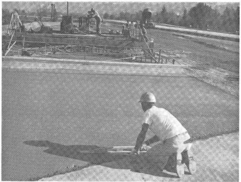
Concrete finishing operations must be made at the junction with the previous day's run.
