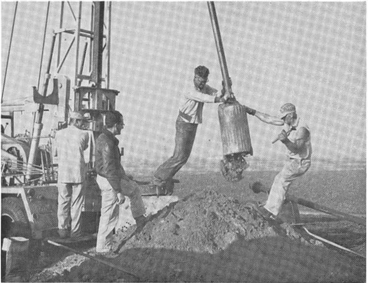
Drilling operation in Orange County to obtain soil samples for testing purposes.
