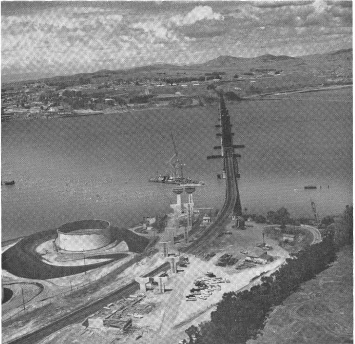
Construction is continuing on the new Carquinez Strait toll bridge between Benicia and Martinez. This photograph, taken in April, shows the nearly completed concrete approach piers on the Martinez side. The large floating derrick in the water is used to set steel caissons in place.
