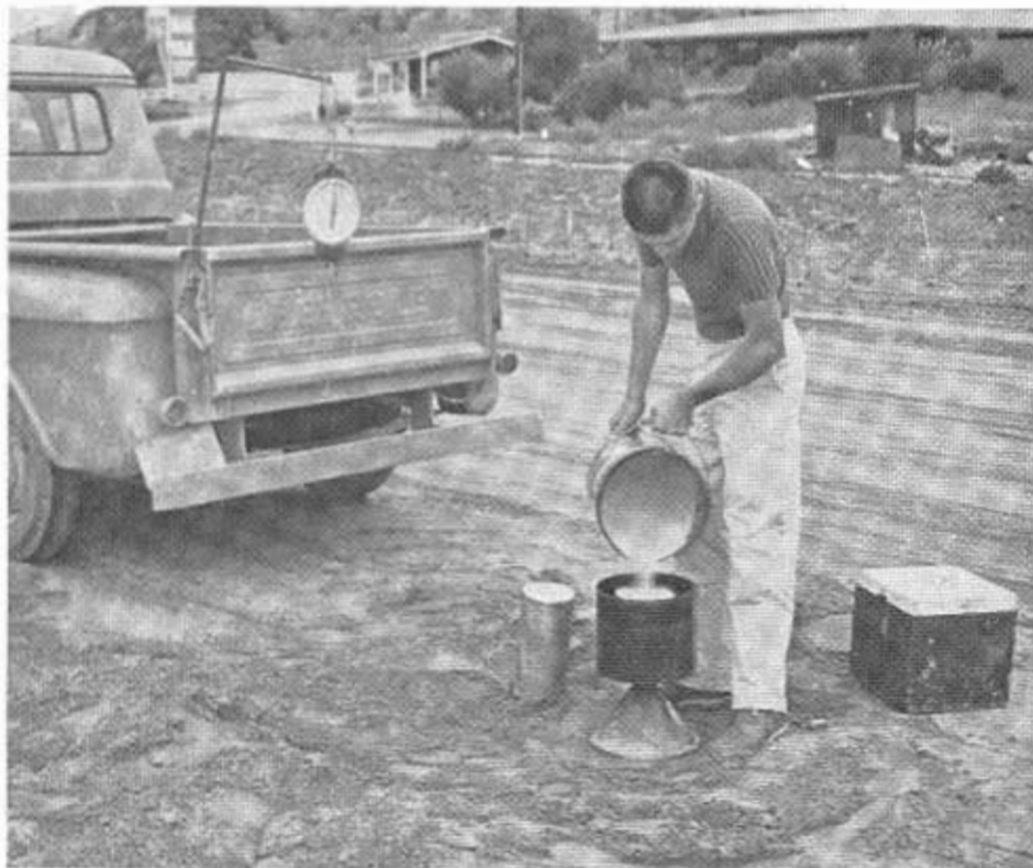
A sand volume test is used in checking compaction qualities on a highway construction project in Southern California.
