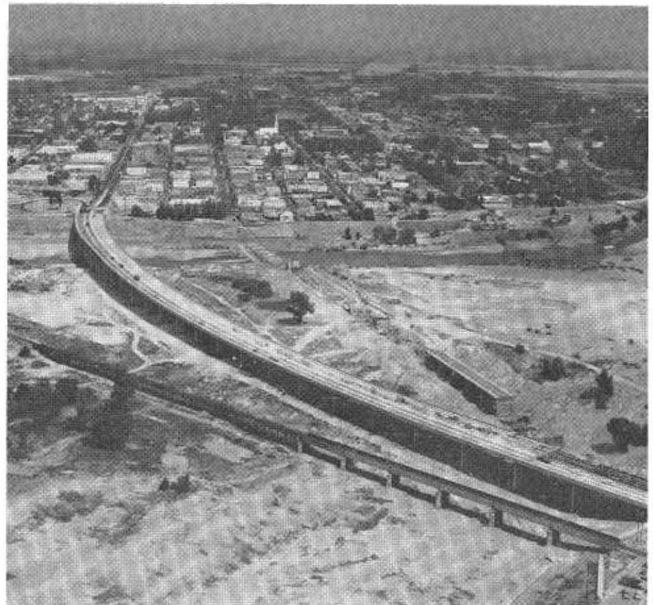
A new bridge over the Yuba River on US 99E at Marysville was completed earlier this year. This aerial photograph shows the structure while construction was still in progress. Note old bridge (right) being removed.
