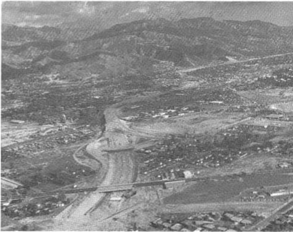
Work is now under way or budgeted on a spectacular series of large scale freeway projects on the Golden State Freeway portion of the future east-loop bypass around the central district of Los Angeles. One of these big jobs is this two-mile project in the San Fernando Valley between Roscoe Boulevard and Lankershim Boulevard (foreground) near Sun Valley.
