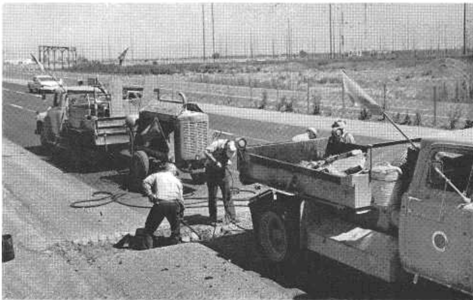
Division of Highways maintenance crew repairing the pavement base on a section of the Bayshore Freeway in San Mateo County.
