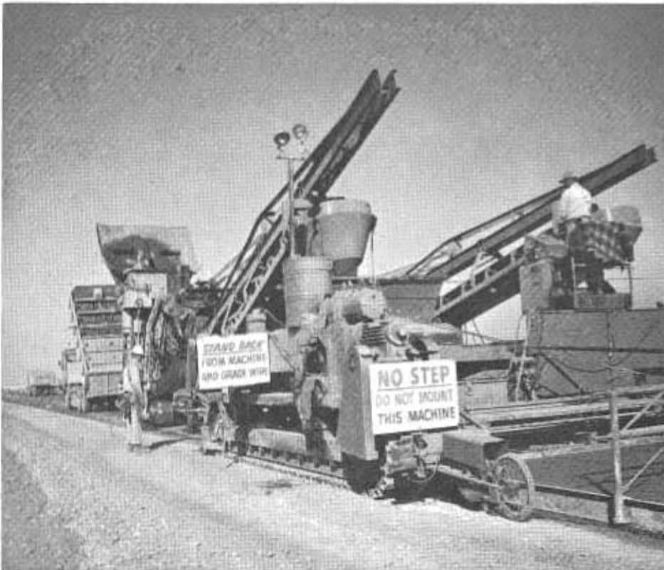
The slip-form method of paving (above), in which the usual form construction is not required, was used on several projects during the year. This new highway construction process is still in the developmental stage. About 40 miles of 24-foot pavement have been constructed by this method.
