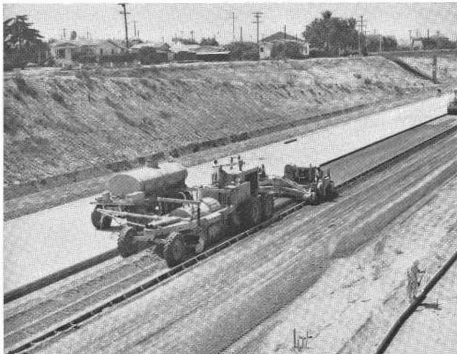
The road-mixed cement-treated base operation uses a pugmill-type mixer and operates between sideforms set for concrete pavement 12 feet wide. (Photo by Pettibone Wood Mfg. Co.)
