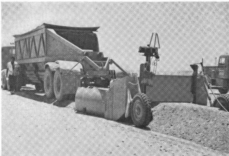
Sizing windrow of mineral aggregate for road-mixed cement-treated base operation. California requires that the quantity of material in windrows shall not vary more than 5 percent from that specified.
