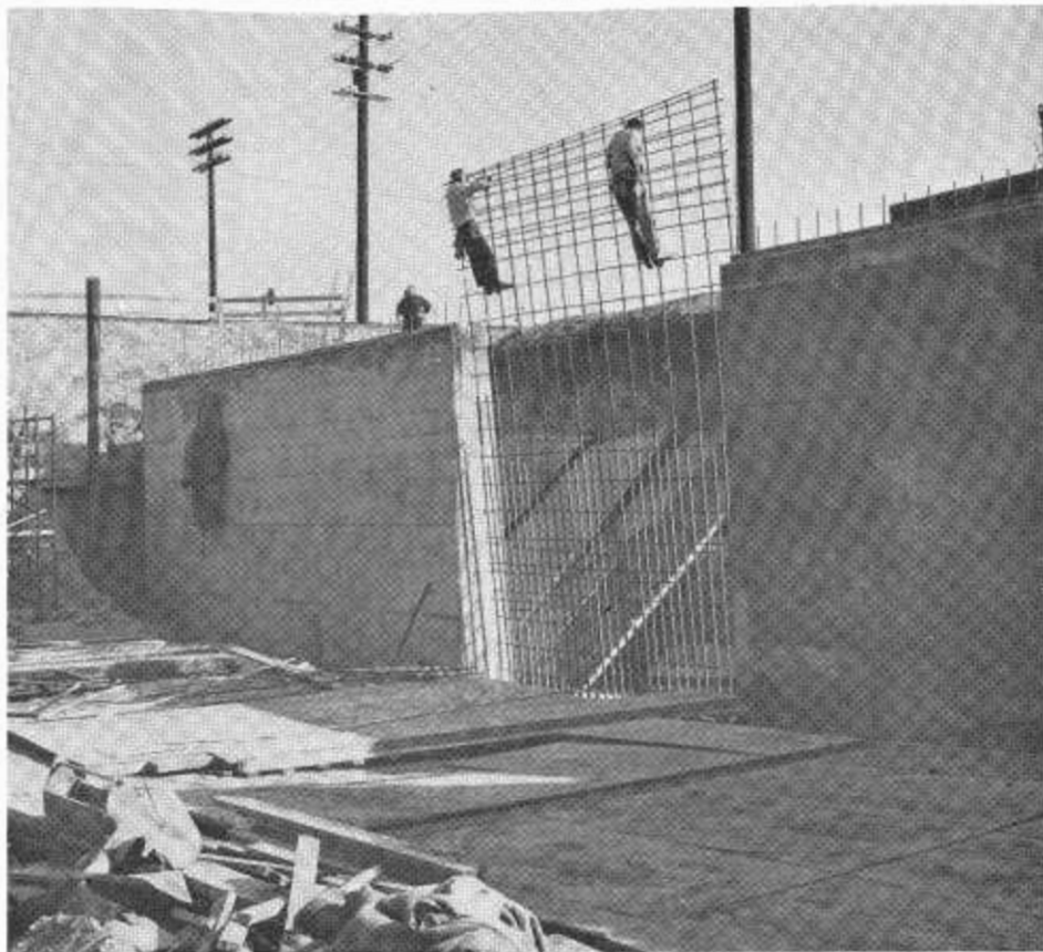
Workmen place reinforcing steel in the south retaining wall of the Harding Way Underpass.
