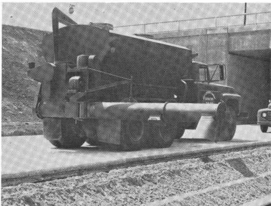
A cement spreader truck. This type of equipment can easily deposit cement within the tolerance allowed by California's 1960 Standard Specifications. (Above photos by Pettibone Wood Mfg. Co.)
