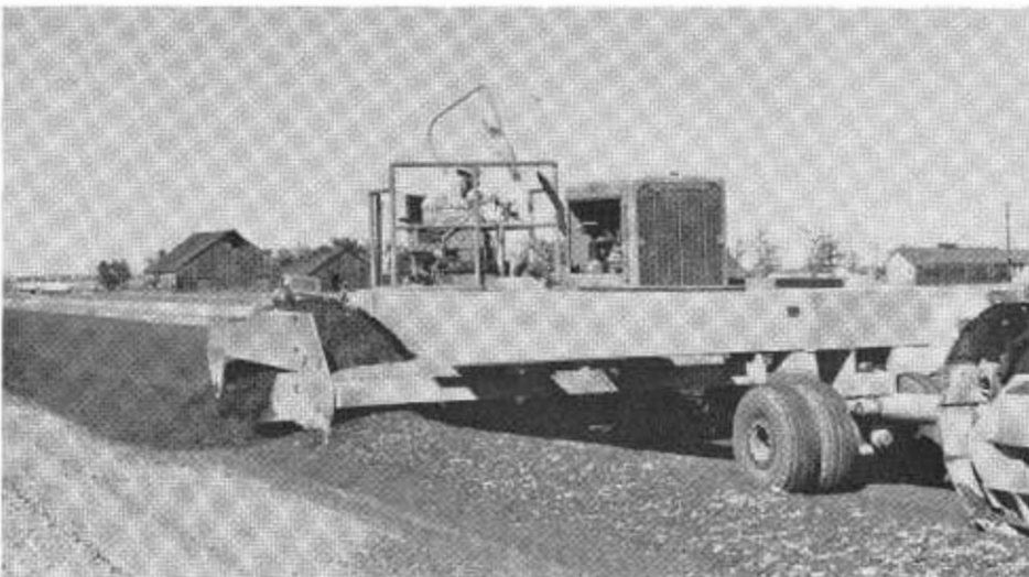
A land-plane type grader finishes the cement-treated base in advance of slip-form concrete paving operations.
