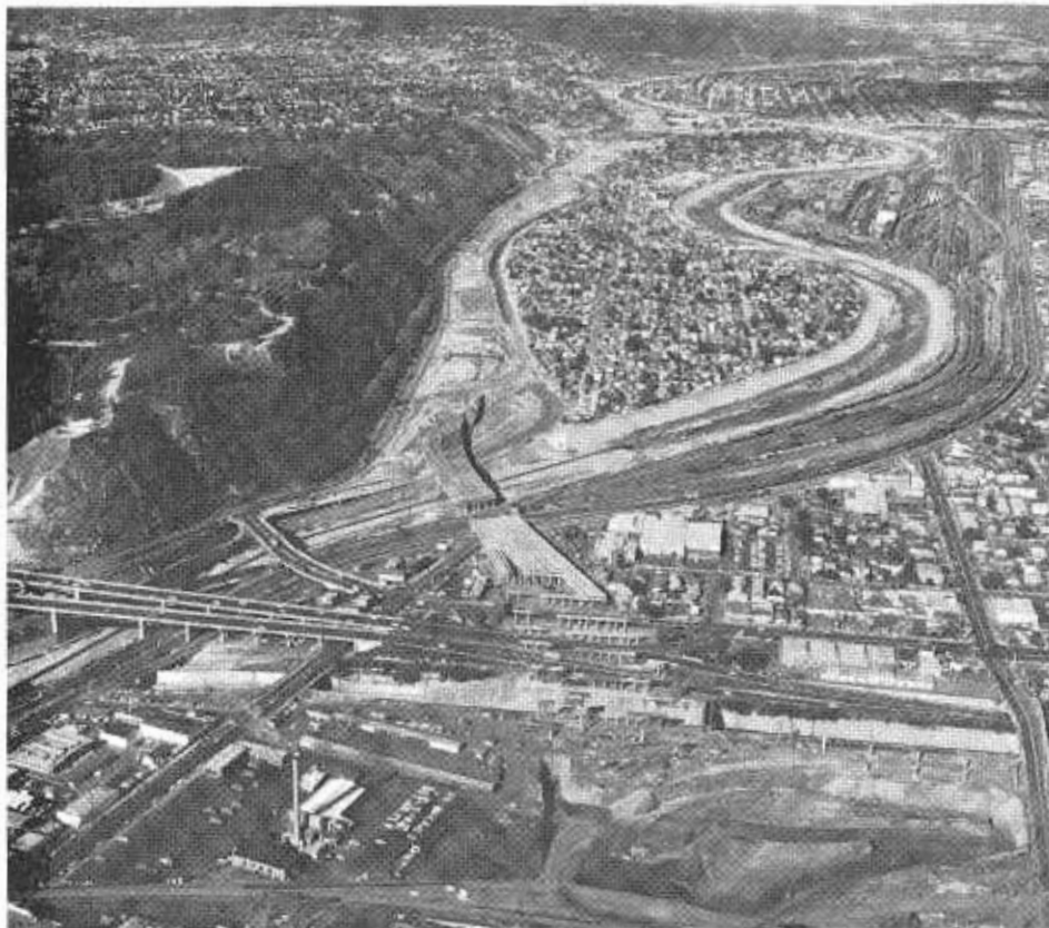
The Elysian Viaduct and Pasadena Freeway interchange on the Golden State Freeway. Note columns and steel already placed. Winding through the photo at right is the Los Angeles River.
