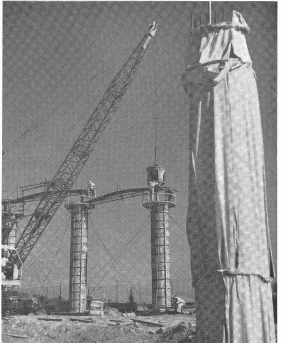
A crane with a hopper and elephant's trunk pours columns for bridge structures on the Golden State Freeway-Glendale Freeway interchange.
