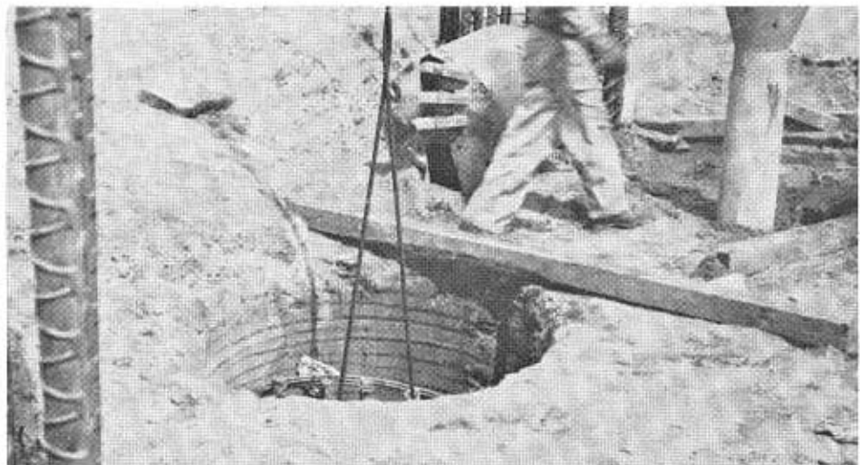
FIGURE 3. Geologic conditions must be right for the pile to be used; namely no ground water, and material that does not cave in.
