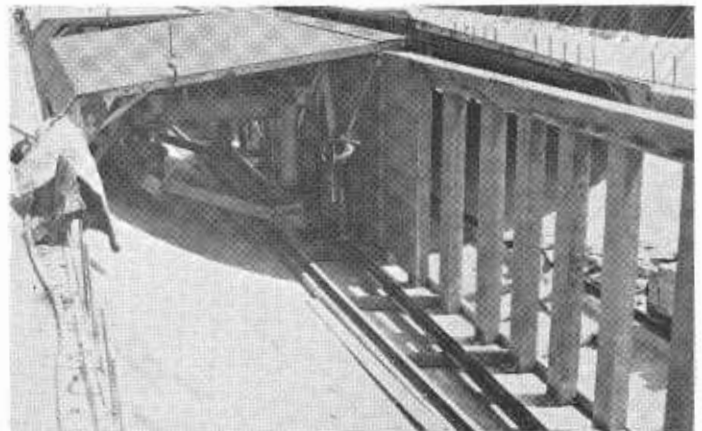
The roadway deck form is being lowered into place and a portion of the longitudinal left open for the construction of a steel transverse bulkhead after completion of the deck concrete.
