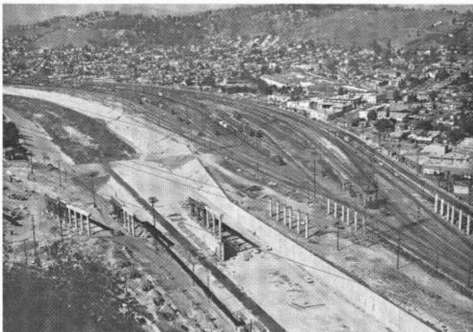
Columns across the Los Angeles River and adjoining railroad tracks prior to erection of steel girders. This is the Elysian Viaduct section of the Golden State Freeway.
