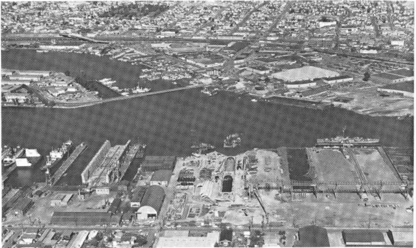
This picture shows the casting yard and the equipment used in constructing 12 precast tube segments, which cost a total of $4,440,000 when delivered to the right-of-way and ready for sinking into position. The amount of the Division of Highways construction contract is $16,641,000, and the contractor has invested about $800,000 in constructing the graving dock and about $300,000 in tube forms. Two segments are constructed at the same time in tandem and launched by flooding the dock and removing the gate. A construction cycle requires about 10 weeks, and a high tide of more than five feet is required for launching. The segment nearest the water is covered with timber lagging installed to protect the waterproofing, while the other segment shows the black waterproofing. (Photo by Aero Photographers)
