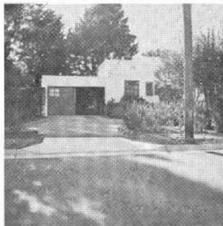
AFTER—The curb, gutter and driveway following reconstruction and resurfacing of the street.
