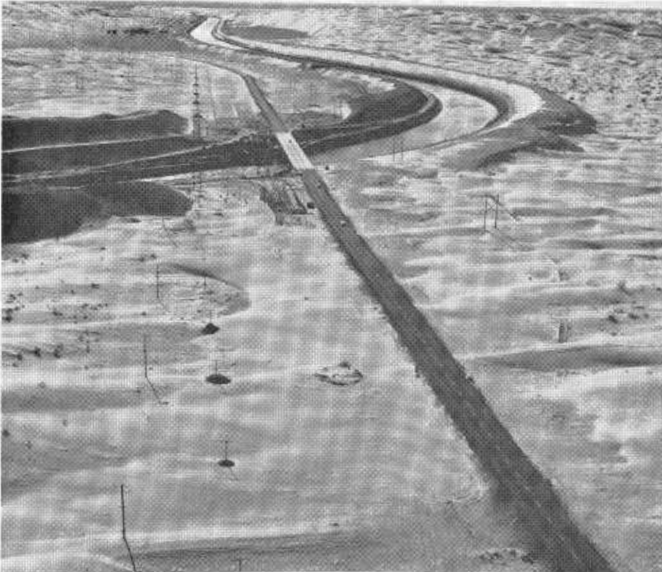
A westward view of construction on U.S. 80 showing the bridge across the All American Canal. A second bridge is being built to the left of the existing one.
