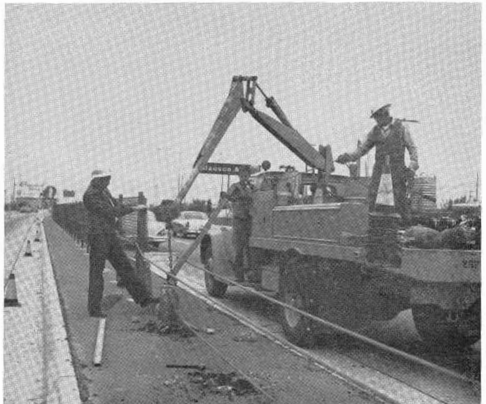
A crew removes a damaged post prior to replacement of a new section of fence.
