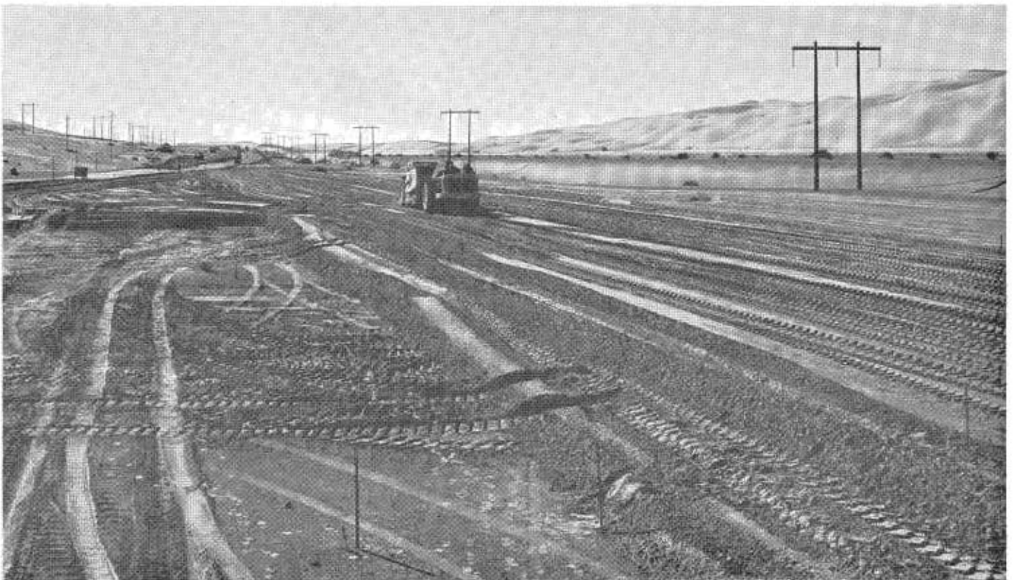
Grading operations on the current reconstruction of U.S. 80 through the Sand Hills. The present highway is on the left.
