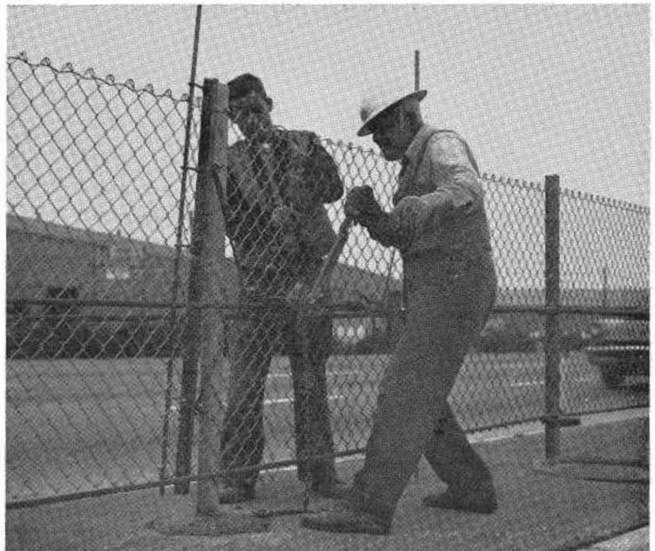
Members of the maintenance crew tighten up the reinforcing cable in the replaced section of fence.
