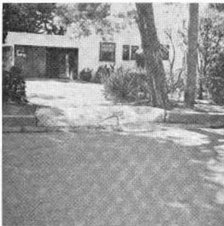
BEFORE—A broken curb, gutter and driveway prior to reconstruction.
