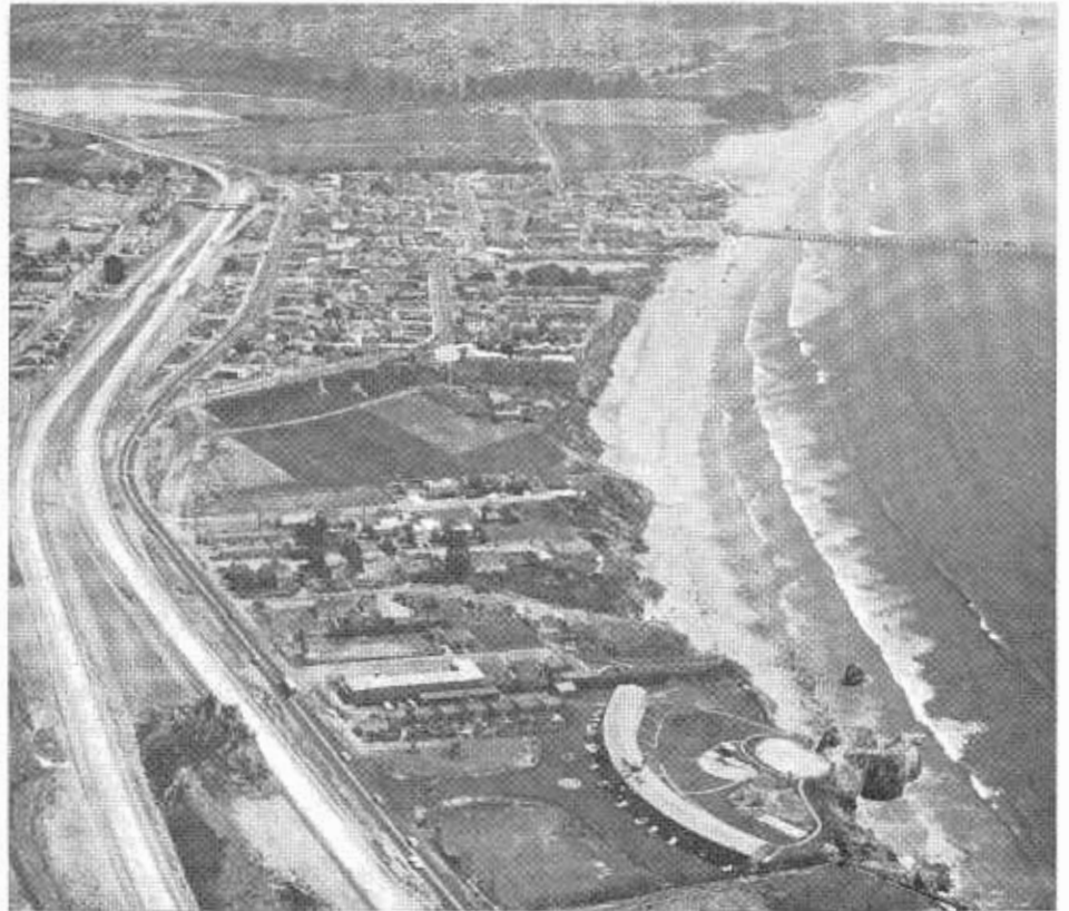
A southward view of the Pismo Beach Freeway under construction with traffic still using the old highway which parallels the southbound freeway lanes.
