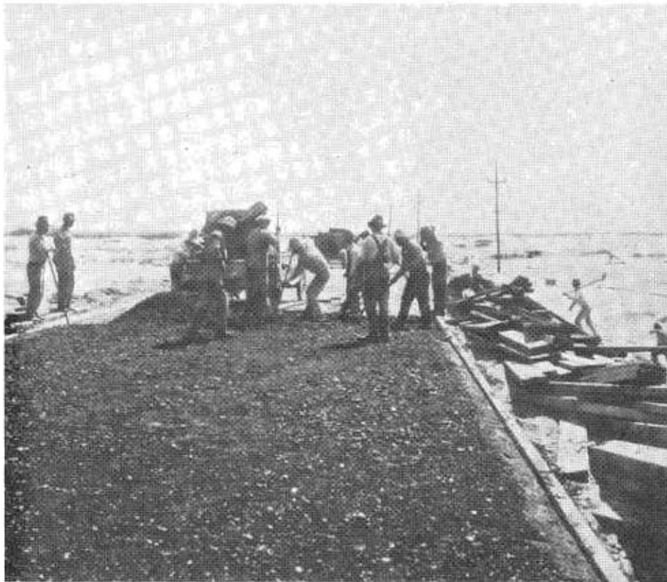
This 1925 photo shows a crew laying pavement on U.S. 80. The planks on the right laid crossways to support trucks carrying asphalt to the construction area.
