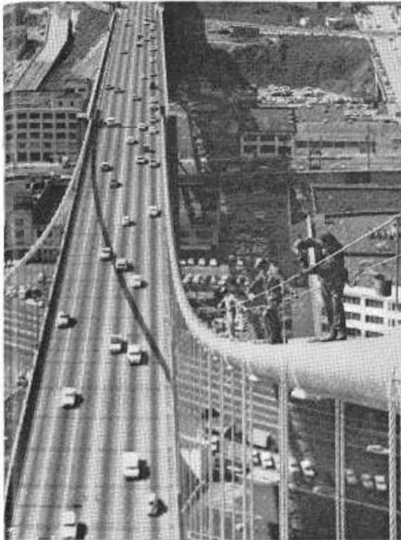
FRONT COVER—Members of the paint crew work on one of the main cables of the San Francisco-Oakland Bay Bridge high above the City of San Francisco. (See "Painting the Bridge," beginning on page 5.) —Photo by Bob Dunn
