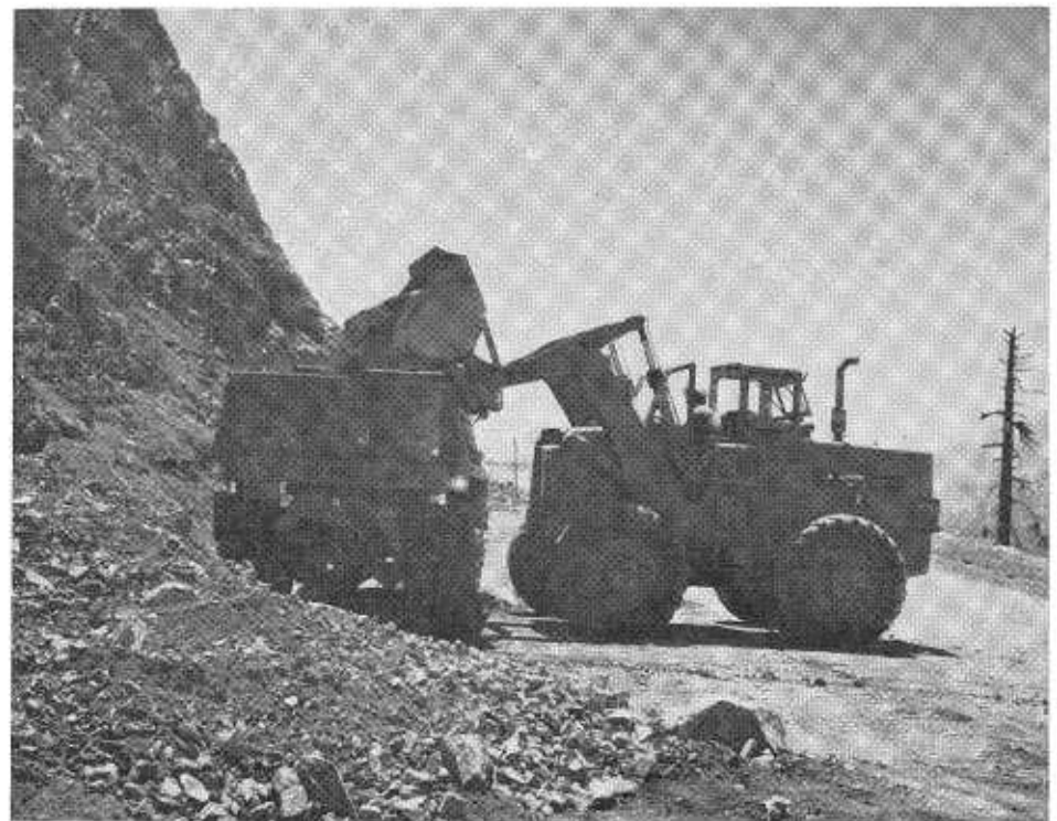
Slide Removal Operation. The rock is then loaded into trucks for removal from the site.
