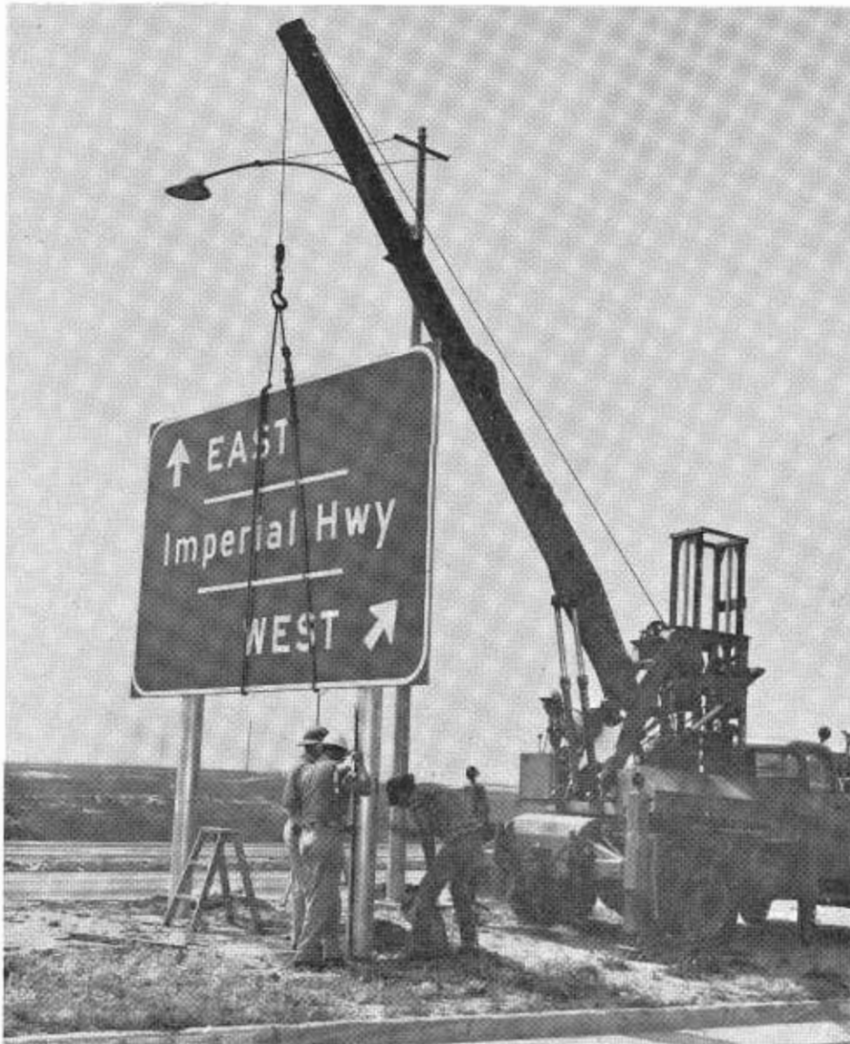
Following assembly, the crew raises the sign and secures the posts in the ground.
