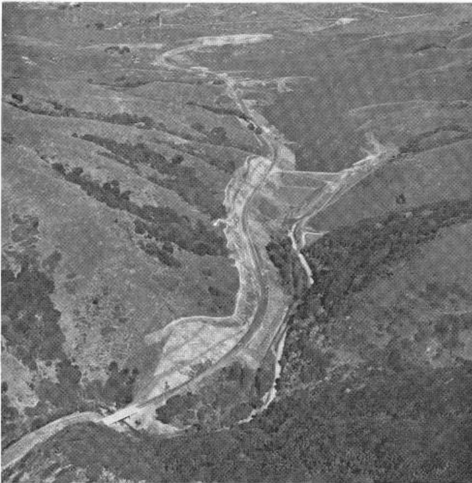
A northerly view of the Marin Water District's Nicasio Dam and rerouted section of Nicasio Road (FAS Route 879). The reservoir behind the dam is not yet full.
