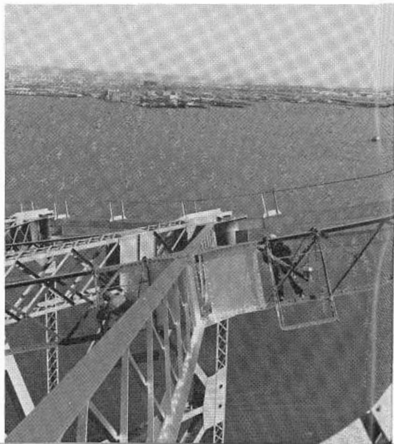
Painting the aluminum finish coat on top of the lateral bracing in the cantilever structure.
