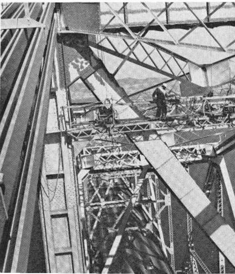
The first spot coat painting is applied on one of the towers of the East Bay cantilever section using air-powered hoists on trussed aluminum scaffolds designed by members of the Bay Bridge staff. The view is eastward with the Berkeley hills in the distance.
