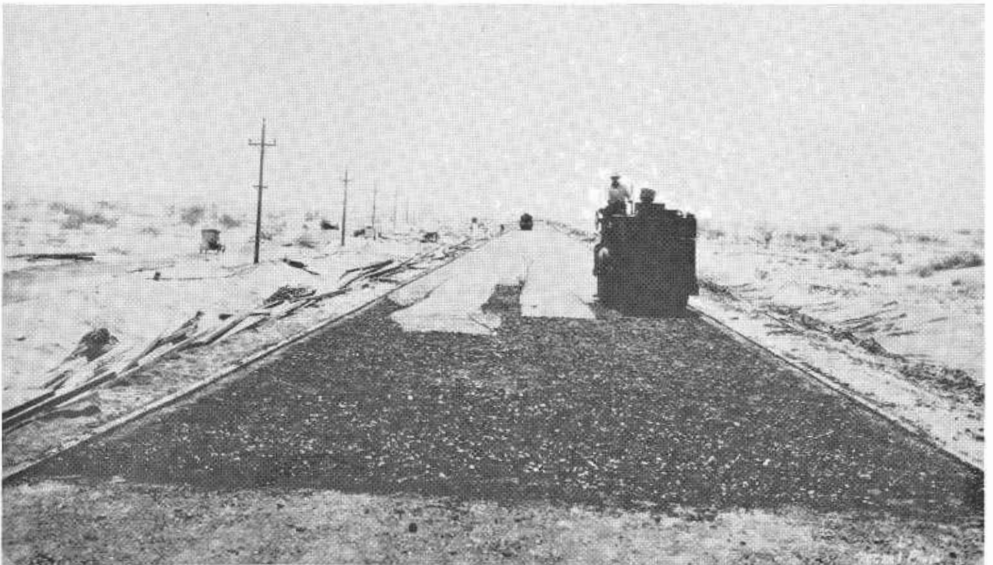
This photo was taken during construction of the 20-foot wide asphalt concrete road built in 1925.
