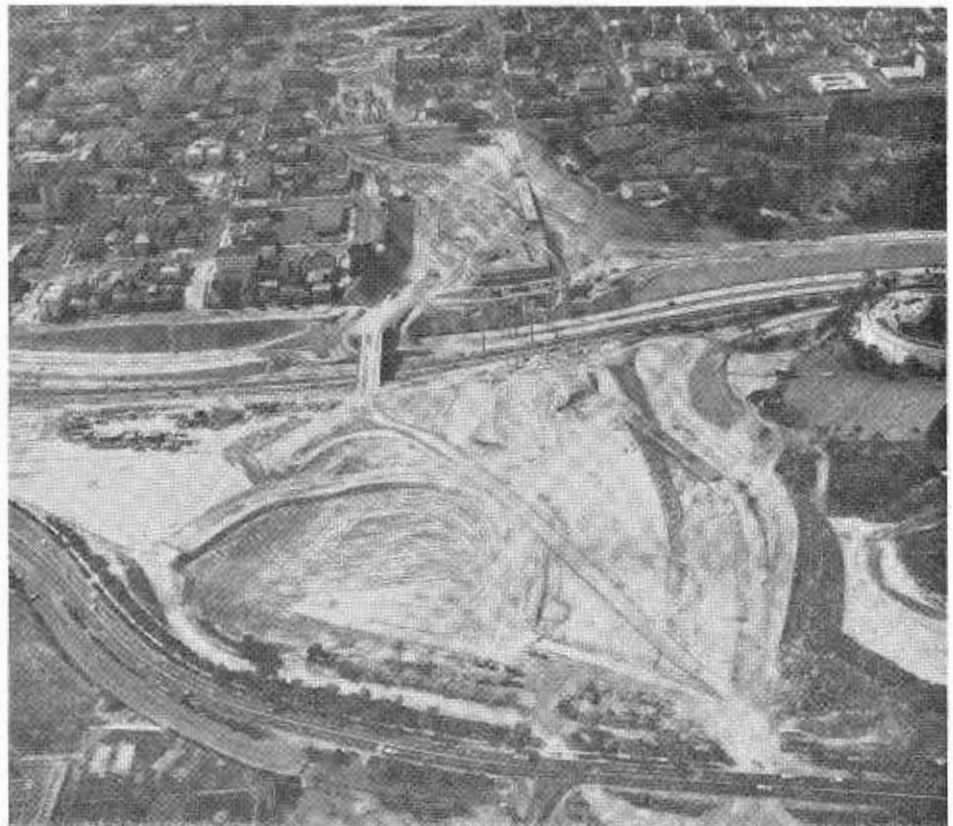
The four-level interchange under construction in San Diego showing the temporary haul bridge over the Cabrillo Freeway. The view is westward.
