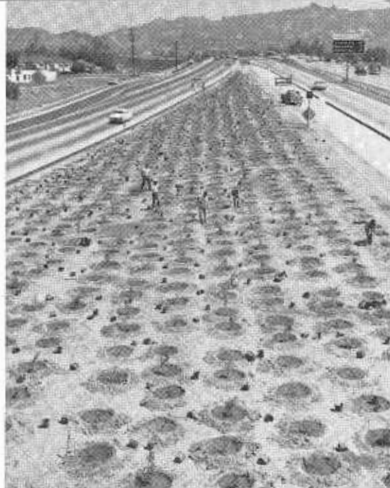
Photo of contractor's crew planting interchange on Hollywood Freeway Extension in North Hollywood gives good idea of scope of planting jobs. Small circles are wetted planting holes with newly planted shrubs. Dots are empty gallon cans.
