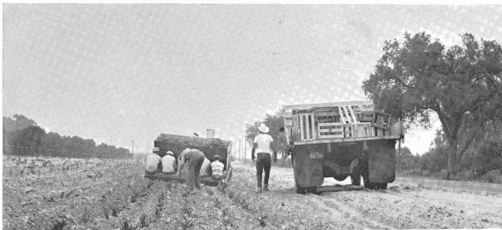
BELOW. Contractor's crew and equipment planting iceplant cuttings in median, Santa Ana Freeway, near Tustin.
