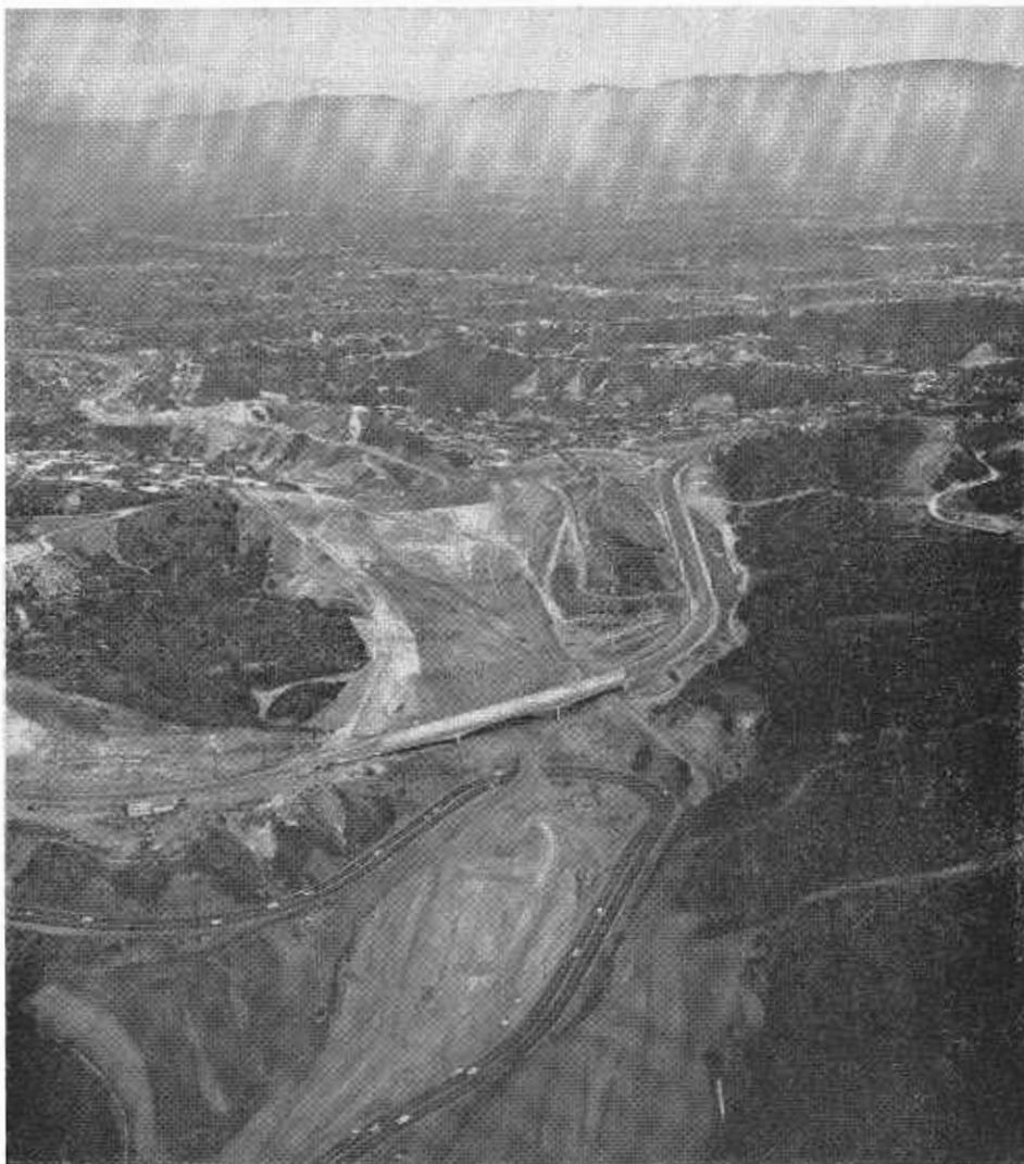
Looking north along the San Diego Freeway construction area. Existing horseshoe curve on Sepulveda Boulevard, center, and relocated Mulholland Drive and bridge, foreground.
