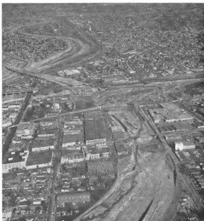
Looking northerly at construction in progress along Golden State Freeway; top, left, Elysian viaduct and interchange facilities with the Pasadena Freeway.
