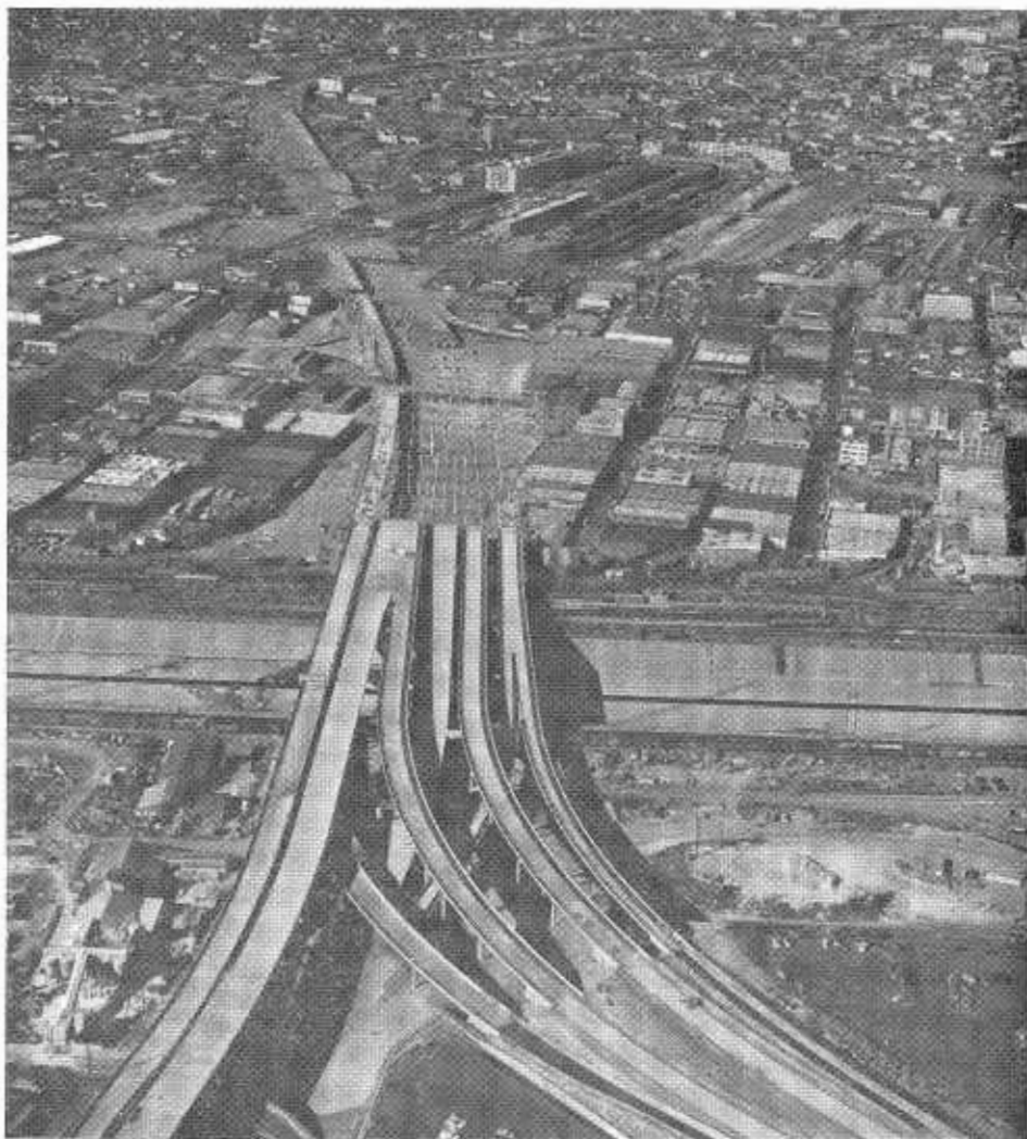
Looking westerly along Santa Monica Freeway (from Los Angeles River) at construction in progress; foreground, part of East Los Angeles interchange.
