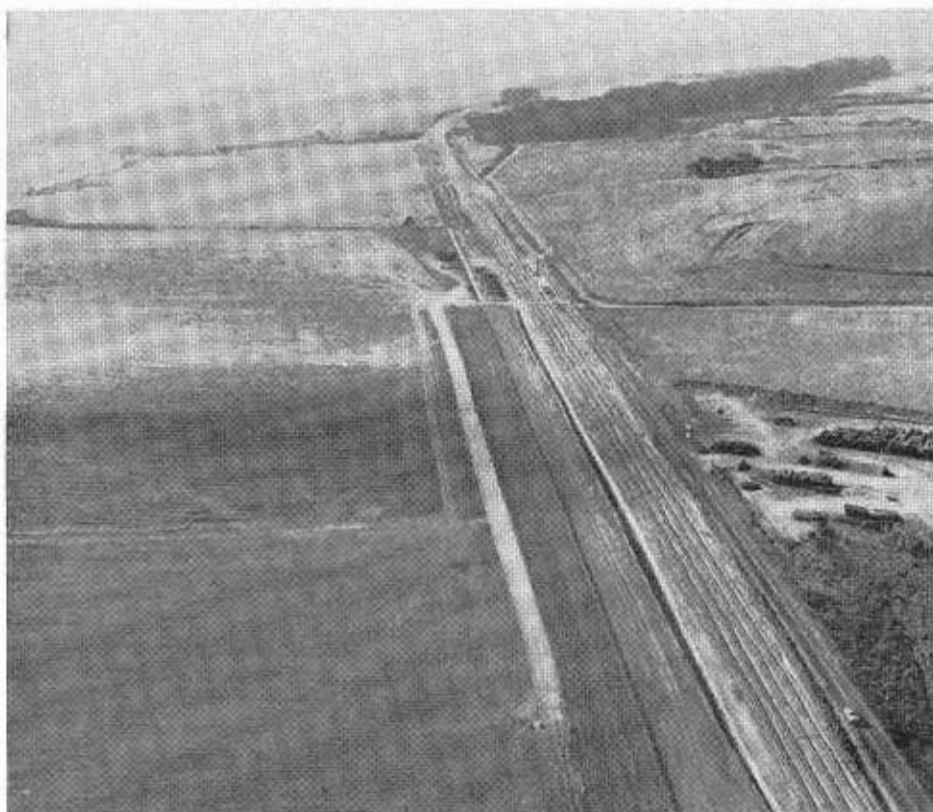
Construction between Whitehouse and New Years Creek on Sign Route 1, the final project to receive a contribution from Joint Highway District No. 9.
