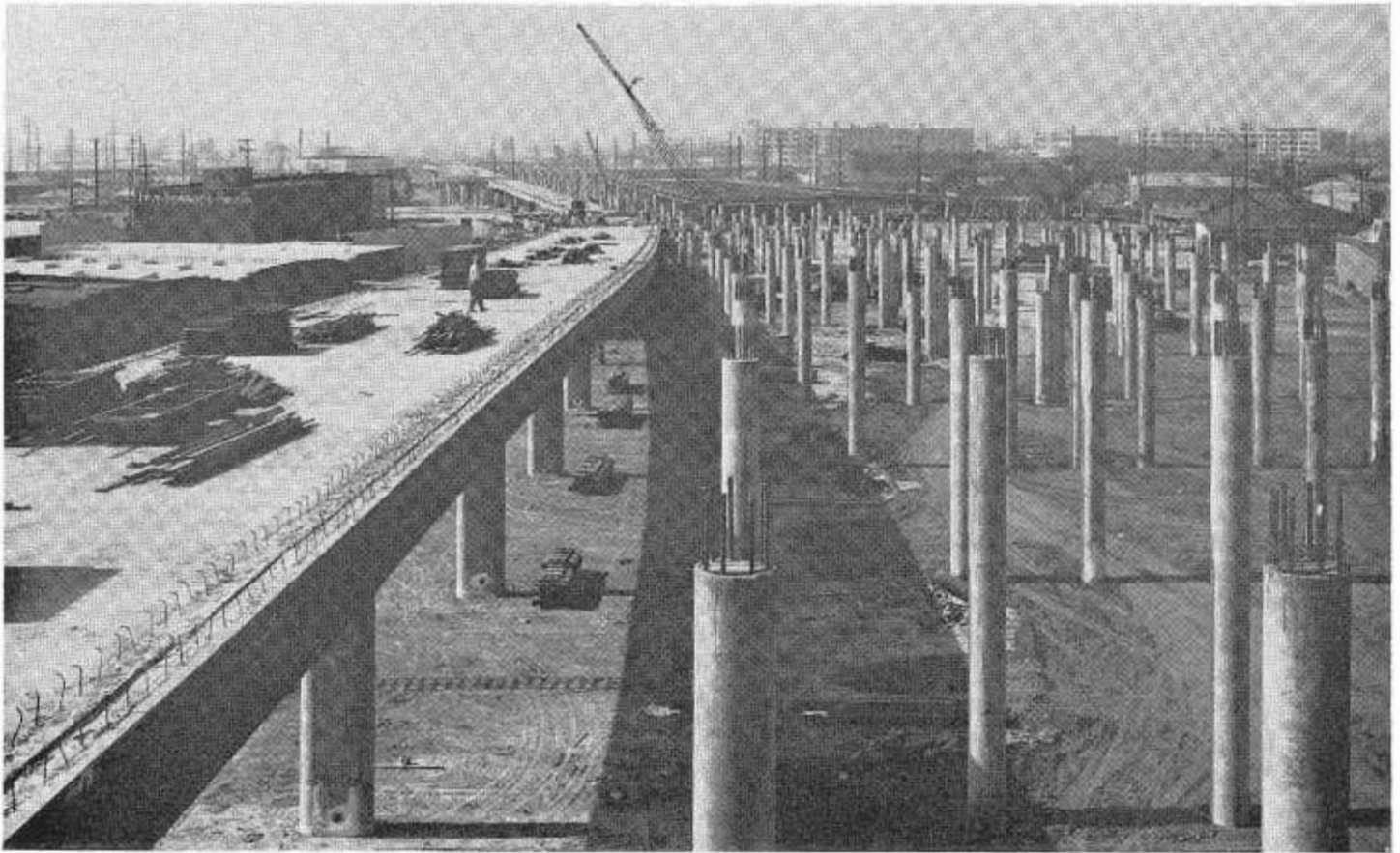
Looking westerly along Santa Monica Freeway construction from Santa Fe Avenue near Los Angeles River.
