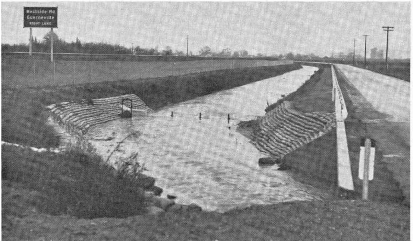
Looking south at the beginning of the Norton Slough channel change. The freeway is shown (left) and the frontage road (right). The flow of water to the slough on the other side of the freeway is controlled by the 24-inch pipe partly visible above the water in the reinforced embankment to the left.
