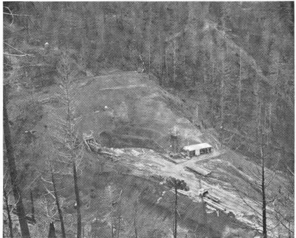
Driving of the pilot bore at the north portal of the new Hazelview Tunnel, part of a realignment project on U.S. 199 in Del Norte County.
