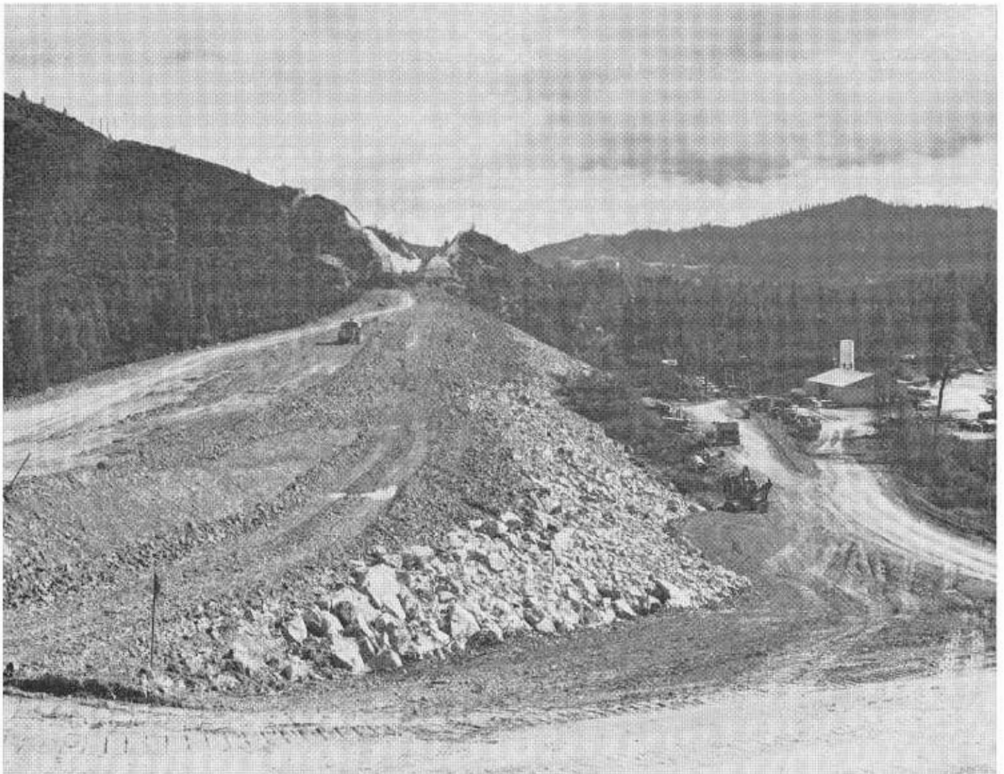
Partly completed embankment across Whiskey Creek Arm viewed from west end. The benched cuts are on the east side of the creek.
