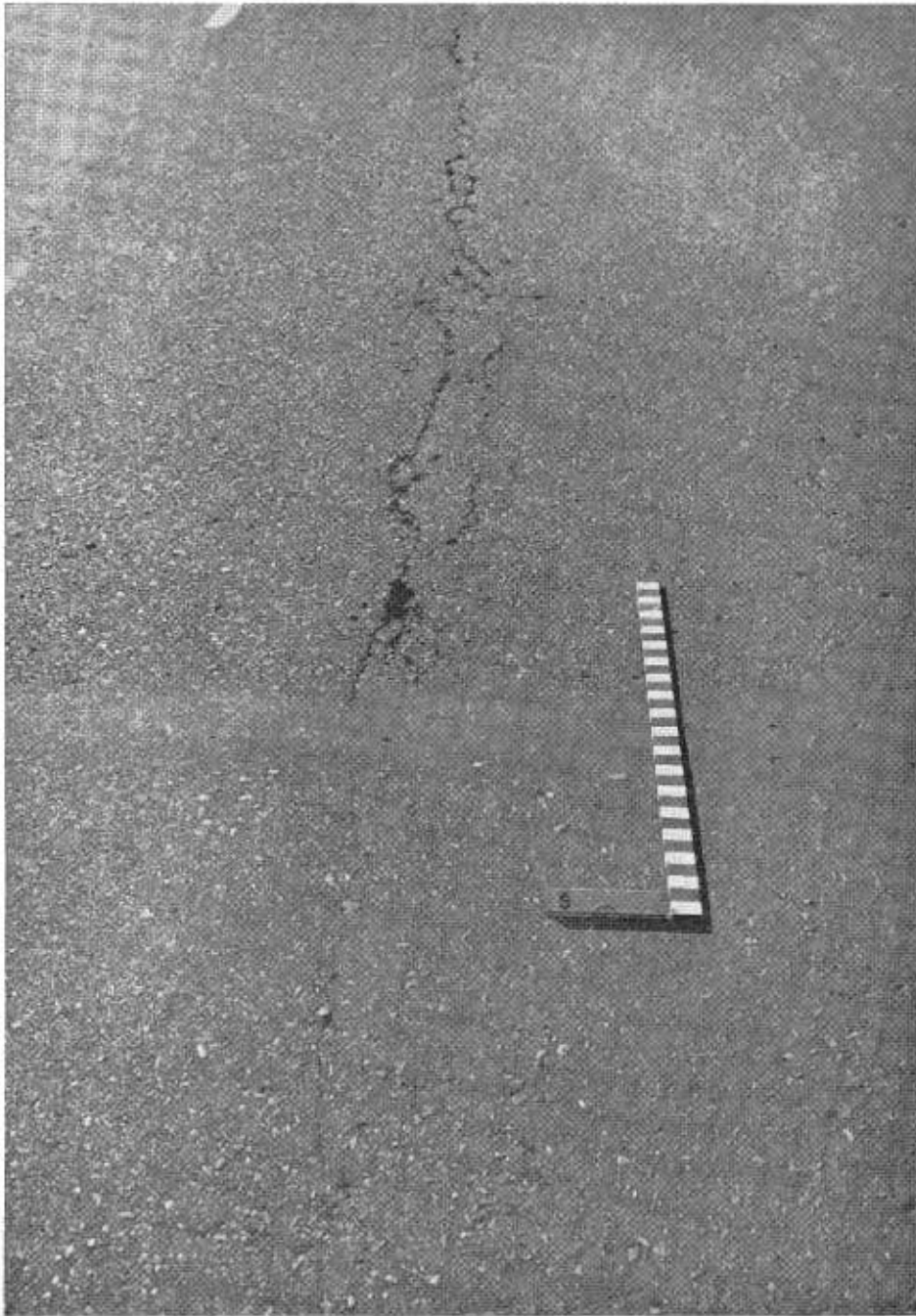
The junction between Asphalts D (foreground) and E (background) after 45 months of service life. Note spalling along longitudinal crack in the E section.
