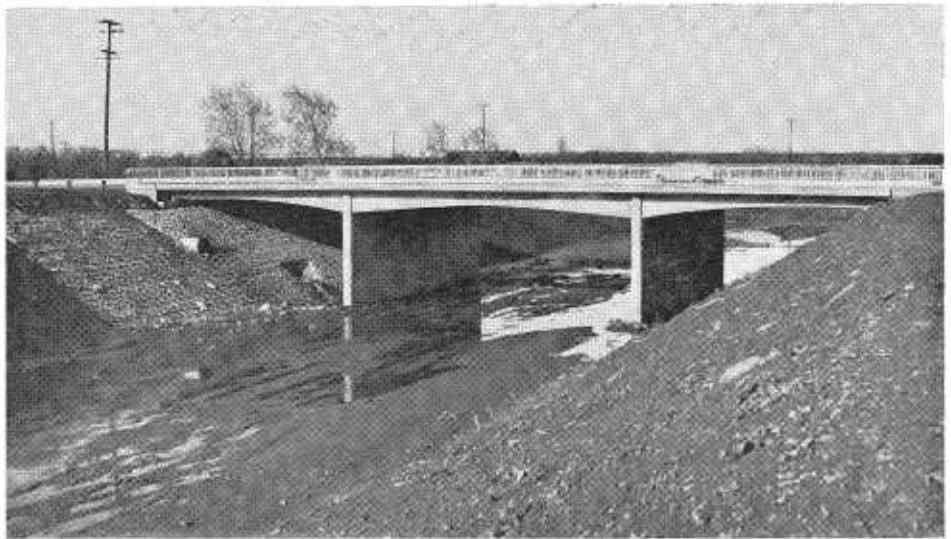
A view of the improved Guadalupe River channel at Brokaw Road Bridge.
