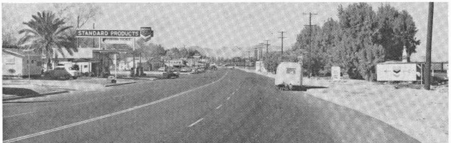
Looking east toward Needles showing new curb and gutter with surfacing striped for four lanes.
