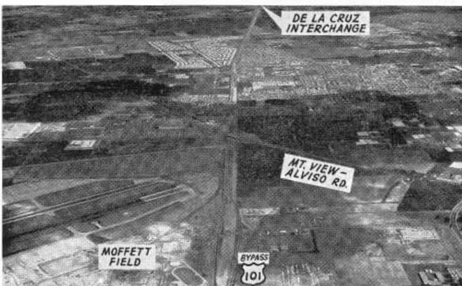
Bayshore Freeway construction in the Mountain View area with Moffett Field indicated (left foreground).
