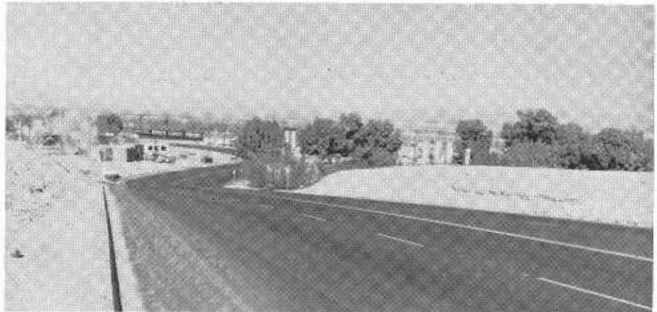
Looking northwest toward Needles showing the widening of the roadway with improved grade and alignment.
