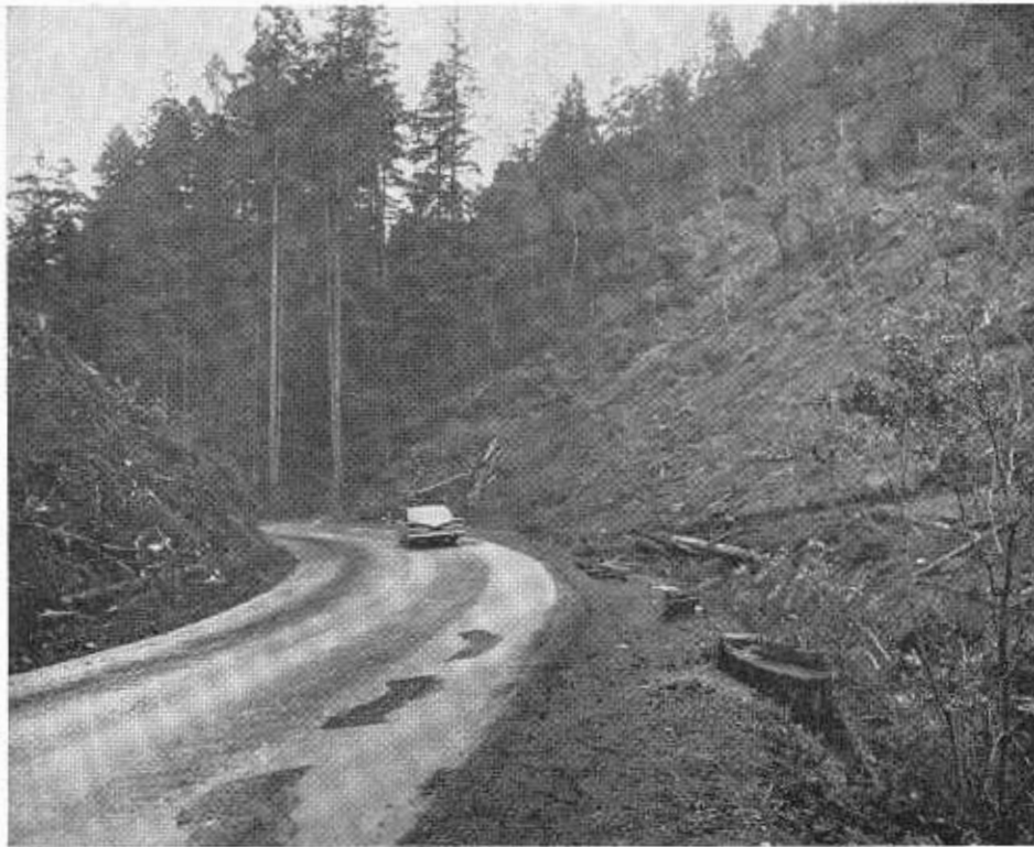
This northward view of the relocation of U.S. 199 shows the present highway and some of the clearing work being done on the new alignment.
