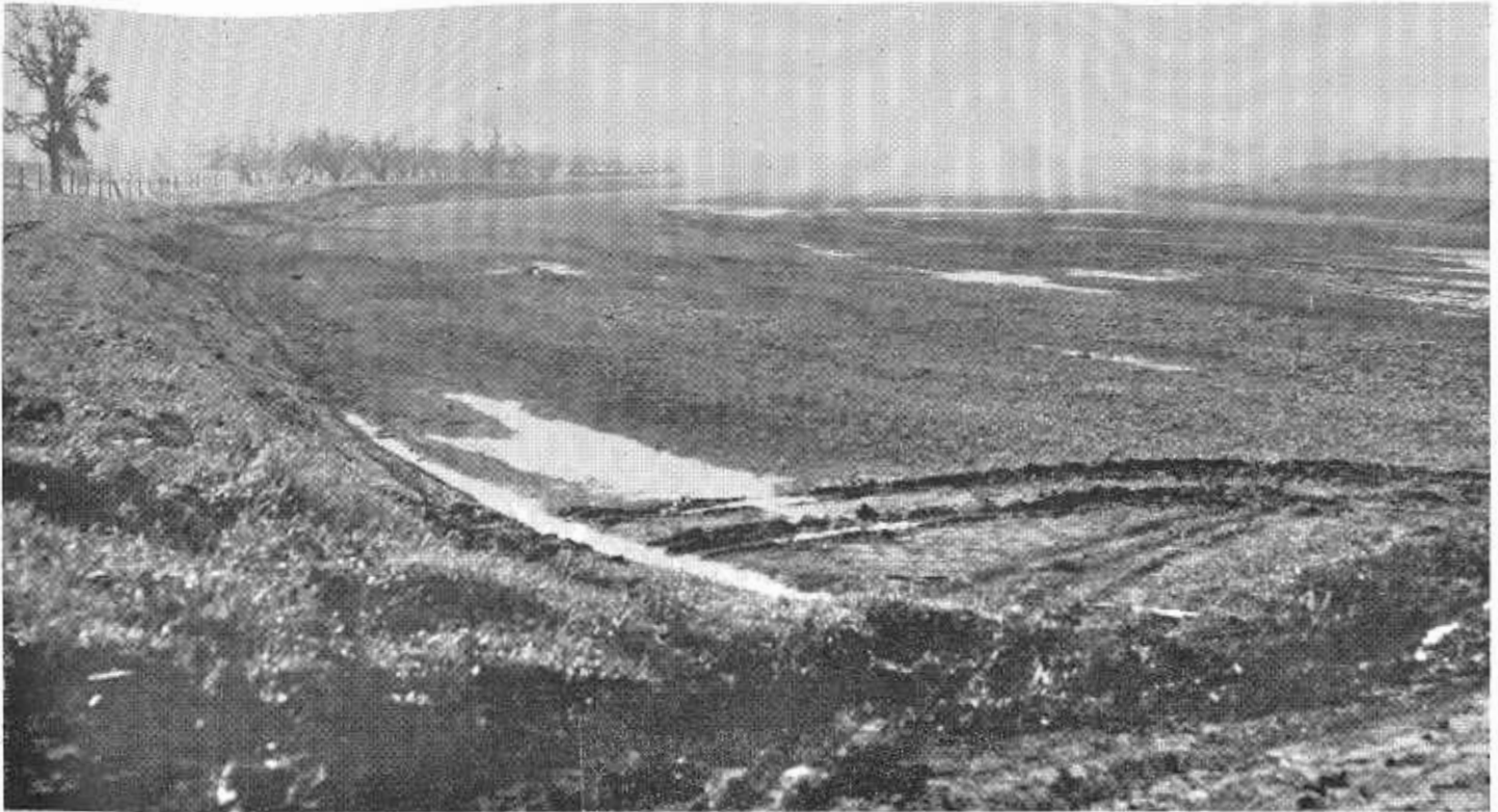
Looking south at the completed first stage of channel relocation which will serve for flows in excess of 7,000 cubic feet per second.
