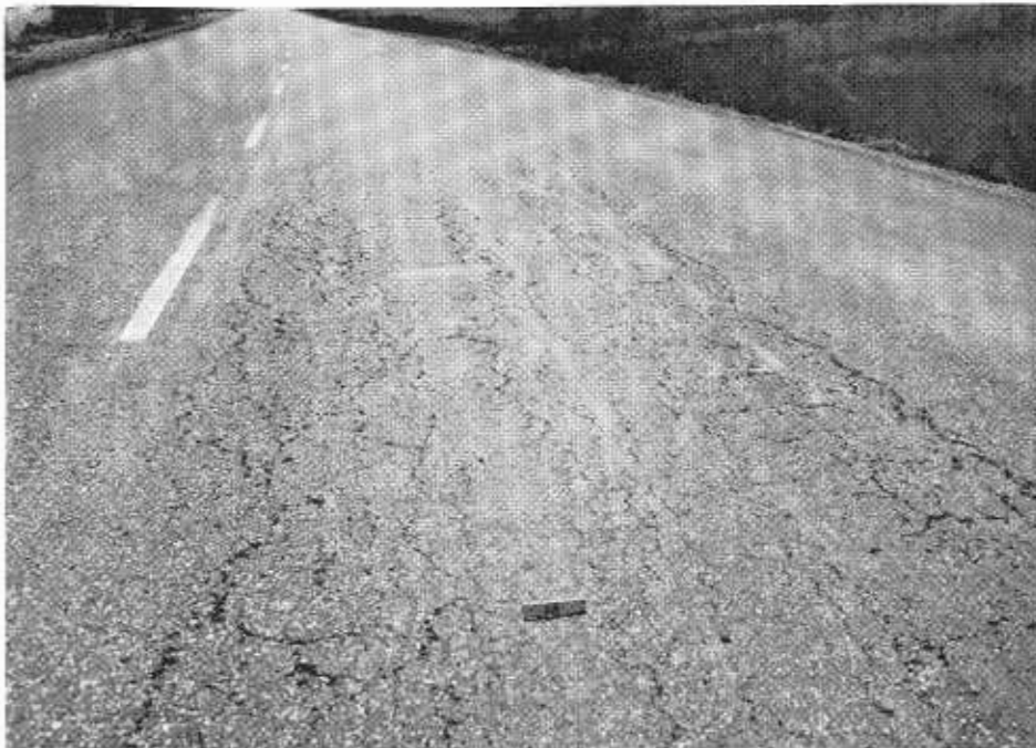
Typical condition of the major portion of the Asphalt E travel lane is shown here after 45 months of service life.
