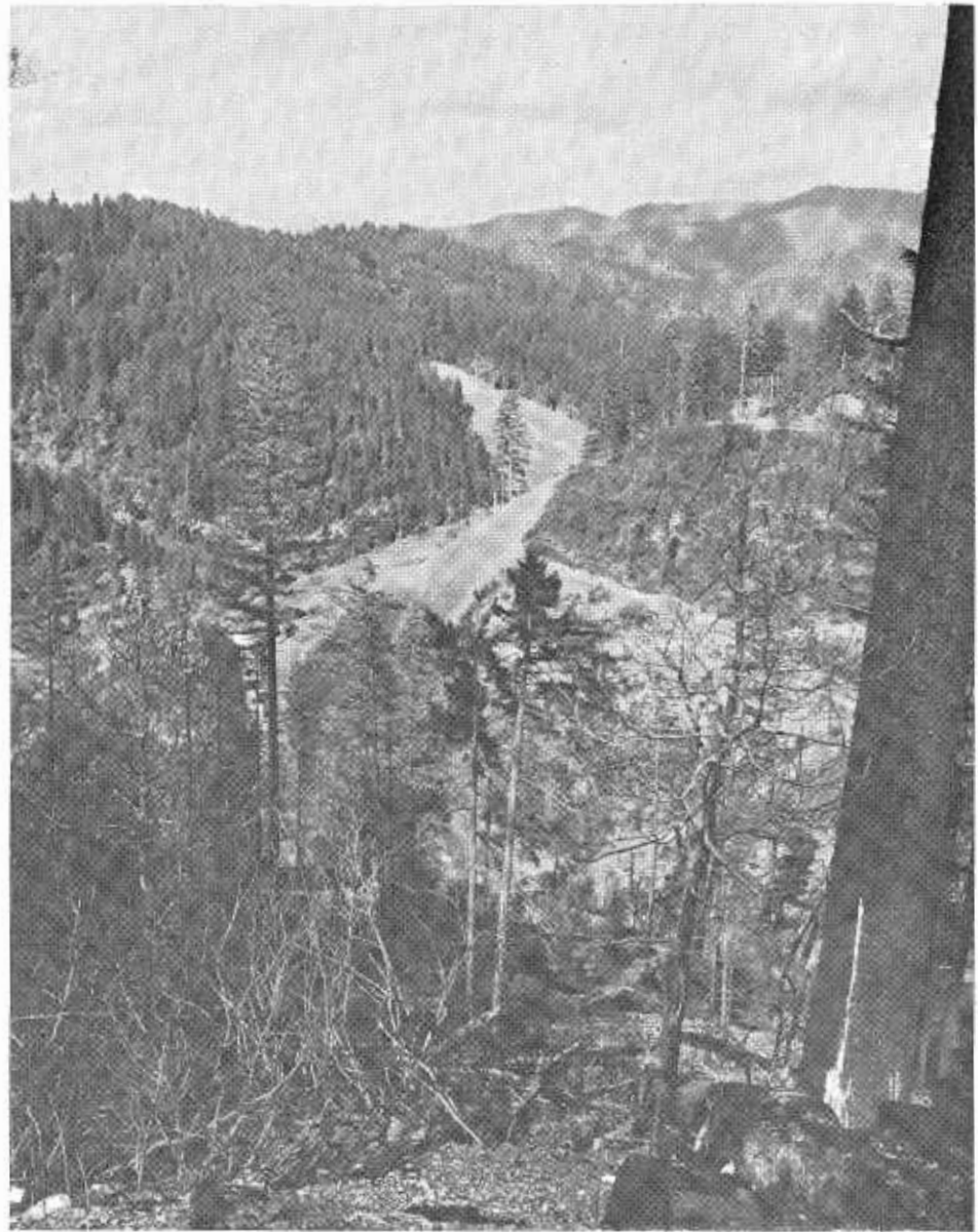
Looking northeast along the completed rough grade of the north approach to the Hazelview Tunnel. North portal of the tunnel is hidden by the trees (left center). The big fill is across Broken Kettle Creek.
