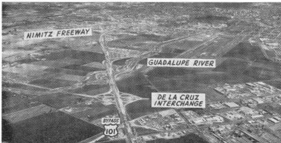
Looking south toward San Jose from above the Bayshore Freeway under construction.
