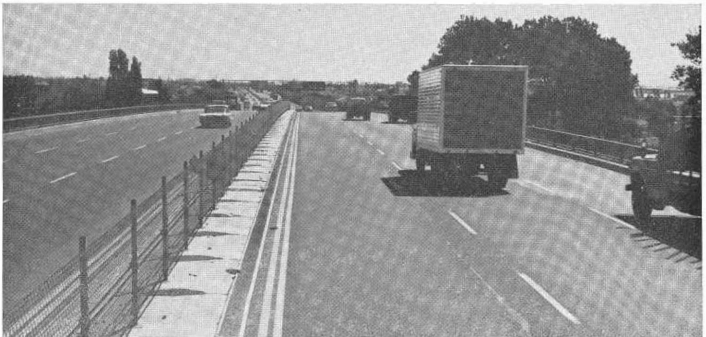
Median barriers are being installed to prevent cross-median head-on collisions on heavily traveled freeways such as this section of the Nimitz Freeway in Oakland. Shown here is the fence-cable barrier developed by the Division of Highways in a series of crash tests.
