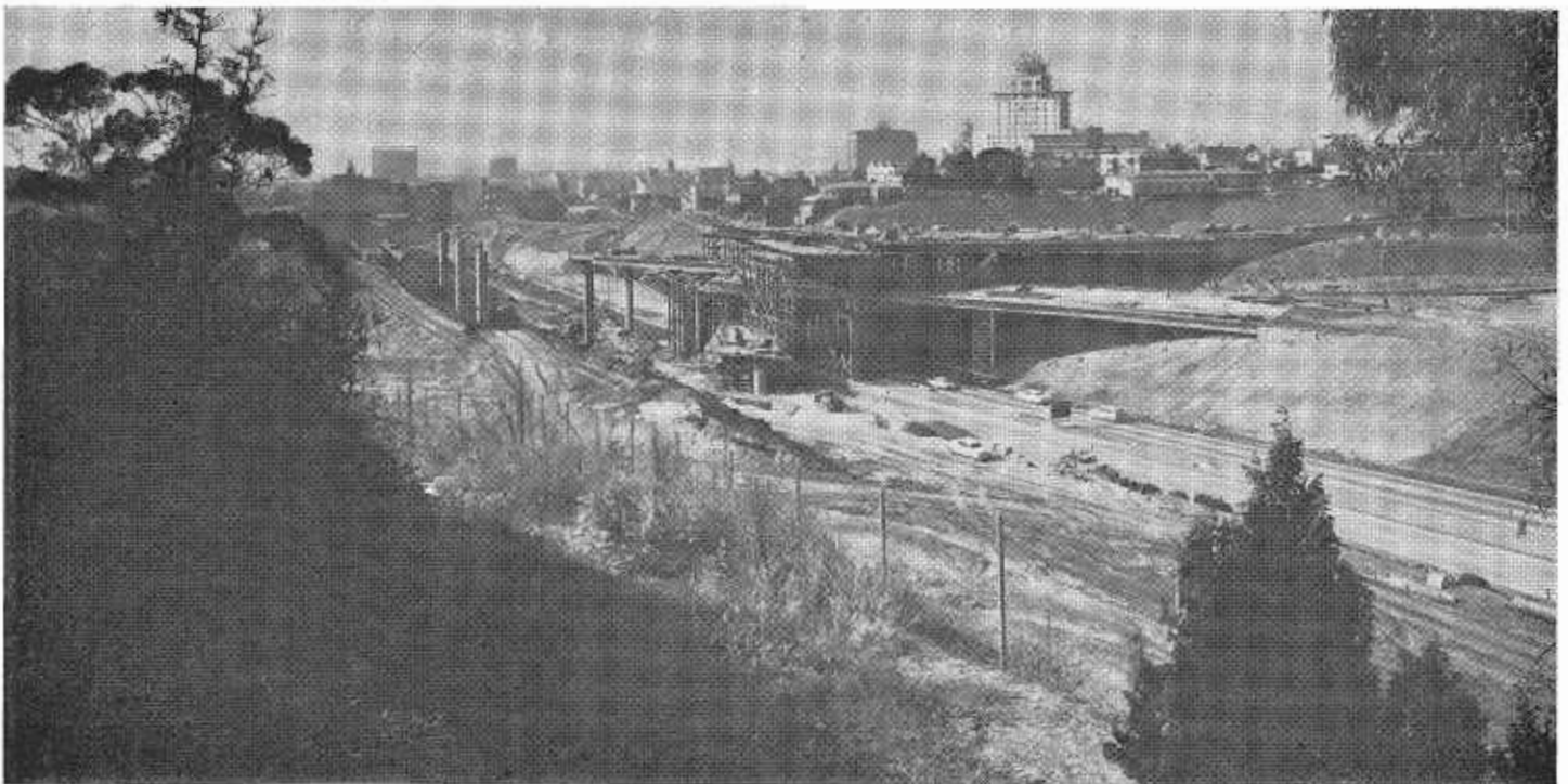
An important element in the future freeway system for metropolitan San Diego will be this four-level interchange which is now under construction.
