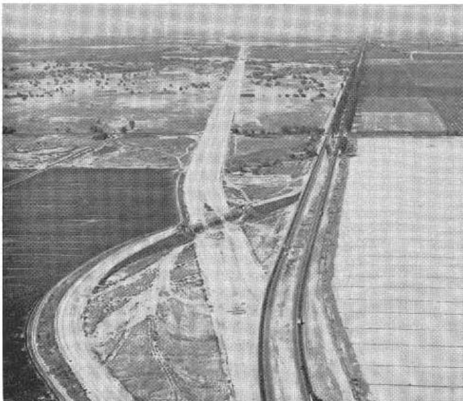
Looking north along the future US 99 freeway route (left) and the present highway near Wheeler Ridge in Kern County. This new freeway section will be a part of a bypass freeway now under construction in and north of Bakersfield.
