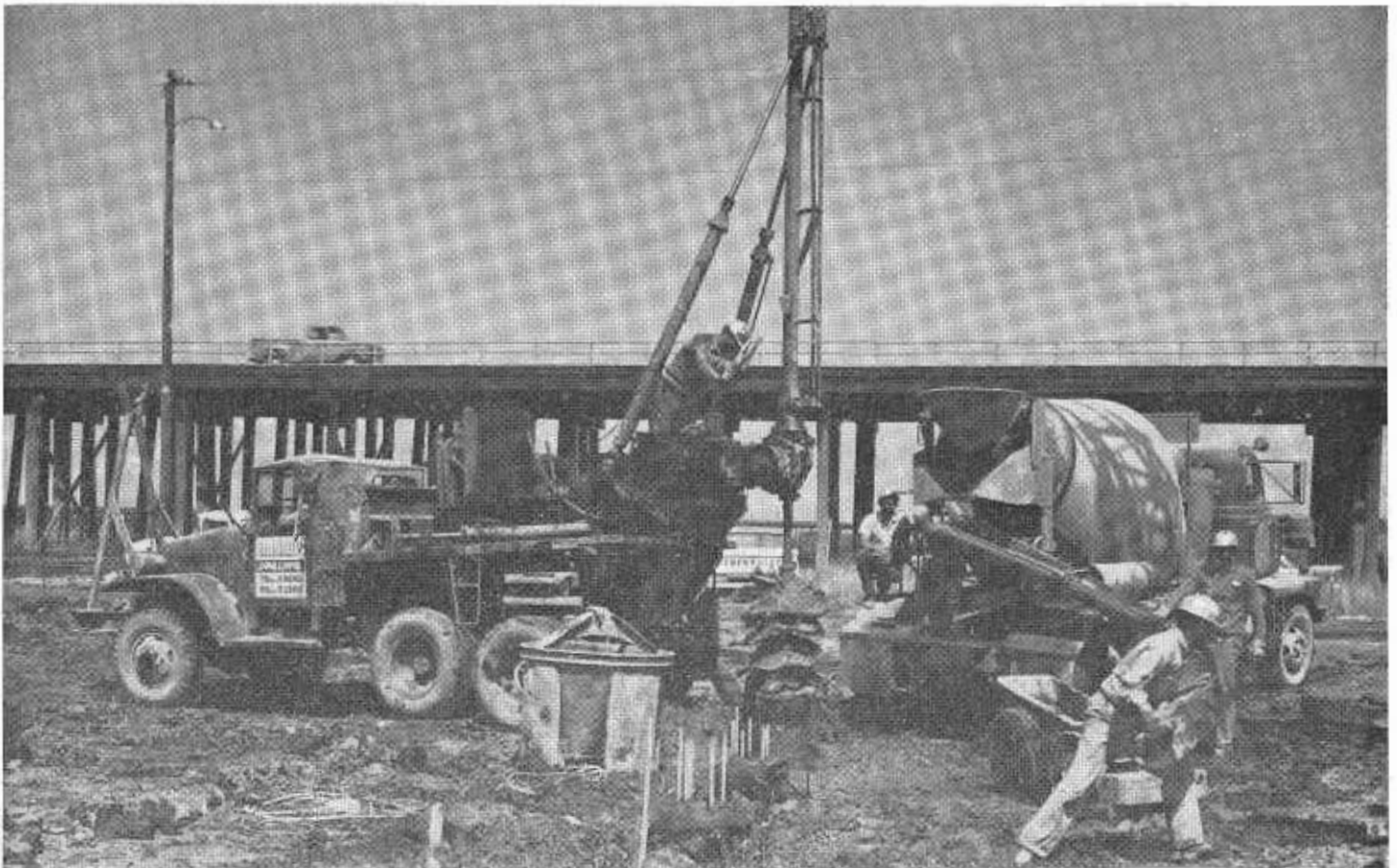
Construction workers are building a new bridge-fill freeway crossing of the Yolo Bypass on US Highway 40 west of Sacramento. The freeway will replace an existing causeway which carries the only remaining section of undivided highway between San Francisco and the state capital.
