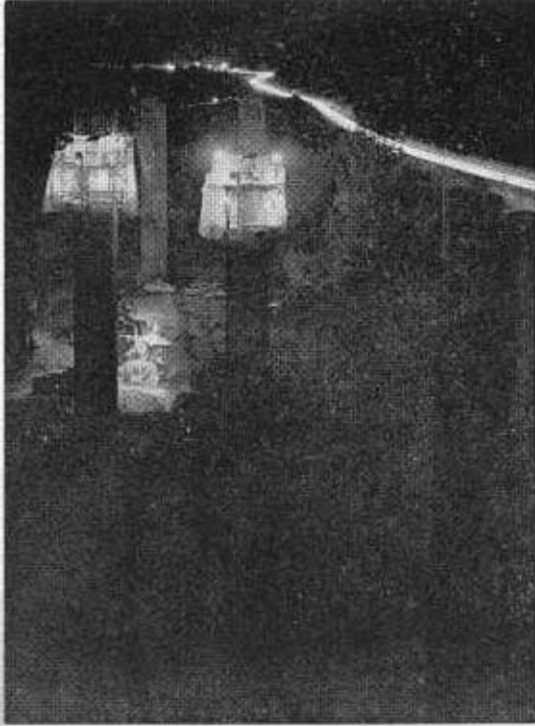
Night construction on the Webber Creek Bridge which will be part of a new section of U.S. 50 freeway west of Placerville.
