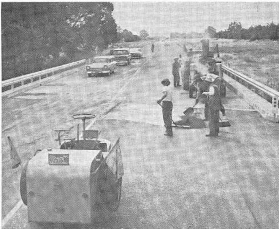
Maintenance crew is shown patching pavement on U. S. Highway 99E near Chico. Work of this type is part of the day-to-day routine for highway maintenance workers throughout the State.
