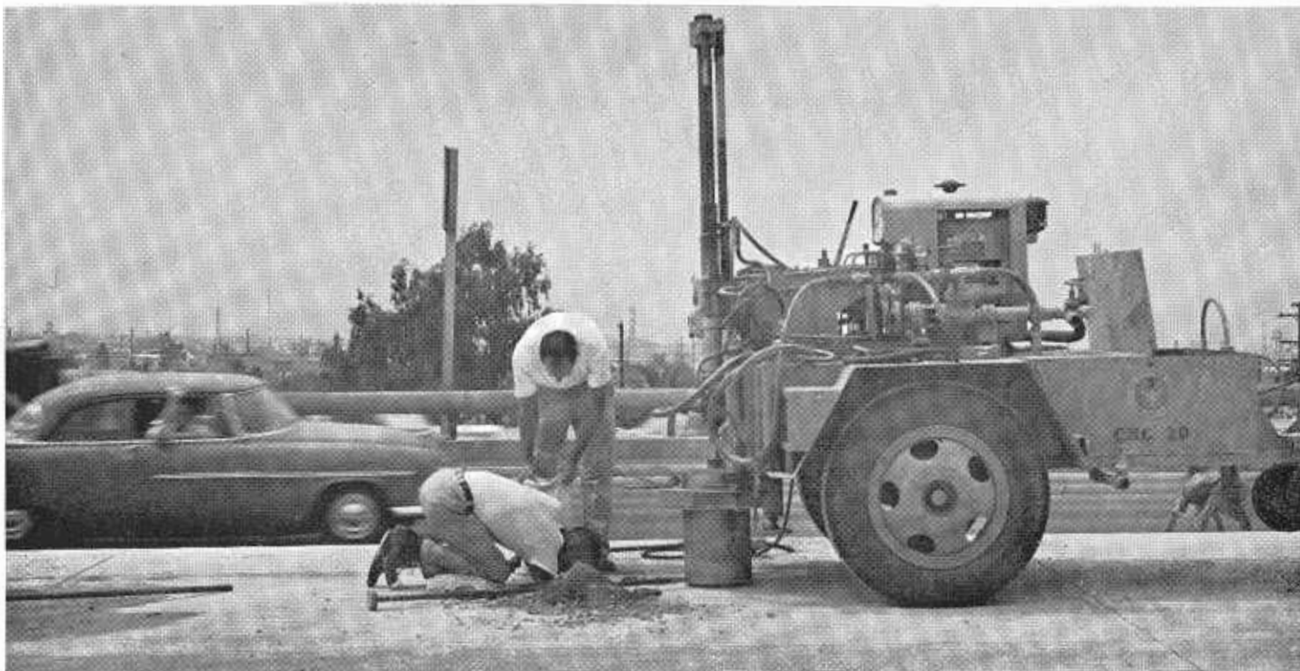
A Materials and Research Department crew takes a sample of pavement base and subbase on a new section of highway. The sample will be checked to make sure that specifications have been met. This auditing of materials and construction assures high quality work on state highway projects.
