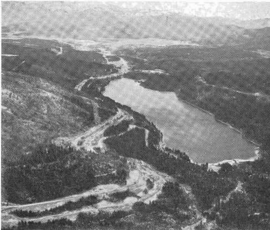
Work is progressing on the relocation of US Highway 40 to provide an interstate freeway over Donner Summit and past Donner Lake. The new freeway will replace the present twisting highway at right. As shown in the photo, part of the summit freeway will be a "split level" design with roadways separated by a stand of trees.
