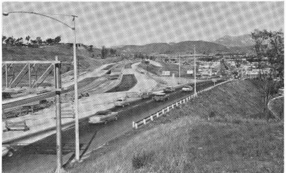
A ground level view showing same section as in aerial above, at later stage in construction. Old road gives access to business section. This portion of freeway was opened in May of this year.
