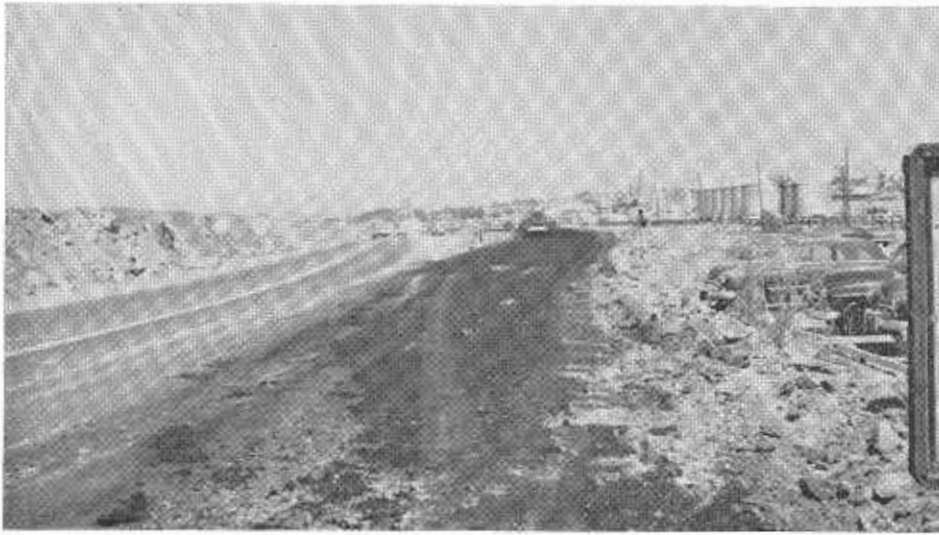
This photo shows the temporary detour being constructed to the right of the existing highway. The main portion of the fill can be seen to the left.
