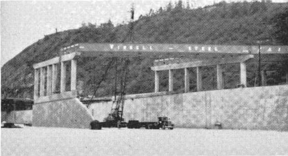
Erection of structural steel for the Elysian Viaduct is shown at the crossing of the Los Angeles River.
