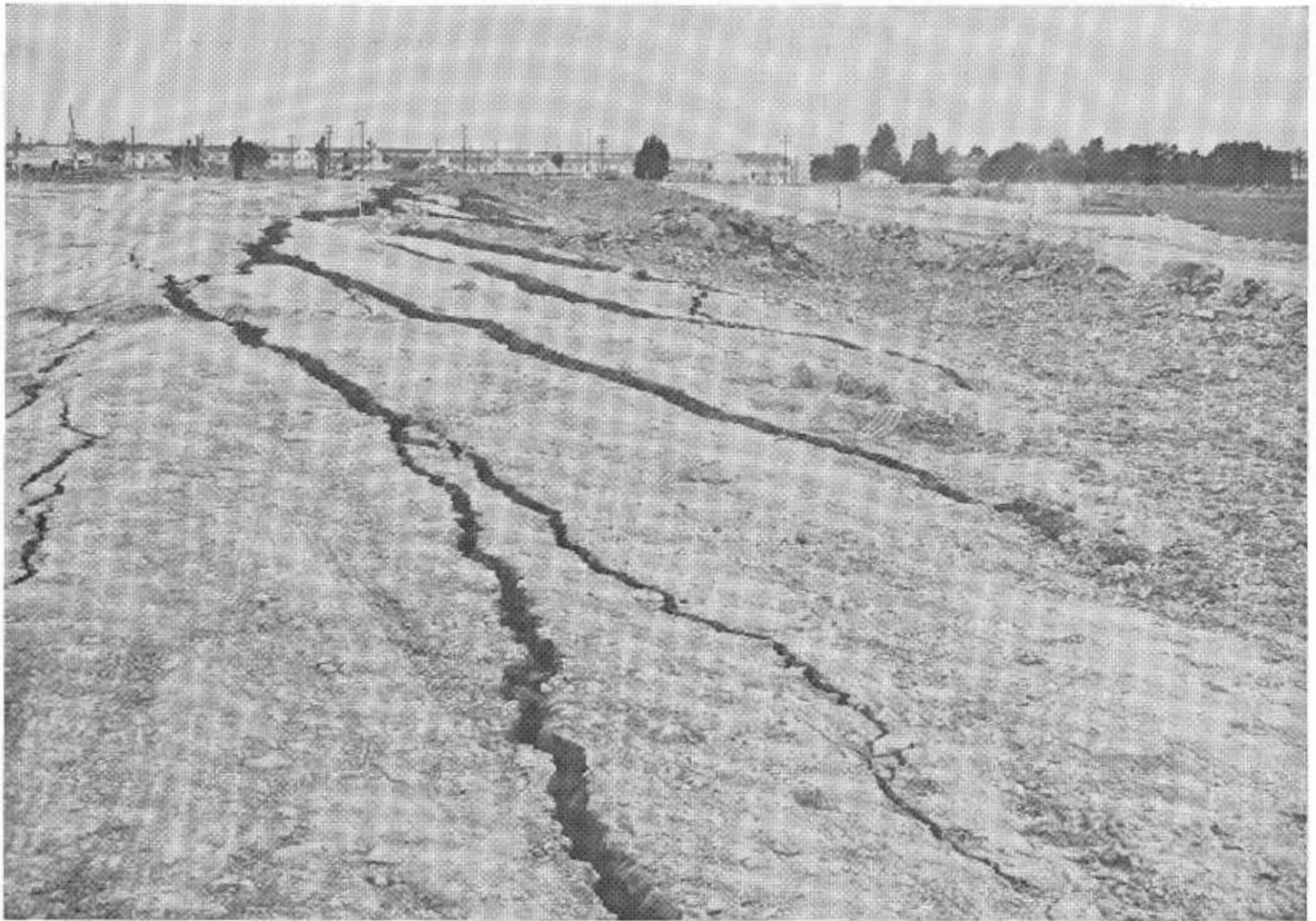
This photo shows the failure of the left side of the main fill which occurred on September 27, 1960.
