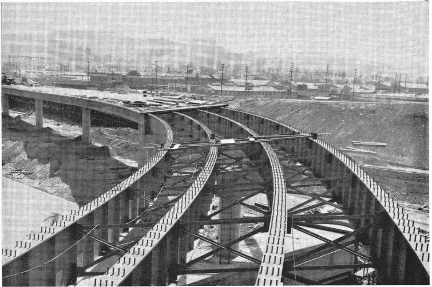
The On-Ramp to the Elysian Viaduct from the south is a steel girder structure curved to fit the roadway curvature.
