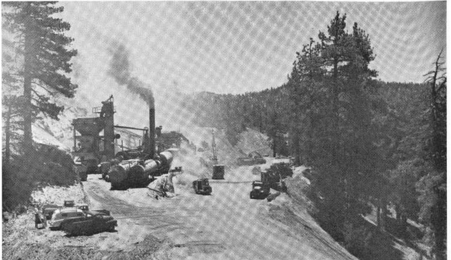
A view of the new highway during construction showing a paving plant in operation to the left of the roadway.
