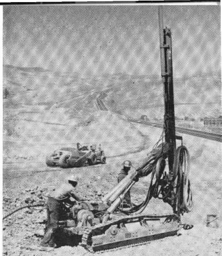
Wagon drill in operation as first step in blasting for roadway excavation and fill at American Canyon. Blasted material will be used for fill below.
