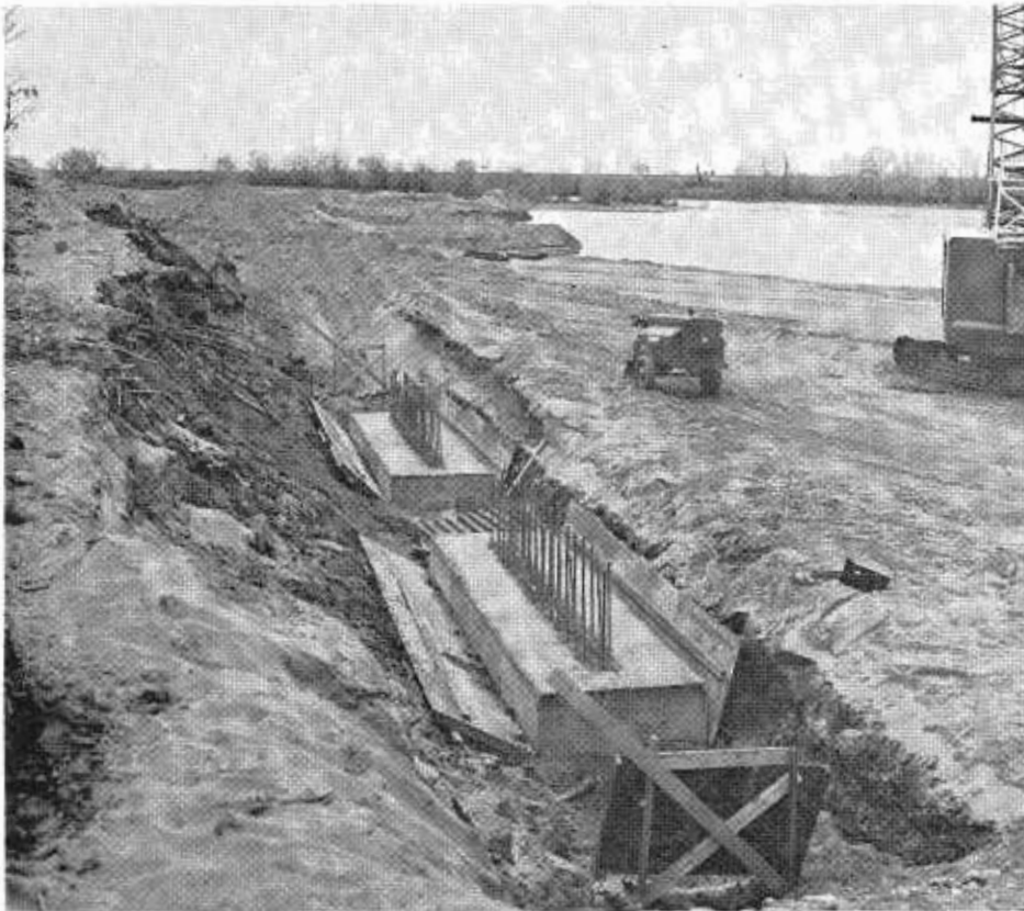
One set of footings for parallel pier columns on the bridge shown just after stripping the forms.
