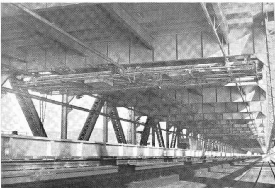
The gantries or upper deck travelers run on a three-rail overhead track with air-powered drive. The working platform is 17 feet wide and 59 feet long.
