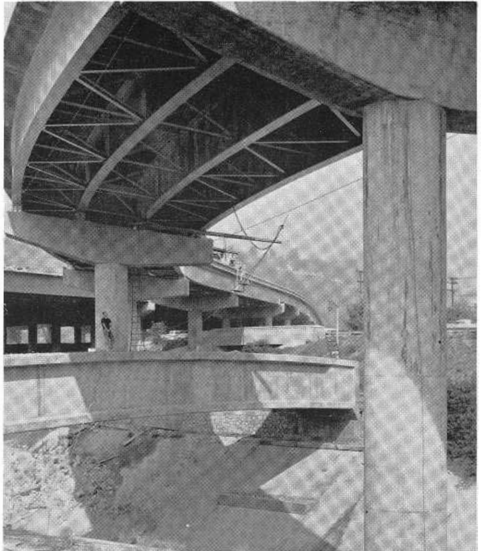
This photograph shows the curved steel girders supported by the prestressed carrying girder over the Arroyo Seco Channel.
