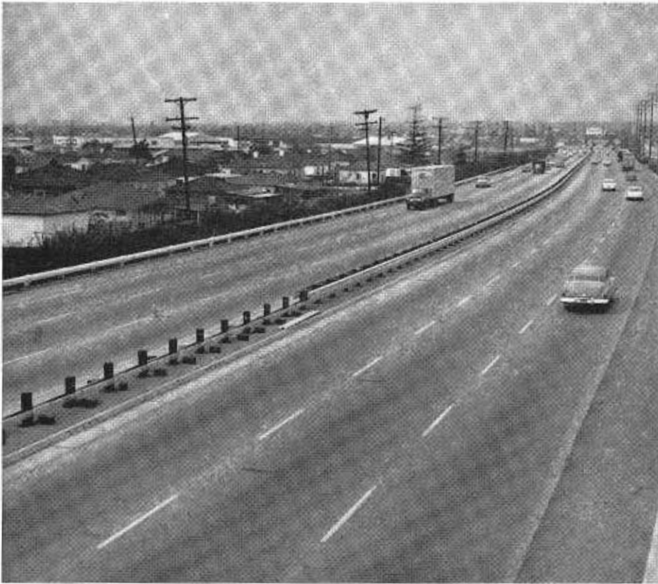
This photo shows a section of the beam barrier as it was being installed on the Santa Ana Freeway last February. Note the portion of partly completed barrier at the lower left.
