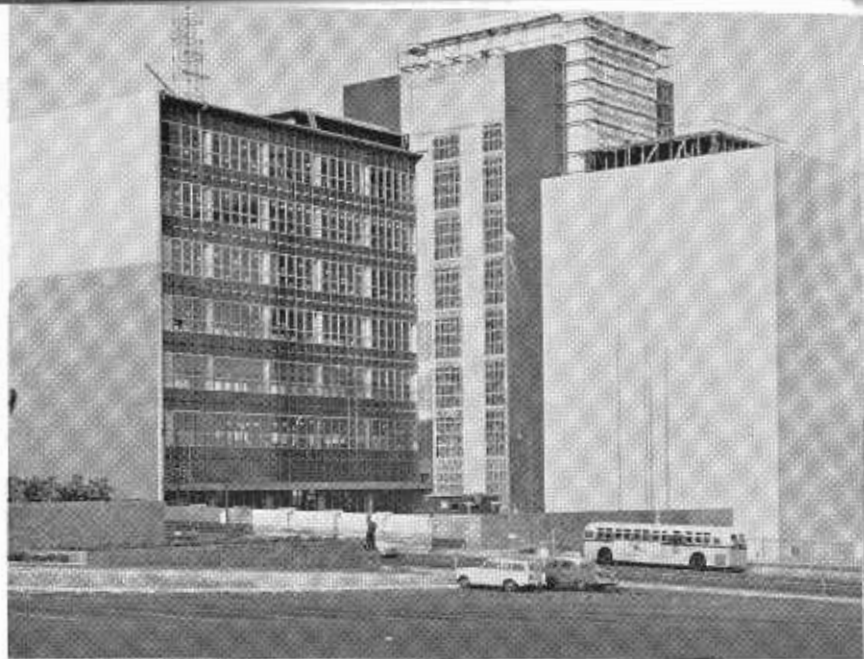
The Los Angeles County Hall of Records under construction in Civic Center.
