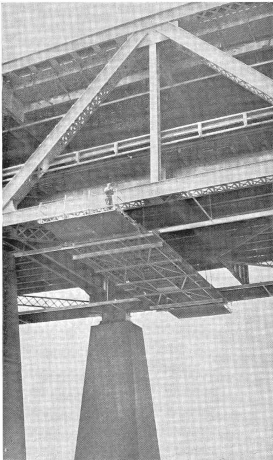
Lower deck travelers used on the East Bay section provide a 19-by-73-foot platform for painting the lower deck floor system. They are hung from air motor-driven trolleys. Folding ends allow clearance when passing through the bridge piers. These are replacing the older Magic Carpets (see photo previous page).
