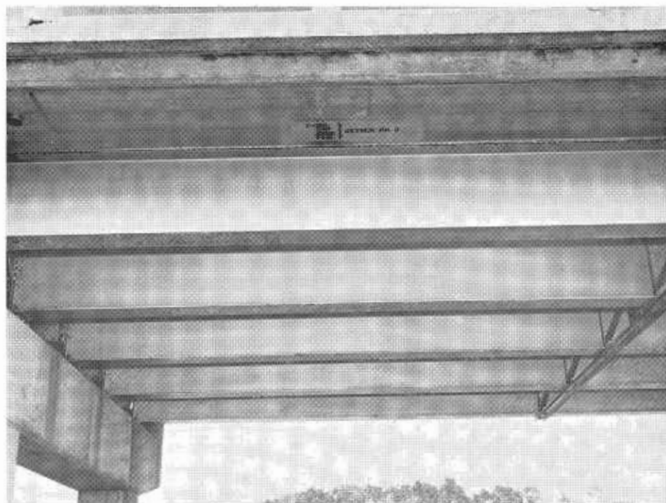
FIGURE 4—Under view of the north portion of Span 2 on which Painting System No. 2 was used.
