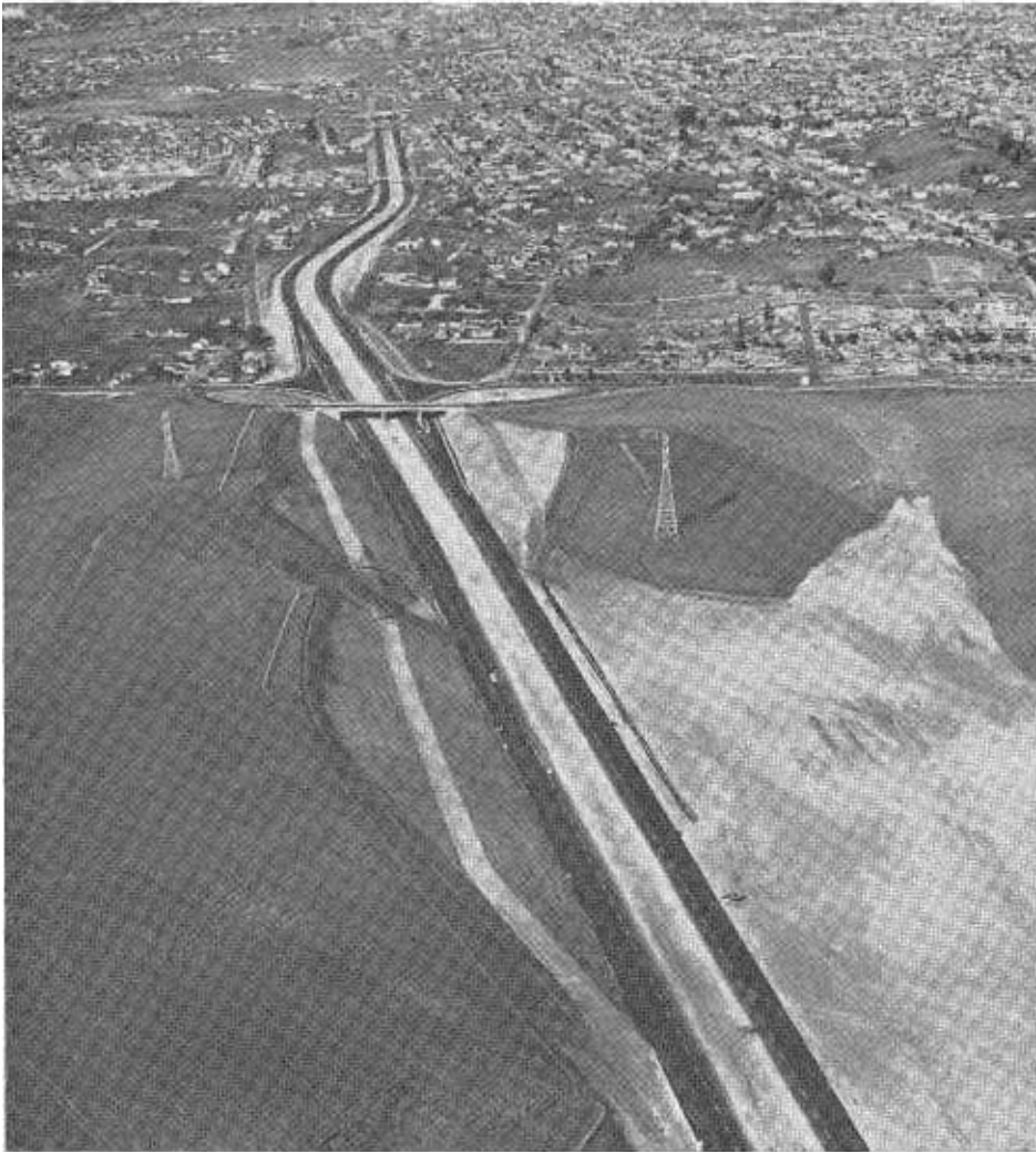
Looking westward from the middle of the project showing the deep sidehill cut in the left foreground and the waste area on the right. The near interchange is Glen Cove Road.
