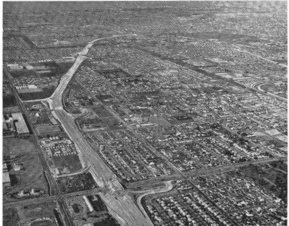
San Diego Freeway construction at Vermont Avenue (bottom). 190th Street parallels the freeway at the left.
