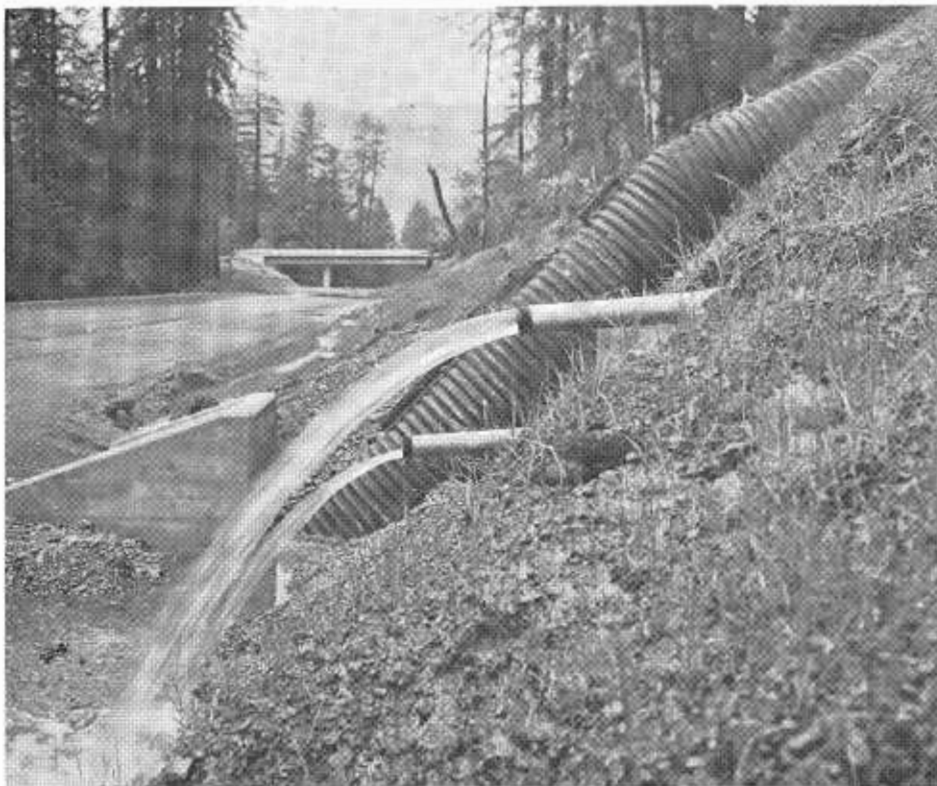
This photo gives some idea of the amount of subsurface water that must be contended with in areas of heavy rainfall such as this section of US 101. Here horizontal drains in a potential slide area carry off water to relieve hydrostatic pressure and lubrication of the earth mass.
