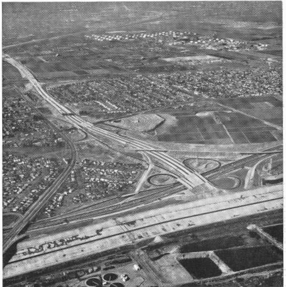
San Diego Freeway construction in the vicinity of the Long Beach Freeway (foreground). The Los Angeles River is at the bottom.
