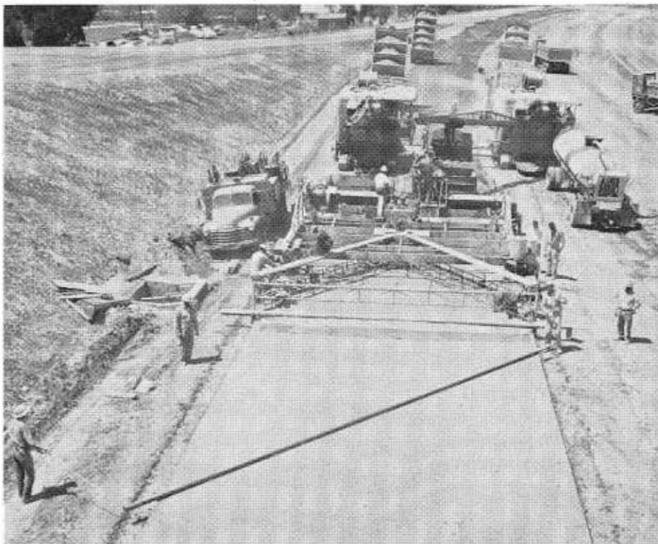
A new slip-form paver used on the job lays a two-lane width of concrete pavement.
