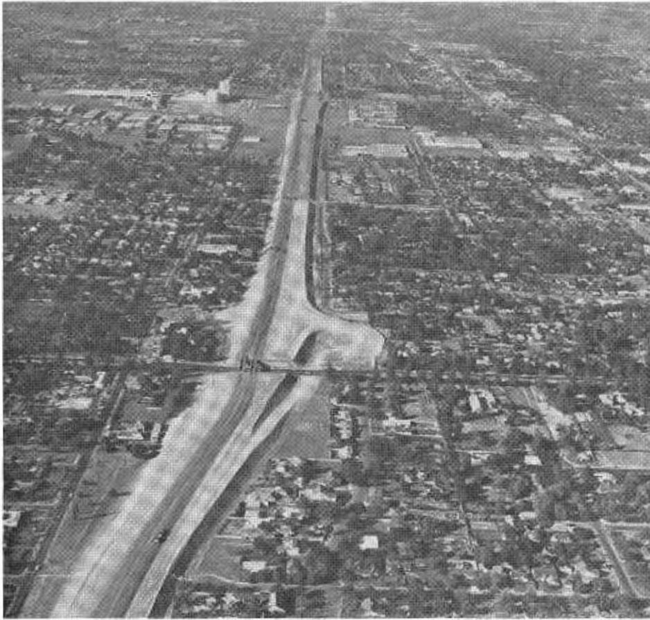
Embankment construction on the San Diego Freeway in the San Fernando Valley. The view is northward from Hart Street with the Sherman Way interchange at the center.
