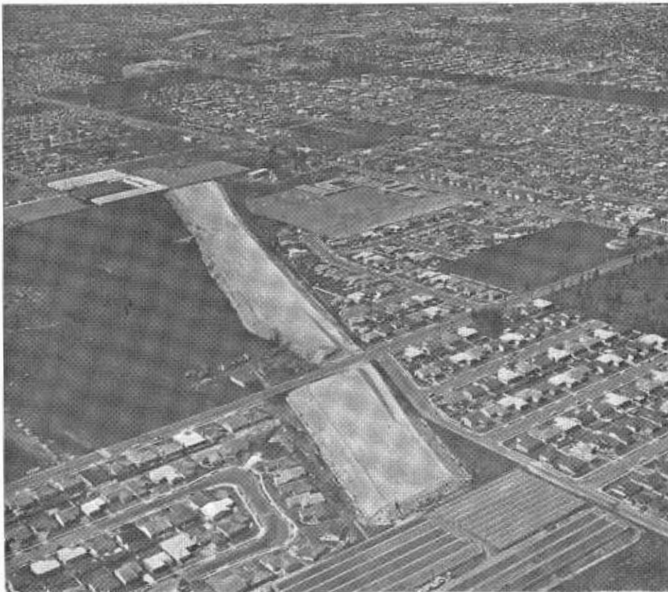
Freeway fill stockpiled within the right-of-way before actual construction of the San Diego Freeway at Arlington Avenue.
