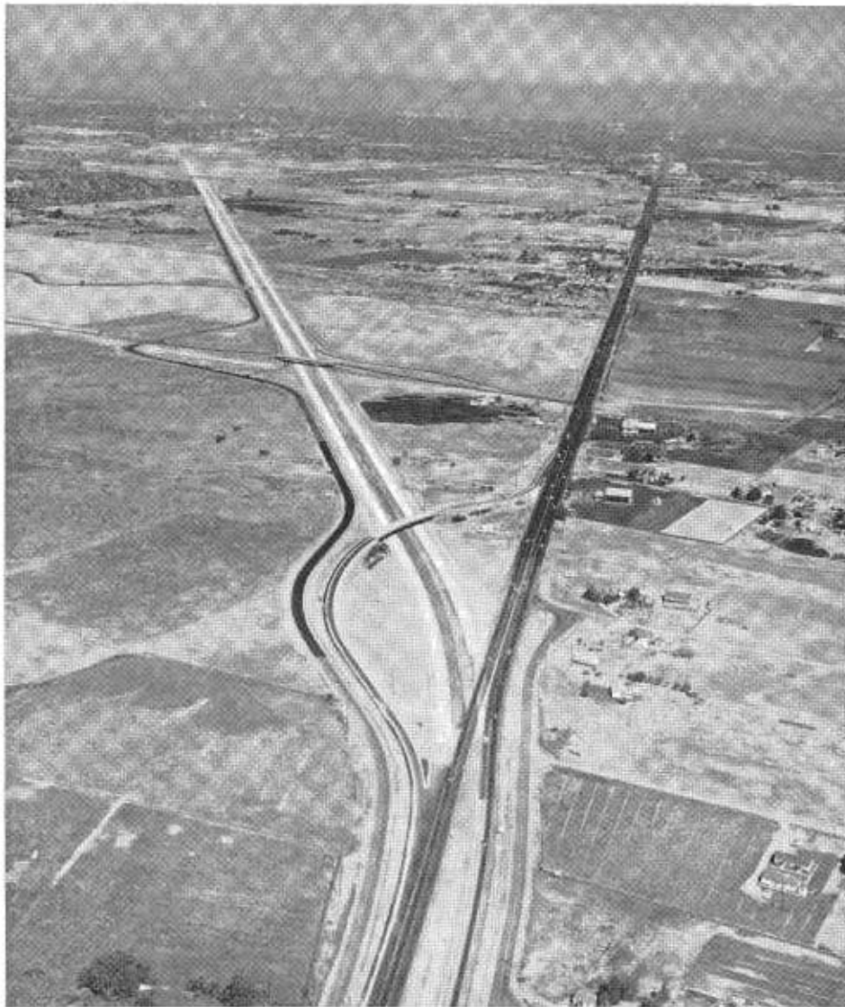
The South Sacramento Freeway during construction showing the connection with Stockton Boulevard (old US 50-99) in the foreground. The view is northward.
