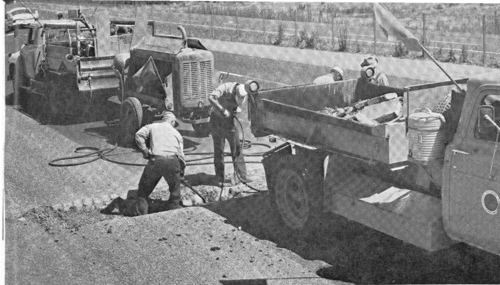
Maintenance crew repairing section of Bayshore Freeway in vicinity of San Mateo. A few decades ago this would have been pick and shovel job for a dozen men and several horses. Mobile aircompressor simplifies task so it can be quickly done by a few men.
