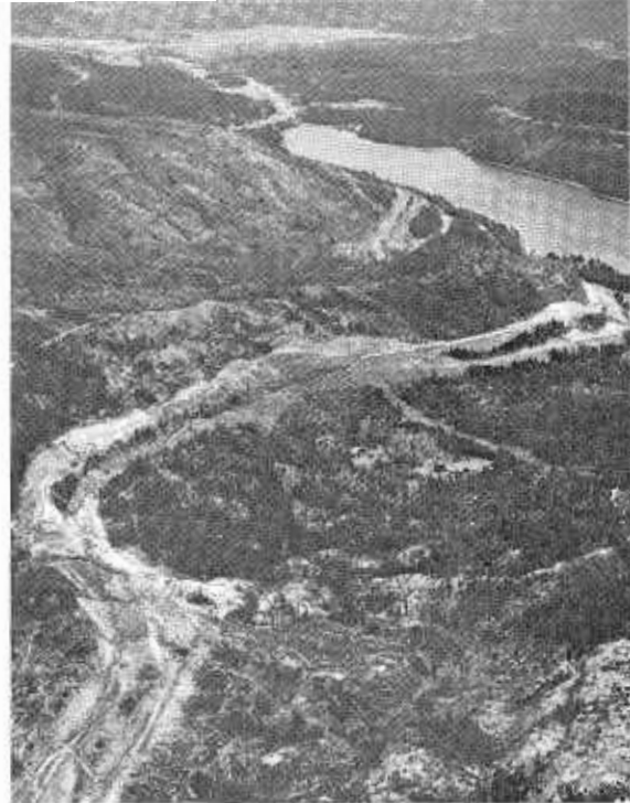
Aerial view in reverse to one on opposite page shows new alignment swinging north and climbing ridge, while old alignment, just visible middle right continues over summit.
