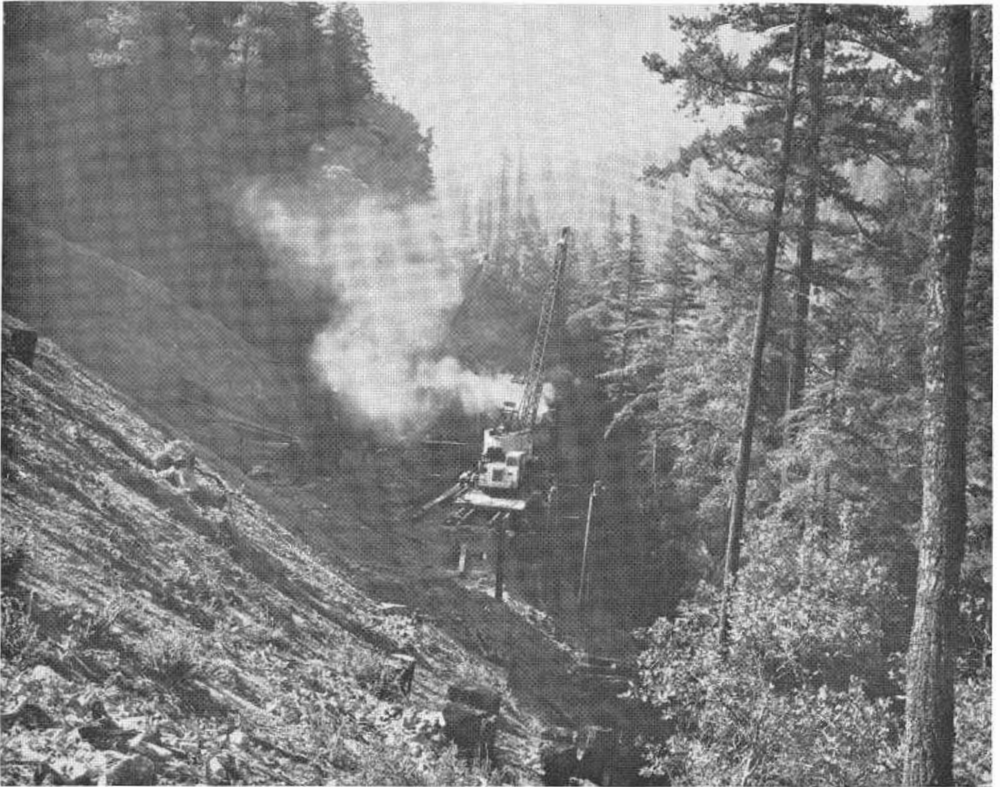
Construction begins on the Eagle Point Viaduct section of the Redwood Parks Freeway south of Myers Flat.
