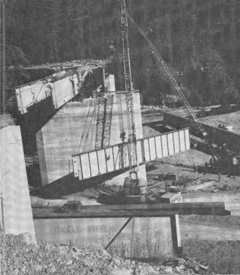
A girder is hoisted into position on the new bridge being constructed across the South Fork of the Eel River.
