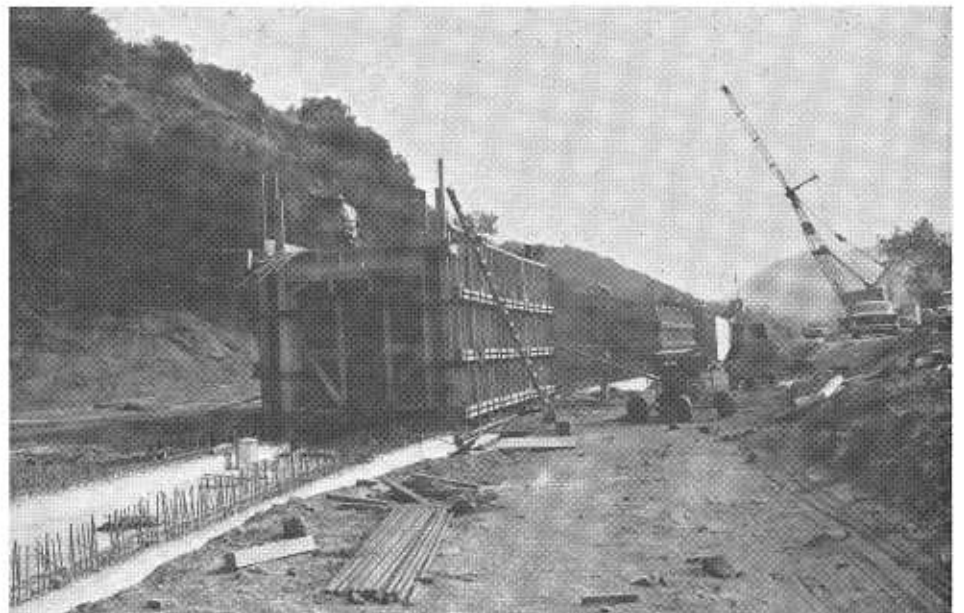
Construction of a huge drainage facility south of Mulholland Drive. The reinforced concrete box passes under the freeway.
