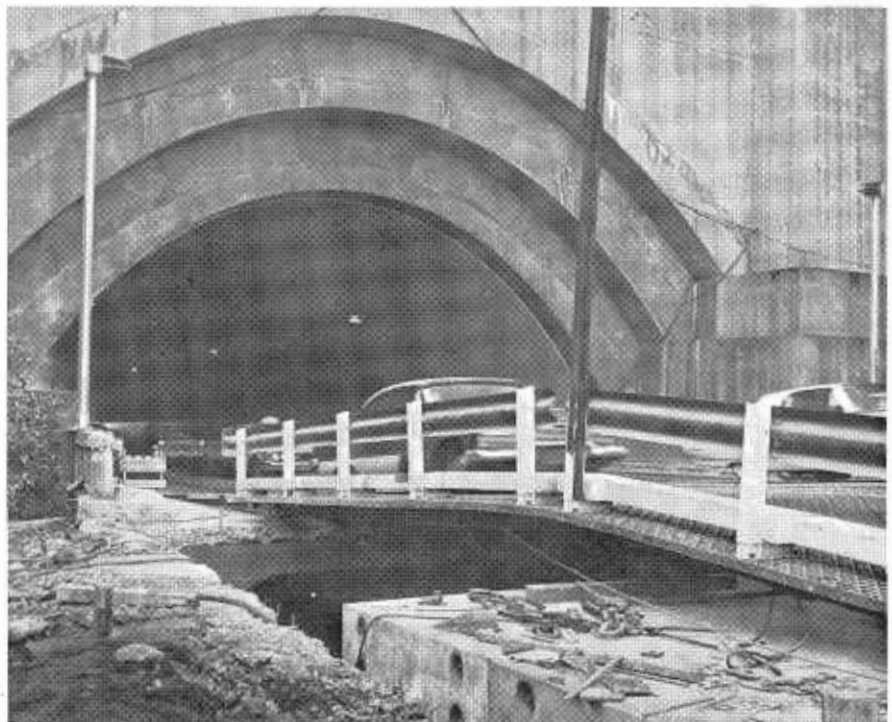
Photograph of movable bridge from viewpoint on same side of bridge as cutaway section of tunnel reconstruction. Outer ends of new deck units are seen in right foreground. The prefabricated, prestressed units fit neatly together, and no additional decking is necessary.
