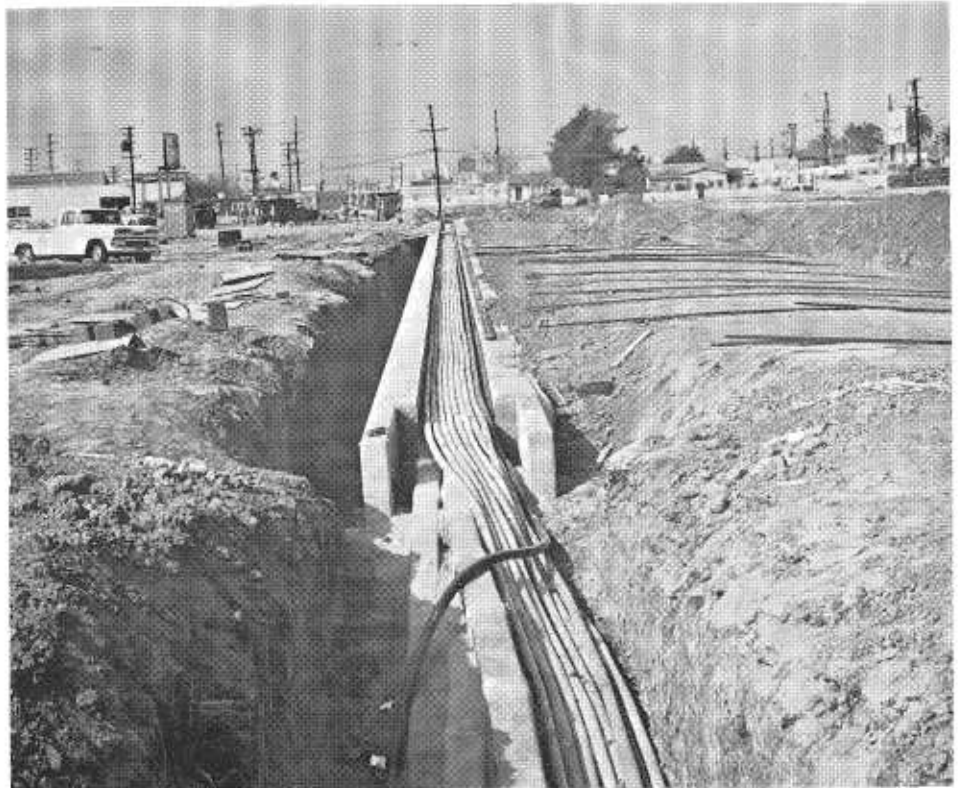
Telephone cables relocated in the new utility overcrossing bridge.
