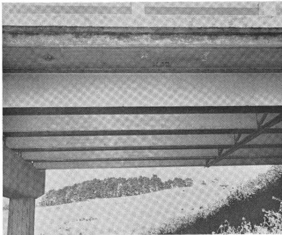
FIGURE 6—Under view of the north portion of Span 1. Painting System No. 4 was used except on the stringer in the foreground on which System No. 5 was used.
