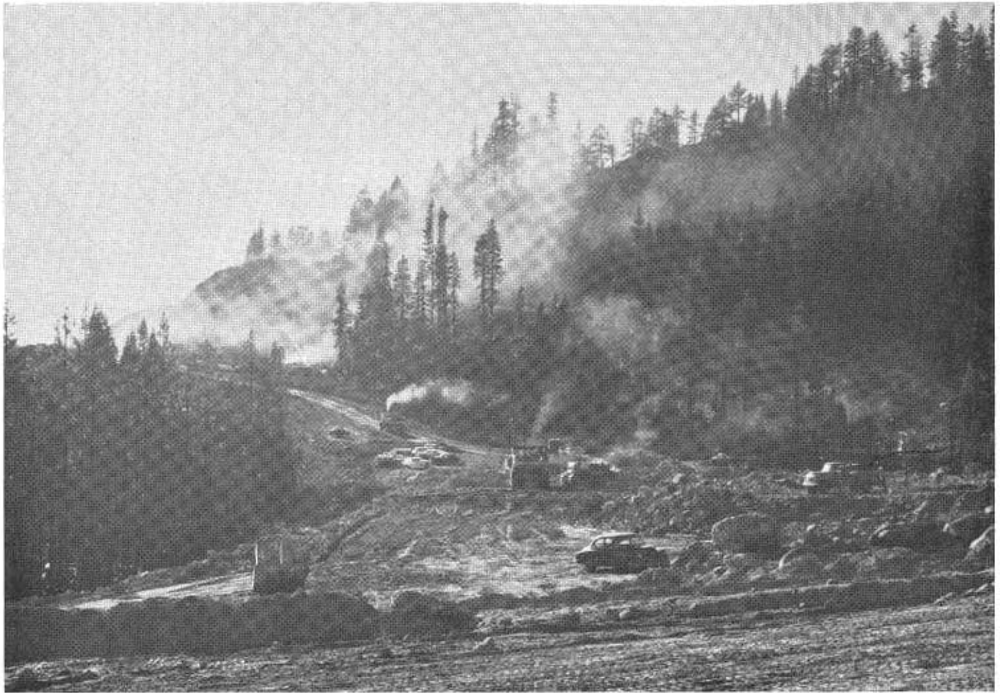
Scene during construction, Donner Lake Undercrossing, US 40 and Interstate 80, on a new alignment north of Donner Lake.
