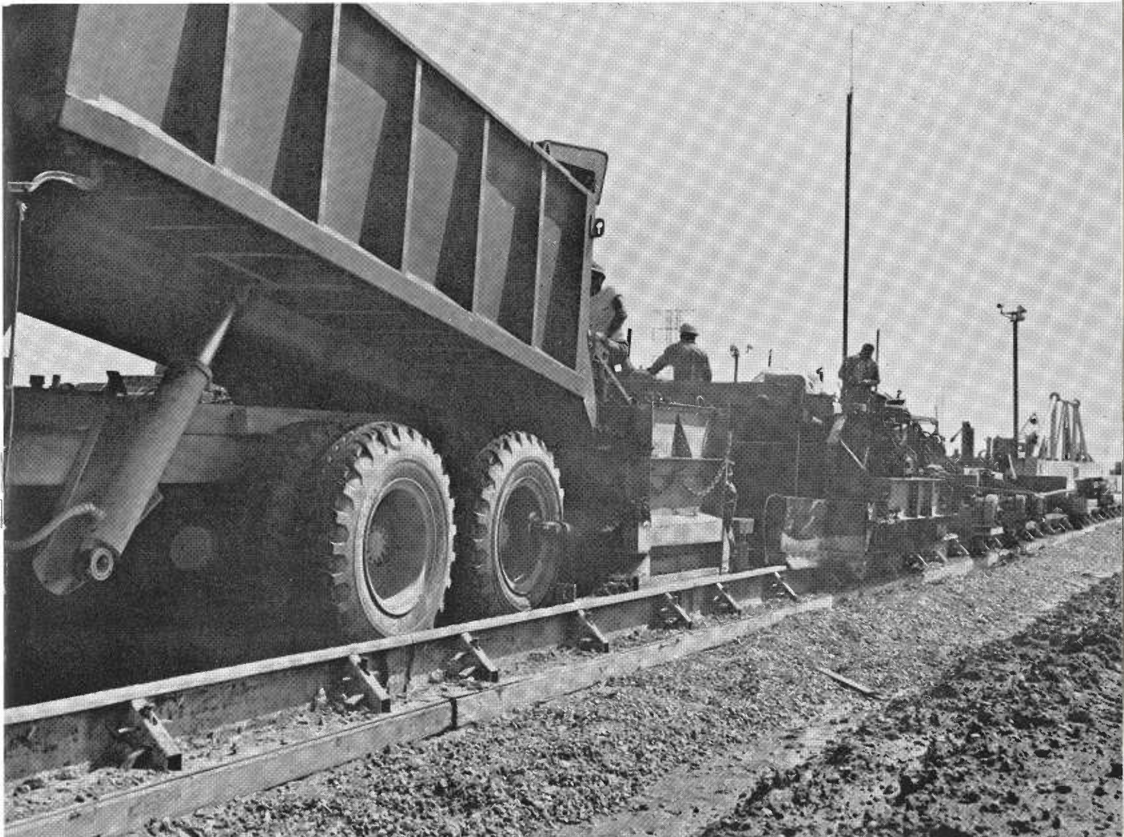
PHOTO BELOW—The paving train in operation. In the foreground the hauling unit dumps into the spreader box. It is followed by the spreader and finishing equipment.
