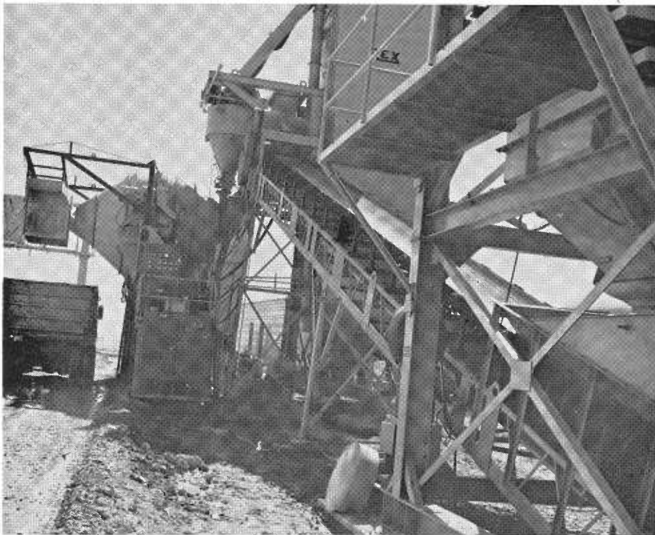
A closeup of the chain belt showing the proportional aggregate conveyor (foreground) and the operator's platform and control panel with main mixing drum (left).
