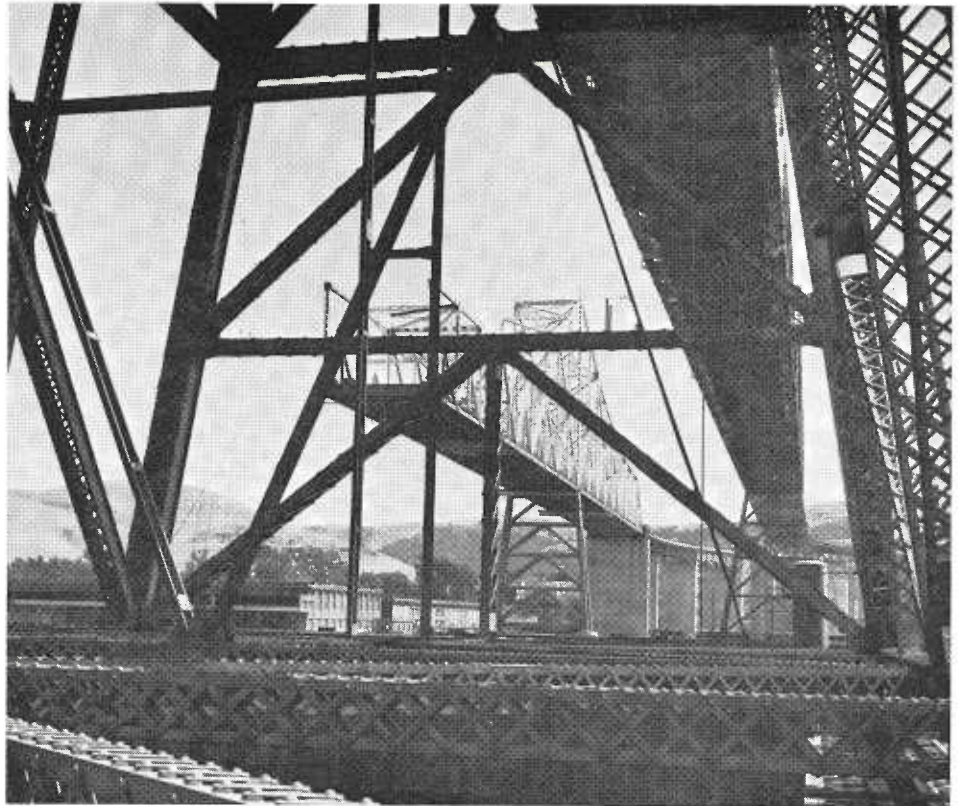
An idea of the extensive riveting involved in creating the "lacework" on the older Carquinez Bridge is given in this photo taken during the construction of the new span (in background). The use of welded perforated box girders has virtually eliminated the use of riveting on such structures.
