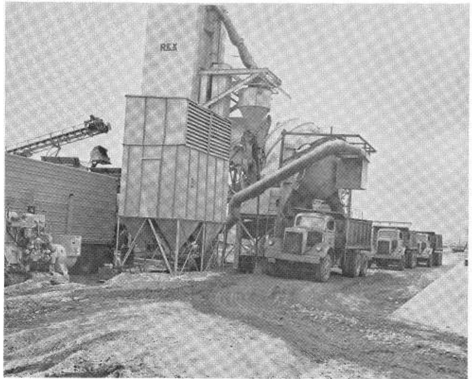
The chain belt at the central mix concrete plant is shown discharging into a nonagitated hauling unit.
