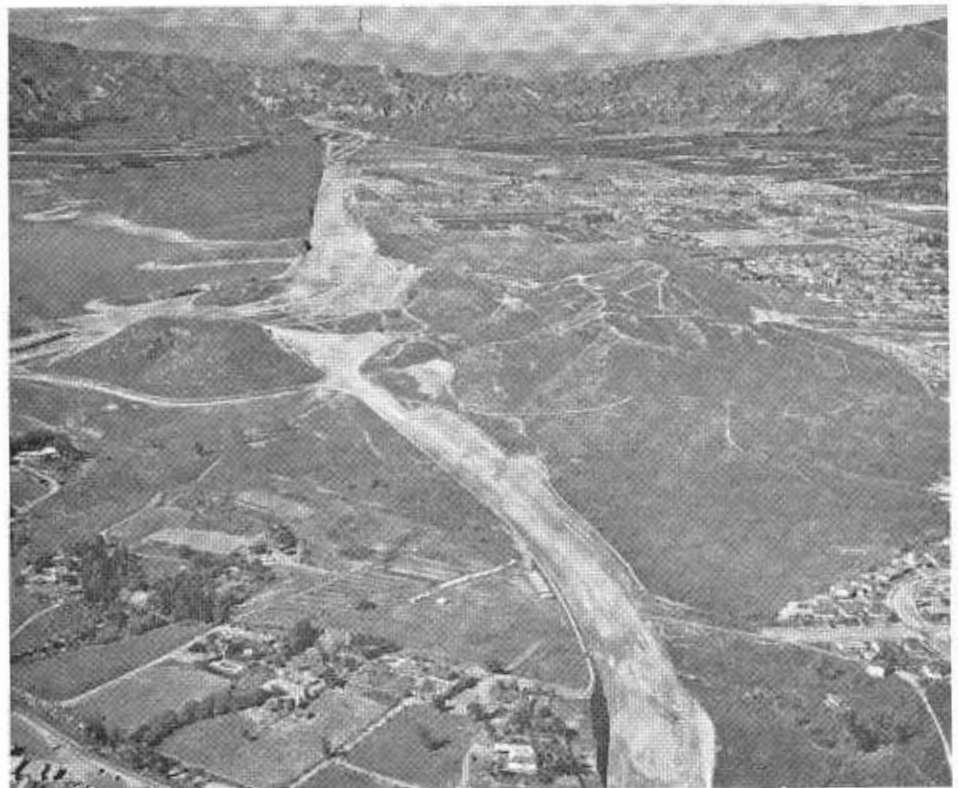
Looking north along construction on the San Diego Freeway at the San Fernando Reservoir (left). This will be the future location of the San Diego-Golden State Freeway Interchange.
