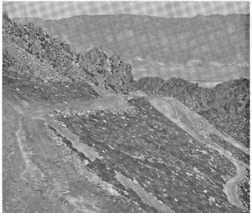
Looking eastward over rough grading operations on the Onion Valley Road project toward Owens Valley in the distance beyond Independence, County Seat of Inyo County.
