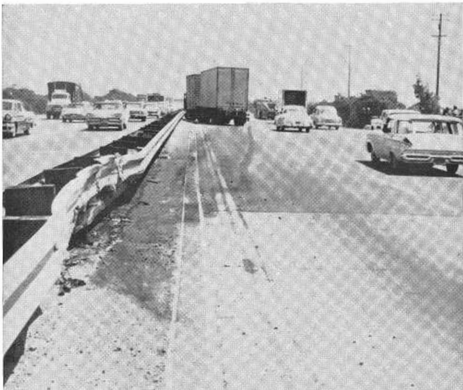
Accident damage to blocked-out metal beam barrier on the Nimitz Freeway. Results correlate well with the experimental full scale crash tests of 1959.
