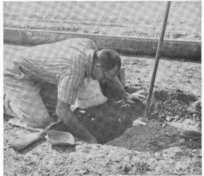
A hole cut in the completed lower portion of the structural section prior to placing the P.C.C. surfacing layer. The hole exposes the planes between each structural layer from which the layer thicknesses are measured.
