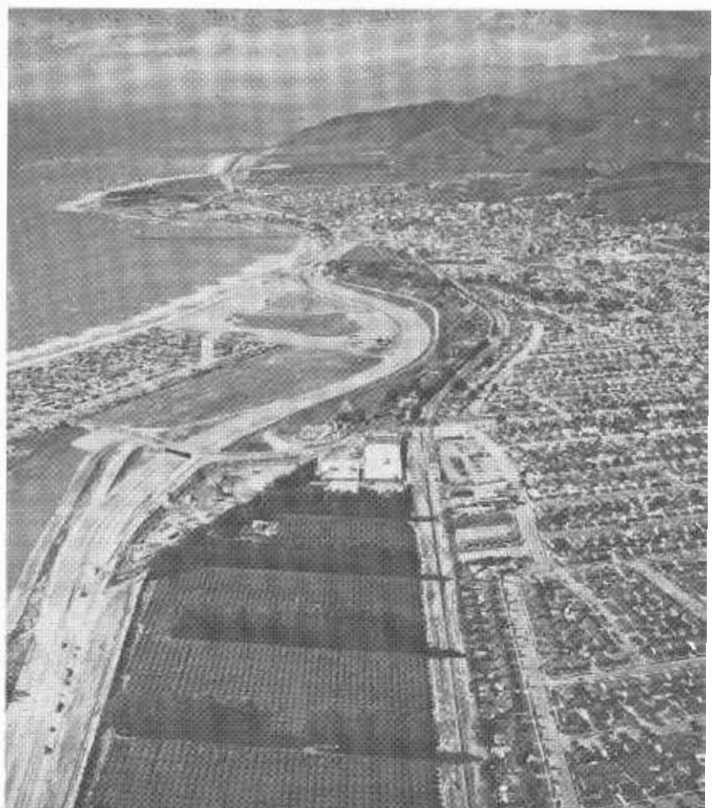
Construction on the Ventura Freeway in the City of Ventura. The view is westward.
