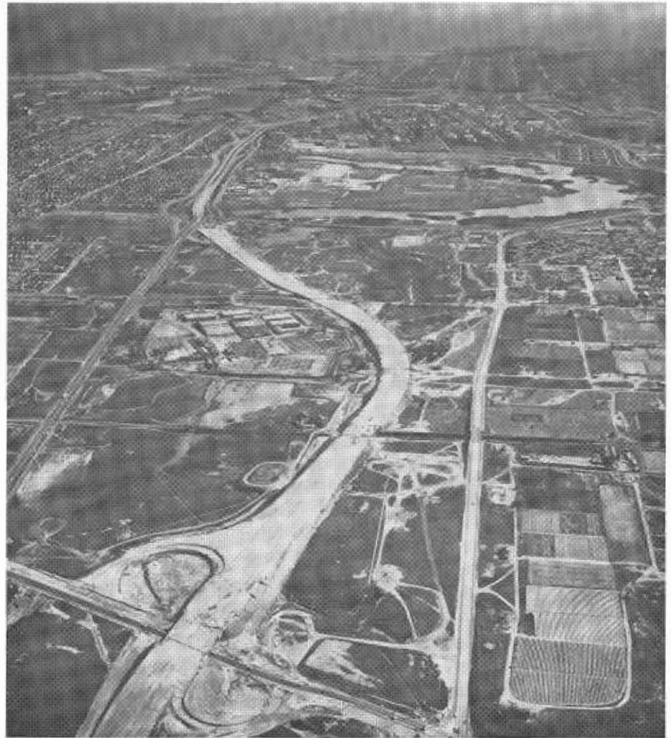
Looking south at construction on the Harbor Freeway toward the Pacific Coast Highway. The diagonal road to the left is Sepulveda Boulevard.
