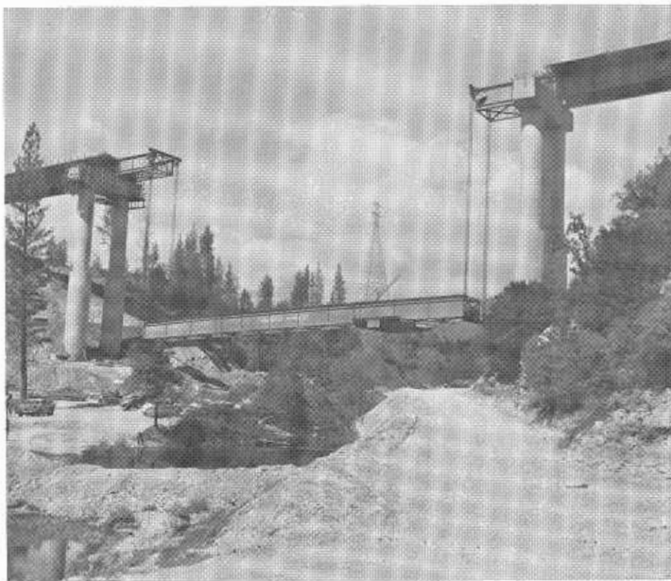
Two 14,000-pound lead line pull engines secured to the bridge approach start to lift the 260-foot center span into place on the new Whiskey Creek Bridge.
