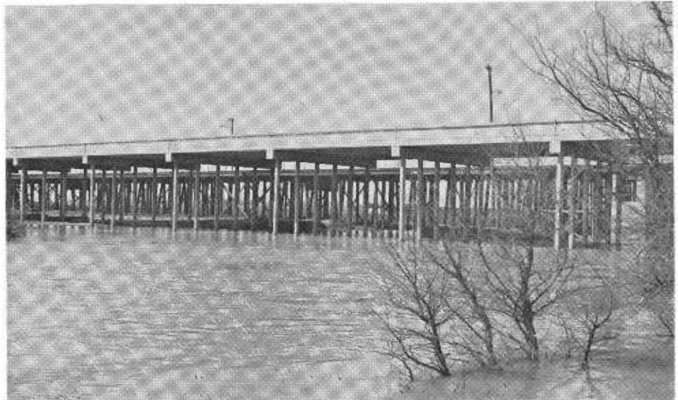
The new eastbound Yolo Causeway structure at its east end. The old causeway is in the background.
