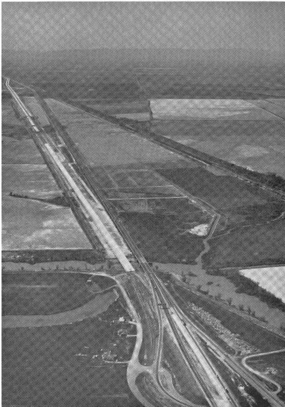
Looking west over the Yolo Causeway project. The 4,700-foot-long fill and pavement is completed. The two 2,800-foot-long structures at the west end are nearly complete. The eastbound lanes of the two 8,800-foot-long structures (broken white line left center) will be completed late this summer and traffic will be detoured over it while the westbound structure is being completed.
