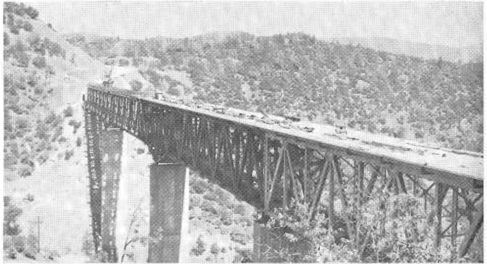
An eastward view of highway deck construction operations. The crane at the far end is filling in secondary structural members.
