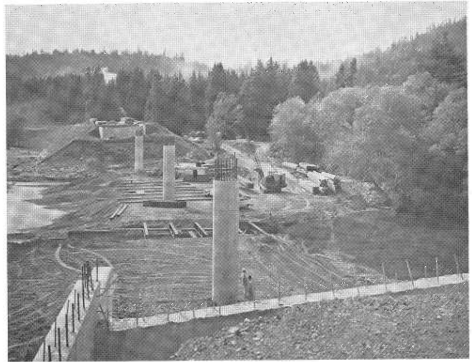
Substructure construction of a cast-in-place, reinforced concrete, box girder bridge over Austin Creek in Sonoma County on the alignment of Sign Route 12 between Austin Creek and Duncan Mills.
