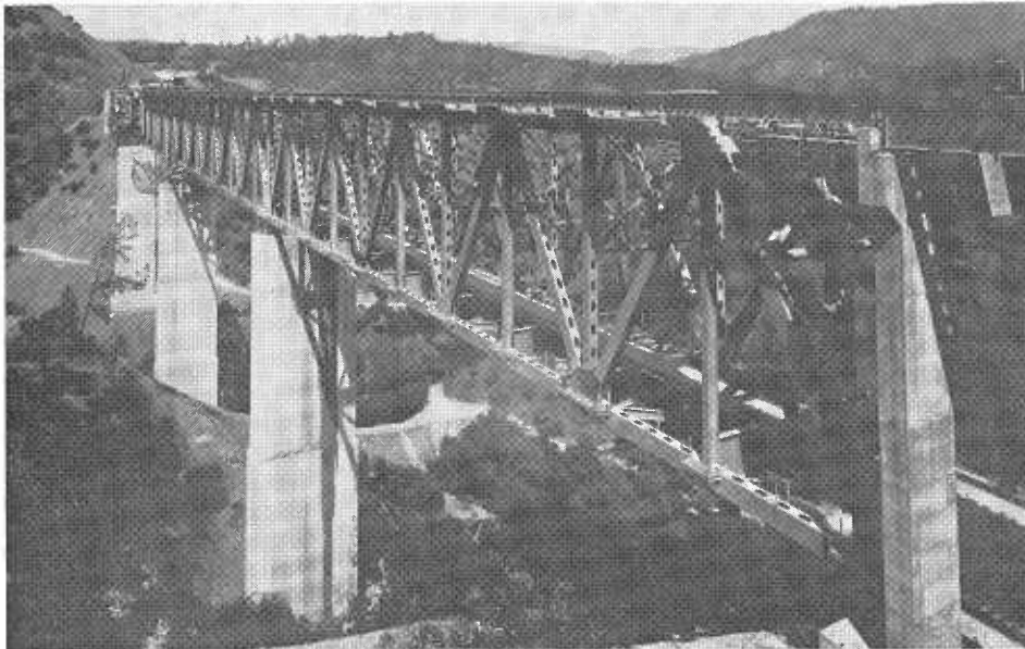
View of the bridge during structural steel erection. The traveller is on the far end. A truck crane over Pier 9 is placing highway deck stringers and secondary truss steel.
