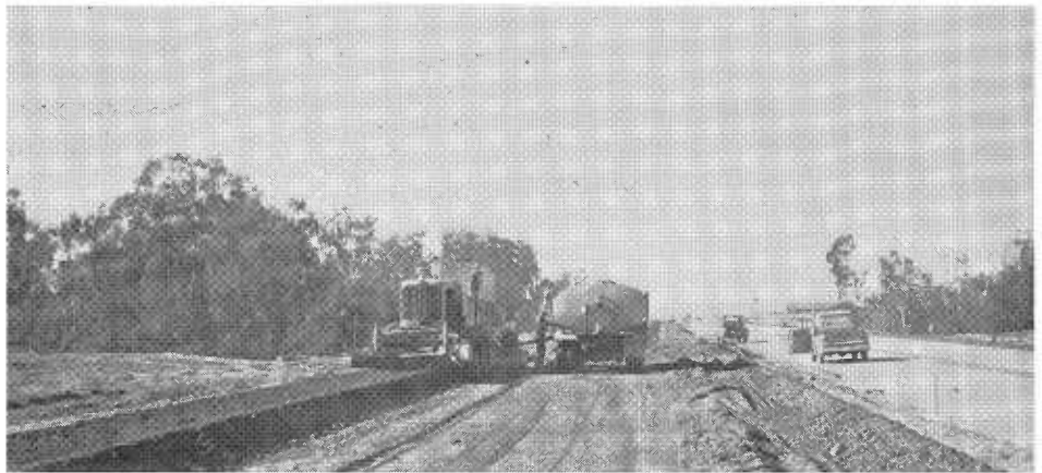
The freeway under construction. A mixer prepares cement-treated base as described in the article.
