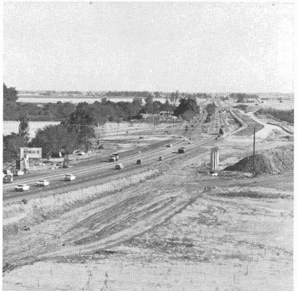
Throughout the State, expressways are being converted to full freeway standards as traffic conditions warrant and funds become available. In the photo above, a section of U.S. 40 (Interstate 80) near Vacaville is being widened and cross traffic at grade eliminated by the construction of overpasses.
