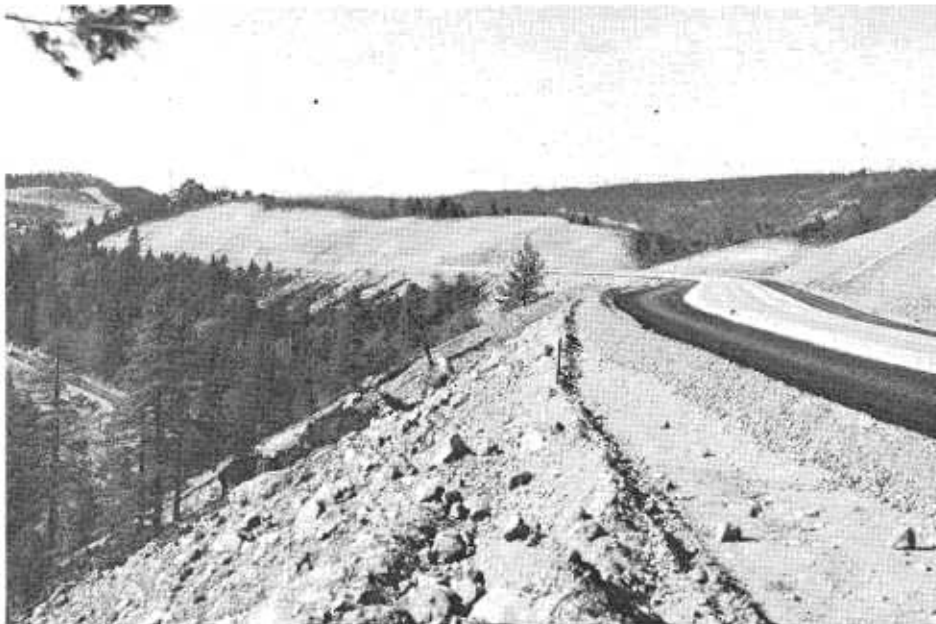
The entire length of U.S. 40 (Interstate 80) between Sacramento and the Nevada line will be raised to multilane freeway and expressway standards by 1964. At left, westbound lanes near Emigrant Gap are nearing completion. The existing highway (lower level at left) will be reconstructed and widened on the same general alignment at this point to serve as the eastbound lanes.
