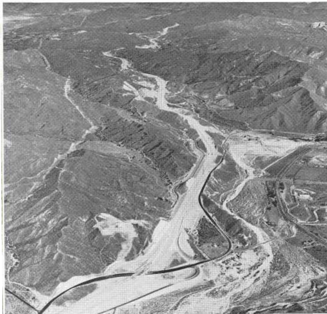
BELOW —Sixteen miles of the Antelope Valley Freeway (U.S. 6), which will run from the Golden State Freeway to the Kern County line north of Lancaster, are under construction and another eight miles are financed in the new budget.
