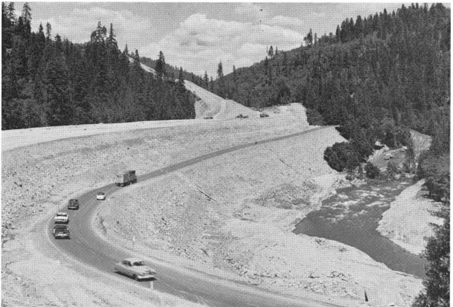
The narrow, inadequate two-lane highway on the lower level was U.S. 99 (Interstate 5) south of Castella in Shasta County. Construction has just been completed on the section to its left, which provides 30 miles of continuous freeway and expressway in the Sacramento River Canyon. Freeway construction is under way on this route north of Red Bluff and along the shore of Shasta Lake, and is budgeted for construction near Redding and Mount Shasta City.
