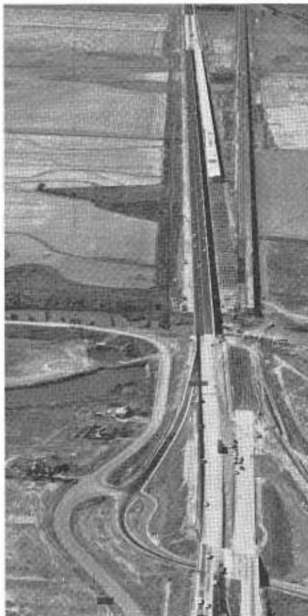
This view looking westward shows construction on the westbound lanes of the Yolo Causeway on U.S. 40 (Interstate 80) which has replaced the three-mile structure on the right, once the longest highway trestle in the world. The eastbound lanes will carry two-way traffic until construction is completed in 1963.
