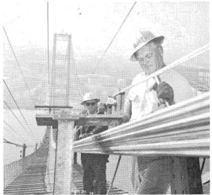
Work continues on the superstructure of the Vincent Thomas Bridge between San Pedro and Terminal Island. The bridge will be opened to traffic early in 1964.
