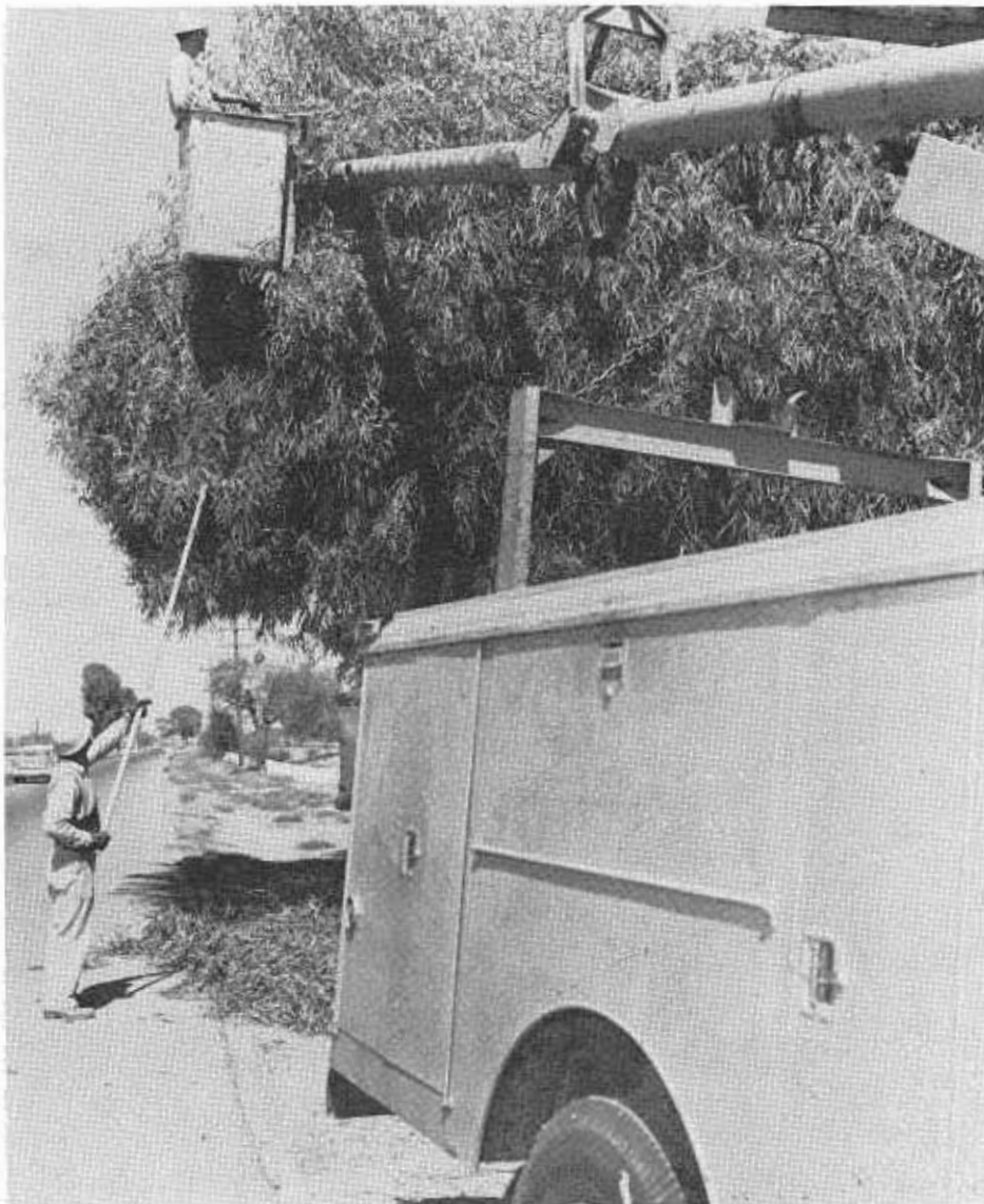
A maintenance crew trim overhanging foliage from a tree along a state highway, one of the many routine maintenance chores that must be performed regularly.
