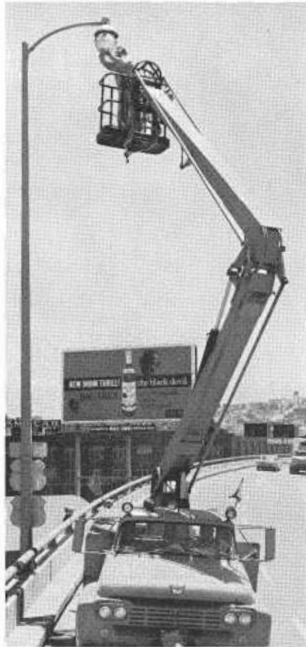
A maintenance worker repairs a lamp on a freeway from one of the division's rotary brush sweeper and giraffe units.
