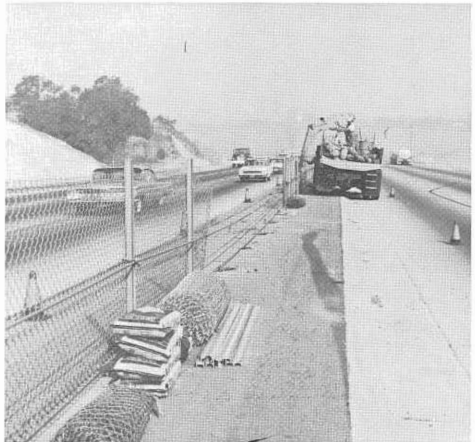
A maintenance crew repairs a section of median barrier fence on the San Bernardino Freeway.
