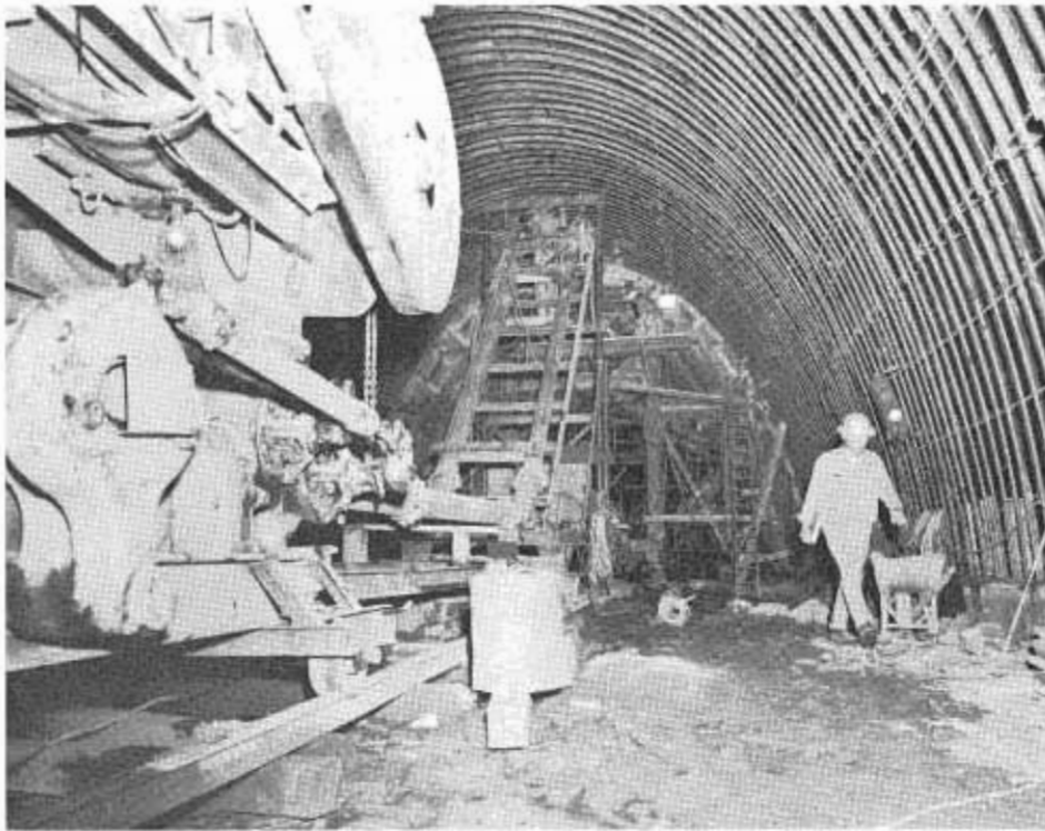
Construction inside the Collier Tunnel through the Hazelview Summit on U.S. 101 in Del Norte County.
