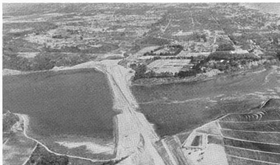
Surcharge fill is being placed across coastal lagoons north of San Diego for the future relocation of U.S. 101 (Interstate 5). This view is southward across Batiquitos Lagoon, toward Leucadia and Encinitas.
