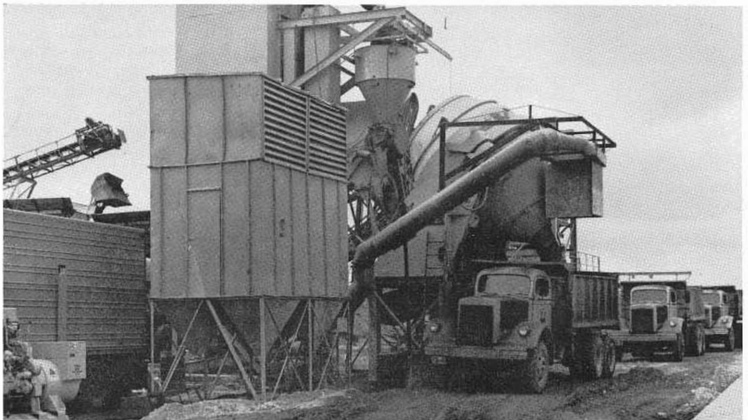
The central mix method of getting concrete to a paving job was used successfully on a section of the San Diego Freeway in the Carson Street-Dominguez area of Los Angeles.
