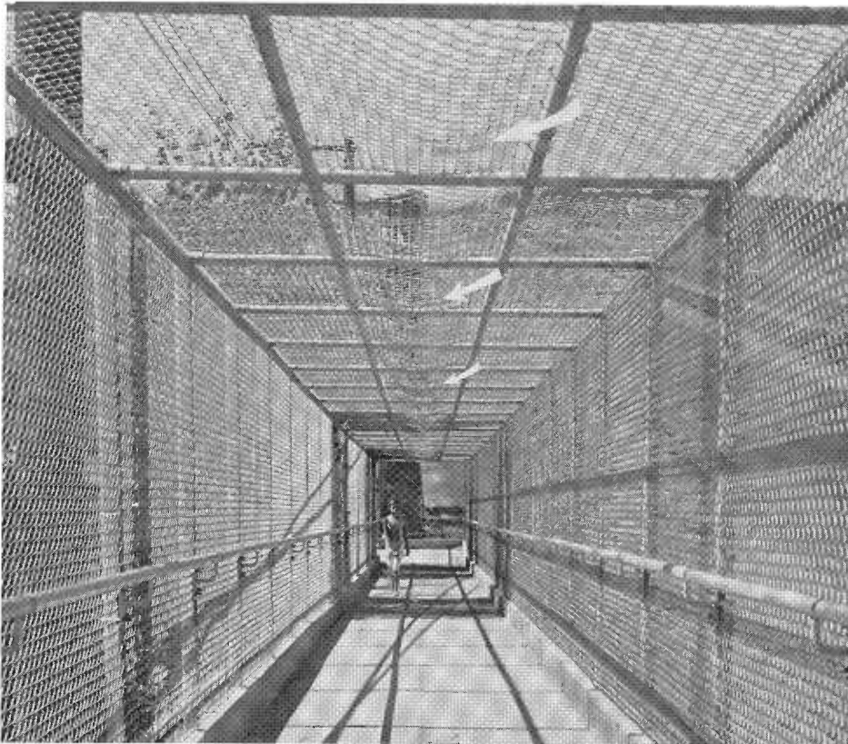
A close-up of the pedestrian overcrossing shown in the above photo. Note how the roof of the enclosure has been beaten down by children climbing on top and bouncing on it as on a trampoline. The next step is to round the top.
