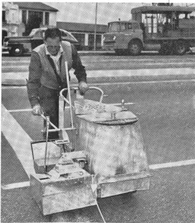
The stripe applicator in operation. Note the base truck parked in the background out of the way of traffic.
