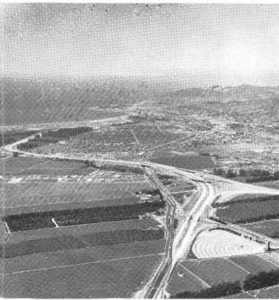
BACK COVER—Looking west along construction on the Ventura Freeway from above Telephone Road in the City of Ventura. Sign Route 126 joins the new freeway at the bend (right center). See "Ventura County Freeways" beginning on page 36. Photo by Robert Rose.
