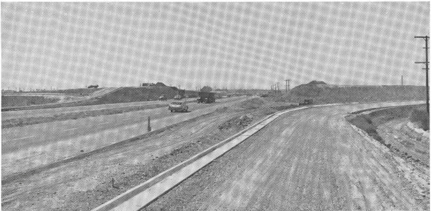
Calleguas Creek Overcrossing under construction on Pacific Coast Highway in the vicinity of Point Mugu.
