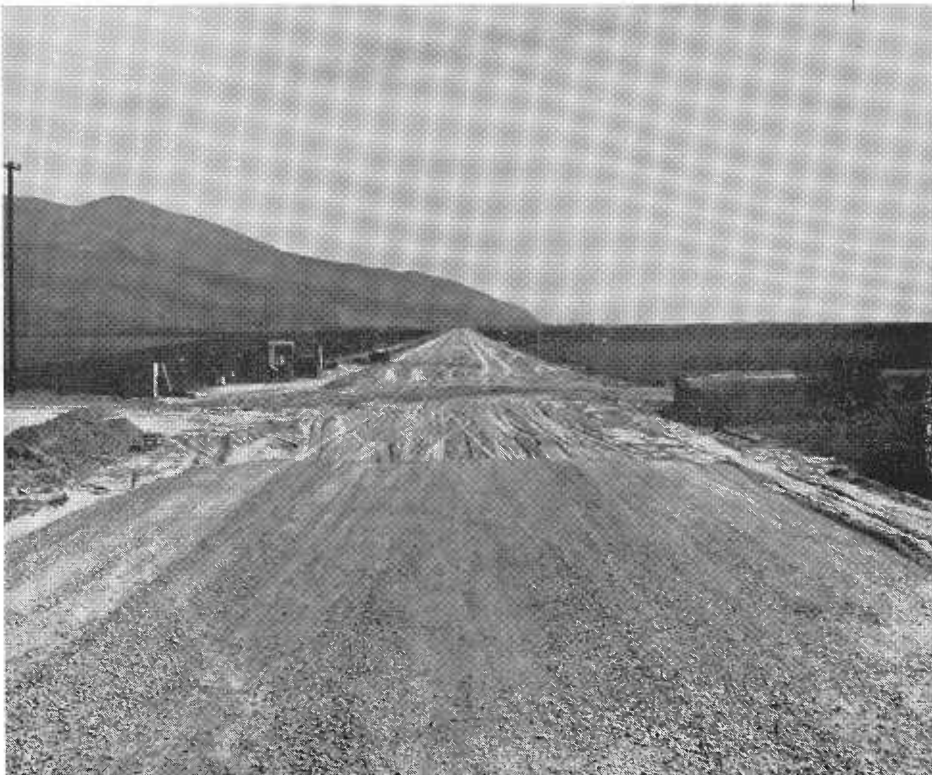
Looking south along the Las Posas Federal-Aid Secondary Road project. At left is Laguna Peak near Point Mugu.
