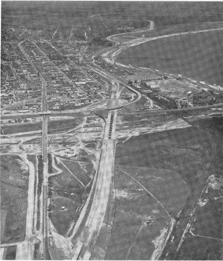
Ventura Freeway construction through the City of Ventura. The view is eastward. The Ventura River and bridge is center and, just beyond, the Ojai-Ventura Freeway Interchange.
