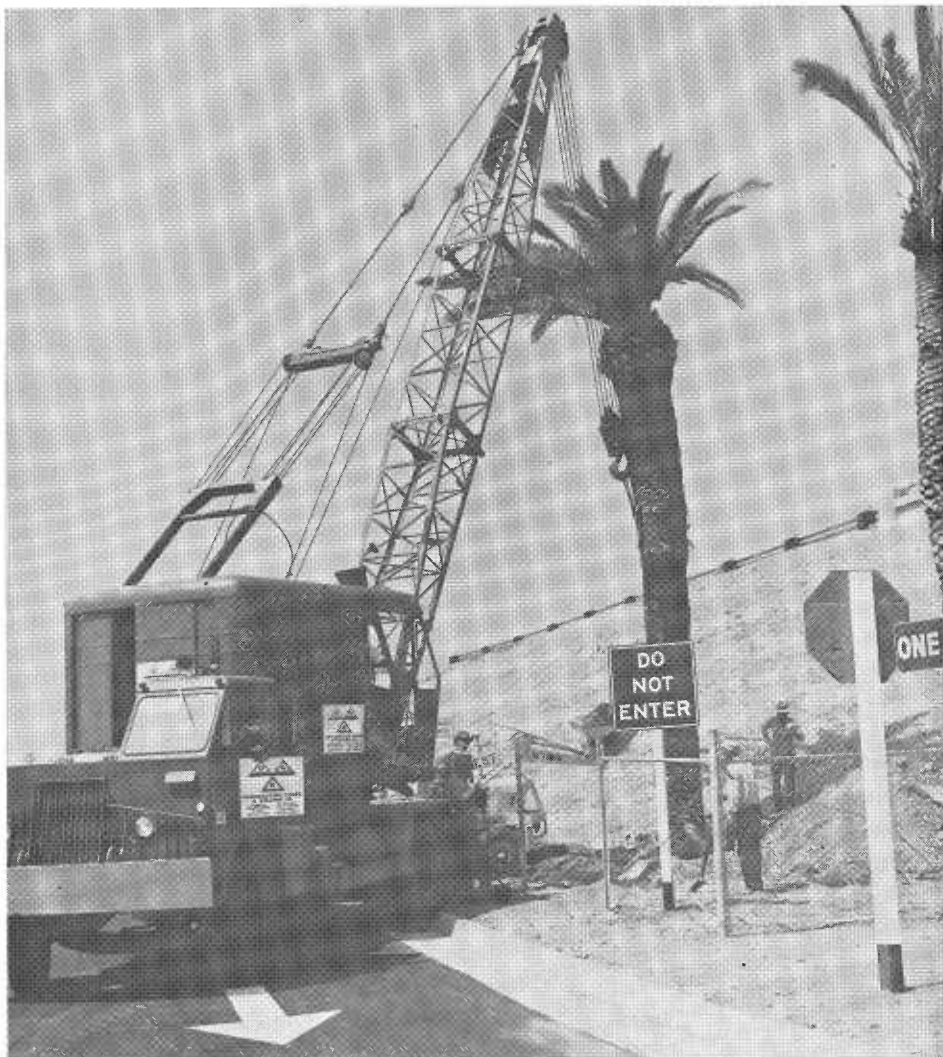
LANDSCAPING—Planting palm trees at the University Street overcrossing along the new freeway.
