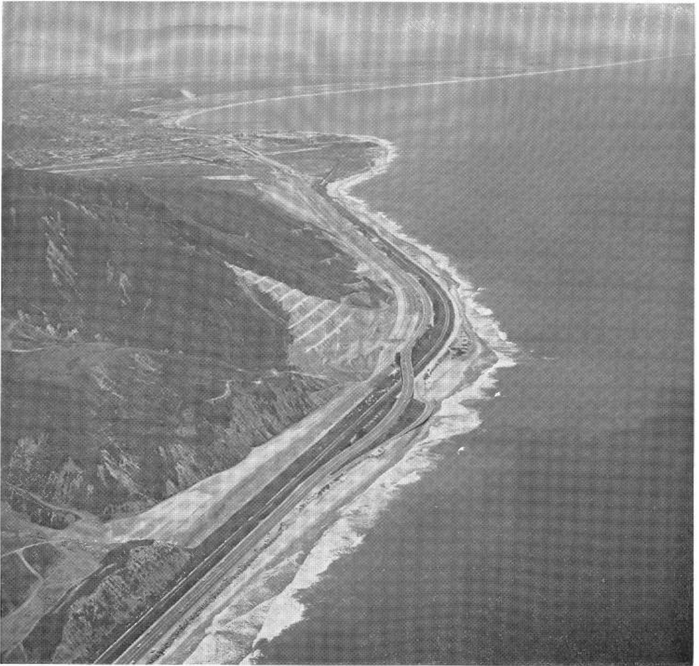
Ventura Freeway construction, looking eastward from the west end of the job. Note the benched slope to the left of the highway.
