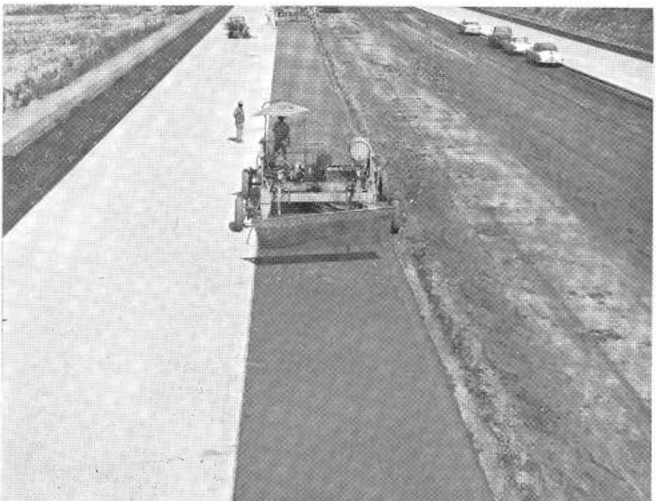
The pipe float finishing machine reduced in width for a 12-foot slab.
