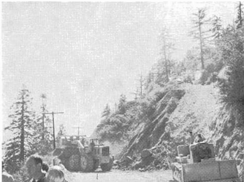
Construction equipment widens the two-lane ledge section of the Big Bear Highway.
