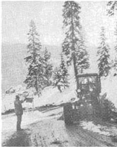
Traffic over detour temporarily halted while grader widens road on one of switchbacks on detour.
