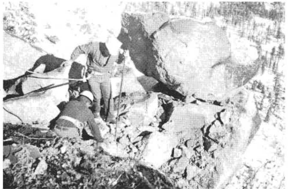
Men working on rim of cliff—note safety lines. Drop here is about 75 feet to highway, nearly a thousand feet more to valley floor. Car parked on closed U.S. 50 may be seen beyond right elbow of upper figure.
