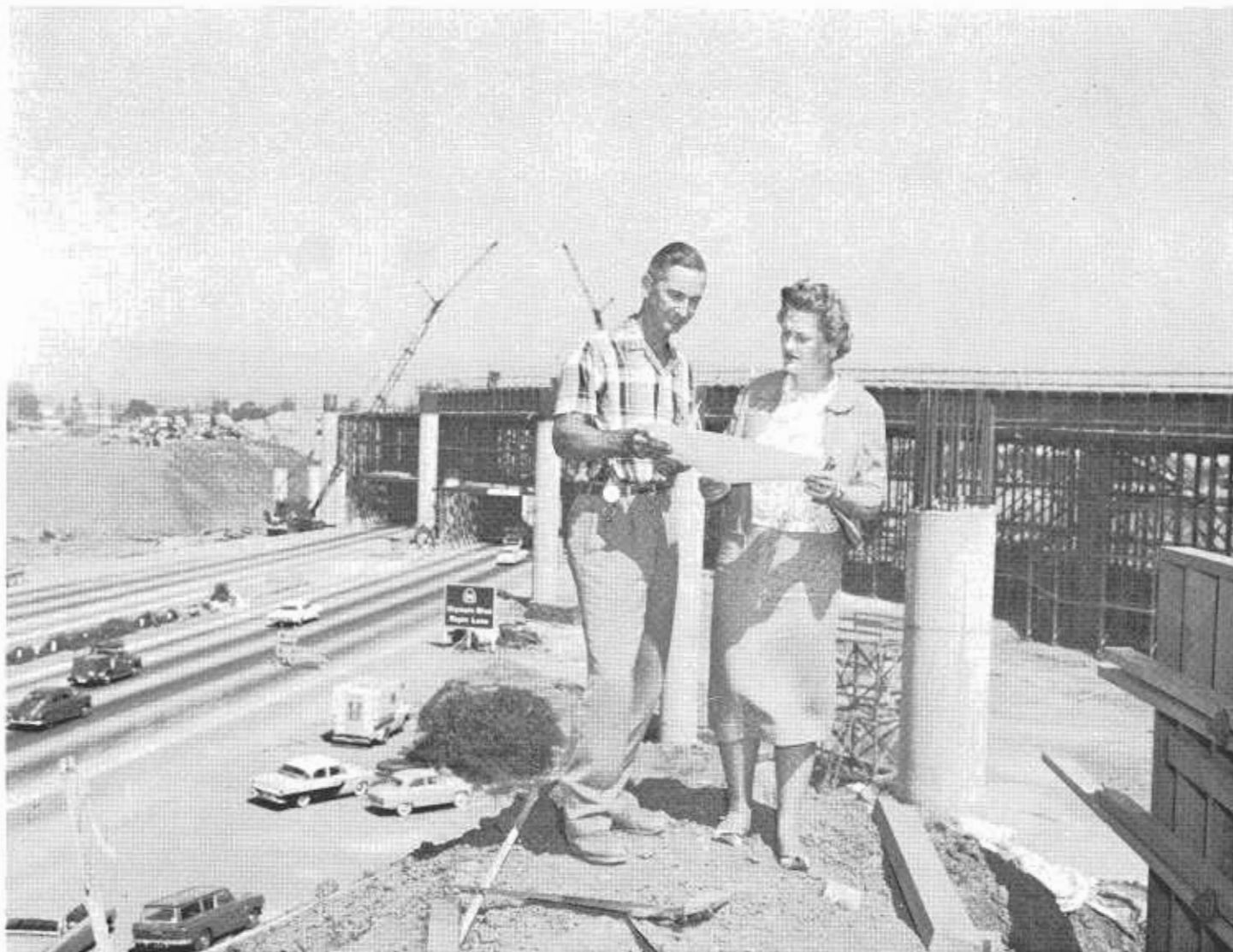
Associate Highway Engineer Marilyn Reece, who supervised design of 3-level San Diego-Santa Monica Freeway Interchange in Los Angeles, has on-site discussion with Assistant Resident Engineer Thomas McKinley.
