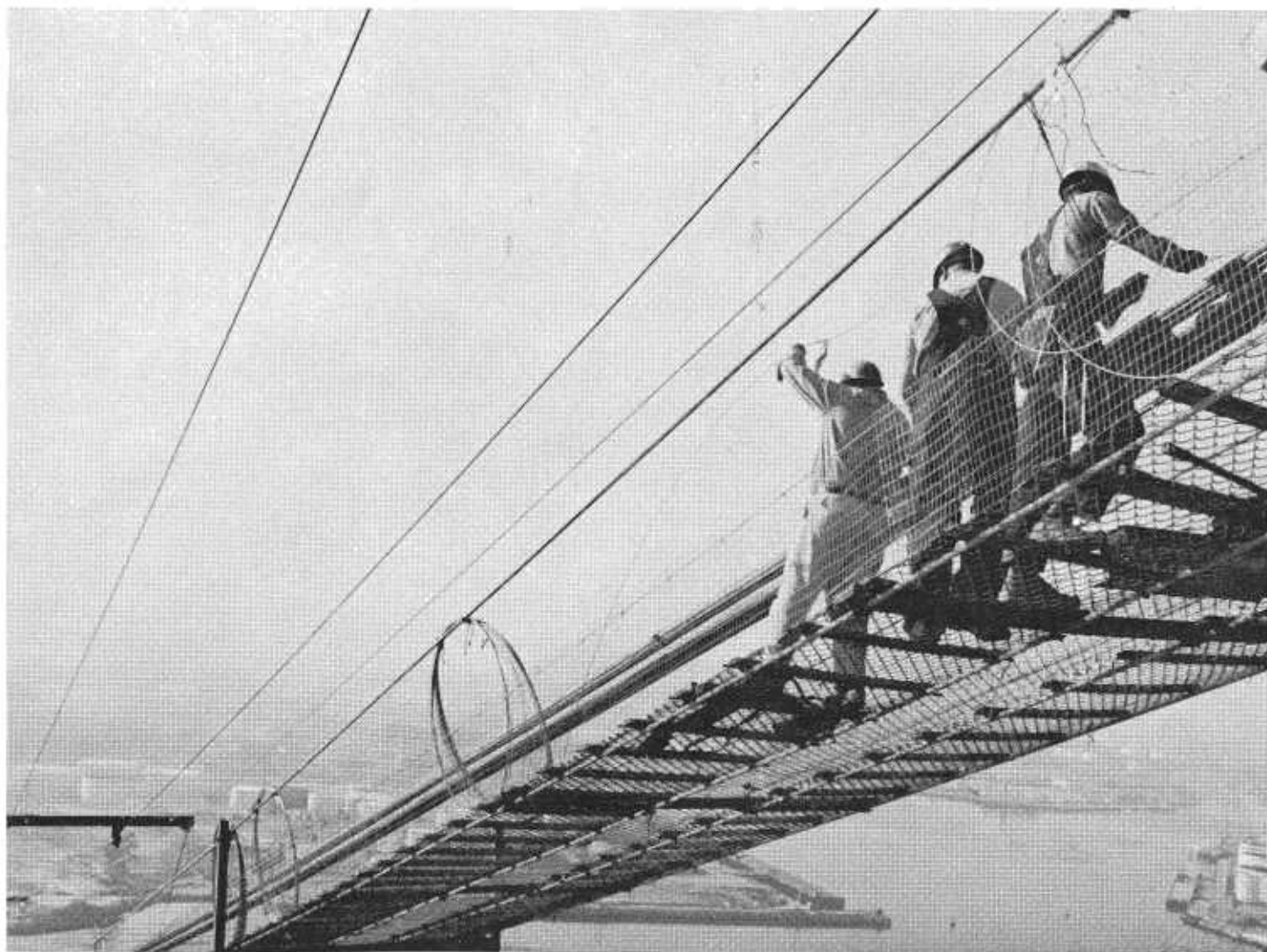
THE CATWALK. The photo shows the four supporting cables, wire mesh, wood cleats, two side cables and side wire mesh.
