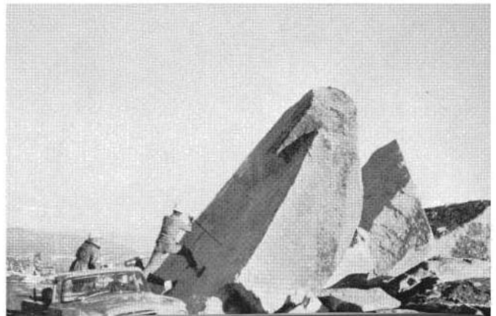
Portion of the same 500 tons of granite dropped by final charge November 29th. Further blasting was necessary to break pieces small enough for bulldozer to handle. (Photos by Robert Dunn)
