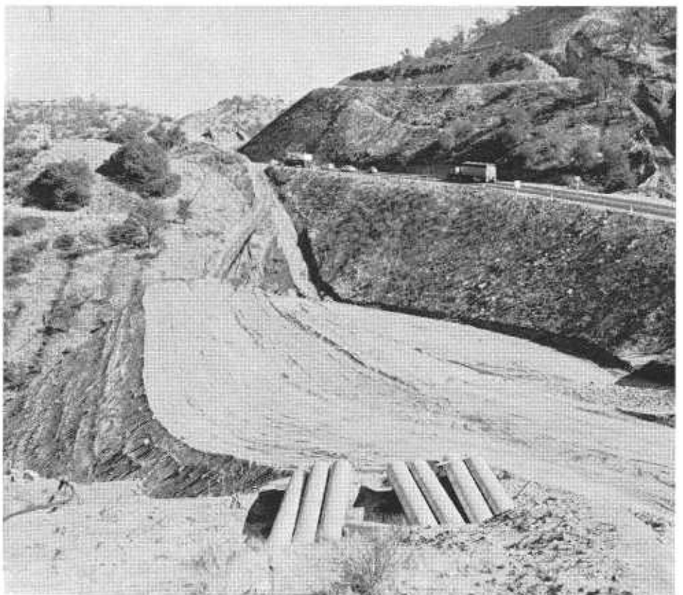
Benched cut and heavy fill partly completed. Note steep haul roads in rugged terrain.
