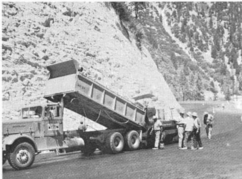
A crew completes paving of the fourth lane on the new widened portion of the Big Bear Highway.
