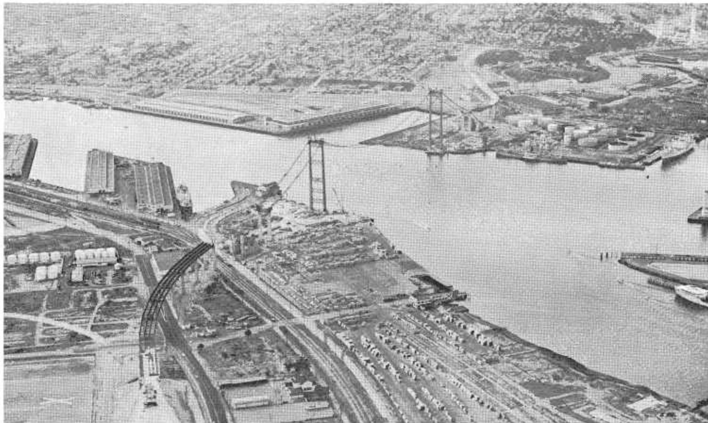
This aerial photo, looking southwest, shows the bridge under construction with the catwalk and partially completed cables suspended between the towers.
