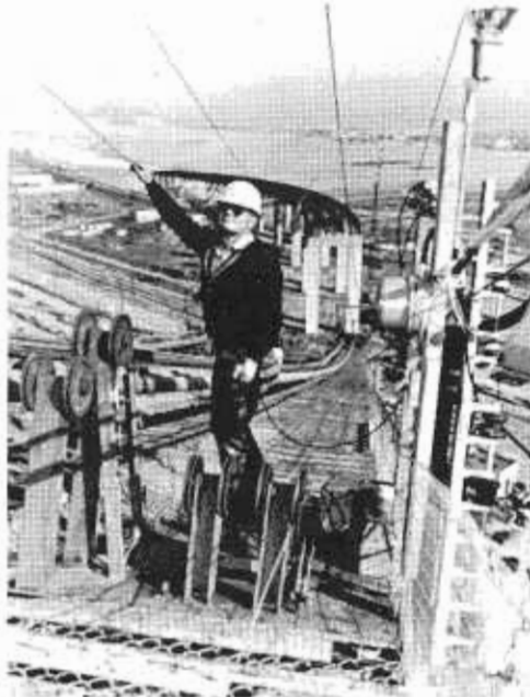
FRONT COVER: Division of Highways Photographer Robert Dunn climbed to the top of the tower to get this shot on the uncompleted Vincent Thomas Bridge connecting the City of San Pedro and Terminal Island in Los Angeles Harbor. Photo shows contractor's man at work on cable spinning, which was completed in early December 1962. (See story page 9 et seq.)
