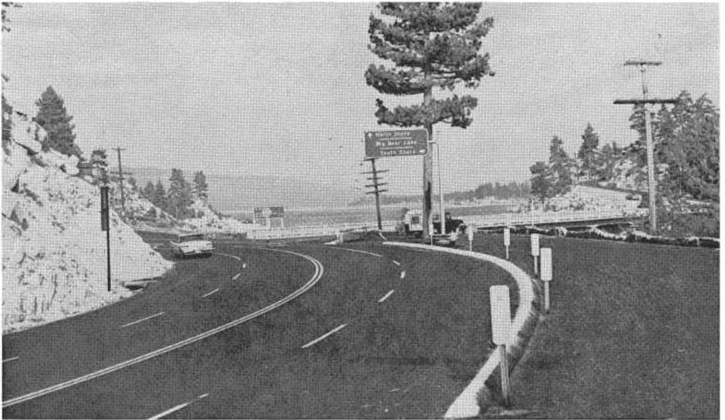
Looking out across Big Bear Lake from the east end of the road widening job.
