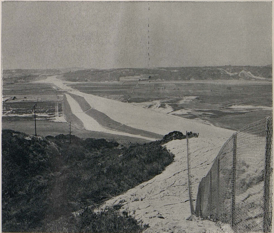
The 4,000,000-cubic-yard settlement fill across the San Dieguito River Channel showing the left strut.
