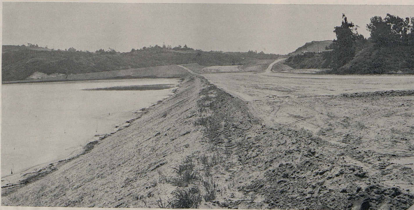
The embankment at the south side of Batiqitos Lagoon. Note the "heave stakes" at the top of the embankment.
