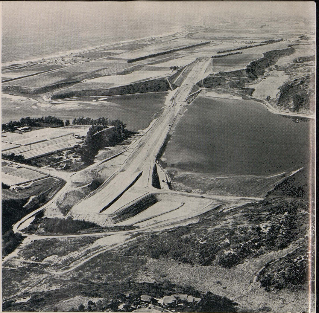
The fill across Batiquitos Lagoon under construction, looking north from Encinitas. The City of Carlsbad is in the far background.
