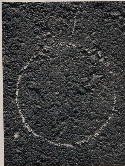
FIGURE 4B. Relation of permeability to surface texture. Penetration rate on this section was 580 millimeters per minute.
