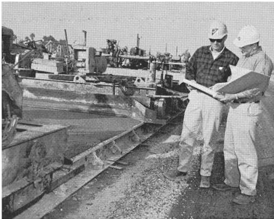
On construction, Steve acts as the resident engineer's representative on one phase of the job. Here he confers with Clarke Tape, contractor's paving superintendent during construction on the San Diego Freeway.
