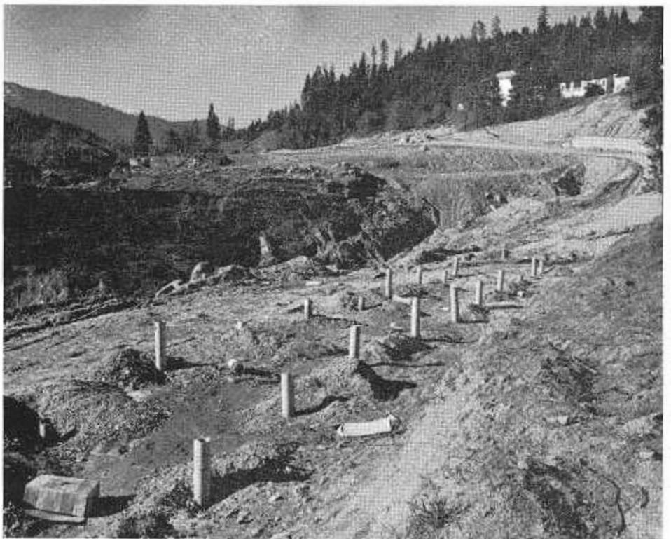
Vertical drainwell installation in Dunsmuir. Pipes were capped and a pervious blanket placed over area.
