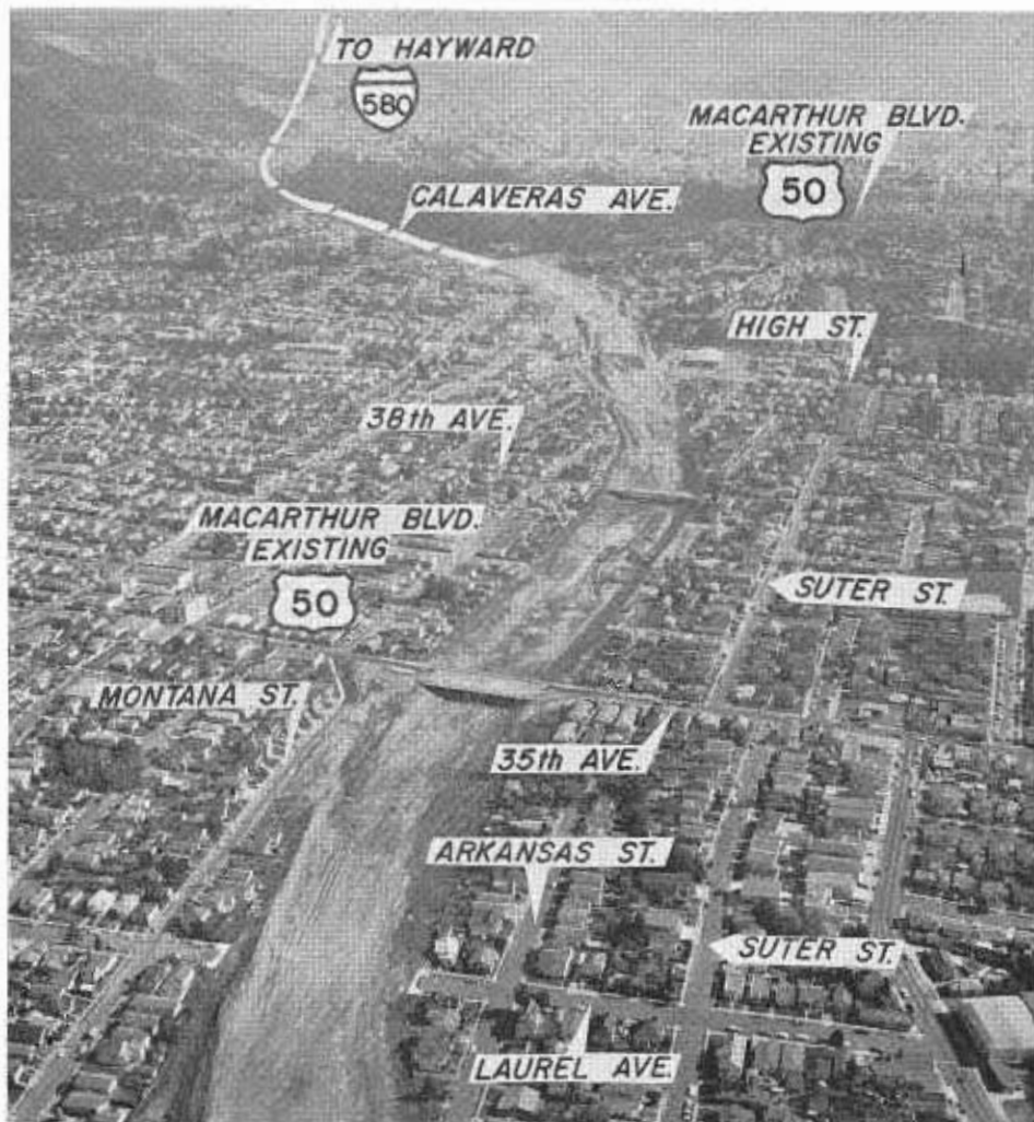
Construction progress on Interstate 580 (MacArthur Freeway) viewed easterly from Maple Avenue towards Calaveras Avenue.
