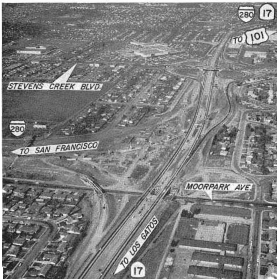
Construction in progress on the Sign Route 17-Route 239 interchange in San Jose. From this point, Interstate 280 starts toward San Francisco.
