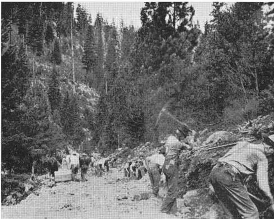
The original state highway through the Sacramento River Canyon was constructed nearly 50 years ago with pick and shovel labor and horse-drawn scrapers.
