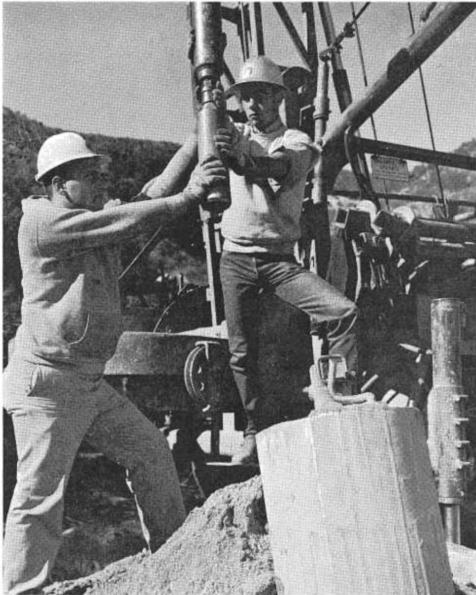
Working with the materials section along the route of a future freeway. Steve removes a soil sample from the drill rig. Assisting is Dick Hubinger, engineering aid.
