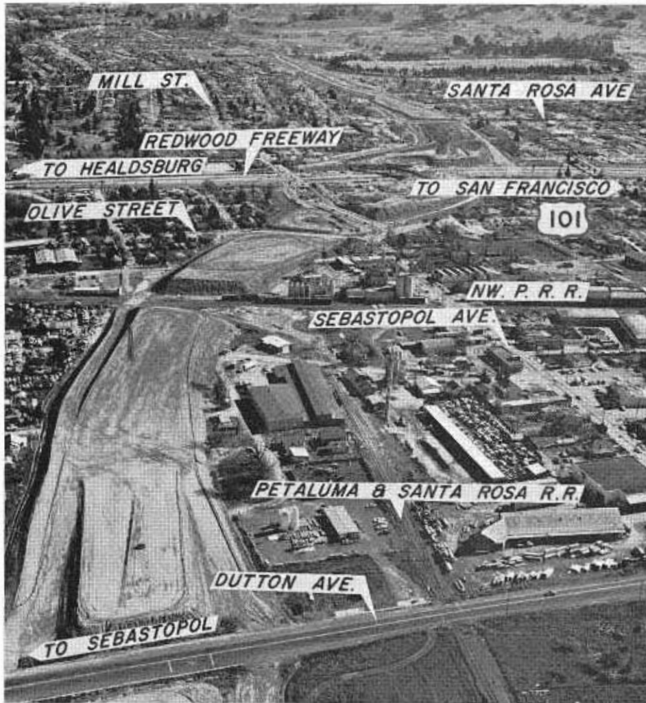
Construction progress on State Sign Route 12 in Santa Rosa viewed easterly from Dutton Avenue.
