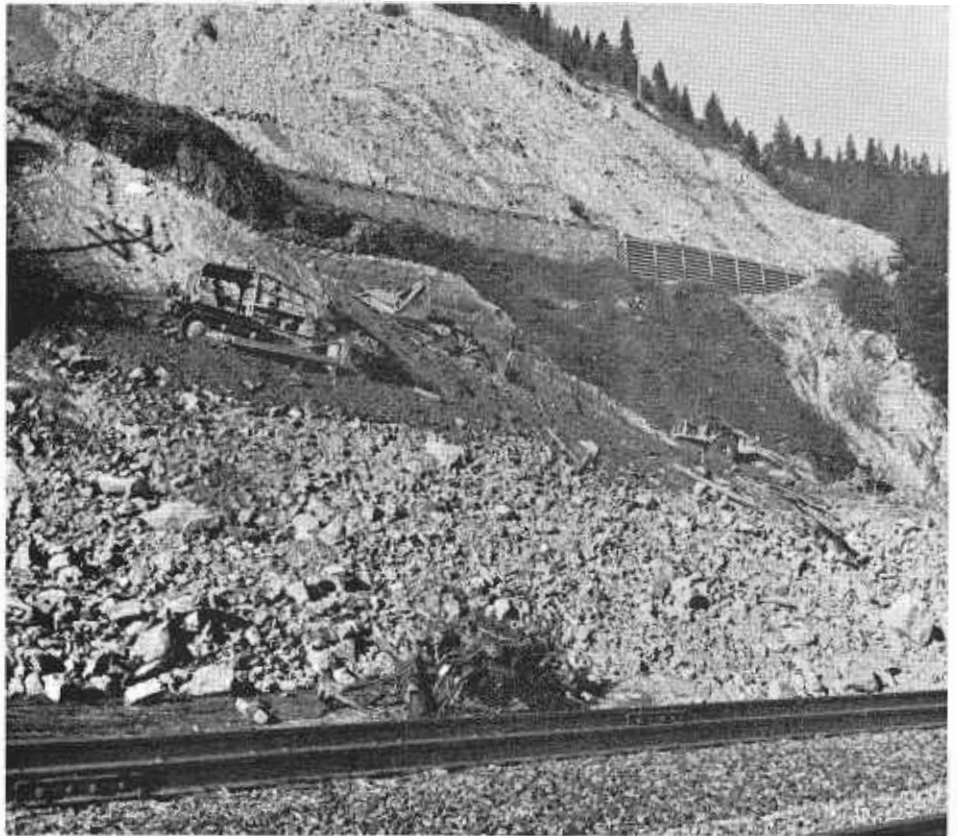
Slide removal operations at site of big slide. Railroad has been relocated from original location at base of bluff under retaining walls.
