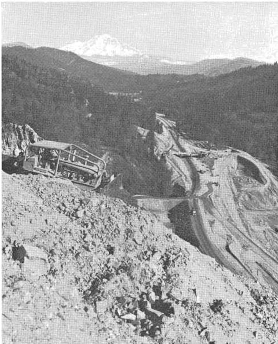
Looking north from top of large slide at Sweetbrier. Bulldozer approximately 500 feet above grade. This was area where channel change was made and railroad relocated.
