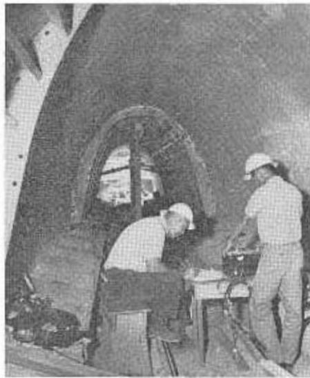
Control readings on stress and strain meter gauges are being recorded on this reinforced steel culvert for design engineers. Readings were taken at regular intervals as the culvert was covered over with a 200-foot-high fill.
