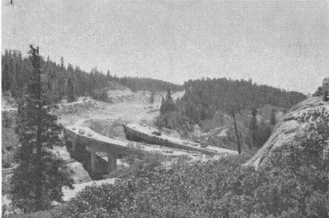
Construction of 22.6 miles of Interstate 80 in the Sierra Nevada will be completed next fall, providing continuous freeway and expressway on this route between San Francisco and the Nevada border. In photo above, the new Interstate freeway crosses over SSR 20. U.S. 40, which will be superseded, carries traffic in the background.
