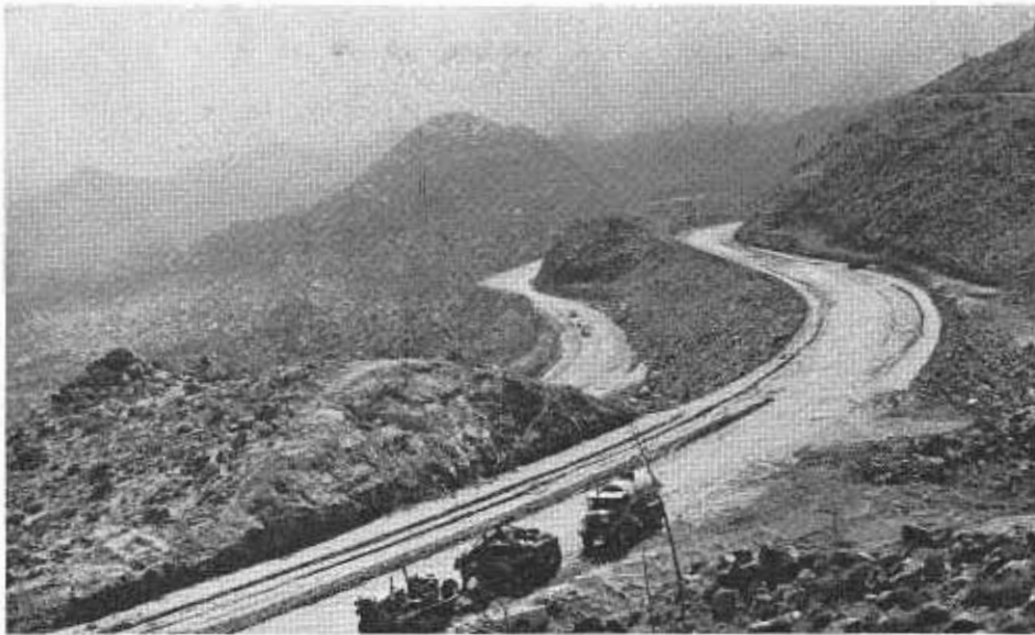
Ten miles of the westbound lanes (lower level) of the Interstate 8 Freeway in the Mountain Springs area near the San Diego-Imperial county line were opened to traffic in December. Work continues on the eastbound lanes.
