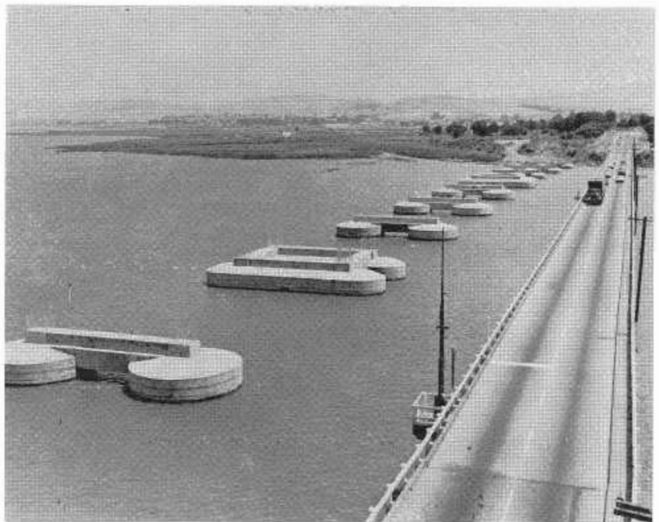
The substructure contract for replacement of the Napa River Bridge at Vallejo was completed in April 1963. The new bridge will be a high-level fixed span to allow waterway navigation to pass underneath. Present span (right) has a bascule span which must be opened an average of a hundred times a month.
