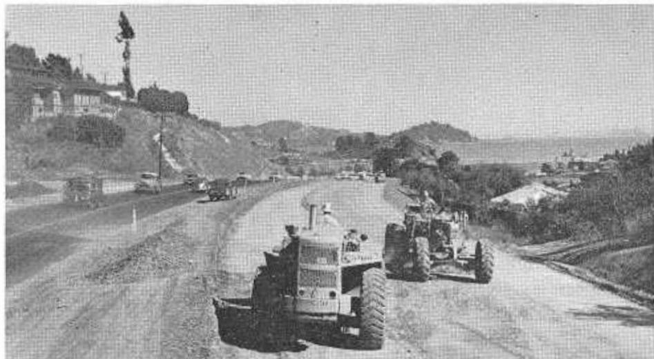
The widening of Tiburon Boulevard (SHR 52) in Marin County typifies continuing attention to conventional highways.
