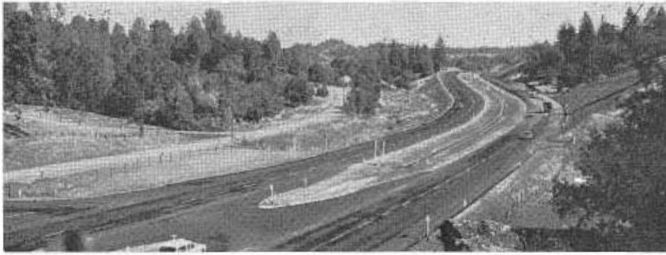
This section of SSR 108 west of Twain Harte in Tuolumne County completed in October typifies four-lane expressway construction in many scenic areas. The former highway, at left, connects with the expressway at left foreground.
