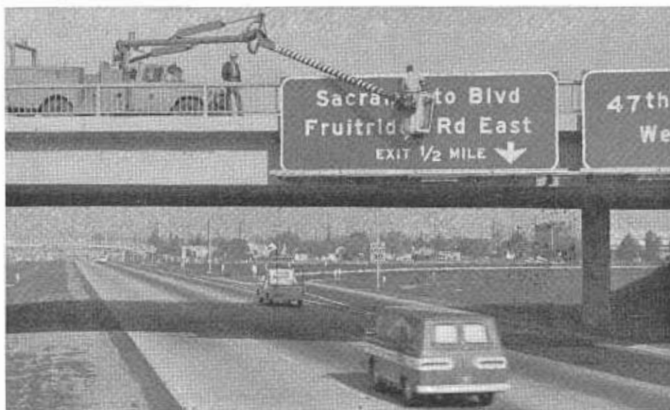
The skymaster being used to wash signs on the U.S. 99 freeway in Sacramento.
