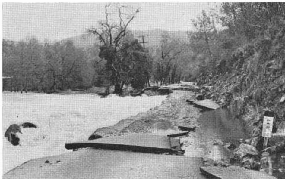
In February 1963 high water washed out this section of State Route 102 near Conn Dam in Napa County.
