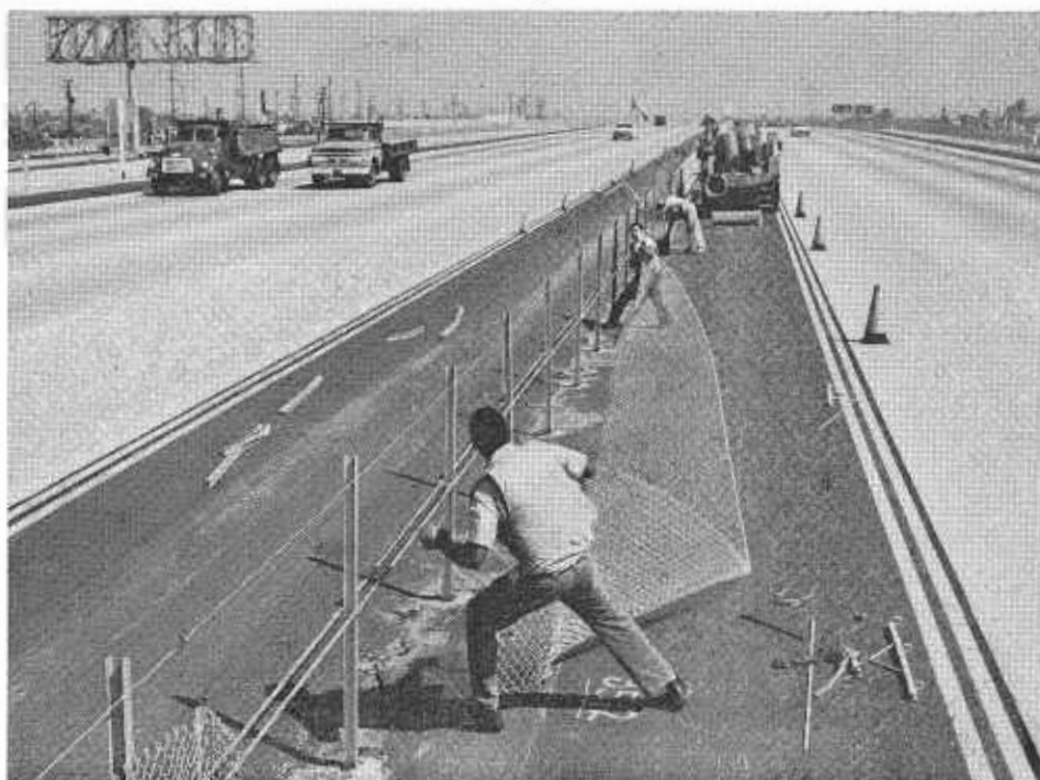
A maintenance crew repairs a section of chain link fence on the San Diego Freeway (Interstate 605) in Los Angeles.
