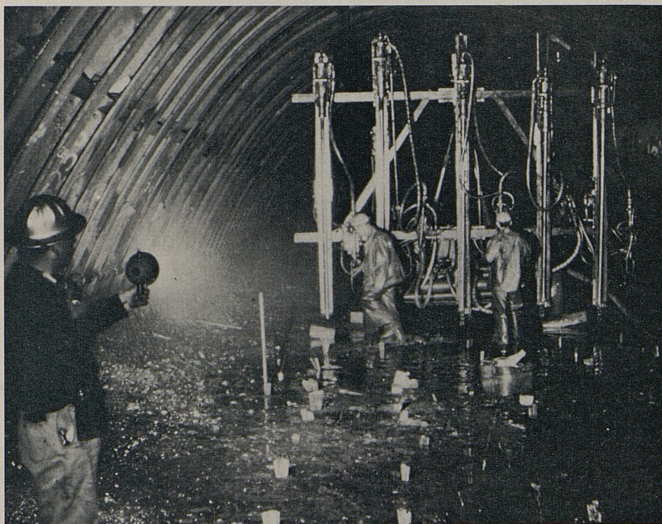
South portal top heading excavation—a bench jumbo drills vertical holes preparatory to lowering the floor of the initial excavation.
