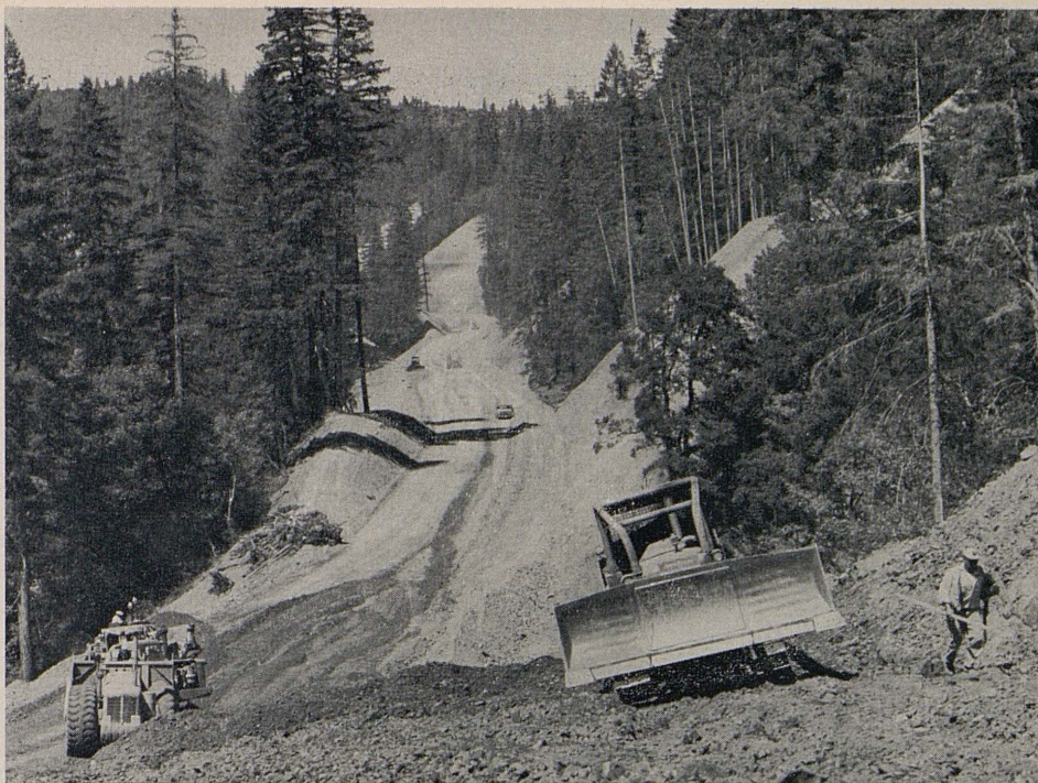
A northward view of heavy grading operations last year near the south tunnel approach.
