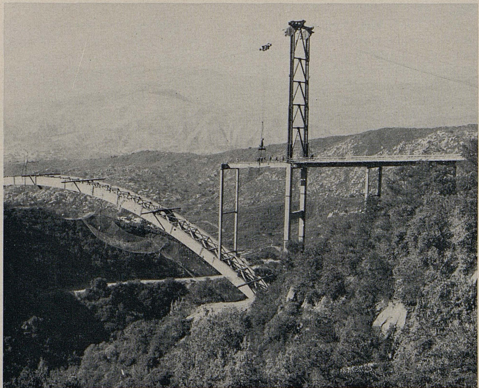
The final operation of setting girder spans on the arch. Girder span 7 is shown in position. Upon completion of this operation all highline rigging and temporary bracing are removed.
