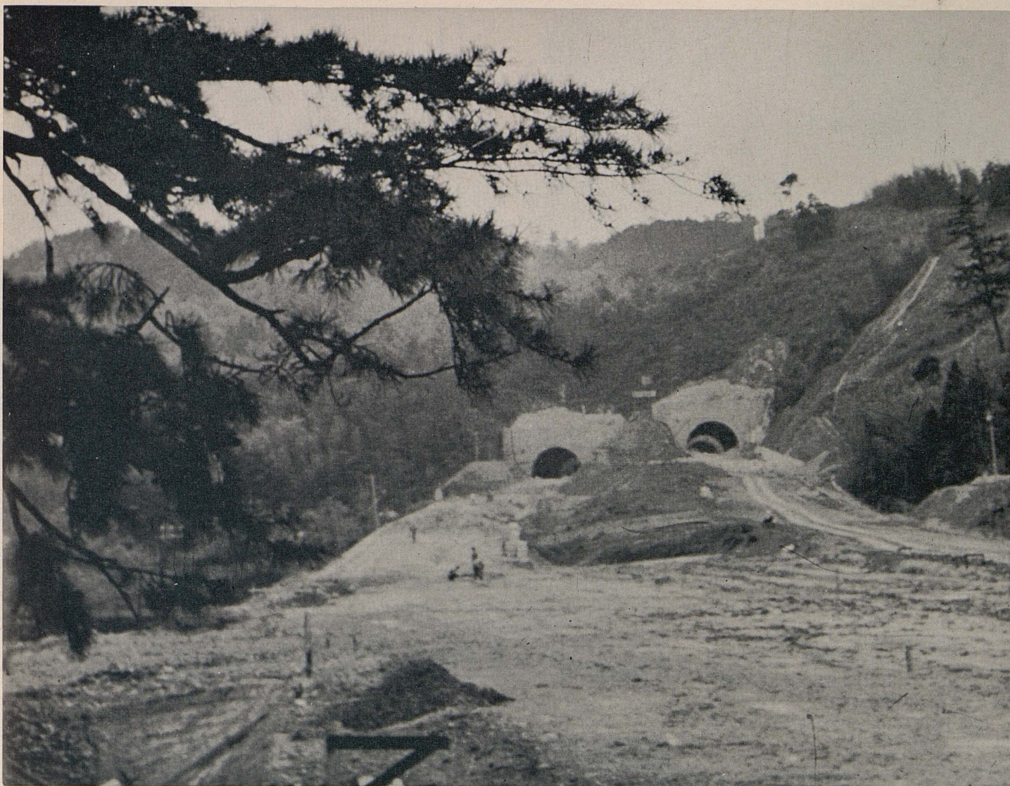
Two-level Shimamoto and Kajiwara Tunnels, also part of the Nagoya-Kobe Expressway, are seen under construction. When completed, the higher level tube will carry motorists to Kyoto and the lower one to Kobe.
