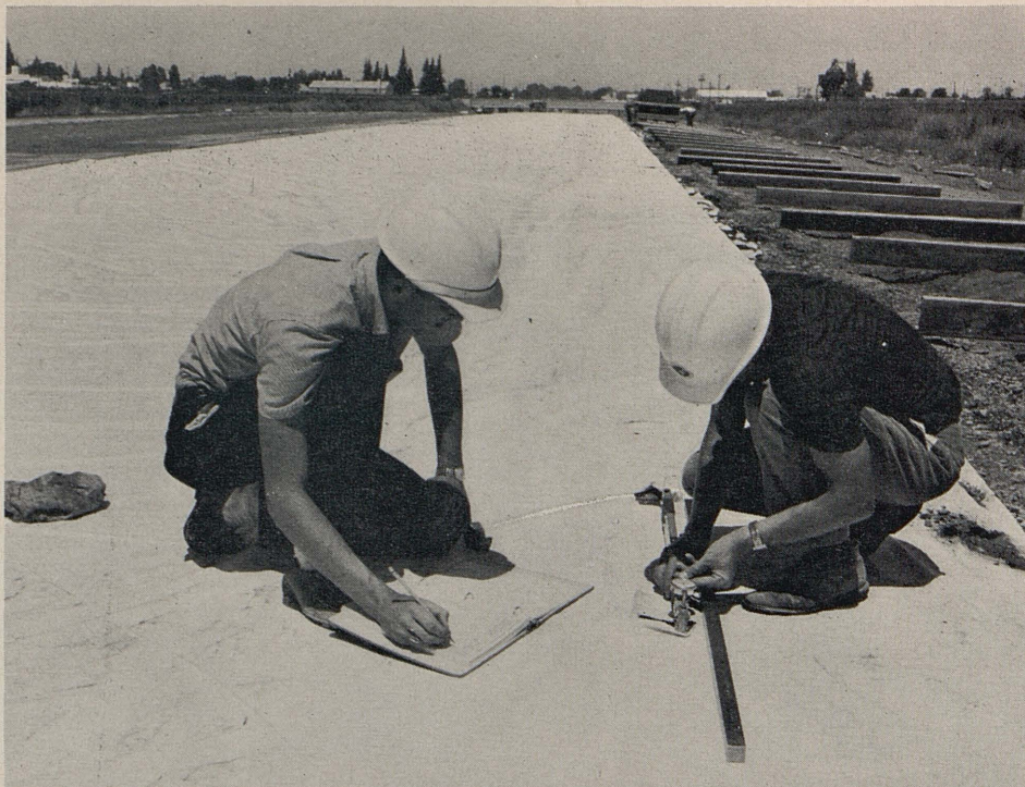
PHOTO 6. Changes in length of the concrete were measured by means of a comparator. Holes were cut in the plastic sheeting to reach gage plugs cast in the concrete.
