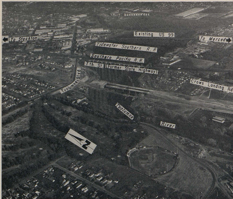
An aerial of the existing bridges across the Tuolumne River with the twin freeway spans under construction in the foreground.
