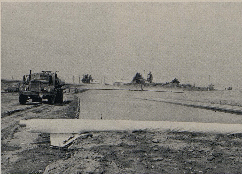
PHOTO 2. Special contractor-built spray rig keeps pavement wet until plastic membrane can be applied.
