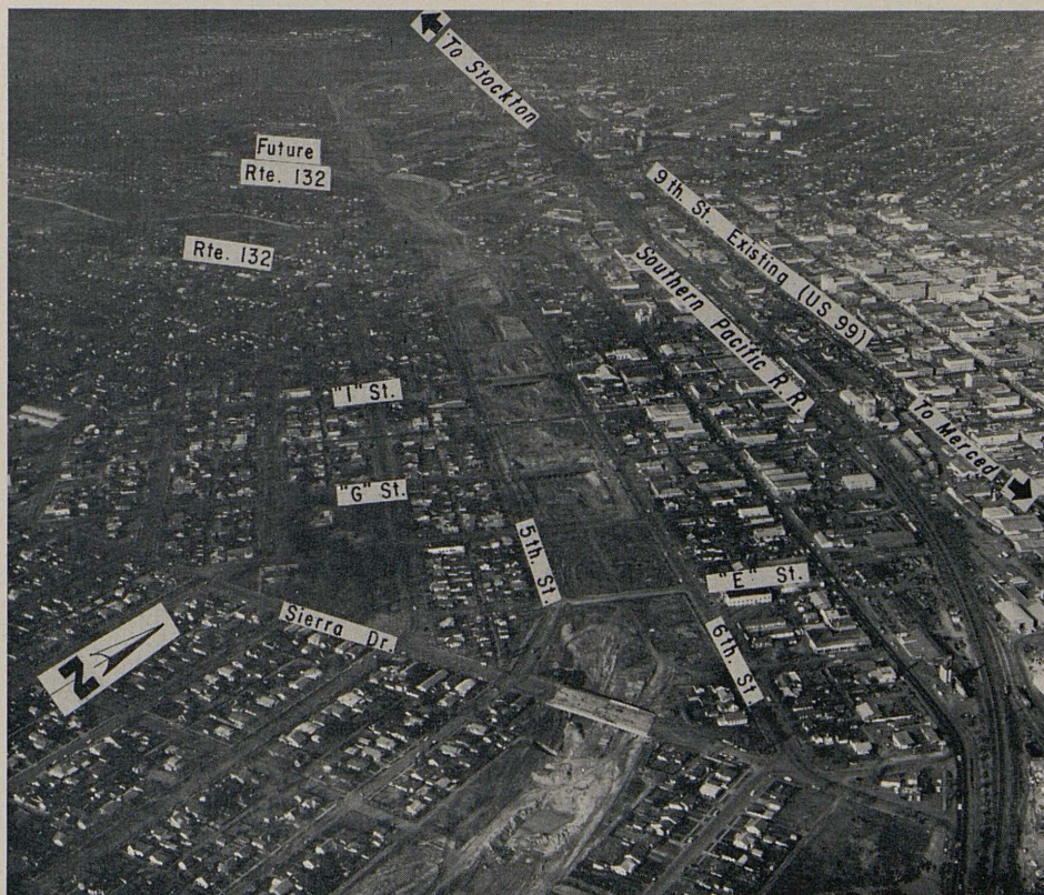
An aerial of grading operations on the new freeway through Modesto. The bridges are under construction.
