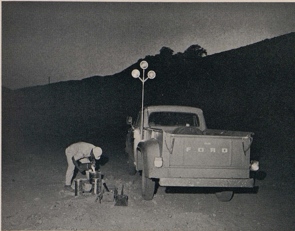
A high-level warning device with flashing lights protects an inspector making compaction tests. Compaction tests are made around the clock, requiring an inspector to make tests at night with contractor's equipment moving around him.
