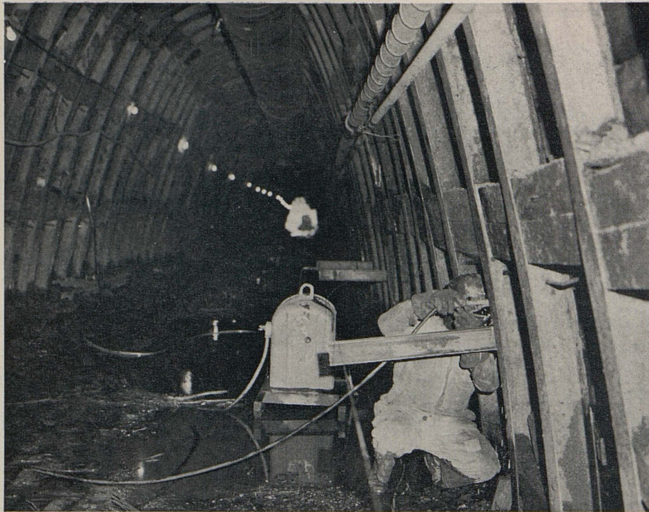
A welder attaches a brace to a steel support of the east footing drift.
