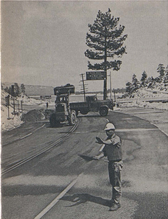
FRONT COVER: Division of Highways Employee Clifford Ahnlund, District VIII, demonstrates correct flagging procedure for controlling traffic when road is obstructed by equipment. Skip loader is picking up debris from slide on Rim of the World Highway near Big Bear Lake, San Bernardino County. Photograph by Lyman Rich, Claims Investigator, District VIII. See story on page 32.
