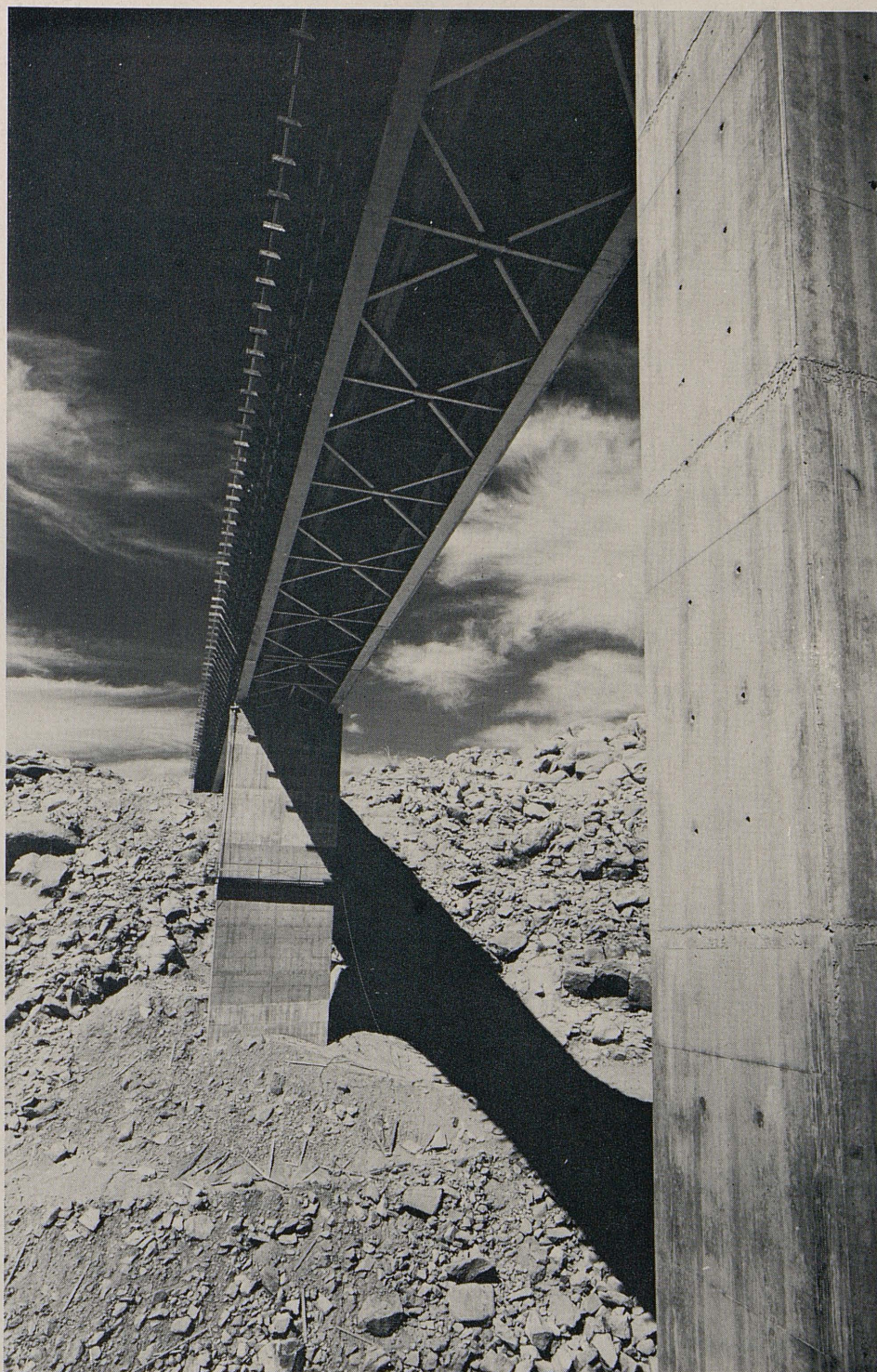
Devil's Canyon Bridge No. 2 under construction. The concrete forming can be seen protruding over the left side of the bridge.
