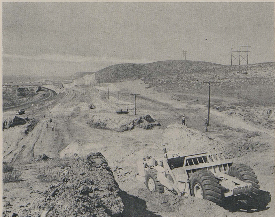
Grading on the new highway. The old highway is to the left. The pole line in the center will be moved outside of the right-of-way.
