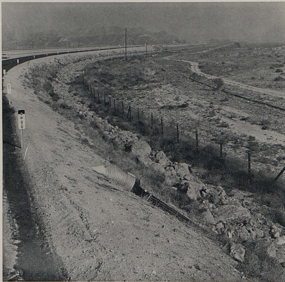
A six-foot-high wall of riprap separates the left bank of the Santa Clara River from the freeway about two miles east of Solemint.
