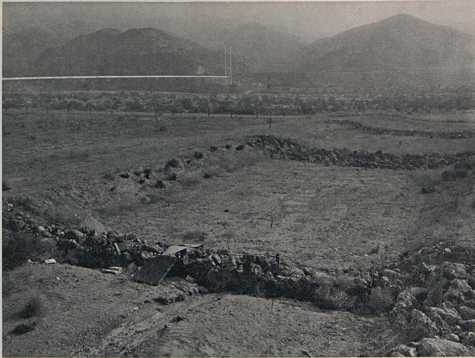
Check dams along the Santa Clara River are composed of steel rail and wire mesh double fences filled with rock. The view is downstream looking from the Tick Canyon Wash freeway bridge. The Southern California Gas pipeline spans the river in the left background.
