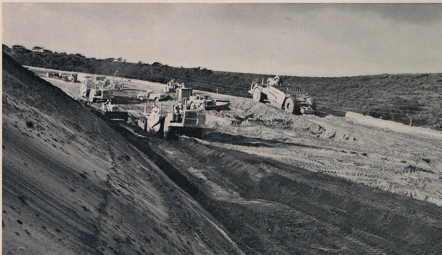
Grading operations on the "Big Sand Cut" section of San Antonio Road east of Vandenberg Air Force Base.
