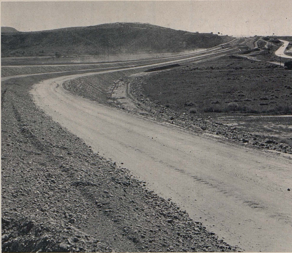
Grading operations on the new highway showing windrowed base material on the southbound lane in the foreground. The northbound lane is in the background; the old highway is upper right.
