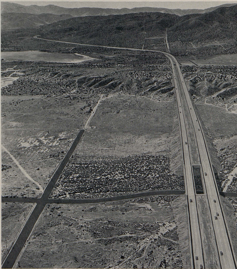
Sometime during the 1964-65 fiscal year, construction of the Antelope Valley Freeway will move north out of the mountains and into the desert. Intersecting road rendered in the foreground is future Avenue R. The road parallel to the rendering of the freeway is Division Street. Water at upper left is Palmdale Reservoir.
