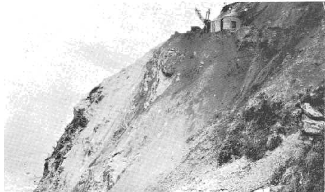
Below: Power shovel working at Alder Bluff in Del Norte County, not far from the Humboldt County line, about 1925. Cut must be made 32 feet deep here to get bench wide enough for narrow two-lane road.
