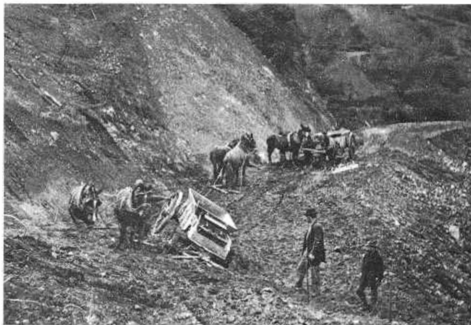
Construction mishap in Sonoma County in the Healdsburg area, in 1914. Establishing a stable road foundation has frequently been a problem on the Redwood Highway.
