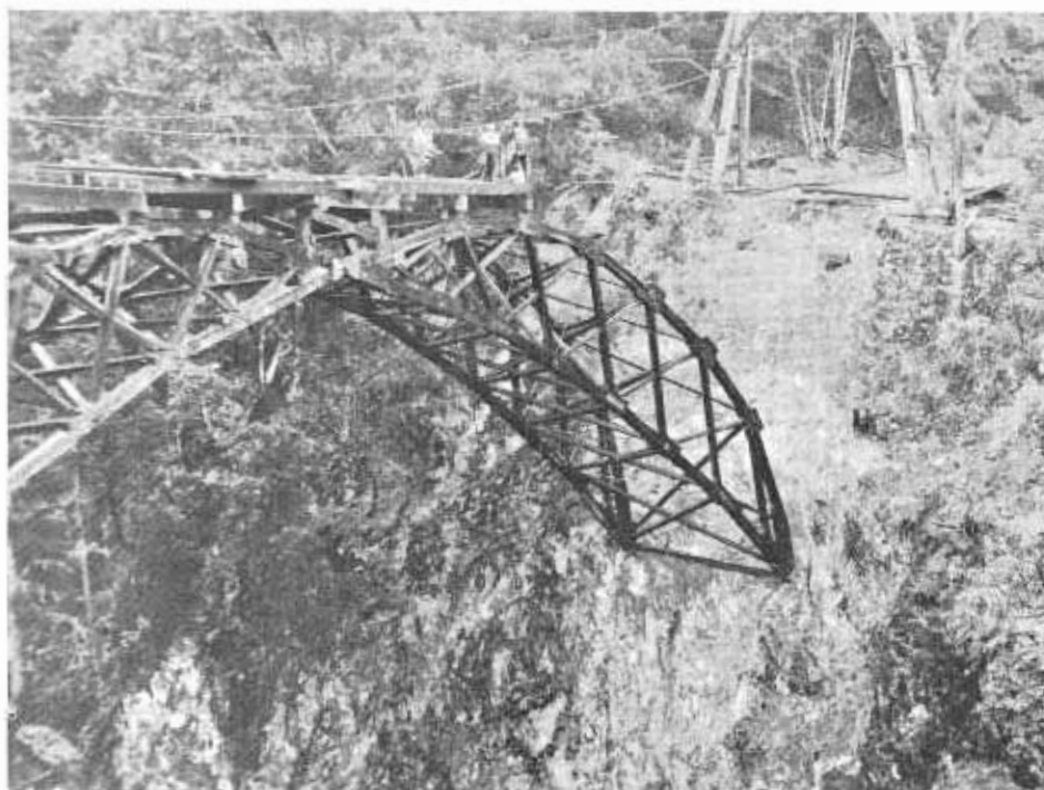
Double arch bridge with trusses made of wood, under construction at Rock Creek, Mendocino County, 1916. Note legs of tower on far bank, used to support lines for transporting materials into position. Bridge was replaced by a concrete one in 1930's.
