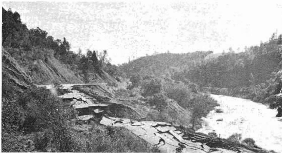
Above: Loss of considerable section of road due to slipout north of Cloverdale, Sonoma County. Stream is upper portion of Russian River.
