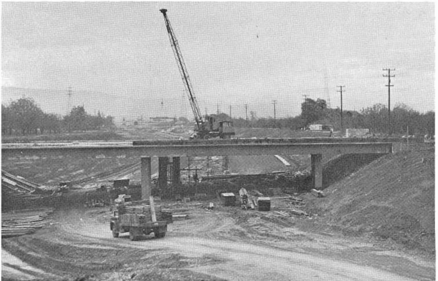
Picture shows cleared right-of-way for the future Route 237, with a closeup of the Dana Road Overcrossing under construction.
