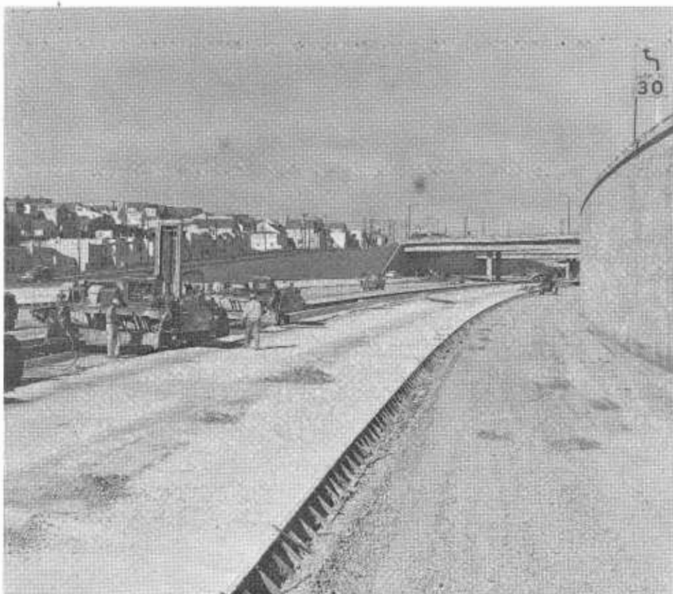
Paving operations along a section of six-lane freeway being built on Route 82 in San Francisco.
