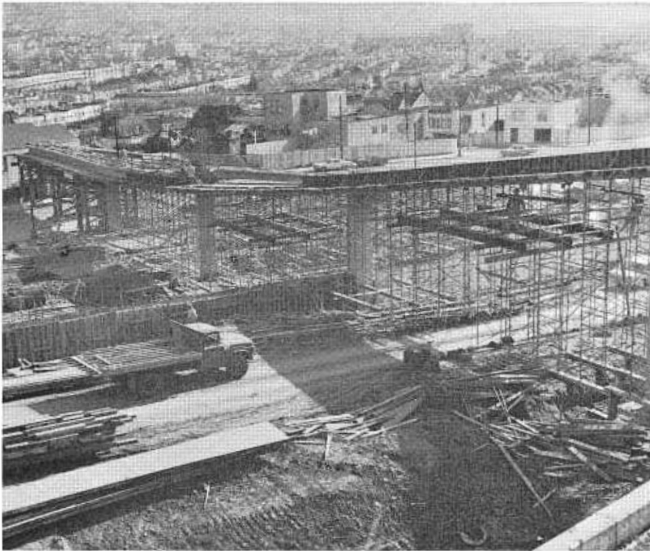
The Theresa Street Pedestrian Overcrossing is shown under construction with forms in place for pouring the side railing. The job is on the Ocean Avenue to Mission Street section of Route 82.
