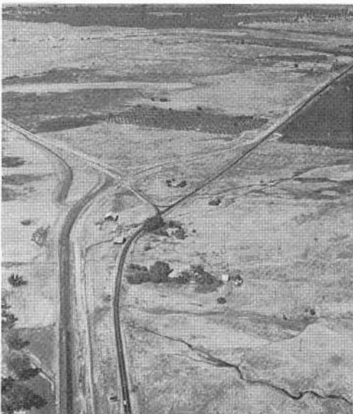
Construction photo shows old and new alignment at Wicks Corner. Relocated highway turns to the right. Road at left goes to Chico.
