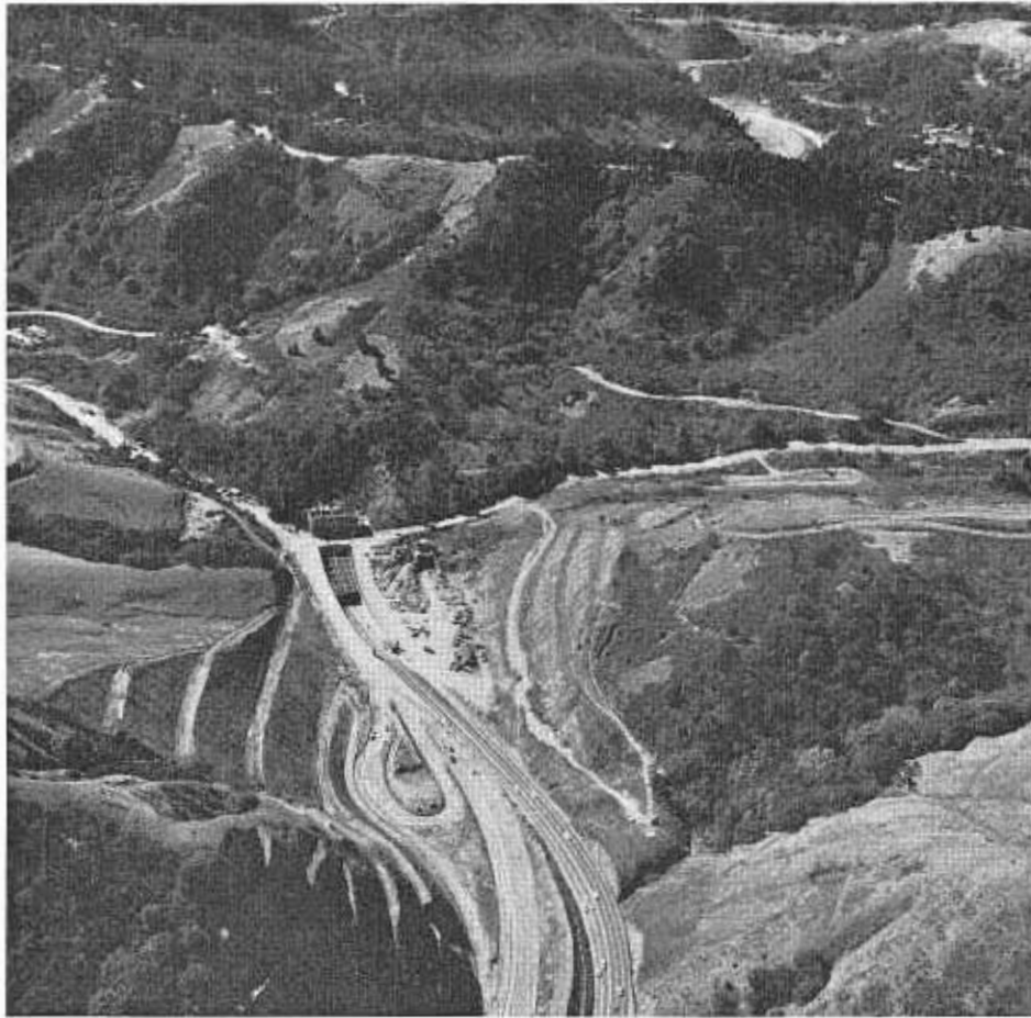
Construction on an eight-lane freeway on Route 24 shows the east portal of Caldecott Tunnel 1 with the new bore directly to the right.
