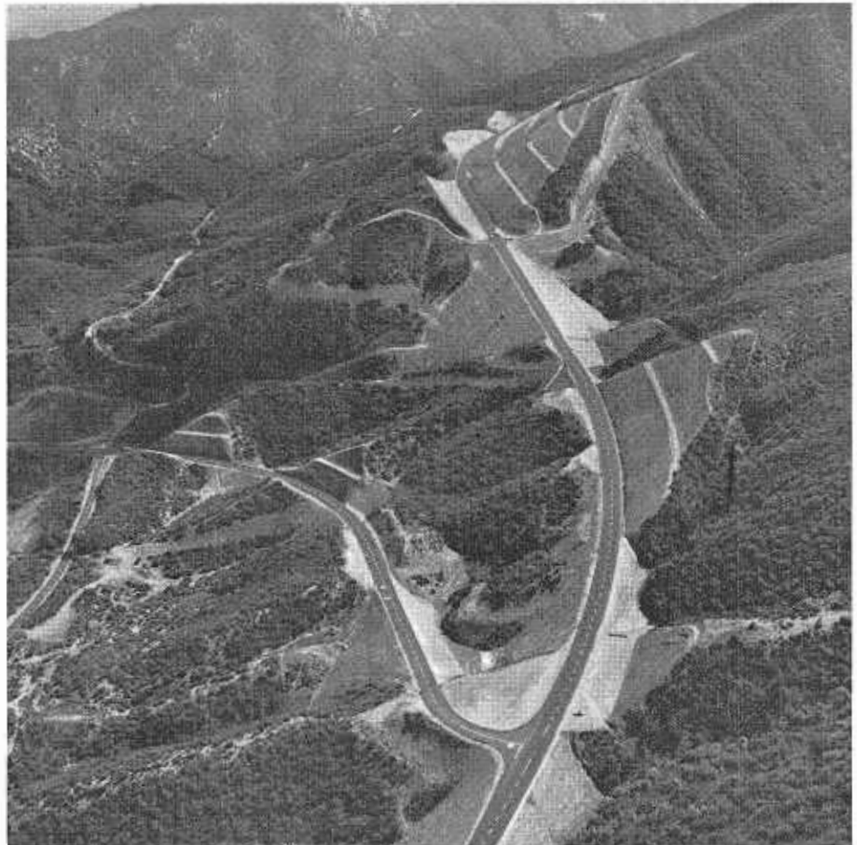
Cut and fill construction on the new highway near the top of San Marcos Pass. Winding sections of the old alignment can be seen in left background.
