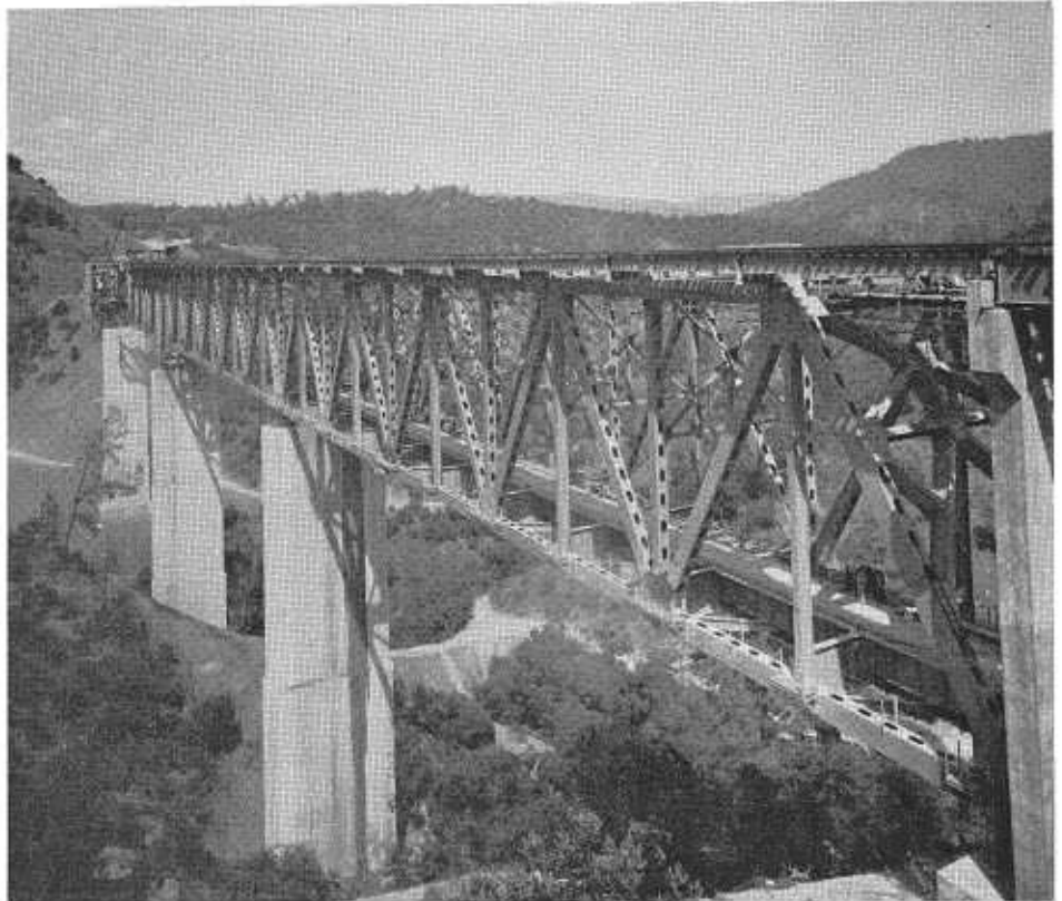
Shows details of bridge construction prior to completion. Total structural steel, 11,000 tons; concrete, 40,000 cubic yards.
