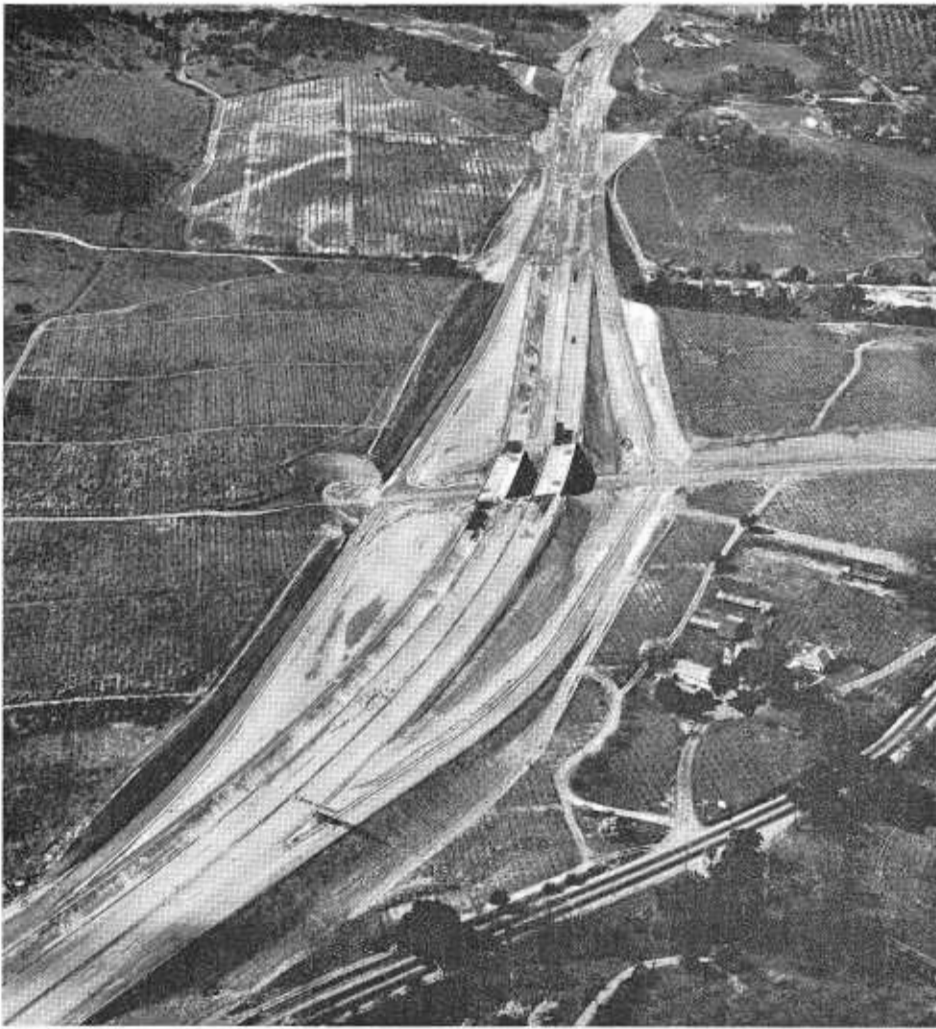
Construction on the new four-lane freeway on Route 101 at Asti, known commonly as the Asti Bypass. This interchange will provide easy access to the Italian Swiss Colony winery.
