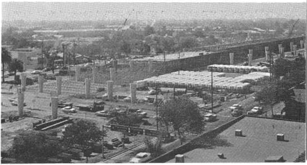
This view looks southeasterly at the 29th-30th Street Freeway (Interstate 80) construction now in progress in Sacramento. The graceful tapered columns will support the viaduct structures.
