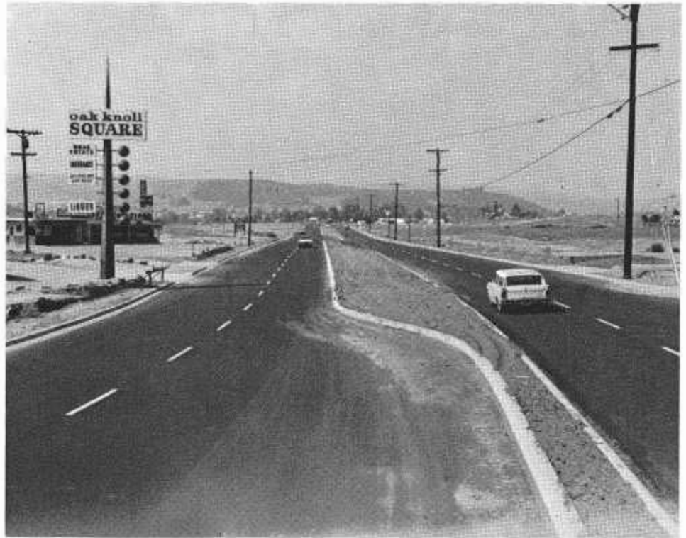
A nearly completed four-lane divided section on Poway Road in a rapidly developing area north of San Diego. This project was financed under the federal aid secondary county road program.
