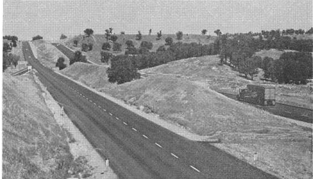
This section of the Interstate 5 Freeway is part of a 12.2-mile project completed in April between Red Bluff and the Shasta county line. A total of 81.5 freeway miles on this route are completed, under construction or budgeted between south of Willows in Glenn County and north of Redding in Shasta County.
