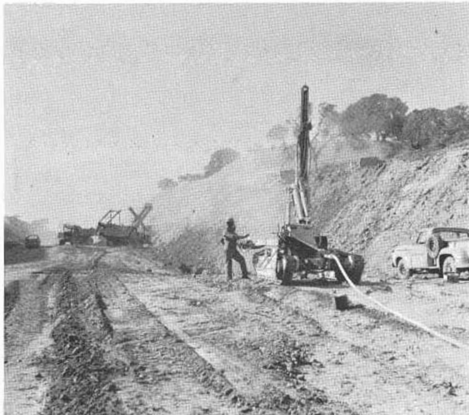
The workmen at right prepare to set demolition charges during the construction of a 12.4-mile, four-lane expressway on Route 152 to bypass an area which will be used for the San Luis Reservoir.
