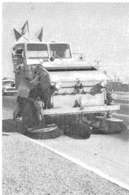
A rotary broom cleaning a gutter on the Bayshore Freeway south of San Francisco.
