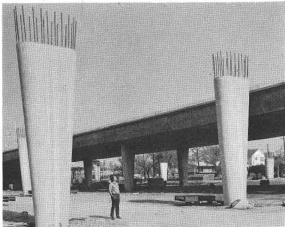
Now under construction is the Fort Sutter Viaduct between 29th and 30th Streets in Sacramento, which will carry traffic on Interstate 80. Tapered piers and sloping sides of girders are used to enhance the appearance of the structure.
