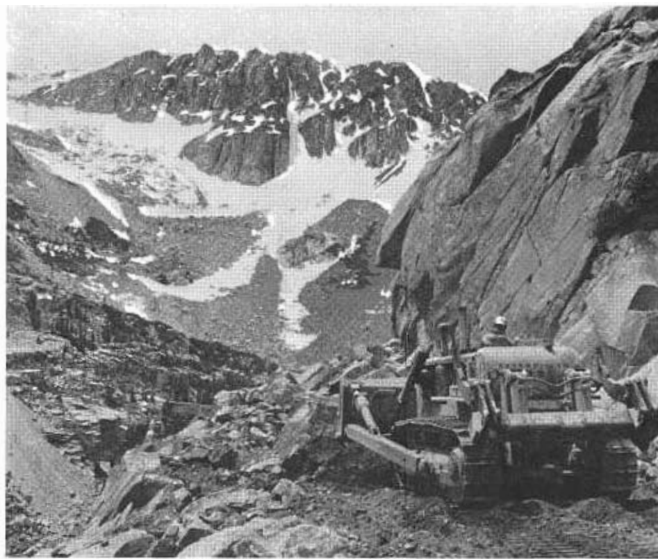
PHOTO LEFT: A bulldozer finds rough going in the difficult terrain of Lee Vining Canyon east of Yosemite National Park in Mono County. Two miles of the Tioga Pass Road (Route 120) are under construction as a two-lane expressway, and another 4.1 miles have been budgeted.
