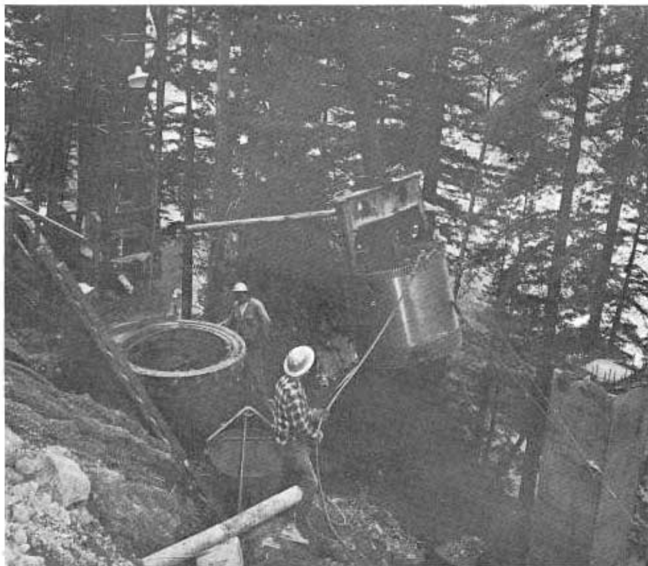
A rotary drill rig excavates for uphill shafts of the viaduct while supported on log cribbing.
