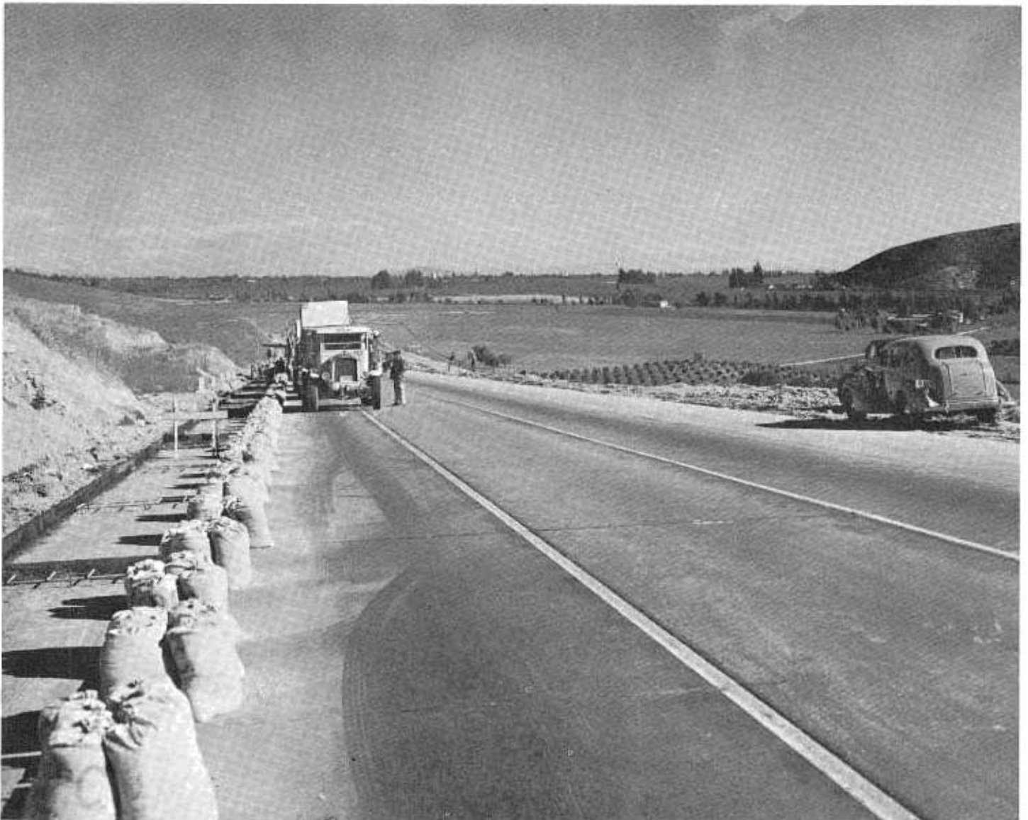
Work nears completion in early 1937 on the new Garvey Avenue "superhighway" in Los Angeles County, a four-lane roadway with only two traffic signals and two boulevard stops in its entire 27 miles. In a few years it had become lined on both sides with small stores and stalls of all kinds bringing with them traffic congestion and the need for innumerable 25-mile-per-hour zones.
