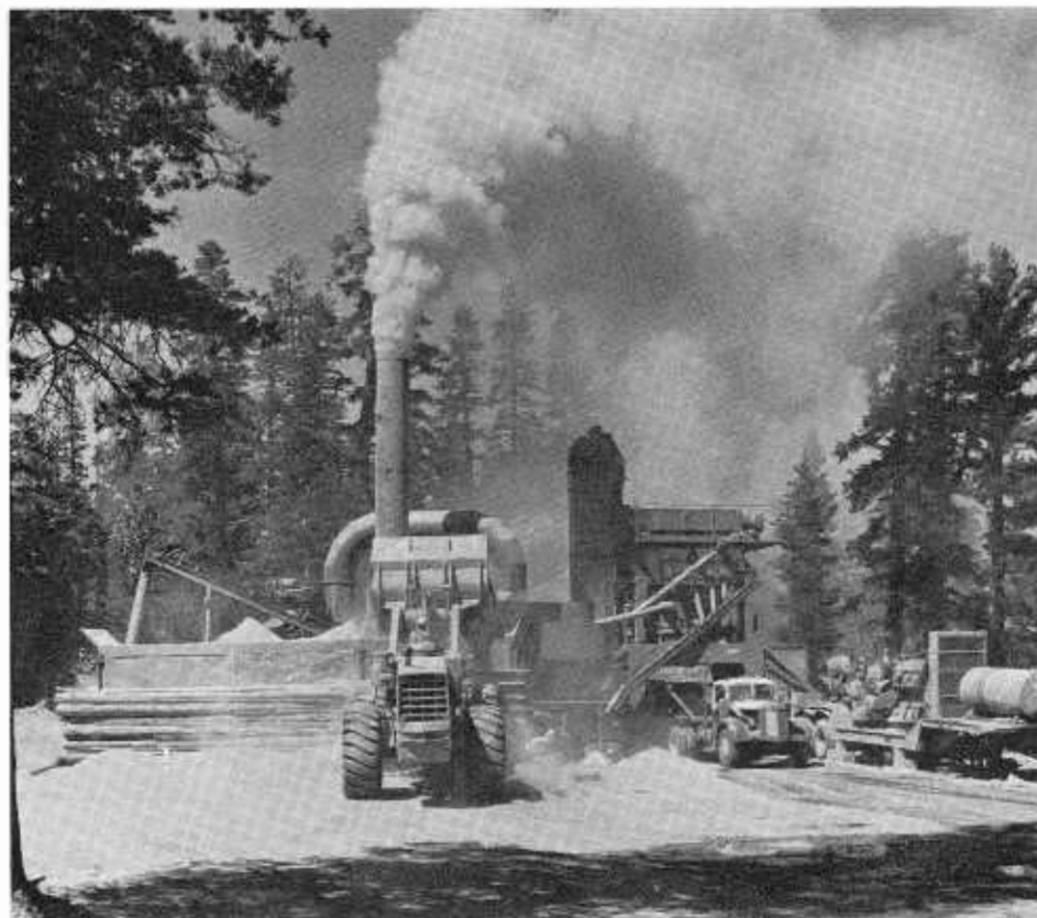
A new portable batch or "hot plant" near Silver Lake prepares asphalt concrete for the new highway.
