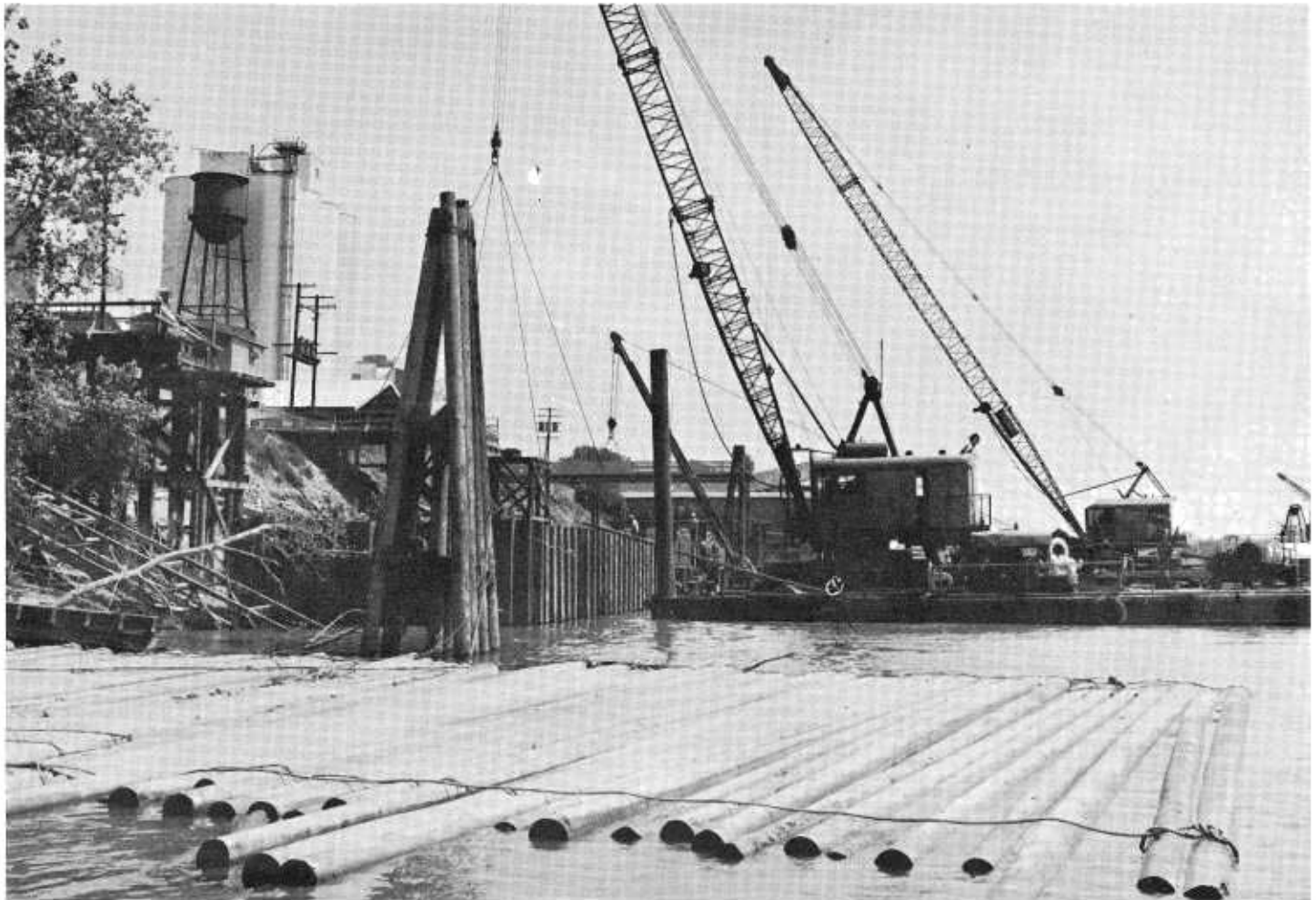
Early construction stage at the Yolo County side. Two large derrick barges lower a 64-ton steel water system inside the sheet pile cofferdam. A raft of timber foundation piles is in the foreground.
