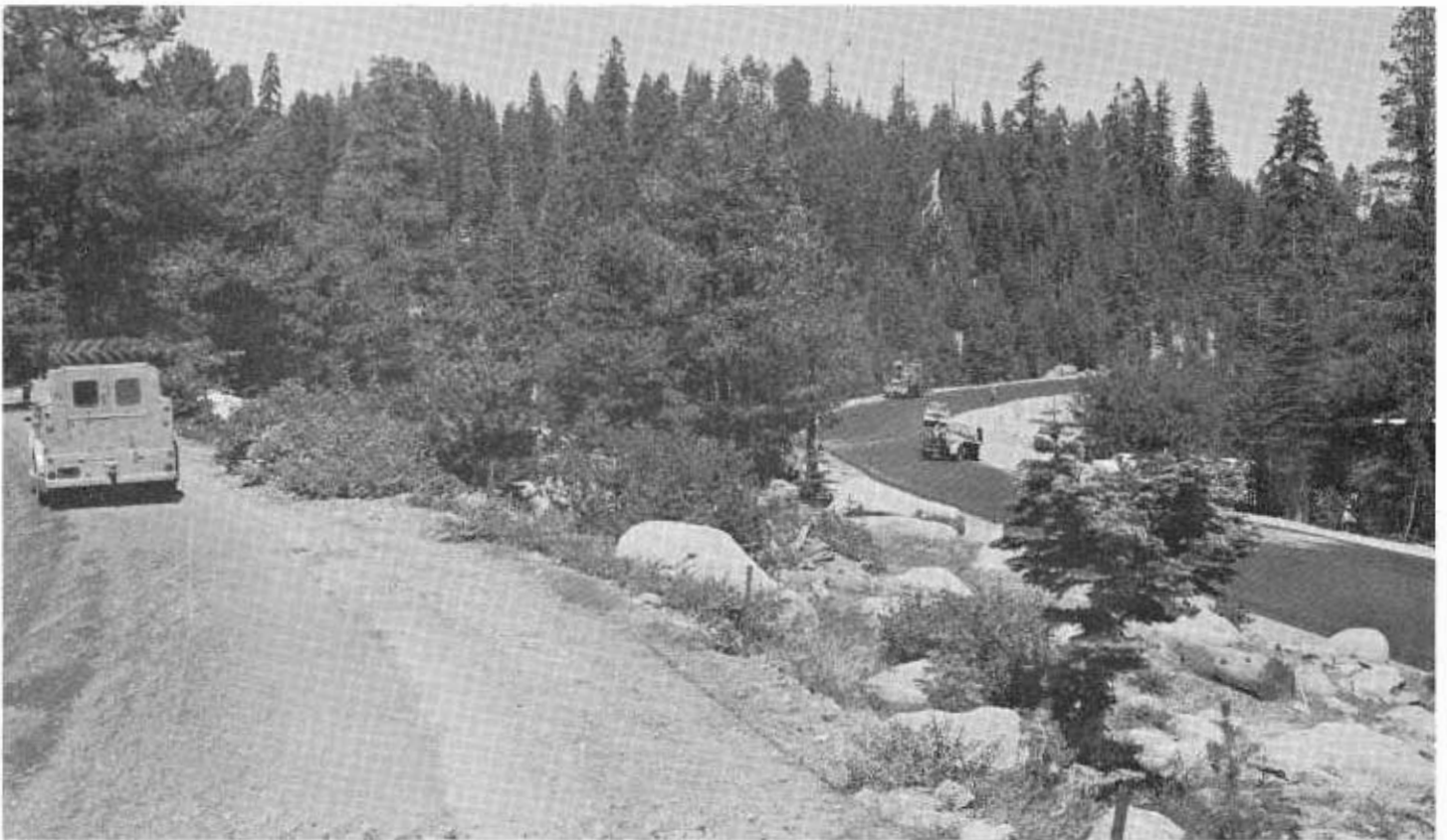
The nearly completed roadway on new alignment (right) has wide, sweeping curves and gentle grades.
