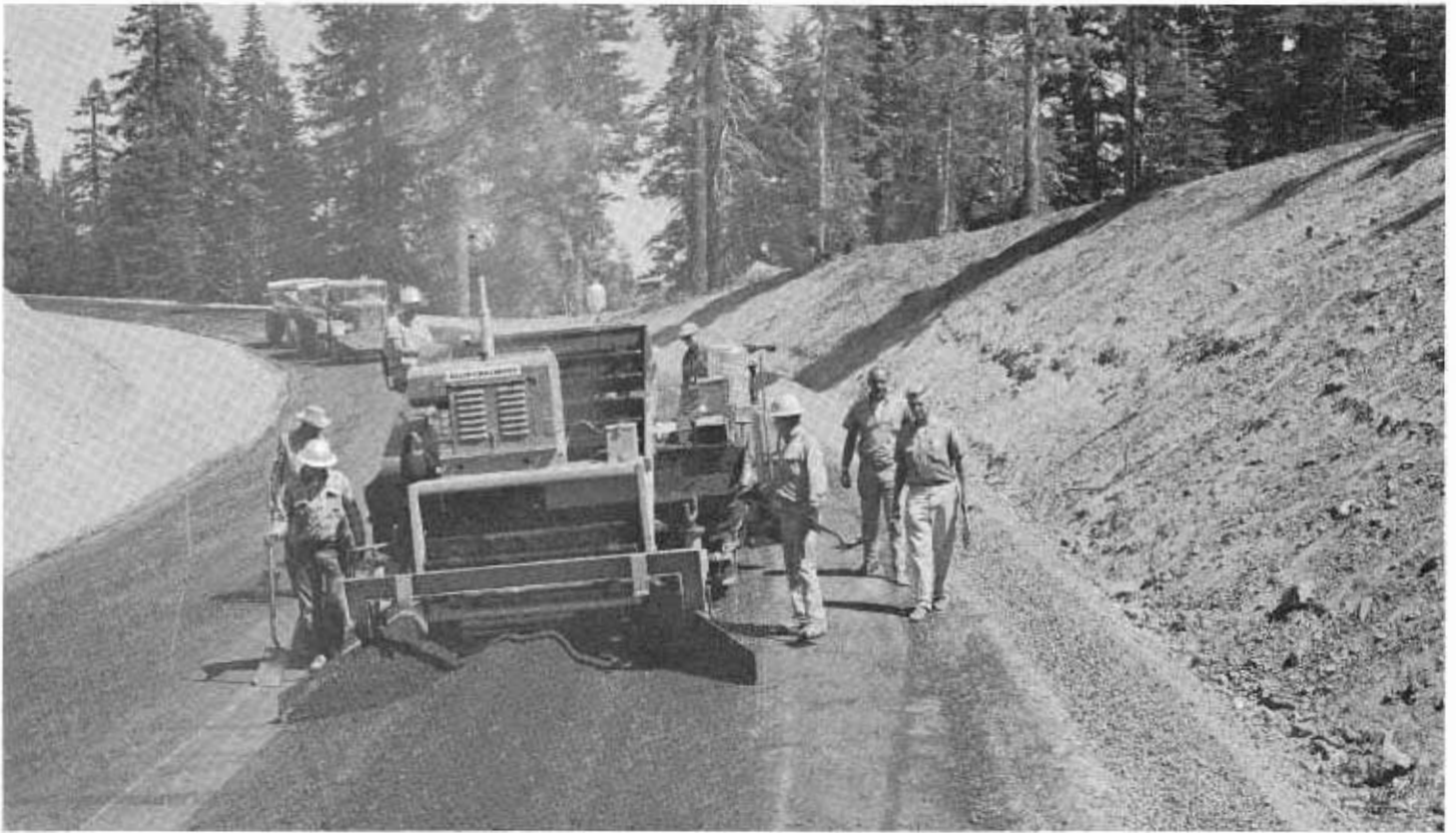
An asphalt spreader (foreground) and a bottom-dump truck add finishing touches to the new roadway between Peddler Hill and Tragedy Springs.
