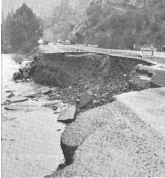
Road destruction may be from several causes. This photo on US 101 in Mendocino County shows the effect of undercutting by a parallel stream.
