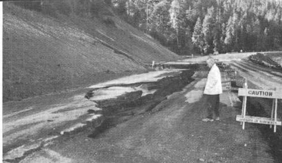
Another kind of damage occurred when underground waters, seeping through fill, washed out part of road foundation.
