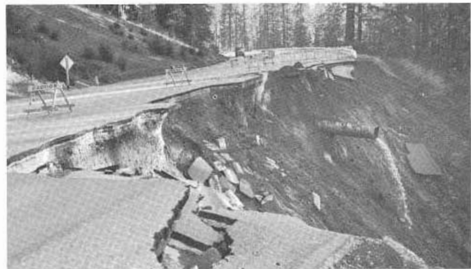
BELOW: This photo shows one of the few places where damage occurred on the Redwood Parks Freeway, resulting in the loss of two lanes. Culvert became plugged and stream went over pavement, "eating back" by washing out slope on outside.
