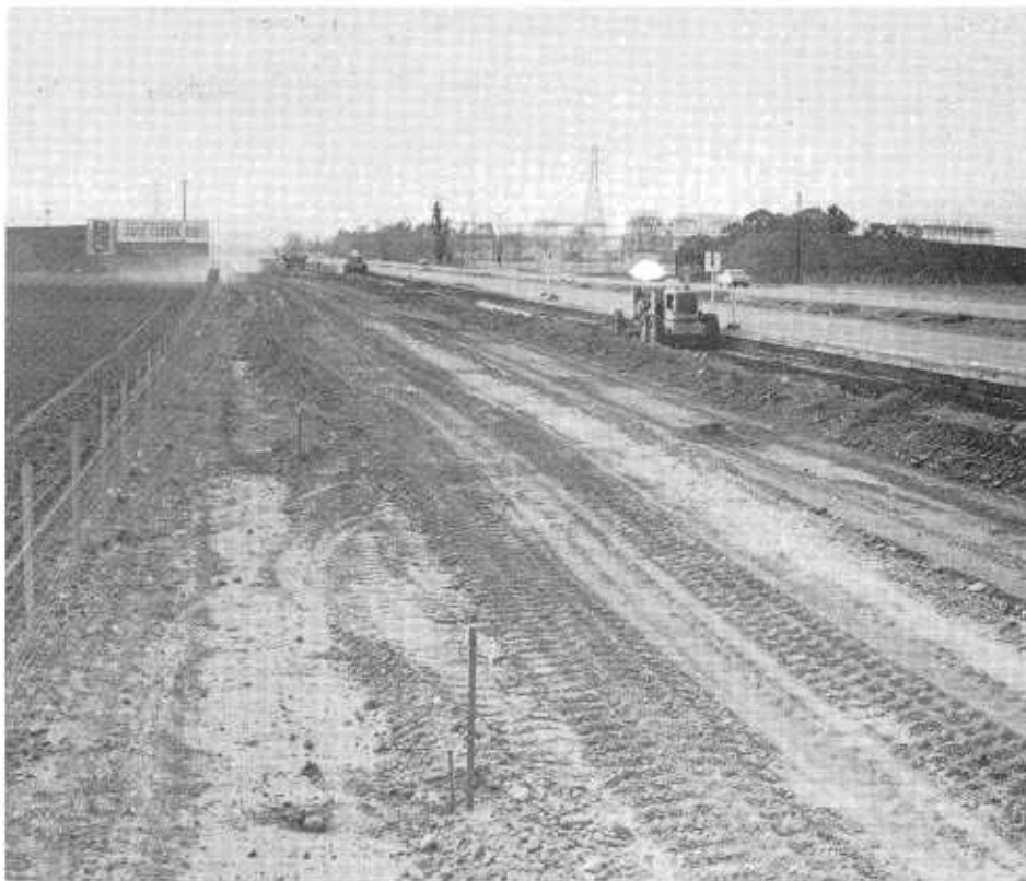
Construction on Interstate 80. The dirt fill (middleground) is the Meridian Road overcrossing. In the background is the P.G. & E.'s Vacaville substation.
