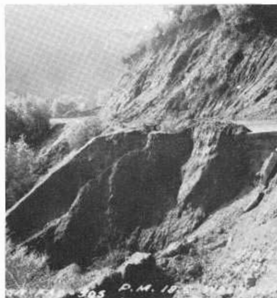
Typical damage to county road, Humboldt County.
