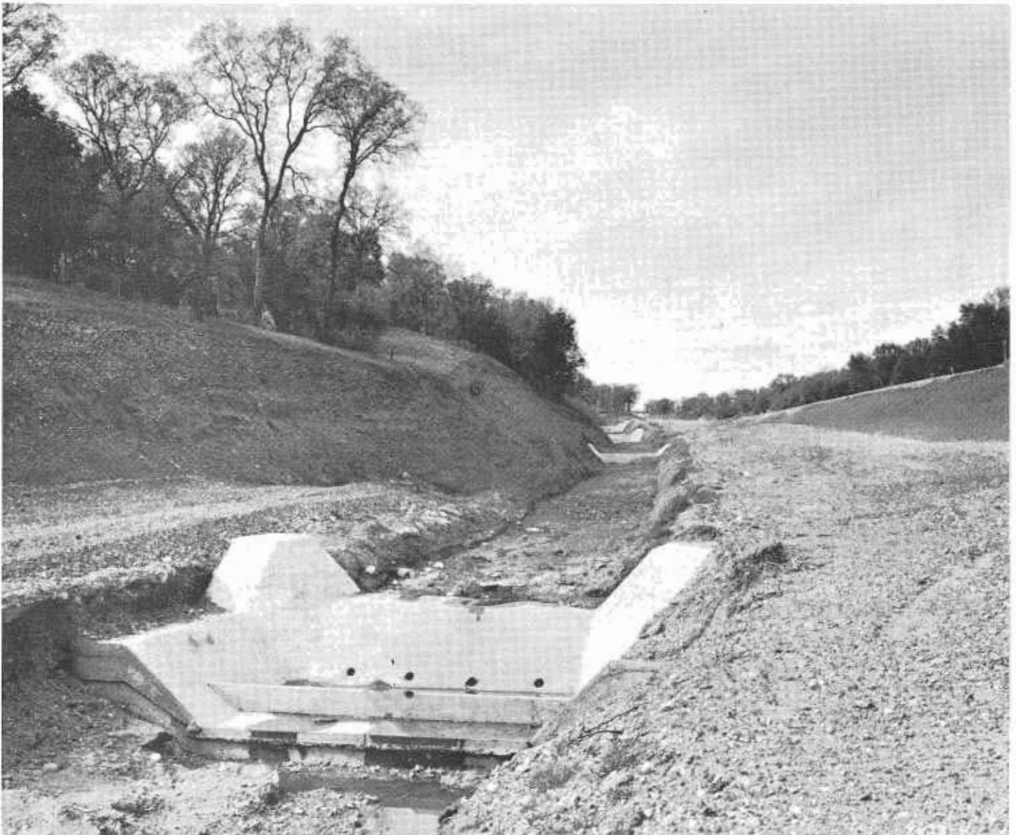
A series of these spillway checks were constructed in a 12-foot bottom channel near the south end of the project. Southbound lanes of the freeway are to the right.
