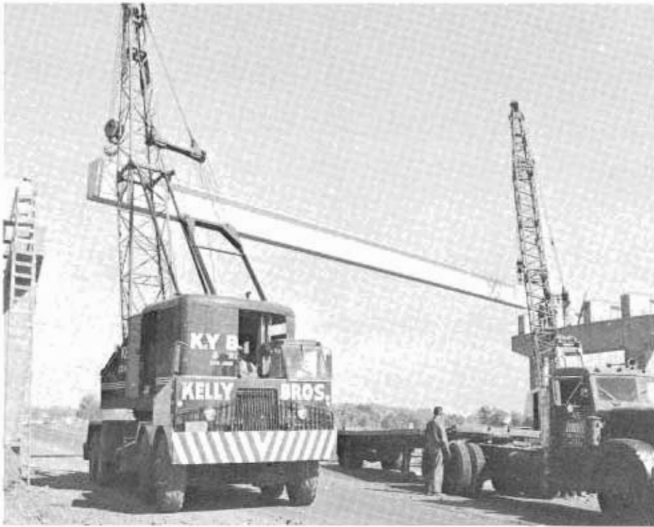
A 30-ton precast prestressed concrete girder is installed at Bowman Road Interchange, south of Cottonwood.
