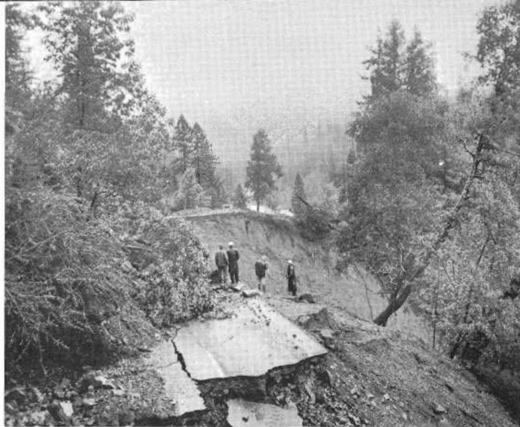
Gaping washout from what is normally an insignificant trickle of a stream is typical of damage throughout the several northwestern counties in the December 1964 floods. This is State Route 208 in Mendocino County, west of Leggett.
