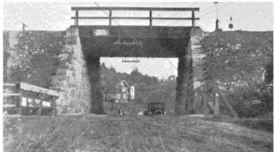
This photo of the old East Auburn Underpass is dated December 15, 1914. The view is eastward.
