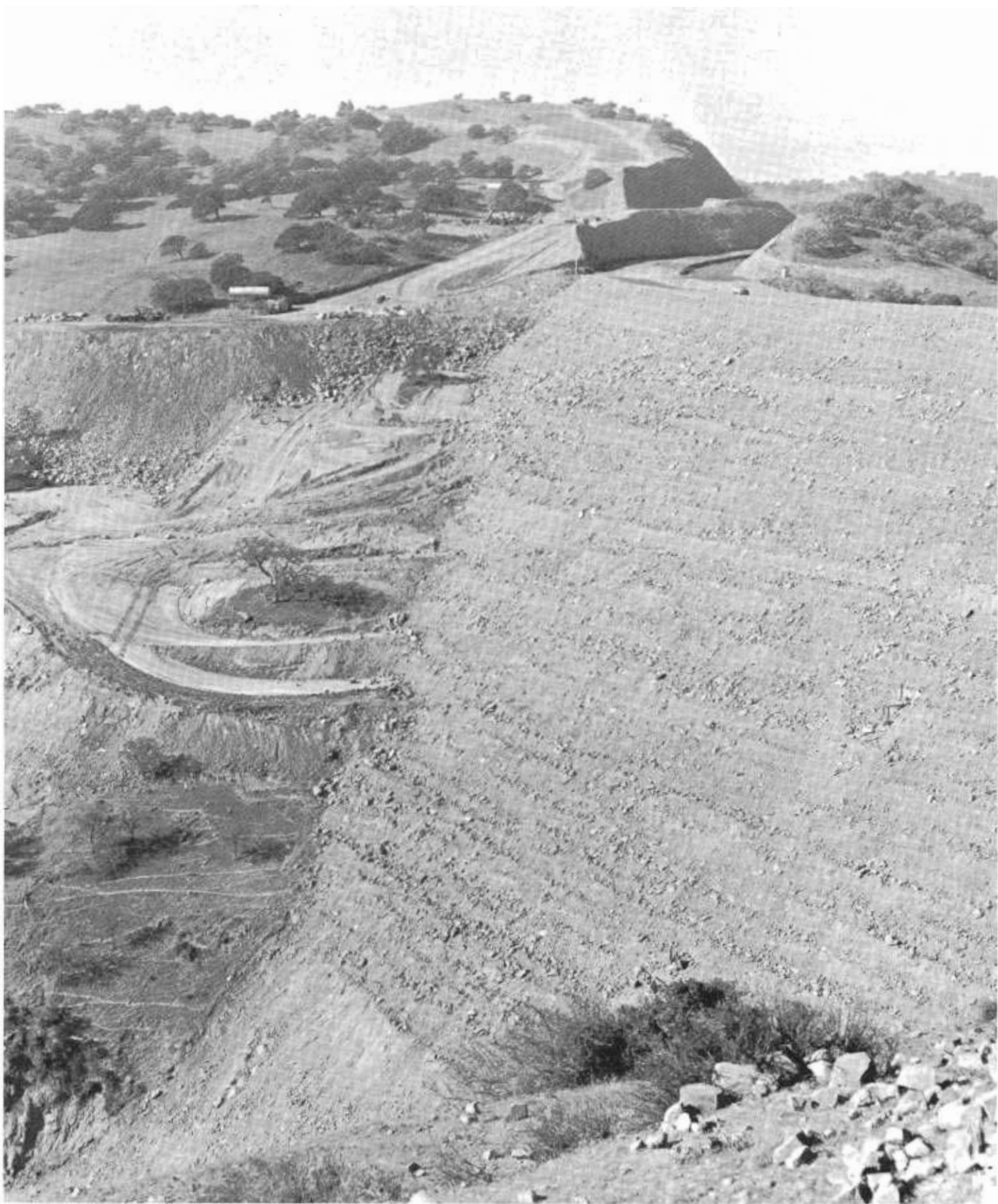
At rough grade level, the "Big Fill" dwarfed the car at the top right.
