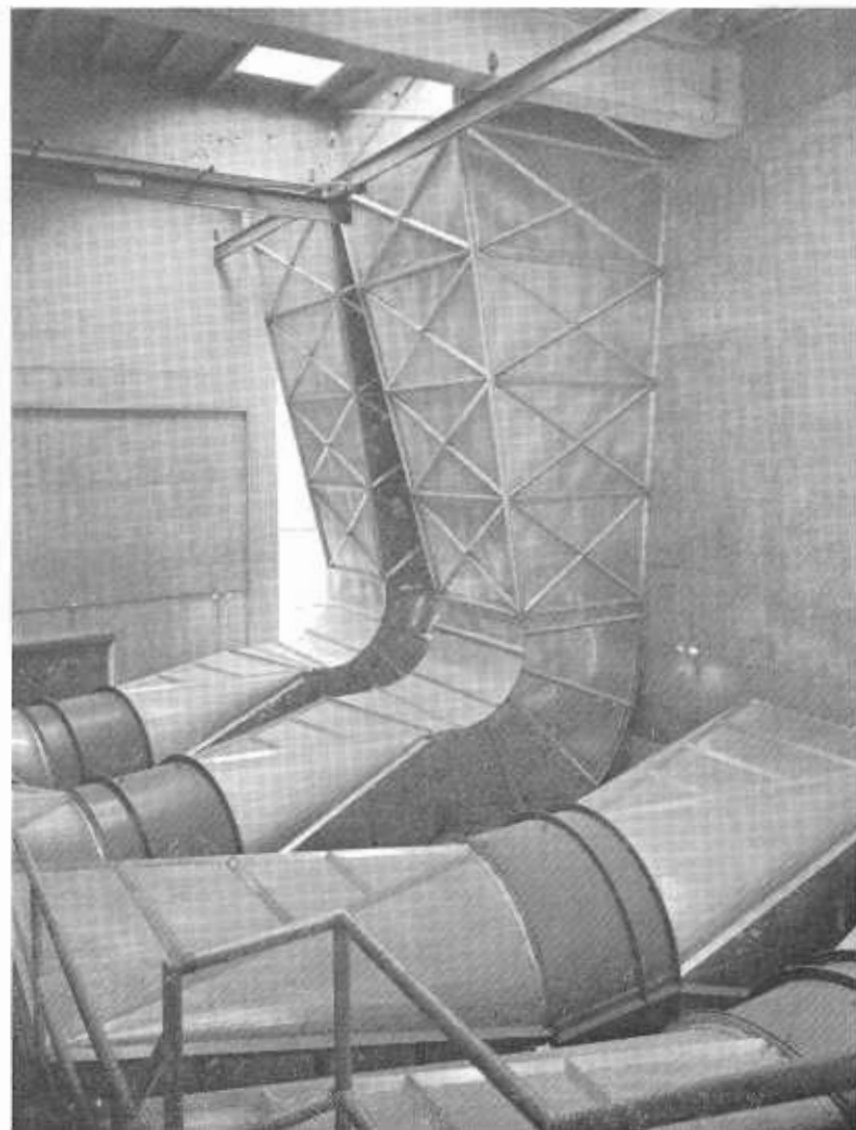
These massive exhaust ducts take the "used" air from the tunnel and arrange for its disposition straight up into the atmosphere.
