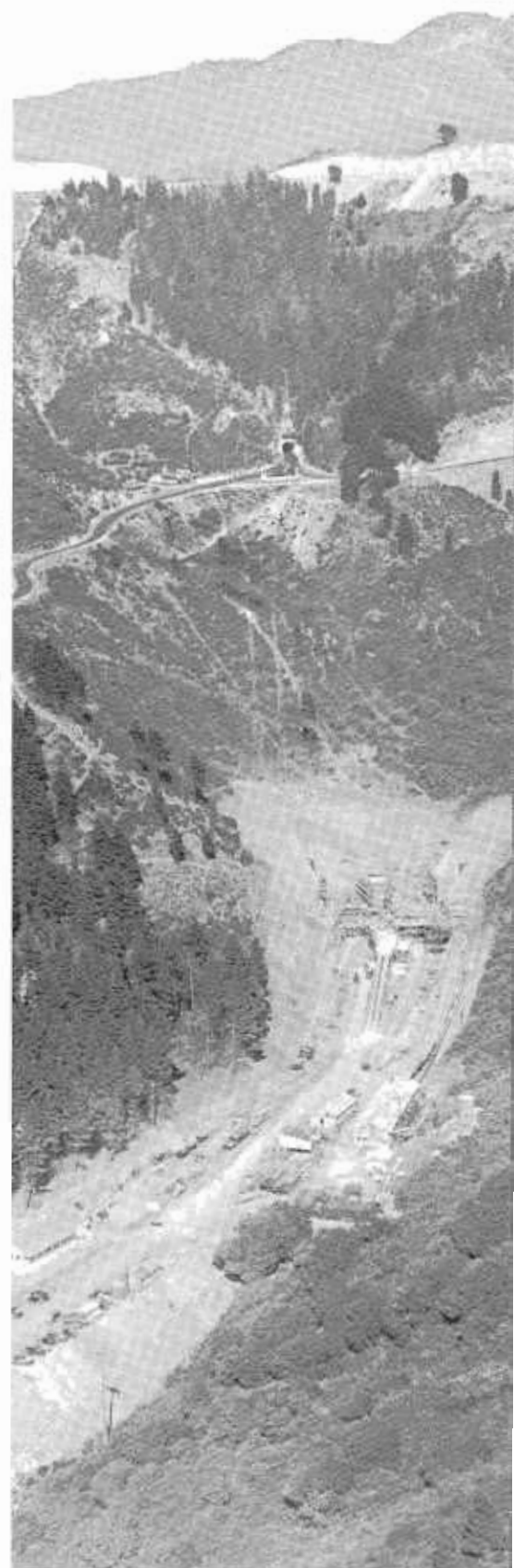
Taken September 1, 1934, this photograph shows construction on the first low-level tunnels as well as the old tunnel (at top center) built at the turn of the century.
