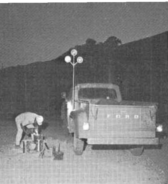
Compaction tests were performed at night to help meet the time limitation on the project.
