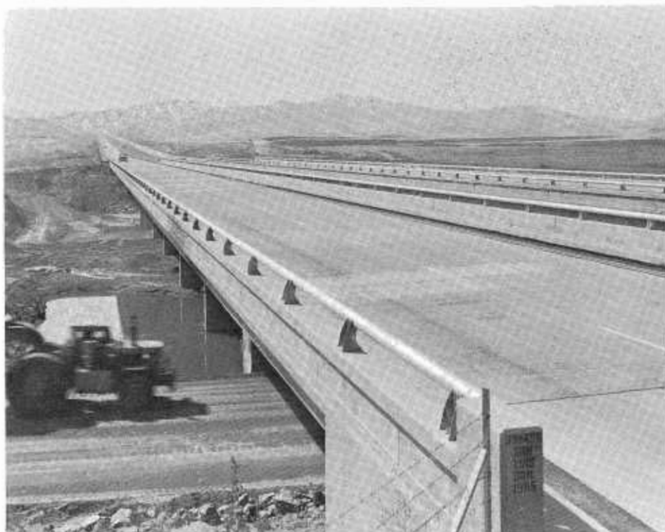
Twin bridges cross the San Luis Forebay channel. The roadway under the bridge will be inundated when heavy equipment used to construct the dam is no longer needed.
