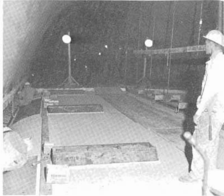
Tiling operations mark the beginning of a more finished appearance for the tunnel.
