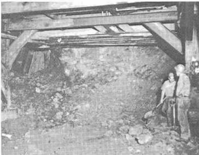
(Above) Working under the protection of the jumbo, construction personnel find that the shovel is still in style for excavation operations.
