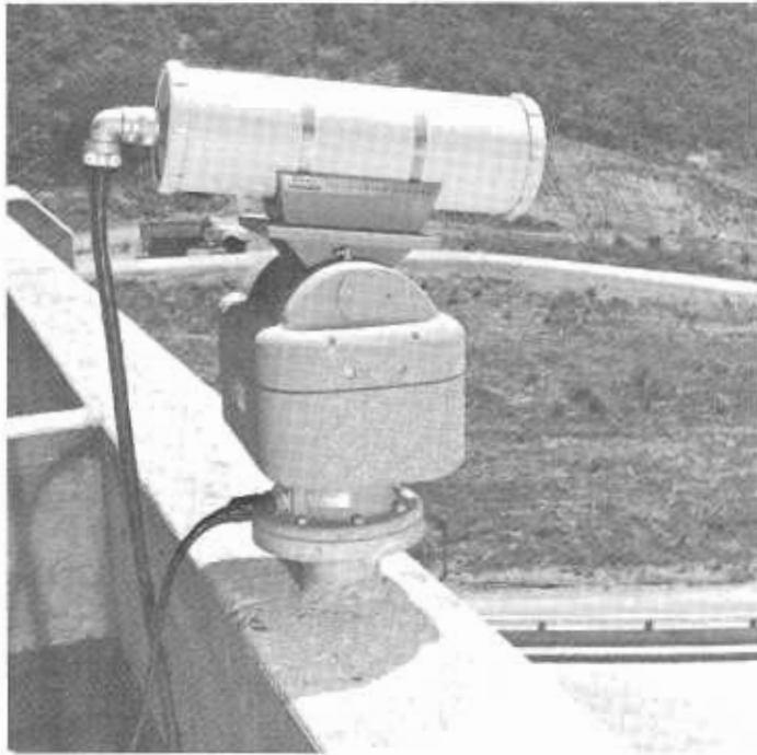
A television camera, mounted at portal top, monitors traffic heading for the tunnel. The resulting "commentary" is watched from the control room to alert the staff of emergencies and/or the need for lane control.
