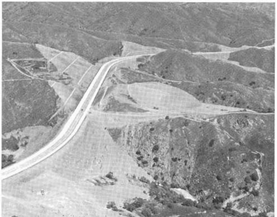
The "Big Fill" is over 280 feet high and the "Big Cut" is over 300 feet deep.
