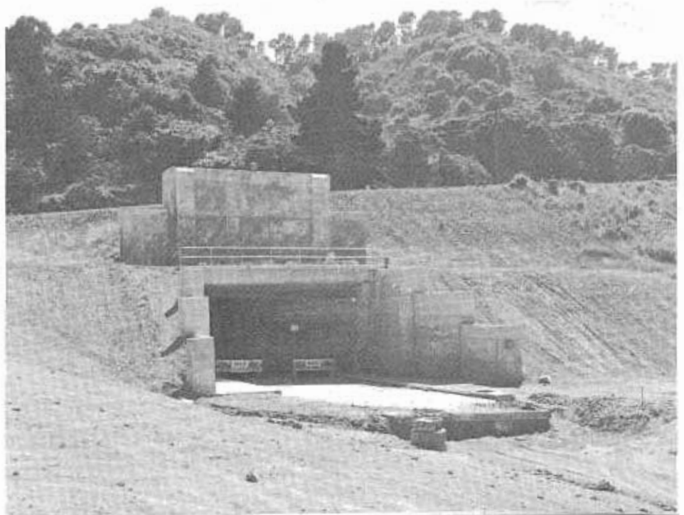
The third tunnel as it looked in the later stages of construction.
