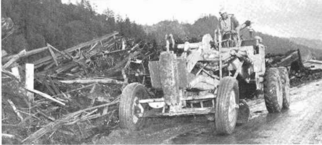
Grader is engaged in cleaning silt and debris off Redwood Highway four-lane section south of Fortuna.
