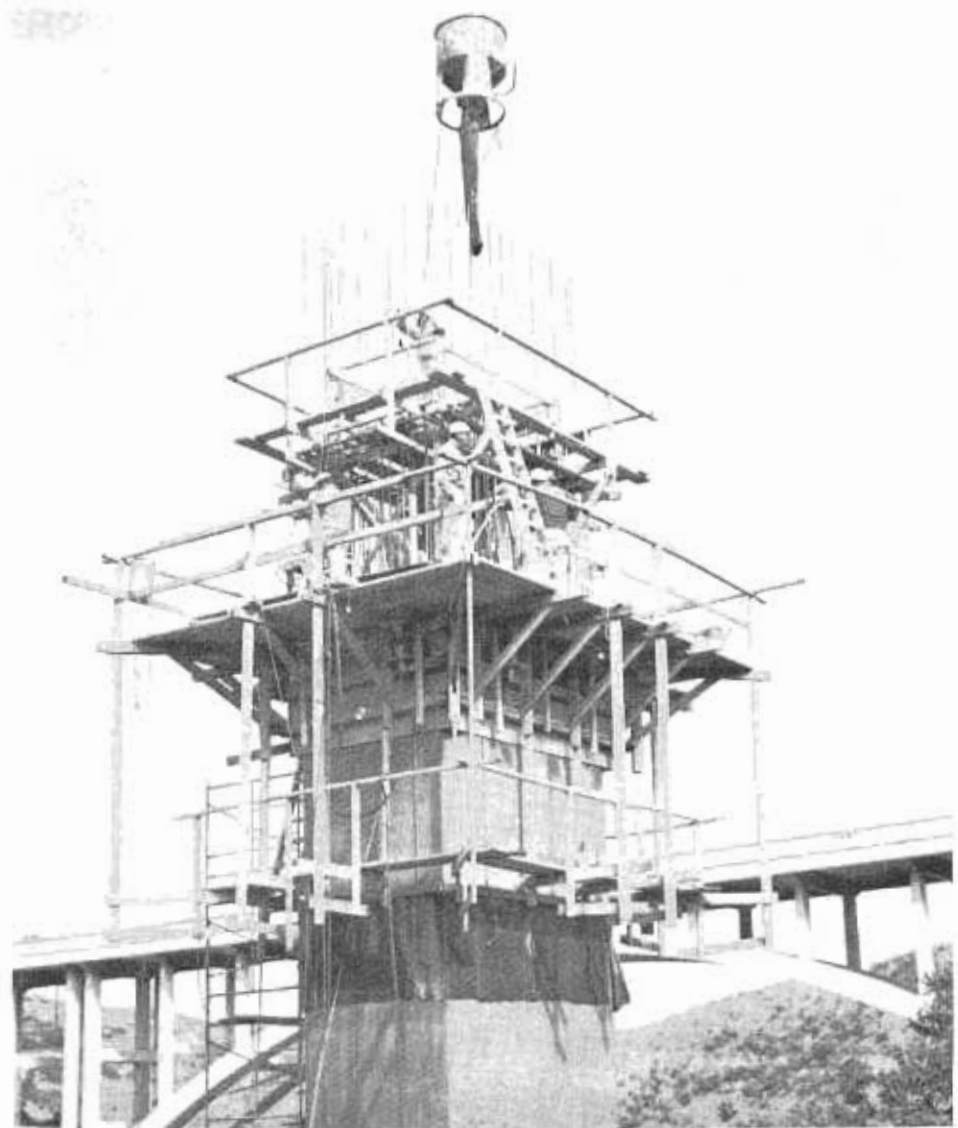
A continuous concrete pour on the new Penasquitos Creek Bridge with slipforms. Existing two-lane arch bridge is in the background.
