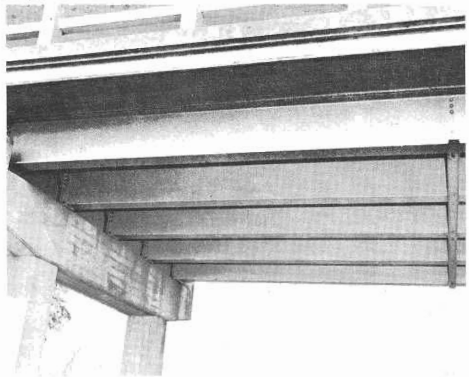
FIGURE 4—Condition of paint system No. 4 applied in 1958 after six years' service. This is the same area as shown in Figure 3. The condition in Figure 4 is typical of system No. 4.
