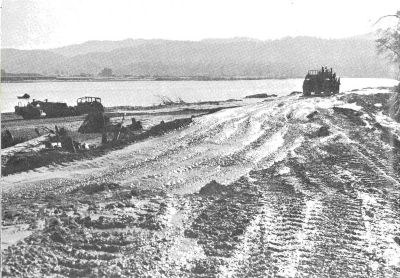
At right DW-21 loaded with gravel is proceeding to fill point, and at left tractor pushes another unit as it scrapes material from river bar, rebuilding road after Christmas 1964 flood. Scene is along lower Eel River, and some of material being replaced as road base probably previous to flood was road base farther upstream!
