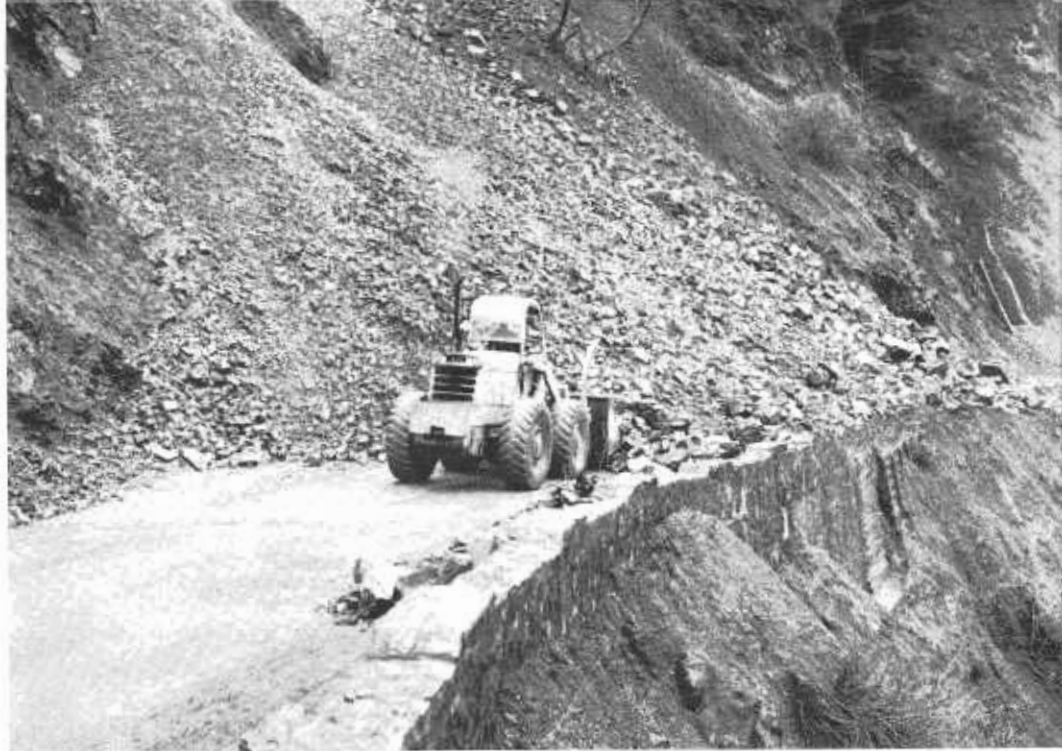
Small slide such as this on precipitous section of Route 299 can be handled by front-end loader and few trucks. This material is good for subbase and will be used for fill.
