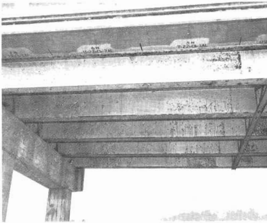
FIGURE 3—Condition of average paint system applied in 1952 after six years' service.
