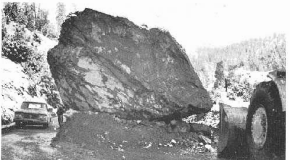
Boulder which slid down mountainside onto Route 299 must be broken up by blasting before removal.
