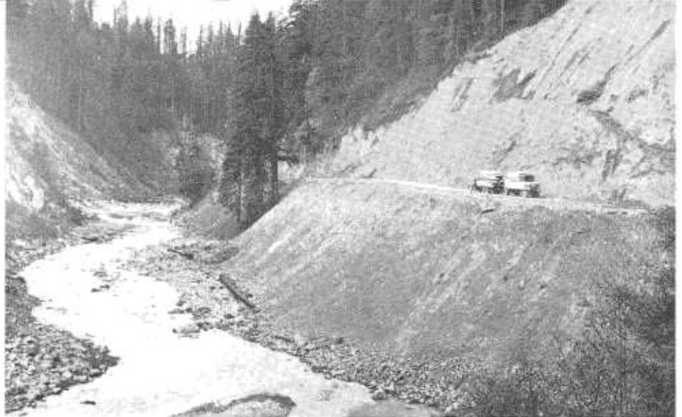
Reconstructed Sign Route 36 in Van Duzen River Canyon. Height and extent of raw slopes indicate amount of undercutting by stream in flood.
