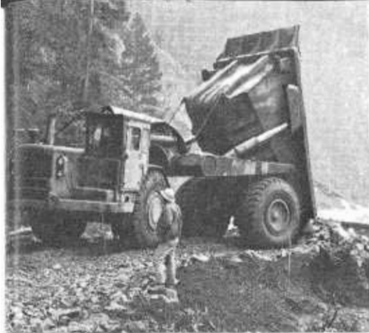
Fortunately, several contractors already had big rock trucks such as this in the vicinity, and they were invaluable in replacing road base.
