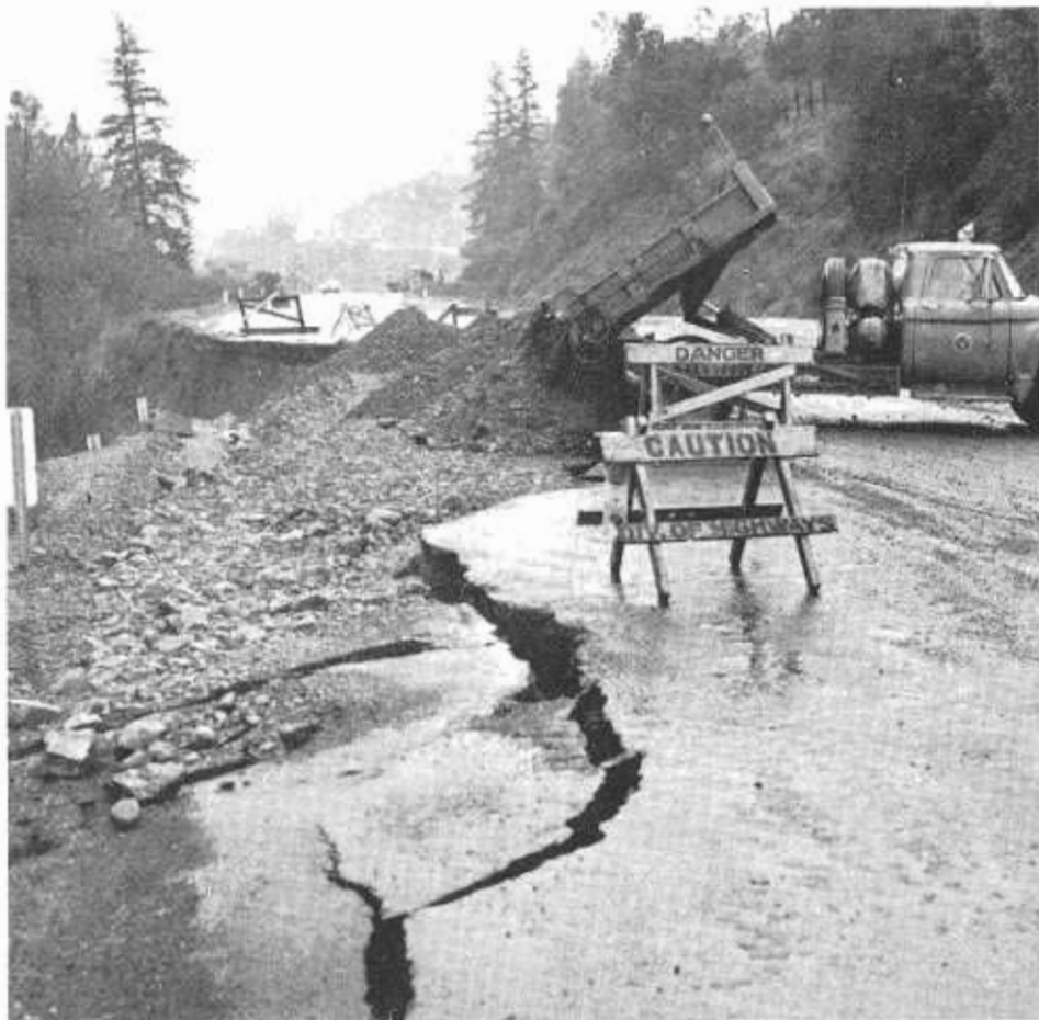
ABOVE: Amount of fill required to repair such slipouts was dependent upon how far down "toe" of slope lay. BELOW: Grader, front-end loader, and dump trucks work together to remove silt in Orick, several feet deep in places, as can be seen beyond highway shoulder.
