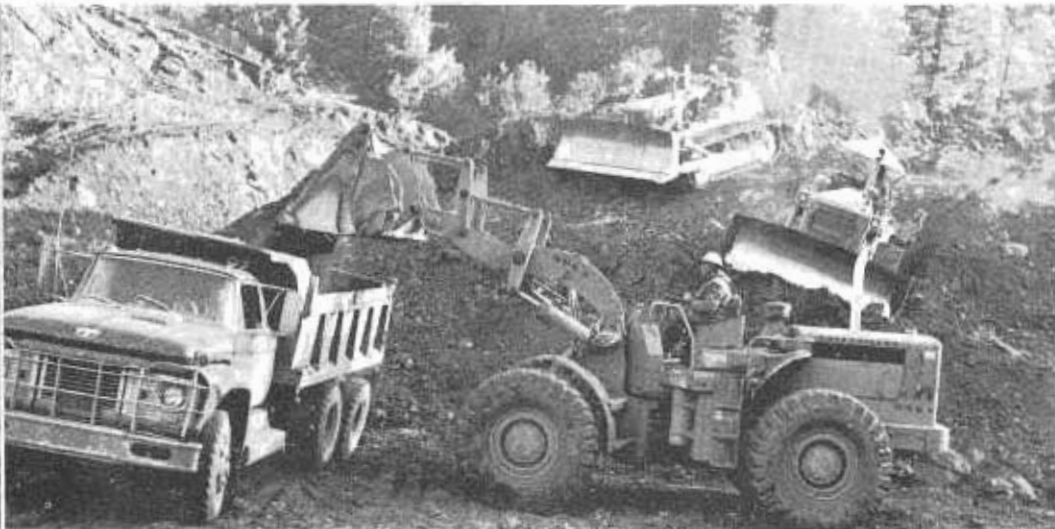
Front-end loader, assisted by tractors equipped with both blades and rippers, keeps stream of material flowing in trucks from "borrow" site selected to provide fill for washed-out sections.
