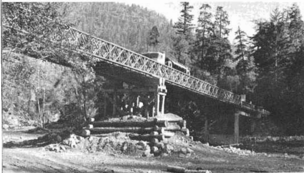
Another Bailey Bridge replacement on US Route 199 across Smith River. This is only one girder high, but can carry legal loads by virtue of center pier.
