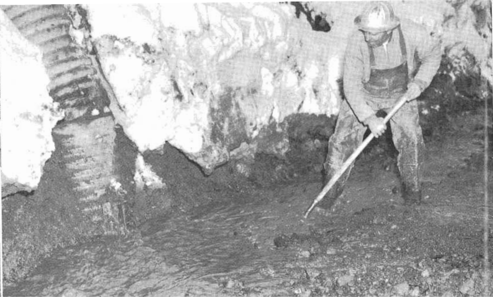
Much of the work of reopening highways after a disastrous storm is like this—wet, cold, and muddy.
