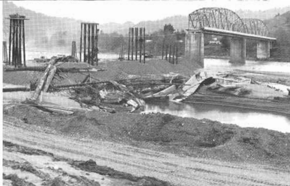
Repairs going forward on Robinson Ferry Bridge over the Eel. Crews gambled stream would not flood again this winter, and as payoff bridge will be opened to traffic in May. Wreckage of old spans lies in center foreground.
