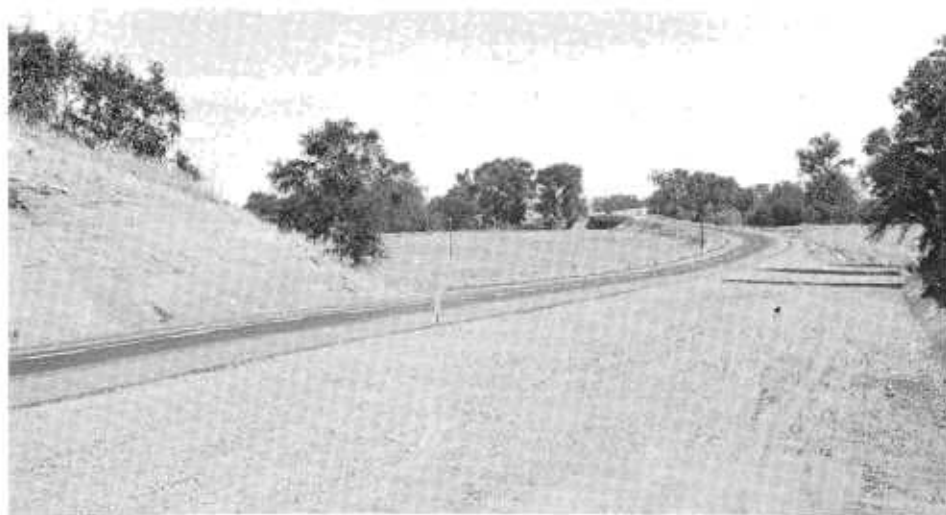
The Dillard Road reconstruction looking north toward the bridge over the Cosumnes River in the distance. Grading for future addition of northbound lanes can be seen to the right of the roadway.
