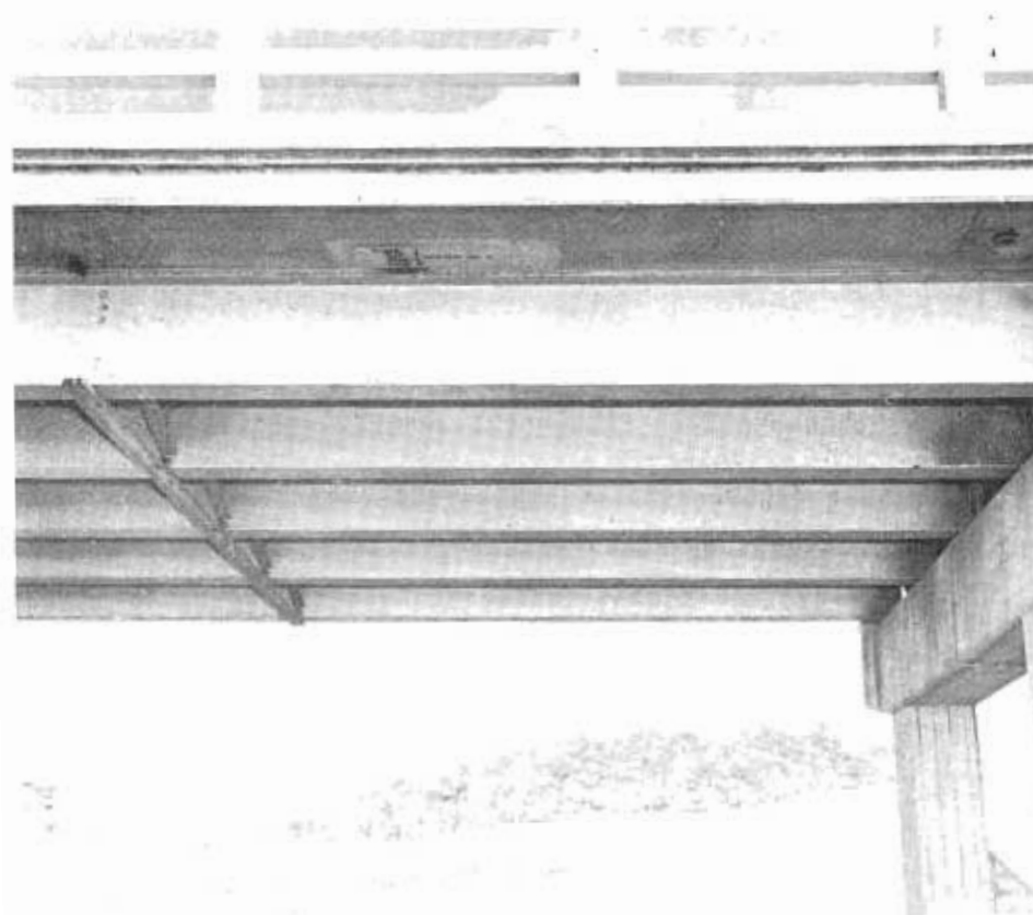
FIGURE 6—Typical condition of paint of system No. 2.
