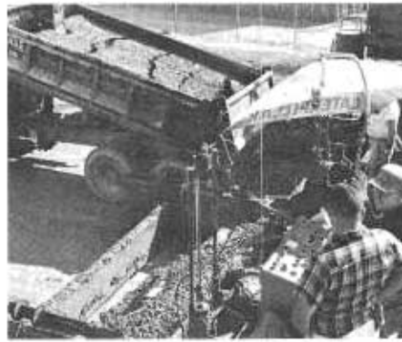
Central mix concrete is deposited in slipform paver, thus expediting construction of Garden Grove Freeway. This section of freeway—from Harbor Boulevard to Haster Street—is now complete.
