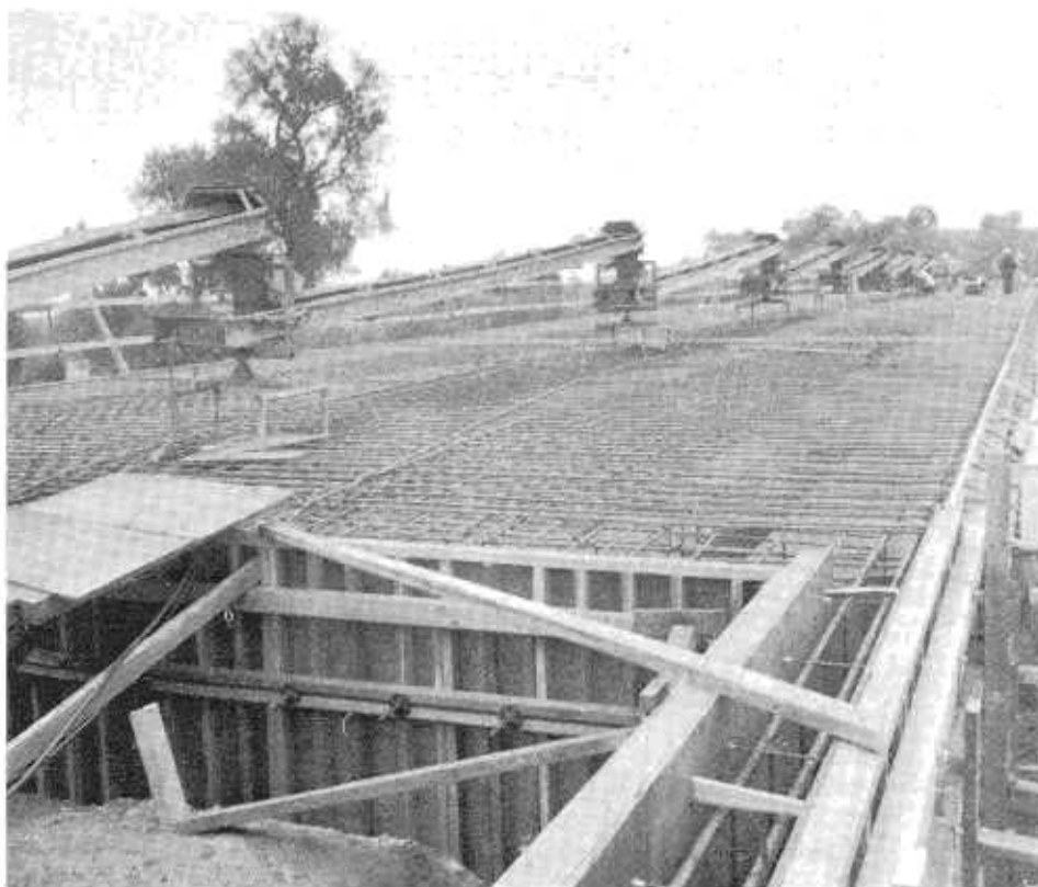
To simplify placement of concrete for the superstructure, the contractor resorted to an elaborate portable conveyor belt system.
