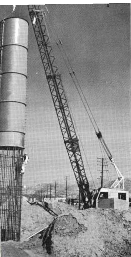
A massive bridge column form dwarfs construction men at work building the Long Beach-Pomona Freeway Interchange. When completed in the fall of 1966, this structure will be the second four-level interchange in Los Angeles.
