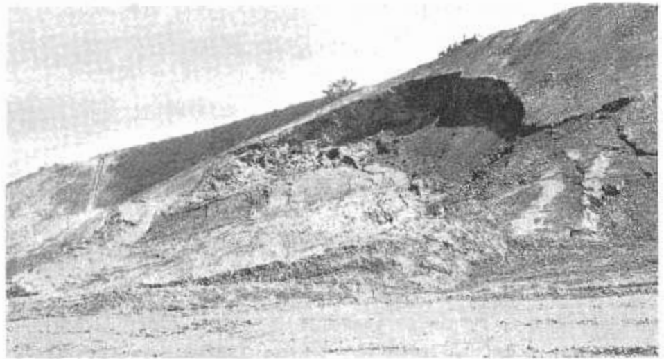
The east face of the "Big Cut" on Unit 1 construction showing the 100,000-cubic-yard slide after the third and final phase.
