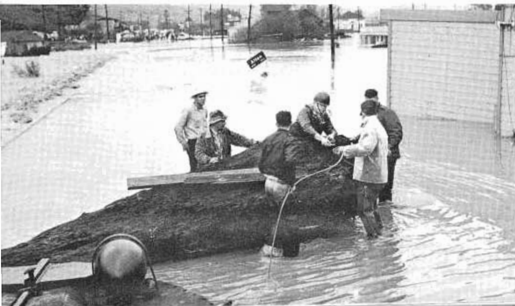
BELOW: Workers from various agencies clearing highway on Christmas Day. This is State Route 36 at Alton, near its western terminus. (Photo courtesy Eureka Newspapers, Inc.)
