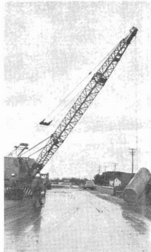
Crane removes logs washed up on undamaged section of county road near Ferndale in order to use it for detour for Redwood Highway.
