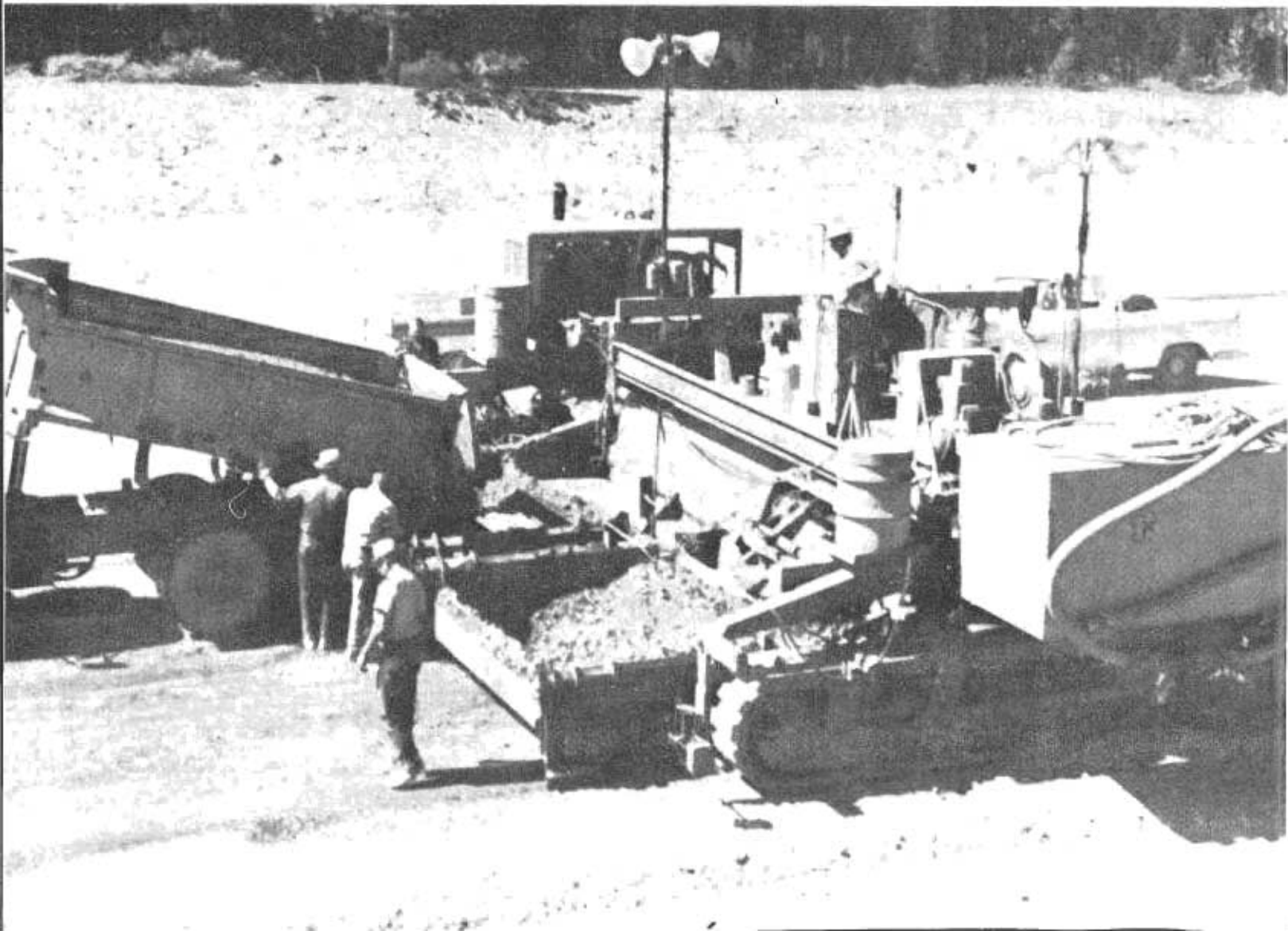
FIGURE 9—The sliding front plate on the slipform paver can be seen just to the right of the three men in the photo below.
