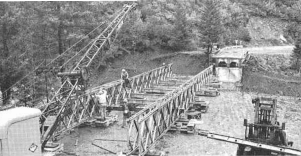
First girders of Bailey Bridge being assembled to cross Smith River on US 199. As sections are joined they are pushed out over opening by rollers set on the little platforms. (This is bridge seen on back cover.)
