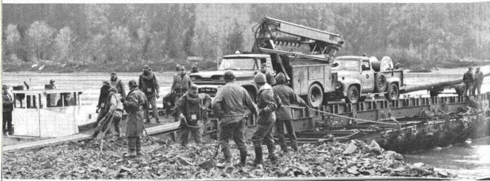
Pontoon ferry landing with load of emergency utility repair vehicles borrowed from Oregon early in January. Ferry had been operating only a few days at this time. High water and current were serious problems.
