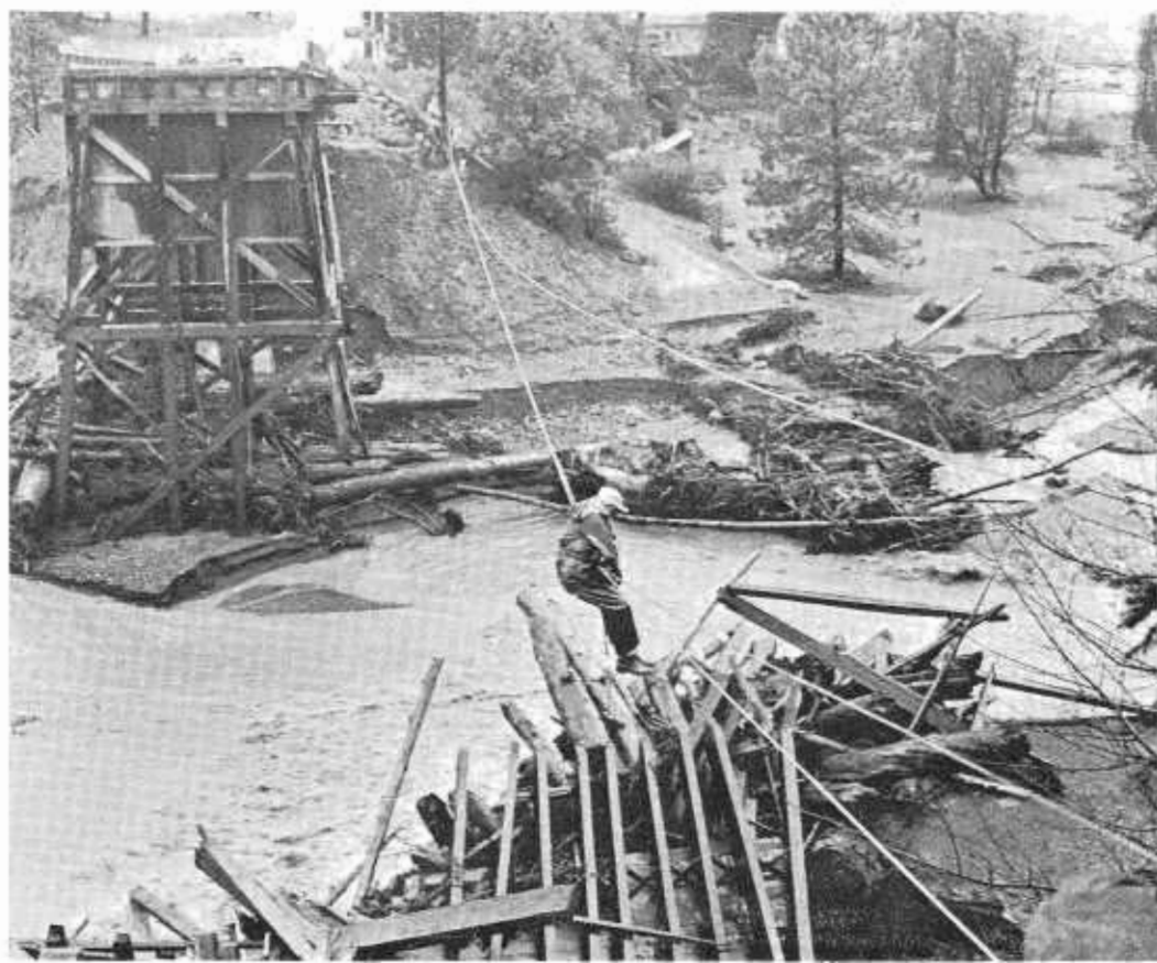
Breeches buoy rigged at Willow Creek Bridge to carry people across during first days of recovery after flood. Note debris and silt left by receding stream. (Photo courtesy of Eureka Newspapers, Inc.)
