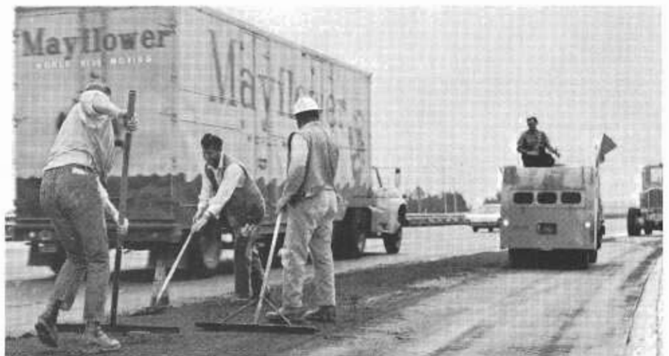
A maintenance crew does patching work on the Eastshore Freeway in Alameda County.
