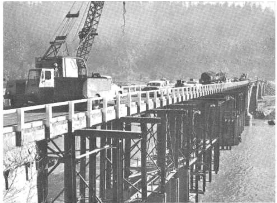
The Klamath River south span repairs shortly after the bridge was opened to traffic in March 1965. The span was washed out during the December 1964 floods. Contractor's crews are completing the timber sheathing of the pile bents to protect them from floating debris. (See next photo.)
