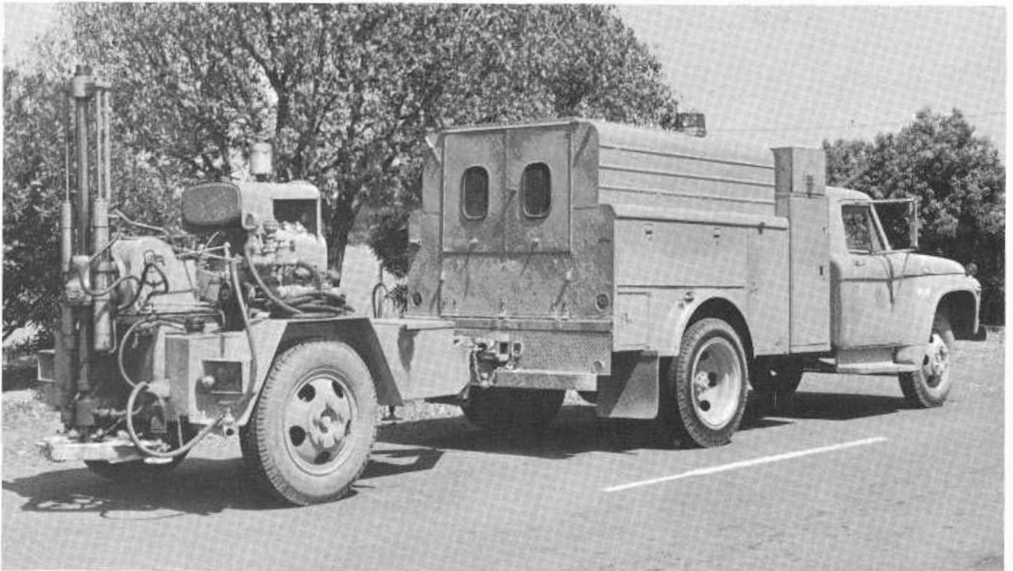
Mobile coring machines like the one shown here are used for cutting cores up to 12 inches in diameter from finished roadways to check compliance of the as-built roadway against the specifications.
