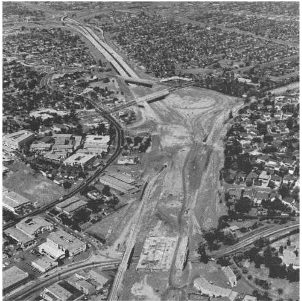
Completion of the Santa Monica Freeway, shown above under construction, will provide West Los Angeles with its first east-west freeway.
