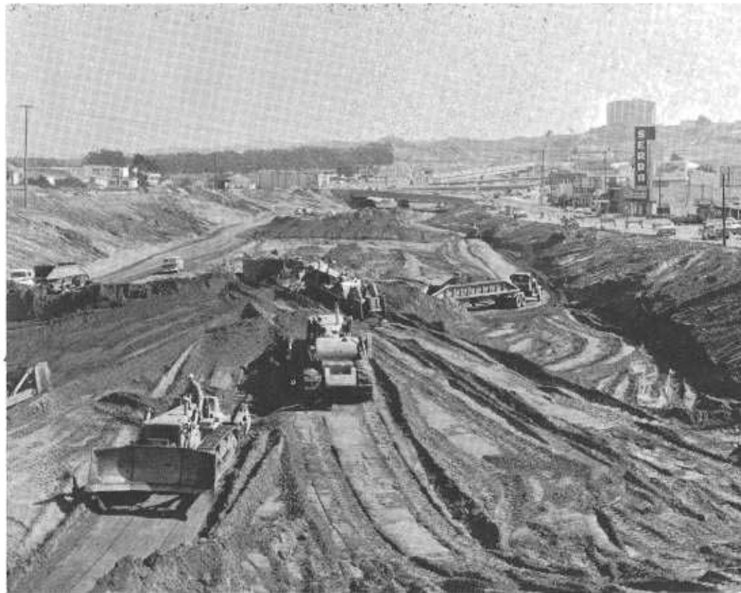
The Junipero Serra Freeway (Interstate 280) under construction between Eastman Avenue and Orizaba Avenue south of San Francisco.
