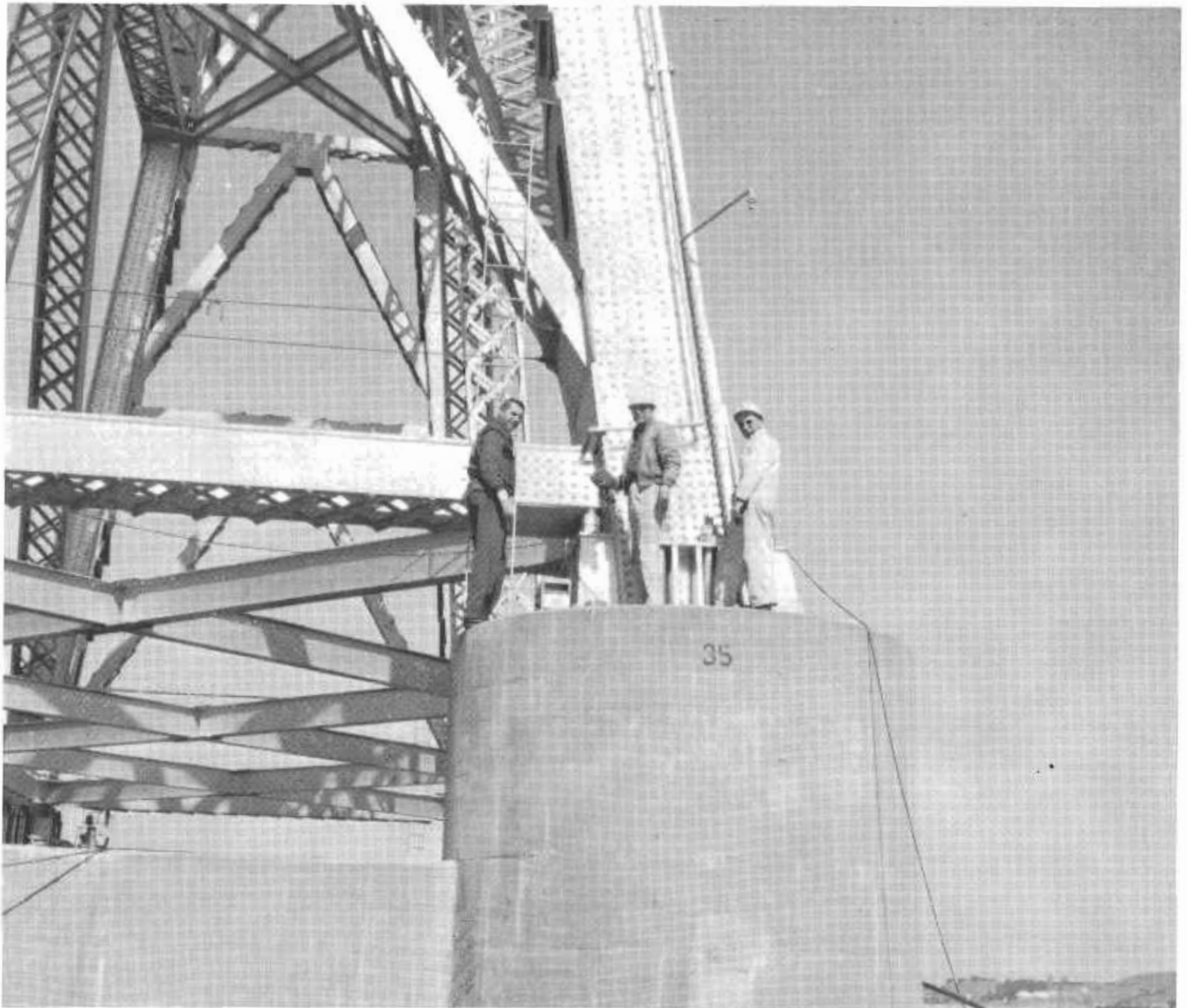
Using ultrasonic equipment, a Division of Highways crew checks the anchor bolts of the Richmond-San Rafael Bridge which were feared to have been damaged when a ship collided with the bridge pier.
