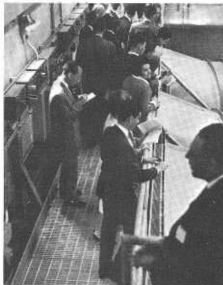
FOREIGN VISITORS. French engineers inspect fanroom controlling ventilation in the Caldecott Tunnel.
