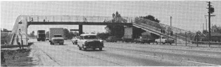
New in-the-railing fluorescent lighting fixtures are being installed on pedestrian overcrossing structures. The new fixture eliminates lighting poles (see next photo) and improves the appearance of the structure.
