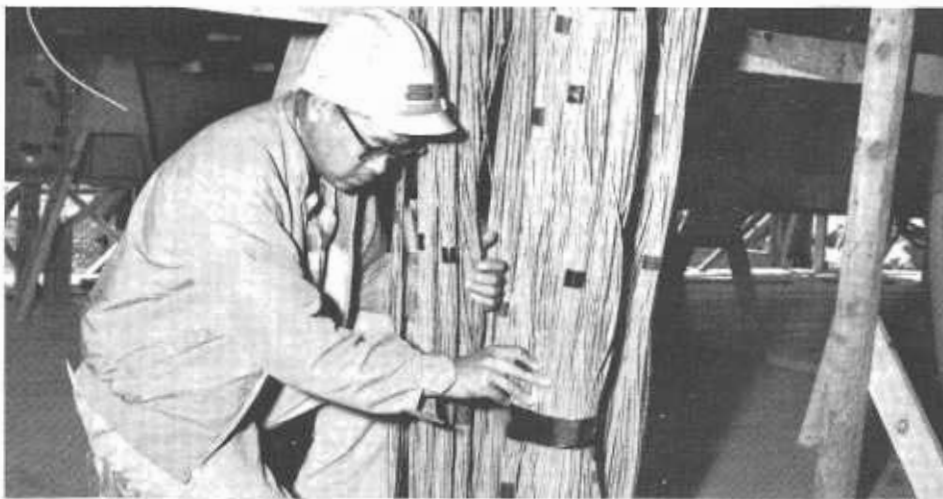
An electrical engineer checks some of the 30 miles of cable necessary to instrument an orthotropic bridge for research purposes.
