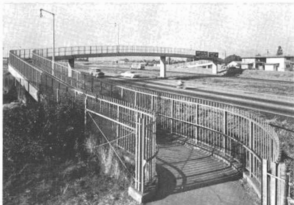
This pedestrian overcrossing on the Highway 99 Freeway through Sacramento shows the old-style lighting poles on the structure which are being replaced by new in-the-railing fixtures. (See previous photo.)
