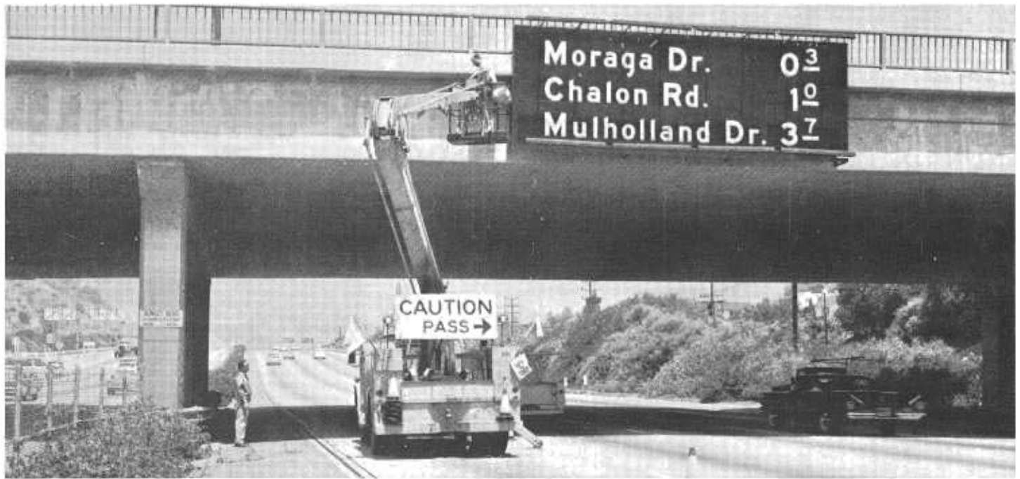
A maintenance crew use a giraffe and personnel hoist to make sign repairs on the San Diego Freeway in Los Angeles.
