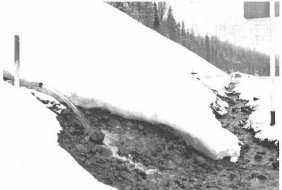
Heavy ground water runoff through one of the horizontal drains near the Whitmore slide area in Interstate 80. The drains were successful in preventing further earth movement and damage to the roadway. Previously, slides induced by excessive trapped water had caused complete failure of the roadway.
