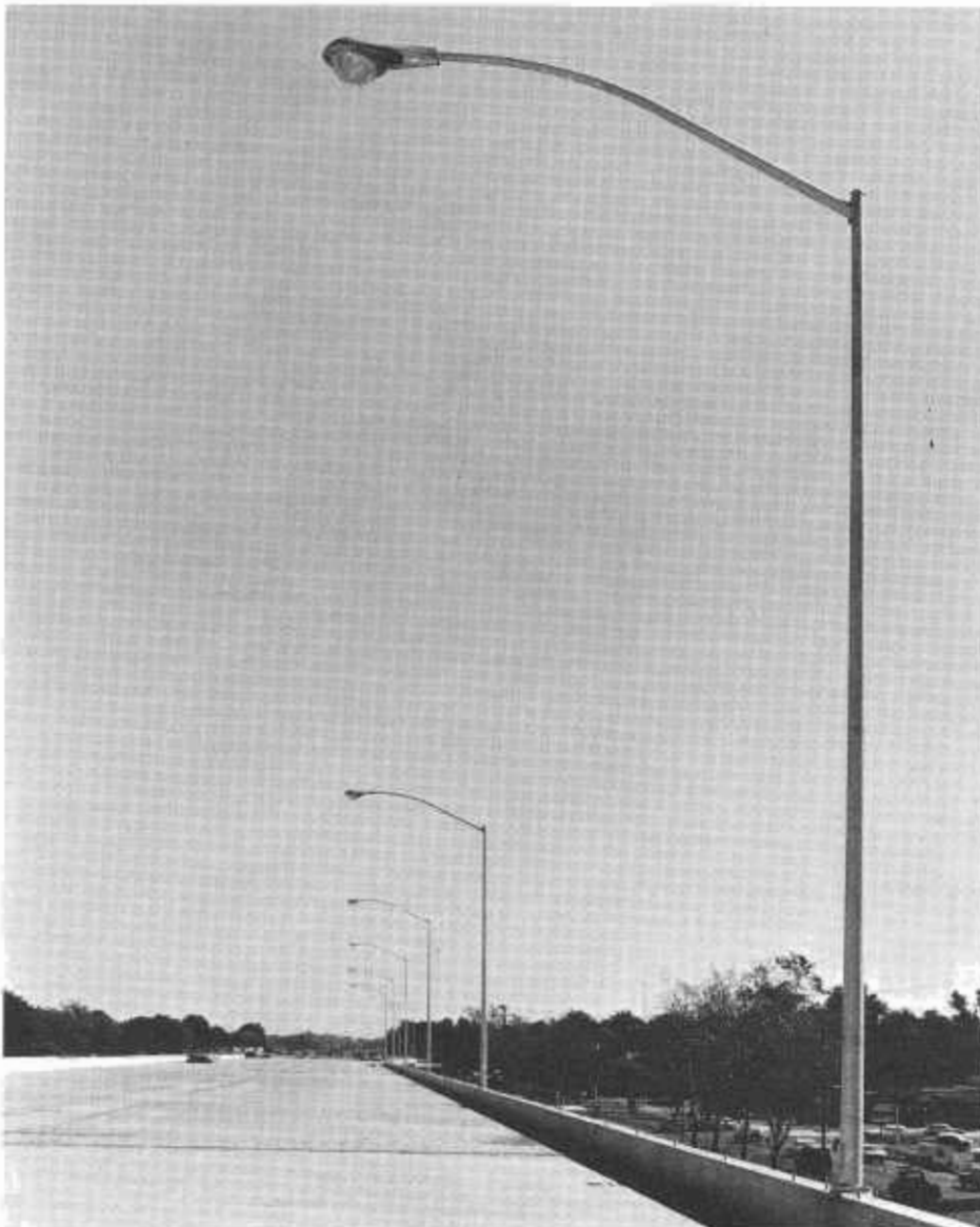
The mastarm for newly designed lighting standards on freeways is a tapered curve which improves the overall aesthetics of the freeway. The standards in the photo are being installed on Interstate 80 through Sacramento.
