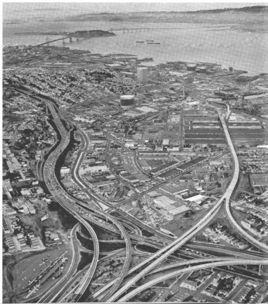
An extension of the Route 82 (southern) Freeway in San Francisco is shown under construction toward the site of an interchange near Islais Creek with the future freeway via Hunters Point. The section shown under construction will connect with the Embarcadero Freeway at the San Francisco-Oakland Bay Bridge.
