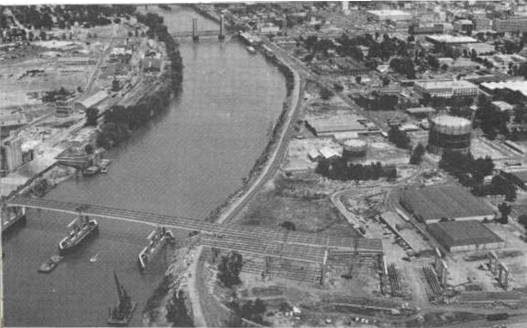
The bridge shown at bottom under construction across the Sacramento River will carry I-80 traffic between Yolo County (left) and the W-X Street extension of this route in Sacramento, to the 29th-30th Street construction, scheduled for completion by late 1966.
