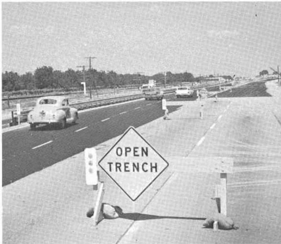
High speed detours were well posted and the double-blocked-out median barrier protected motorists against oncoming traffic.
