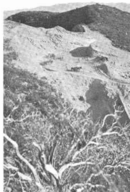
Four-horse Fresno scrapers gnaw their way through the mountains for the original Ridge Route in this photo taken June 24, 1915.
