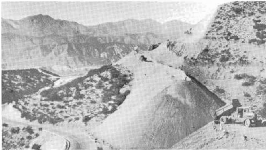
Construction near Cajon Summit in 1930, when the winding old road at the left was replaced on new alignment. A crew of laborers is finishing excavation slopes.
