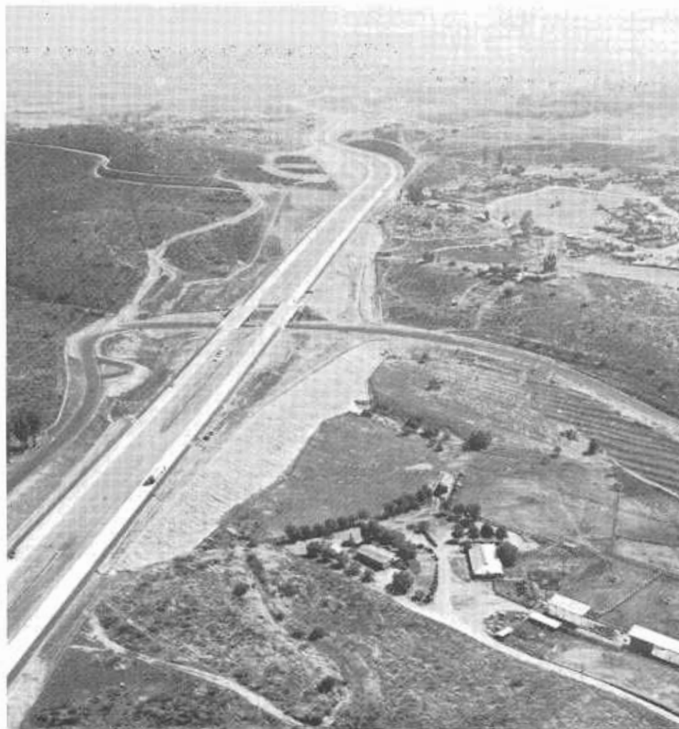
Looking west on Interstate 8 toward the Los Coches Road undercrossing with adjacent grading for a future interchange. Beyond is the Tunnel Hill cut.
