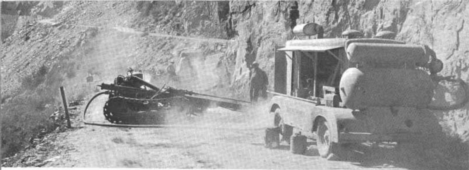
Handling traffic on road while reconstruction was in progress was difficult. Drills had to be moved out of position in cases like this, when traffic passed through.
