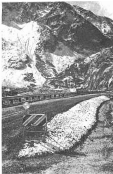
Widened route near Dodge Point here awaits final asphalt surfacing. Note snow on windrow of material which must be applied warm.
