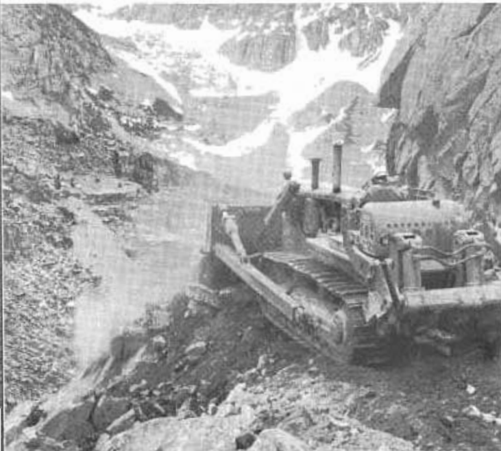
Bulldozer operator here clearing blast debris from right-of-way in Tioga Pass widening operation bears out resident engineer's comment—"They had to be the best equipment operators in the world."
