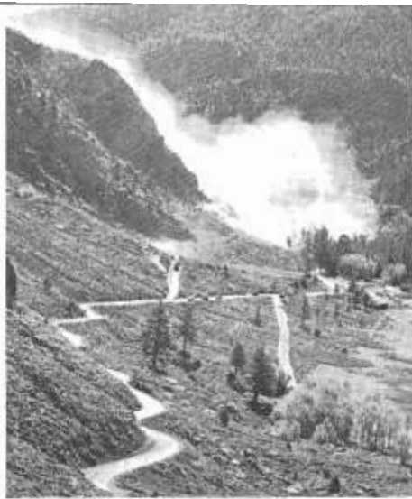
Same view as on left, about a minute after blast. Dust has cleared sufficiently so notch blasted for new right-of-way can be seen.
