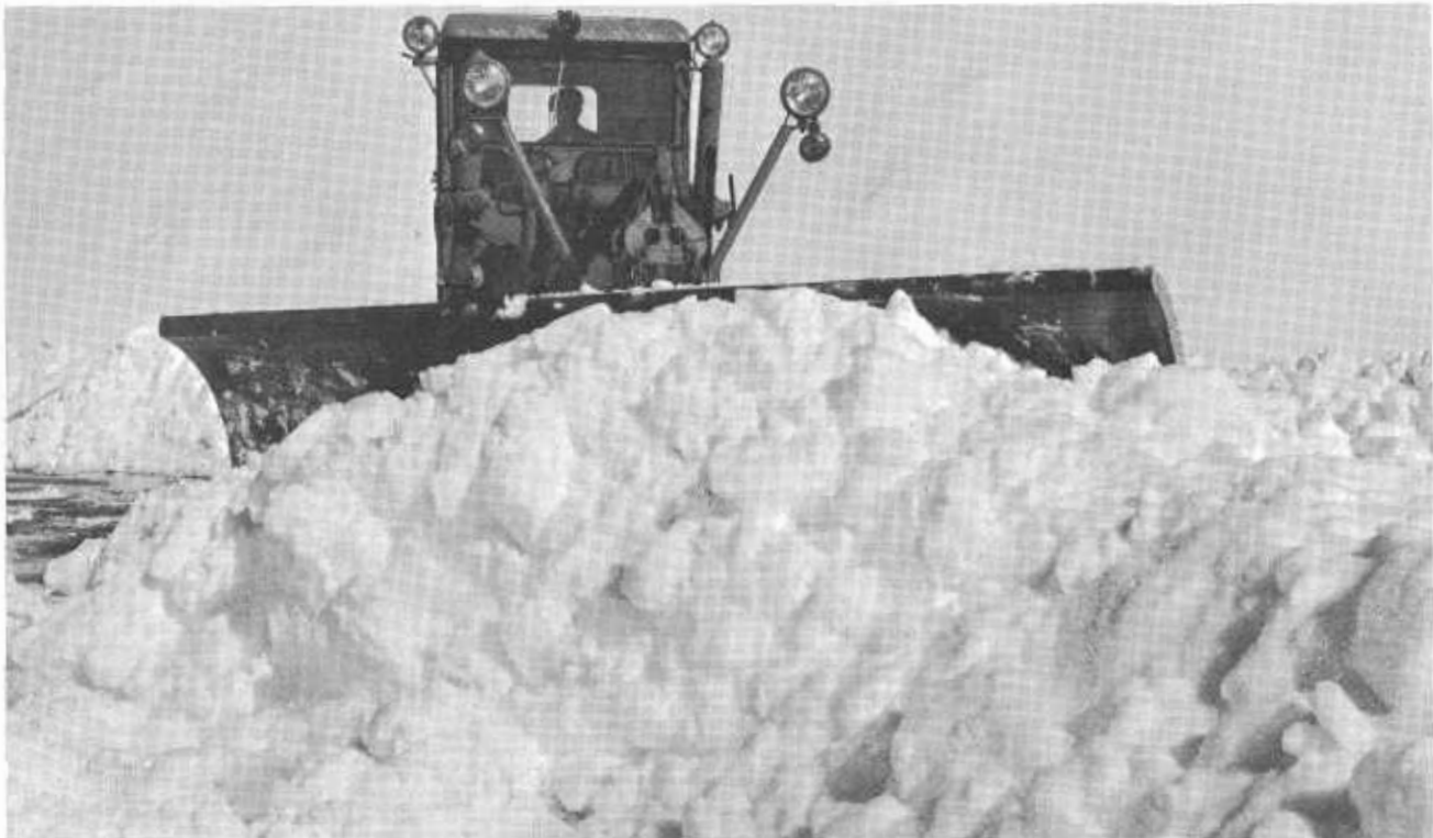
It takes a massive grader and lots of power to push snow from the traveled way.
