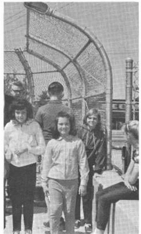
A conduit fitting (upper left) on the end post of the chain link railing on a pedestrian overcrossing.
