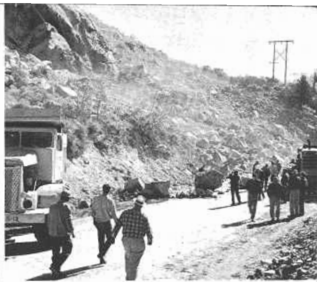
View of old section of Route 120 just after Elephant Head shot. Small amount of rock on road from blast directly above shows excellent control of the shot.
