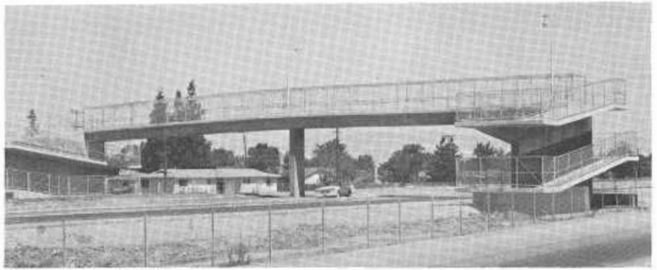
A pedestrian overcrossing with the old-style luminaires mounted on 20-foot standards.
