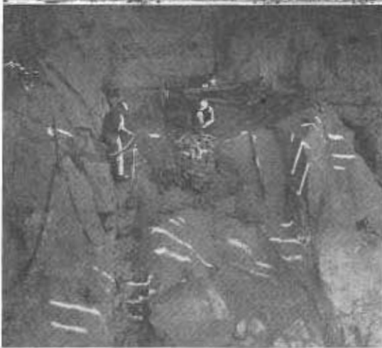
Men working in shadow of bridge are doing preliminary work on supports for new sidehill viaduct. Bailey bridge carried traffic for months during reconstruction.
