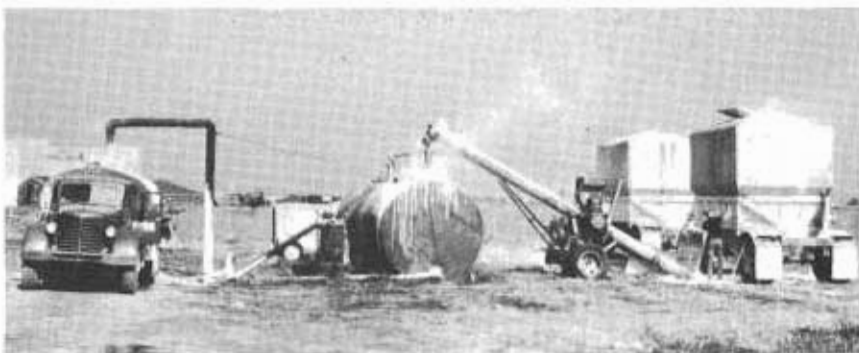
PHOTOS LEFT, TOP TO BOTTOM. A tank truck spreads lime slurry in an area where lime dust could cause damage to airplanes stored nearby. SECOND PHOTO—Mechanical road mixing of lime with damp aggregate. THIRD PHOTO—Large tank truck and spreader used in laying dry lime. BOTTOM PHOTO—Dry lime is converted into slurry in mixing tank.
