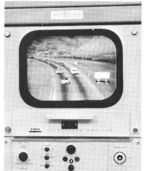
PHOTO TOP—Television camera set into the east portal face of the tunnel. Camera can be made to pan, tilt or zoom in on special area for closer look, all by remote control. LOWER PHOTO—A typical view of traffic as seen on one of the television monitors in the control room.
