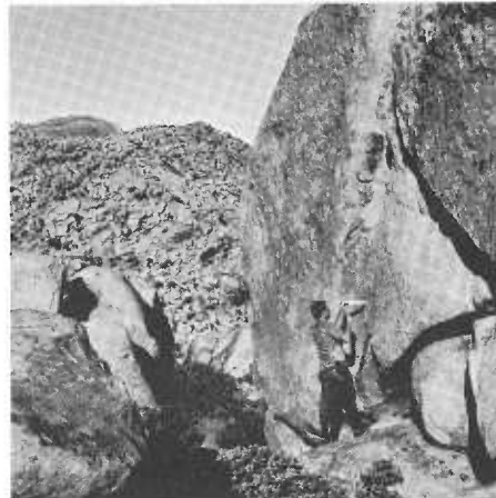
Survey Party Chief Walter Butcher, a District 11 employee, setting slope stakes in rock.
