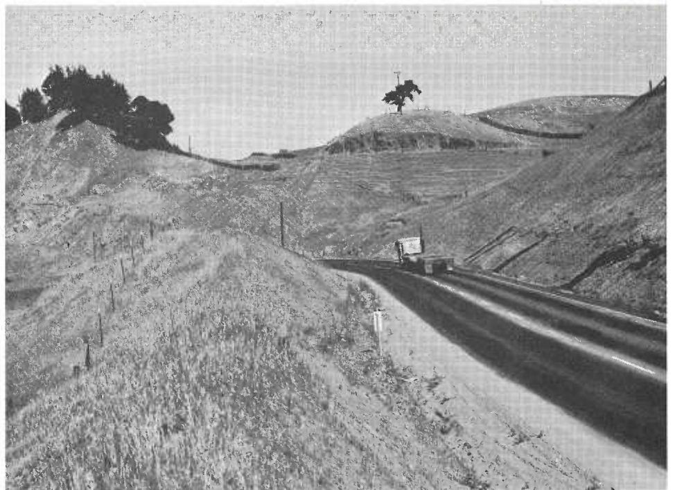
PHOTO RIGHT—Because of unstable soil conditions as much of roadway as possible was built in cut rather than on fill to minimize weight on foundations. PHOTO BELOW—Some typical alignment of the new highway with some of old pioneer toll road visible by barn in upper right.
