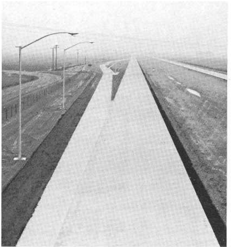
A nearly completed section of Interstate 5 Freeway northwest of Los Banos in Merced County. The area and connecting lanes left of the north-bound roadway are for a truck weighing station. The view is southward.
