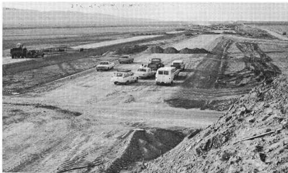
This construction site along Interstate 5 in Fresno County will be the location of an interchange with Panoche Road.
