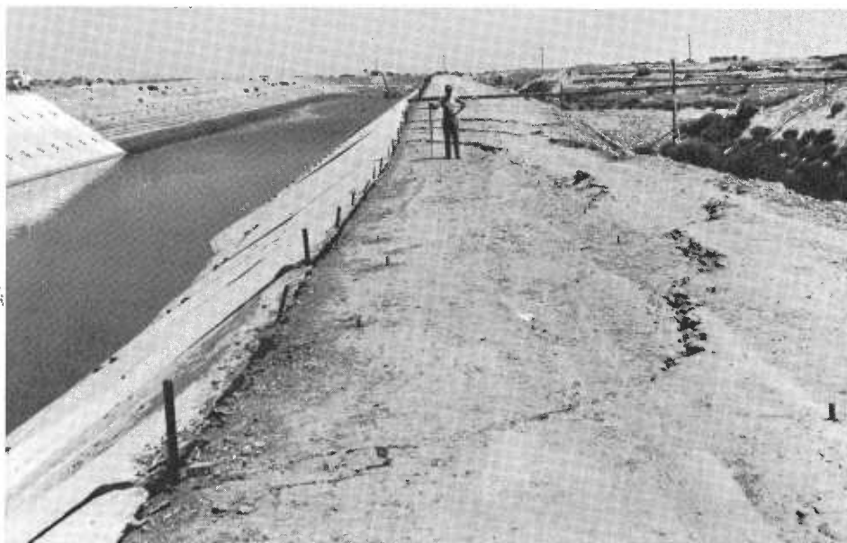
Failure of concrete lining and embankment in noncompacted portion after inundation of the prototype test canal for 90 days.
