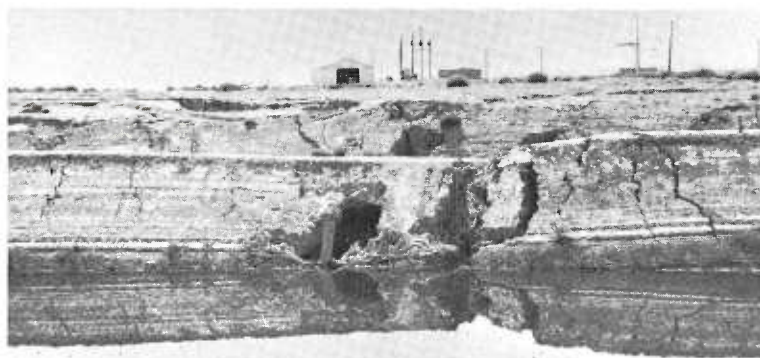
Failure of the earth-lined section in the noncompacted portion of the prototype test canal after 130 days of operation.
