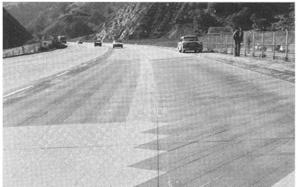
Below: Overall view of test area on Route 5 in Kern County, showing diagonal and longitudinal scoring of a portland cement concrete pavement for improving its skid resistance.
