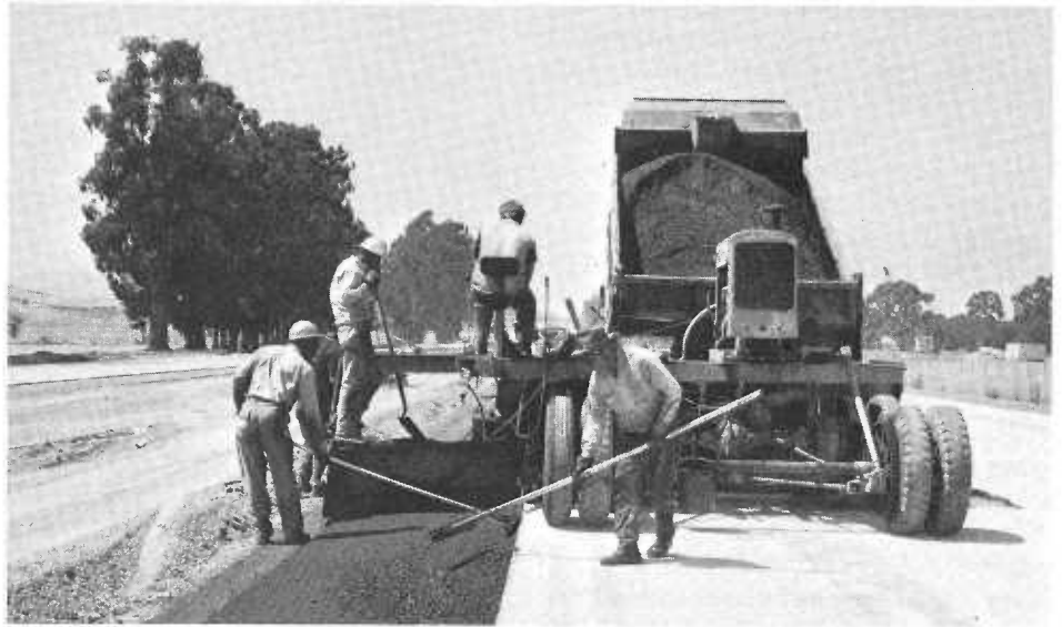
Contractor's crew shown above is completing the asphalt shoulders on a new freeway, only one of the many lesser tasks necessary before a new section can be opened.
