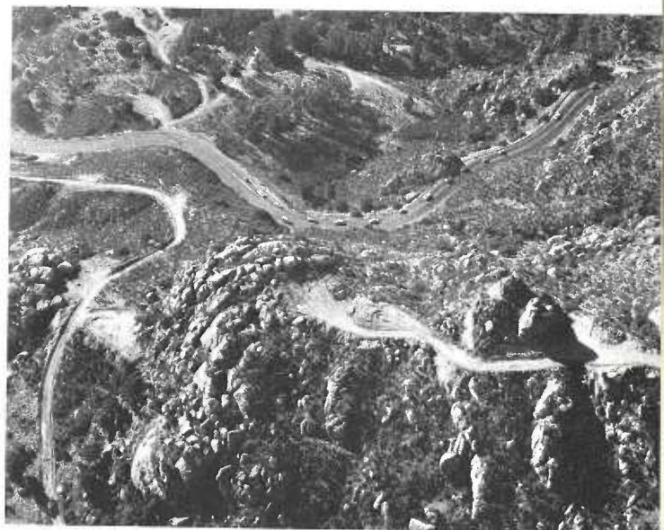
Construction work for new freeway will pass close to old route. Note string of traffic on old road held up by small car laboring up grade.
