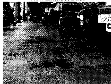
Deterioration of the Floor Surface
