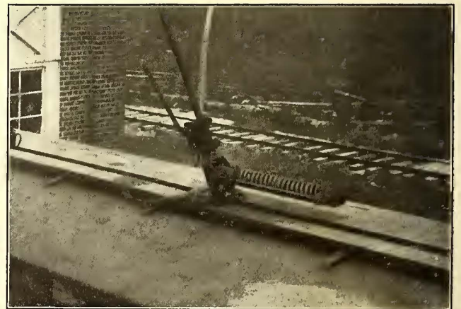
Pole Clamp After Pole Is Replaced and Tightened Up Ready for Use
