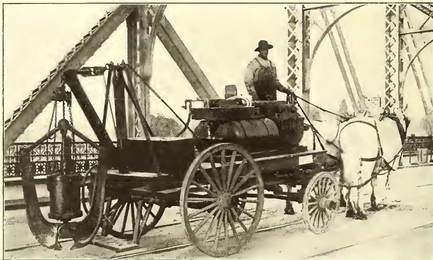
Thermit Rail Welding—Shear for Cutting Off Riser and Compressed-Air Equipment for the Shear and Preheater
