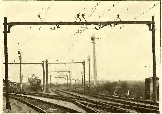
Midland Railway Single-phase Electrification—Construction at a Double Cross-over Consisting of Double Angles Riveted to Brackets Clamped on Wooden Poles
